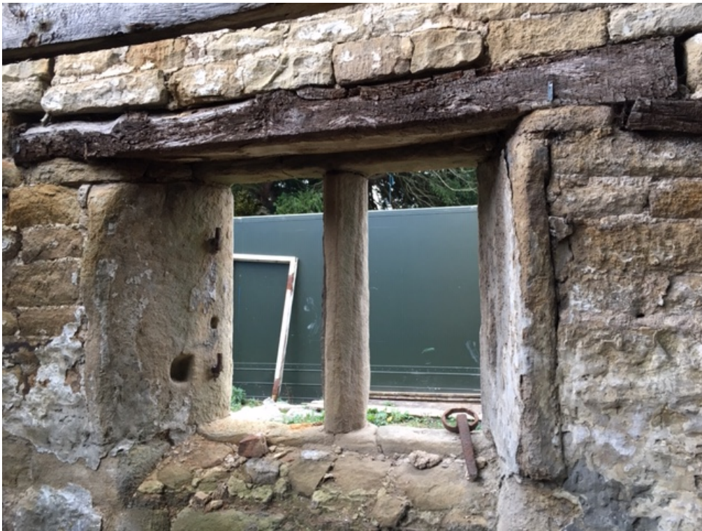
Figure 4a/b: Windows in the east wall (above and below), photograph taken from the west (Alison Arnold)
