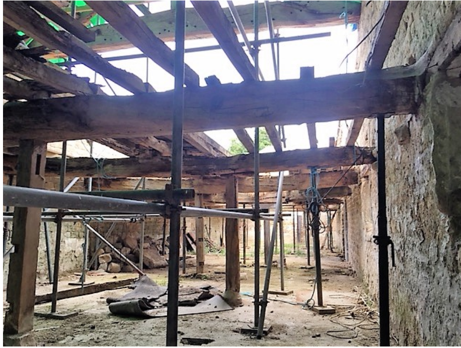
Figure 5: Floor structure, beam 4 in foreground, photograph taken from the south (Alison Arnold)
