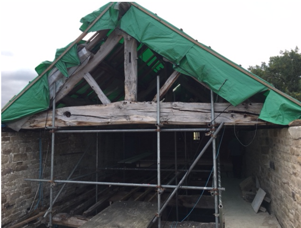
Figure 6: Truss 3 showing principal rafters, single angle struts, and straight braces to a diamond-set ridge. Photograph taken from the north (Alison Arnold)
