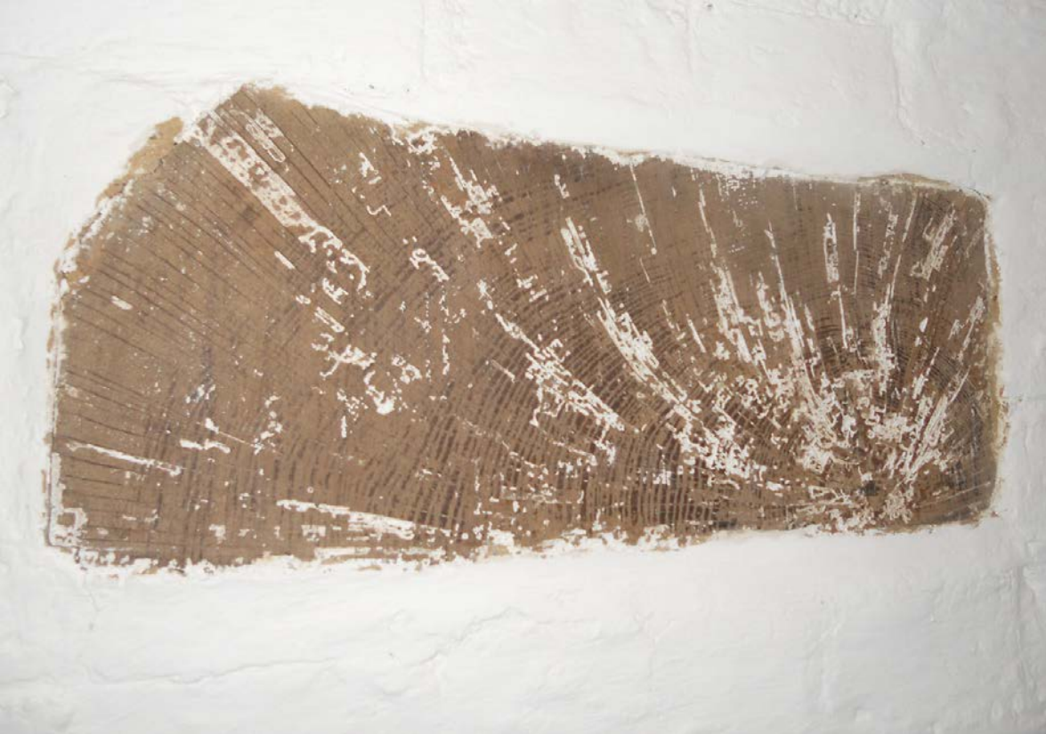
Figure 9: View of the exposed end of the beam in the cellar – hwkb30 (photograph Martin Bridge)
