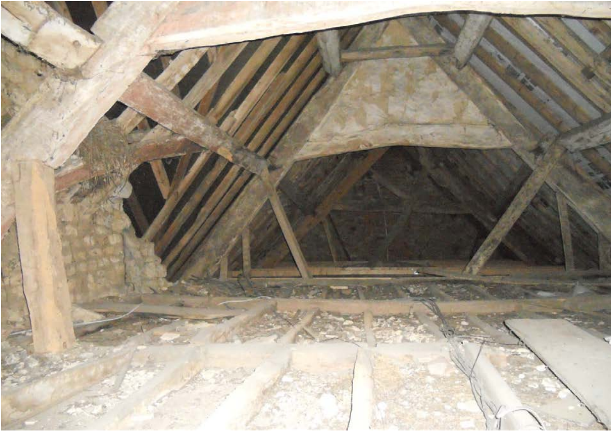
Figure 7: View of the west-range roof, looking south, with the inserted stack to the left (photograph Martin Bridge)
