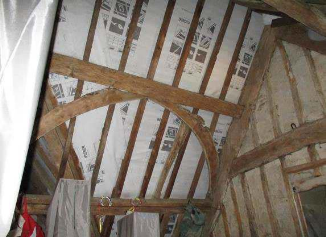
Figure 5: View of truss 3 in the north range, looking south-west (photograph Oxfordshire Buildings Record)
