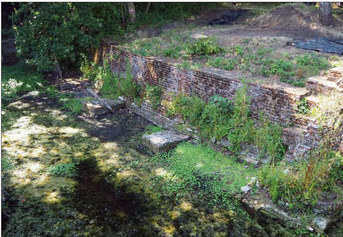
Figure 52 – The southern part of the outer west moat wall with particularly low water level, part of the western bridge abutment can be seen to the right (Magnus Alexander 11/8/2020 © Historic England)
