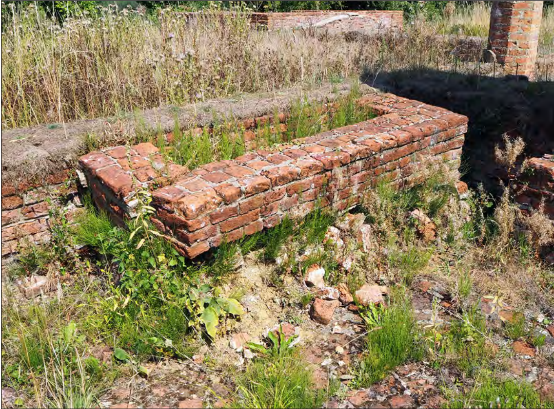
Figure 32 – The collapsing planter built against the south wall of the Parlour and projects into the south of the Herb Garden (Magnus Alexander 11/8/2020 © Historic England)
