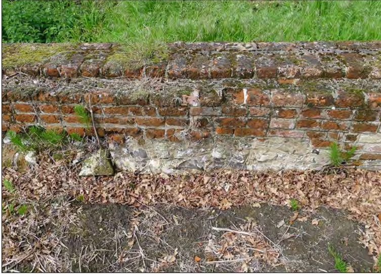
Figure 31 – East face of the Parlour's west wall (the opposite face to that in the foreground of Figure 30) showing the repointed flint (Jonathan Kewley 26/4/2017 © Historic England)
