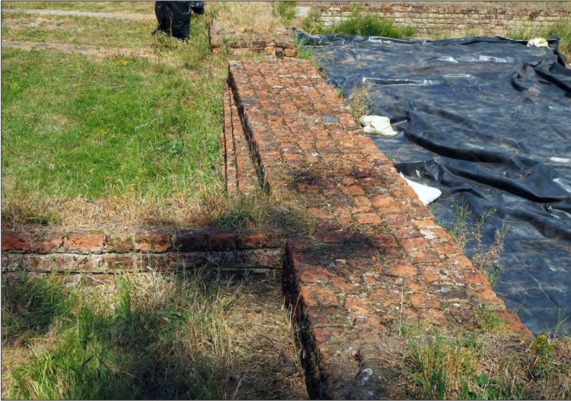
Figure 48 – The west wall of the Kitchen from the south, showing the markedly different orientation of the lower courses (Magnus Alexander 11/8/2020 © Historic England)
