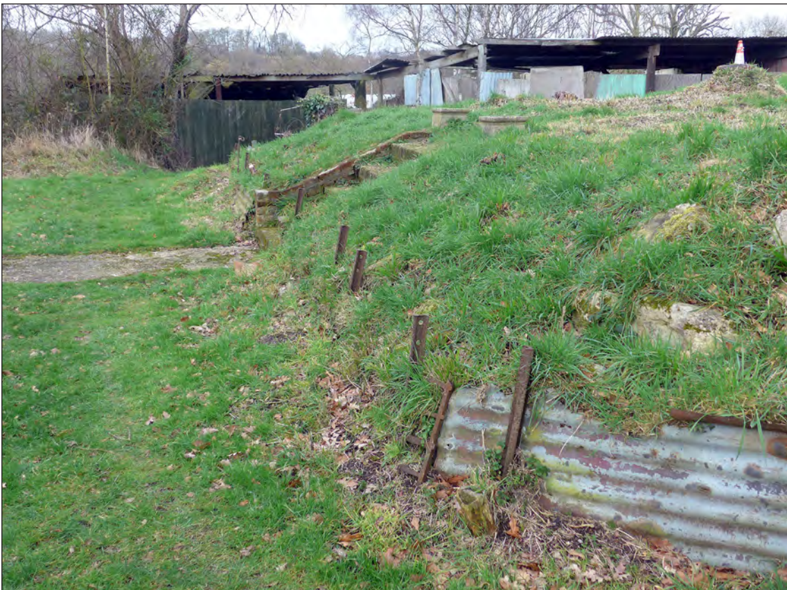
Figure 62 – The south-west side of the same structure from the south showing the metal revetment, garden steps and modern ramshackle sheds behind (Magnus Alexander, 14/2/2018, © Historic England)
