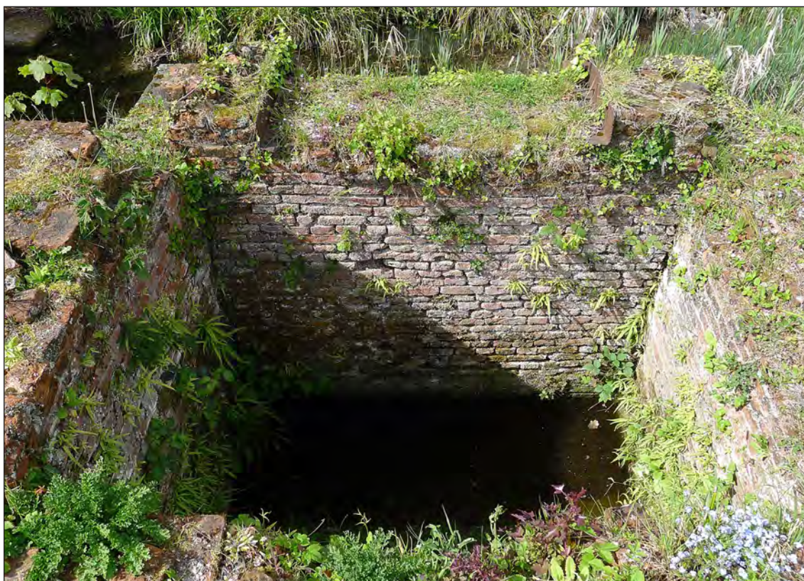
Figure 36 – The eastern bridge abutment and pit from the east, note the poor joints to left and right of the far wall (Jonathan Kewley 26/4/2017 © Historic England)
