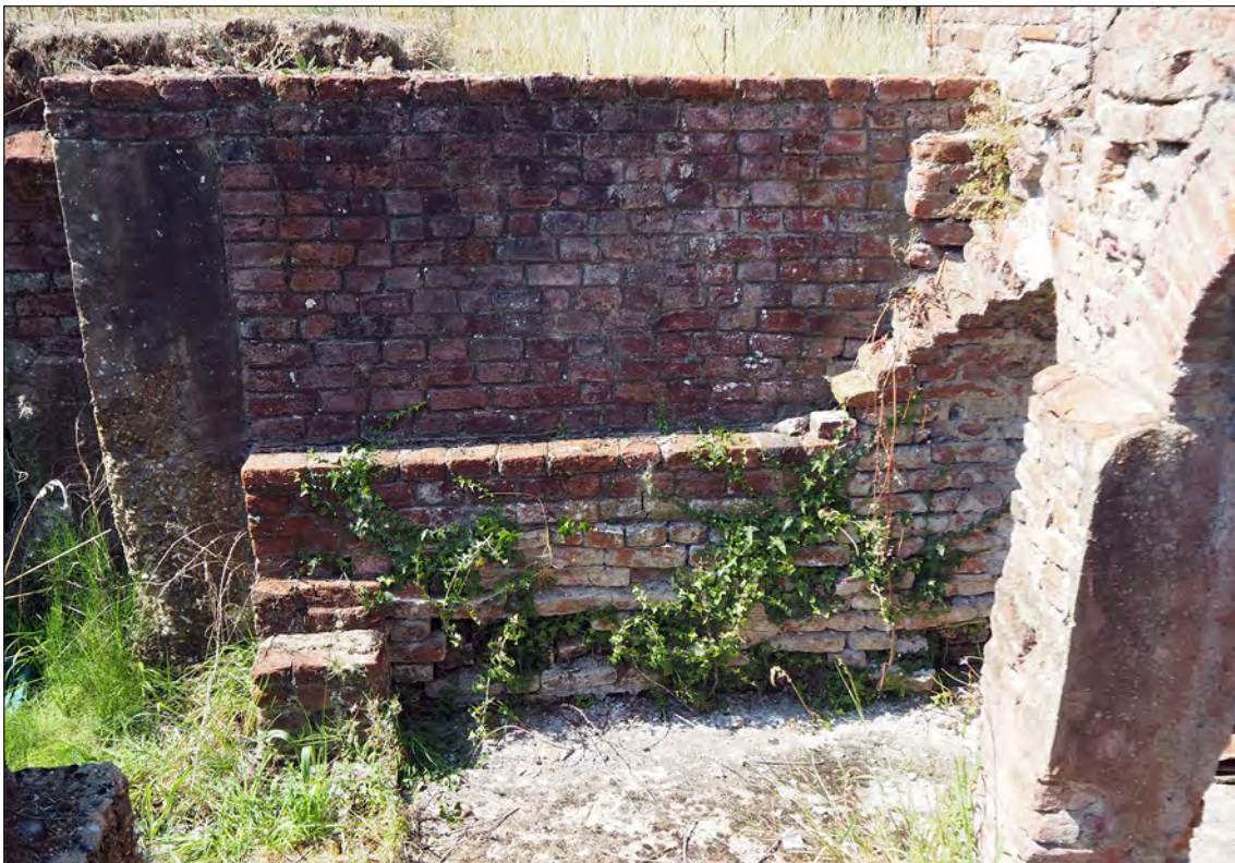
Figure 24 – The west wall of the Undercroft 'area' with the spring for the barrel vault visible to the right. Some early English bond is visible at the bottom of the photograph with clearly late work above the step (Magnus Alexander 11/8/2020 © Historic England)
