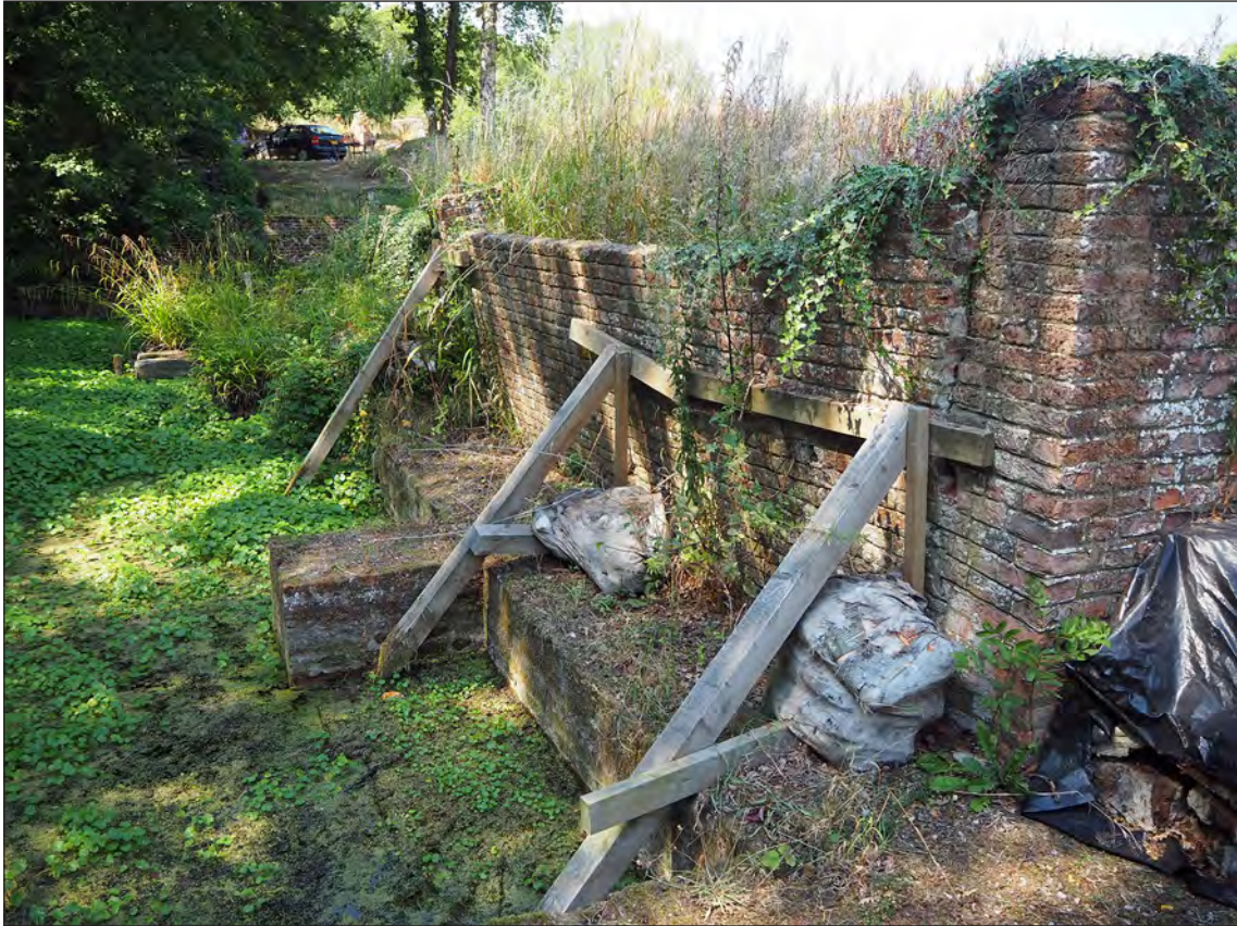
Figure 44 – The collapsing retaining wall to the west of the well enclosure from the east (Magnus Alexander 11/8/2020 © Historic England)
