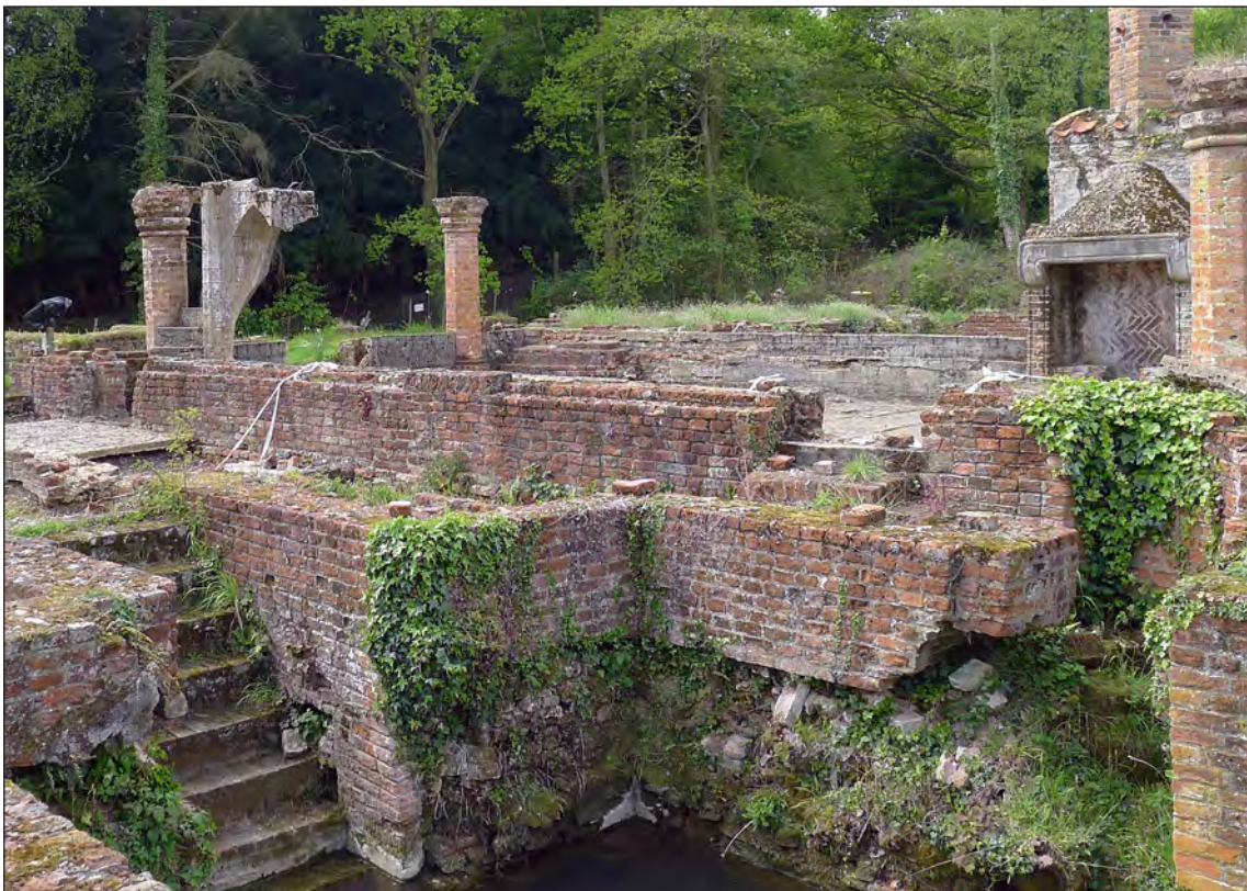
Figure 18 – A view south-west across the south of the Large Cellar with the Hall behind. The south stair is to the left with the small west stair to the right. The extent of decayed early fabric below the late work is clearly visible between the two (Jonathan Kewley 26/04/2017 © Historic England)
