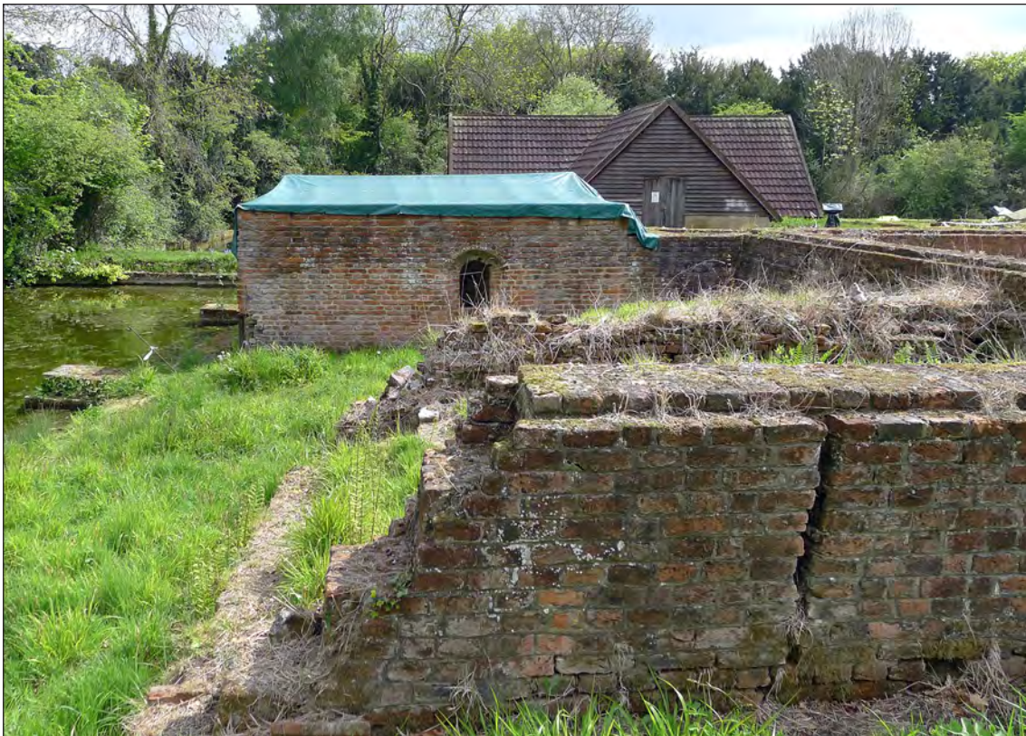
Figure 28 – General view from the west, wall [9] is in the foreground with [7] beyond, the Undercroft and Apple Store are in the background (Jonathan Kewley 26/4/2017 © Historic England)
