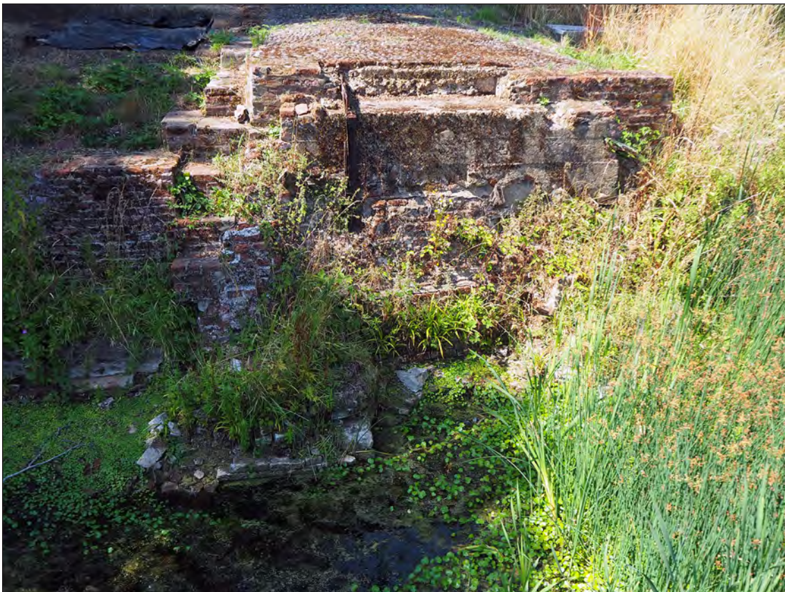
Figure 53 – The western bridge abutment from the east, although overgrown the low water level allows some features not visible during the survey to be seen (Magnus Alexander 11/8/2020 © Historic England)
