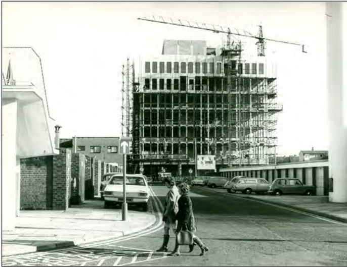
Figure 147. Manulife House, St George's Way, under construction in 1972 – in a view looking east from the East Gate car park, past the boiler house chimney. (With kind permission of Stevenage Museum, P11168)
