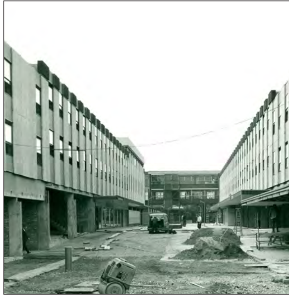
Figure 76. The north part of Queensway under construction in 1969, looking south towards the two-storey bridge. (With kind permission of Stevenage Museum, P11188)
