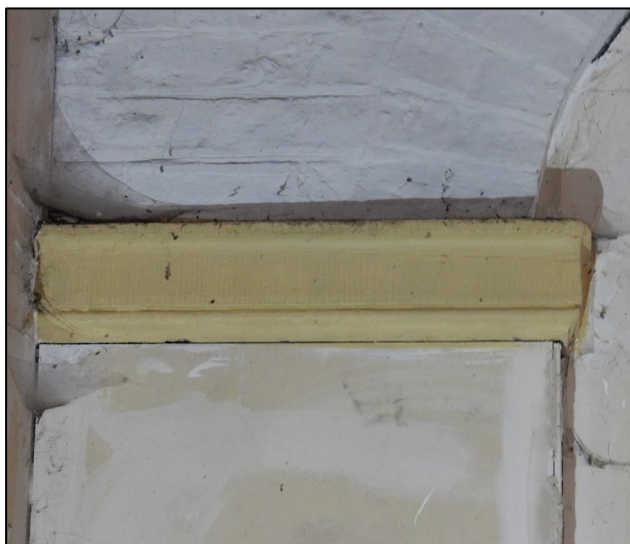
Figure 20: Impost band detailing on SE corner (interior view) with vertical tooling marks and
