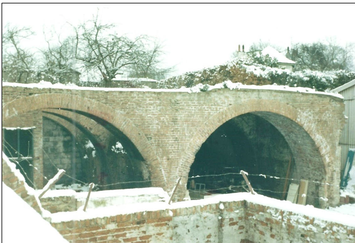
Figure 5: Eaglescliffe/Yarm coal depot in 1971 with distinctive circular arches and the trackbed over the top as seen in early images of Darlington's depot (photo: John Proud, courtesy of Win Proud).
