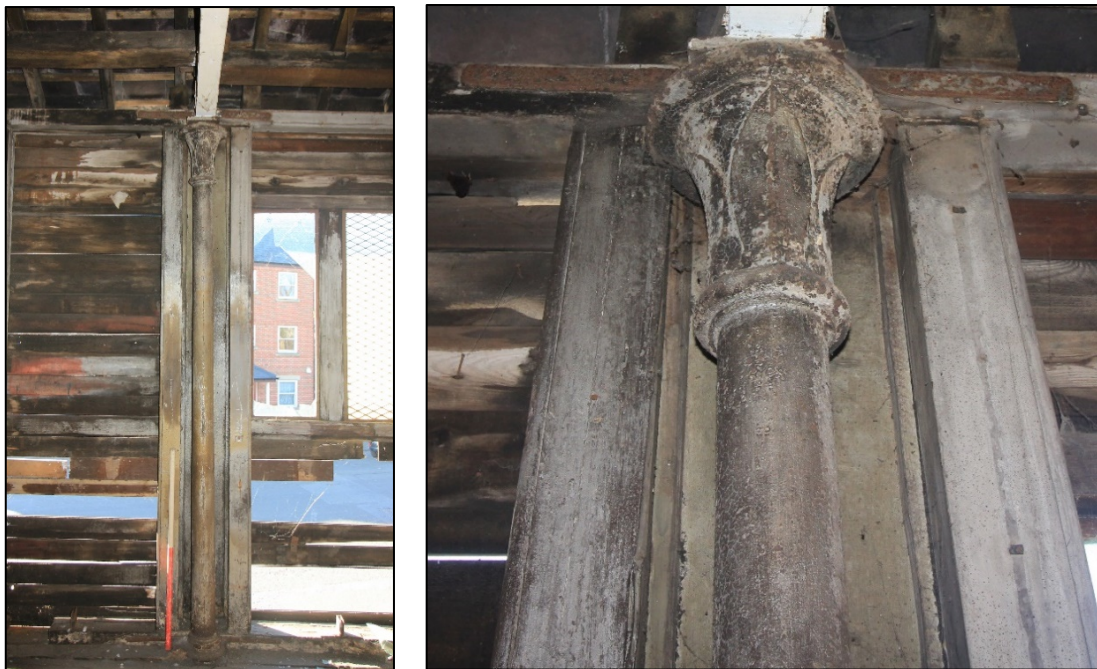
Figure 27: Three cast-iron columns with lily leaf decorated capitals are located along the building frontage, positioned on the upper floor in the division points between the cells below.
