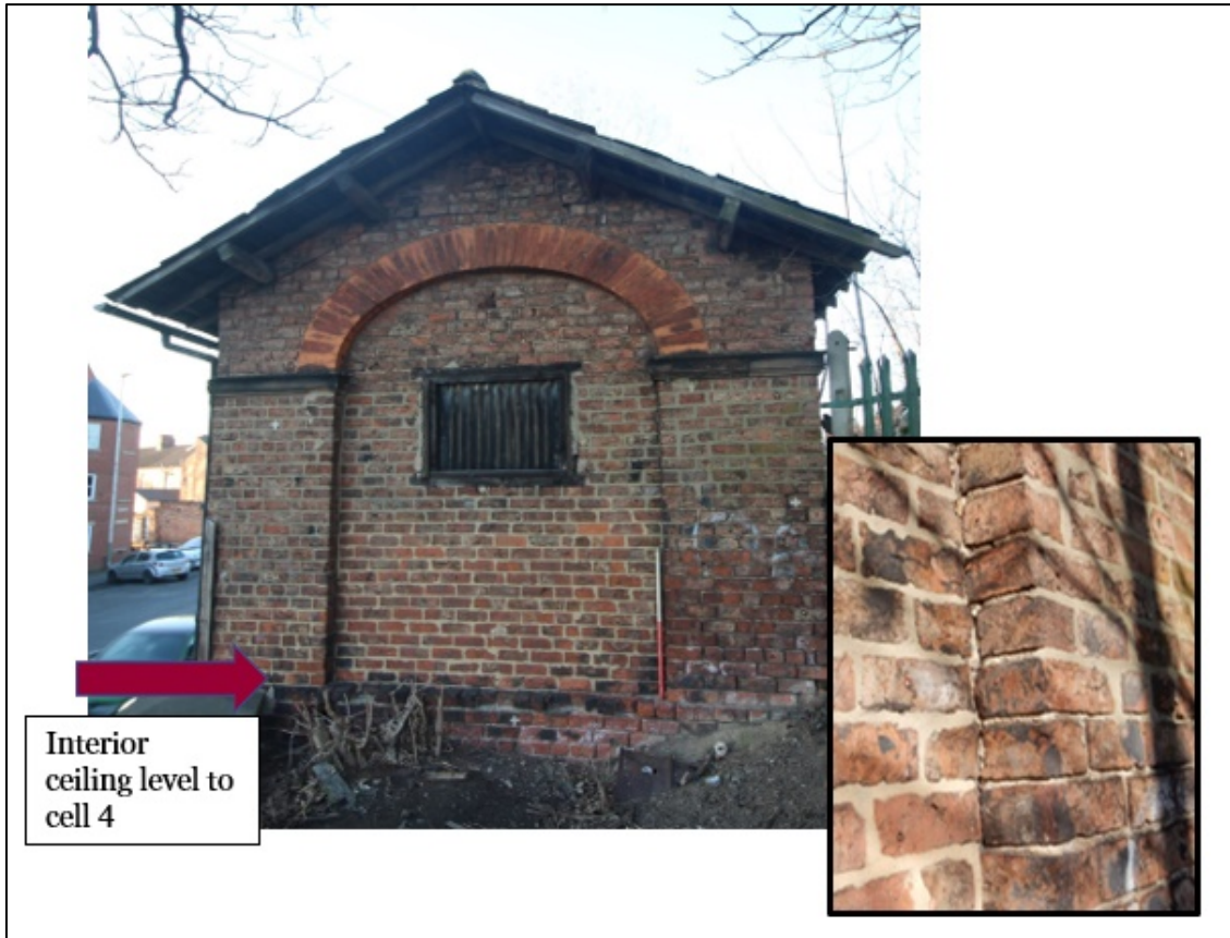
Figure 40: South-east gable end. The base and jambs are bonded in English Garden Wall Bond. The arch fill is in a simple stretcher bond because it requires no structural strength. The arch fill is also not bonded into the jambs suggesting that it could be a later fill or was designed as a decorative pier and panel construction from the outset. Differential pointing methods might simply reflect periods of repair or alterations associated with a short-lived single storey extension seen on aerial photographs dating to 1949. The brickwork above string course height is different from the rest of the arch infill. The brick plinth along the base is not seen on the opposite gable.
