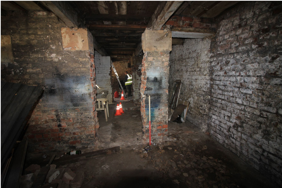
Figure 43: view from cell 4 through later gaps in the cell walls towards cell 3 then 2. The gap on the right is neater and has properly finished edging to the brickwork on the other side; it is an earlier gap possibly late 19 th century when the lime depot was repurposed for light industrial use. The sandstone pads supporting the waybeams which supported the rails above can be seen.
