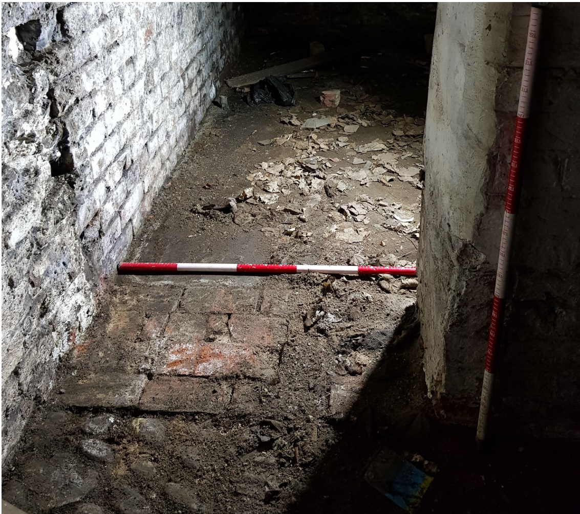
Figure 44: Wall footings visible where a gap was inserted between cells 3 and 4 sometime after the lime depot changed use, possibly in the late 19 th century
