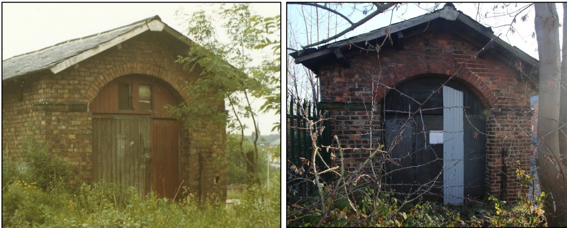
Figure 39: The north west elevation in 1971 (photo John Proud) and in 2019. There appears to have been some historic damage to the arch, also visible internally
