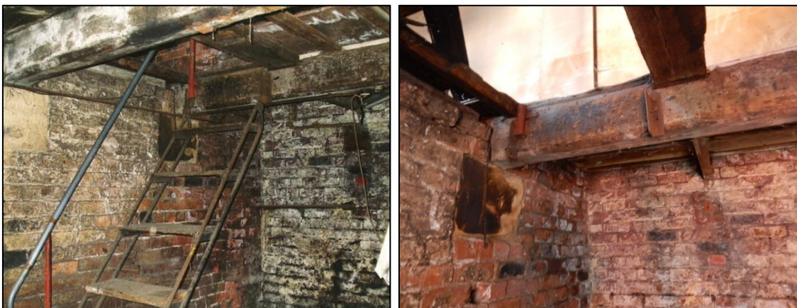
Figure 42: Left: the former iron staircase from cell 2 to the first floor (image courtesy of Darlington Borough Council). Right: the fixings for the metal stair survive in the waybeam. The trapdoor door, complete with circular handle, lies on the floor below in two pieces.
