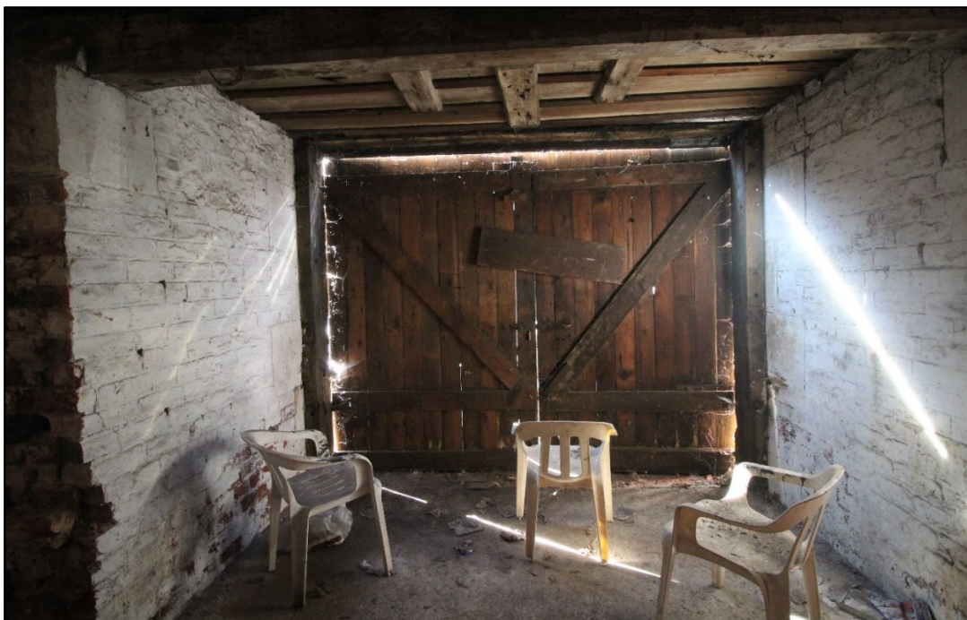
Figure 48: Cell 3 looking towards the street frontage. Dressed sandstone ashlar blocks terminate the brick dividing walls to the street front. The door surround is formed with reused sleepers.
