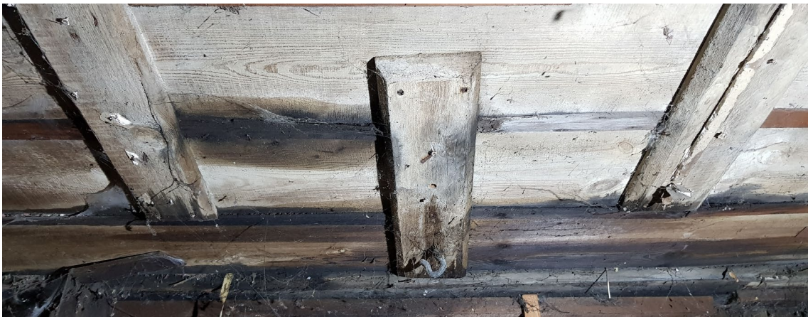
Figure 34: A typical set of three chamfered timbers below the street front lime attendants' platform. The central timber has an iron hoop, and this arrangement appears to have been repeated in all four cells. It may have supported a hoist for moving sacks of lime from cell to cart.
