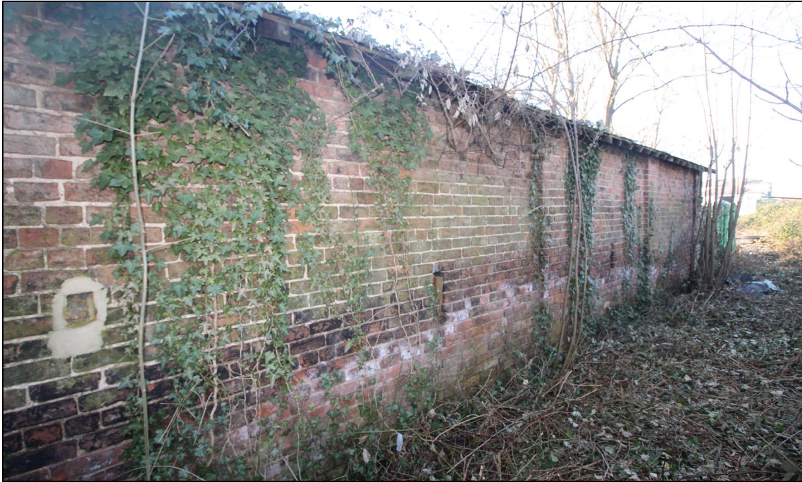
Figure 22: The rear (north-east) elevation with only the upper floor above ground. Each ventilation slit is in the centre of where the individual lime cells are located below. Four slim brick buttresses add support to where the cell walls join below.
