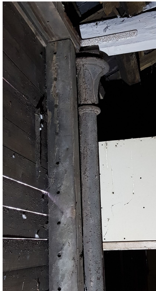
Figure 30: Dowel holes on uprights mark where louvres were attached, the shadows of the shutters can still be seen.
