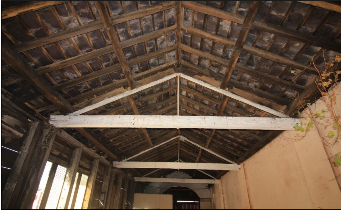
Figure 26: The simple truss roof structure. The cast-iron columns (see left) are however too short to support the tie beams so slivers of metal have been added to make up the difference and to provide a solid level surface to support the tie beams and wall plate (see below, fig 28)
