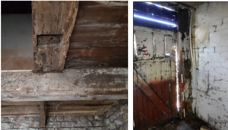
Figure 46: Left: reused sleepers cut into the waybeam to support the infill flooring. Right: reused sleeper used as a door jamb in cell 1.
