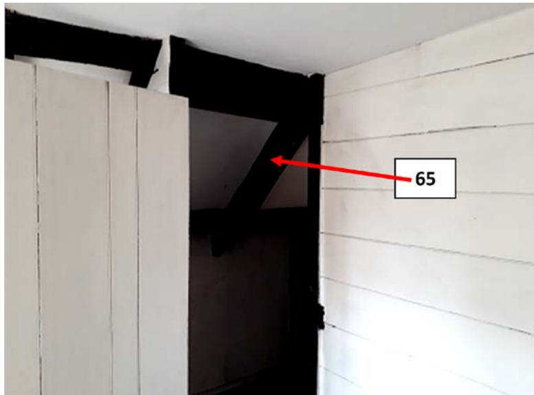
Figure 15j/k: Annotated photographs of the roof space of 42 High Street looking west to east (EXT-M64 and EXT-M66; top) and north to south (EXT-M65; bottom) to help identify sampled timbers (photographs Robert Howard)
