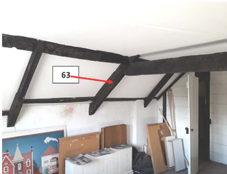
Figure 15h/i: Annotated photographs of the roof space of 42 High Street looking west to east (EXT-M61 and EXT-M62; top) and east to west (EXT-M63; bottom) to help identify sampled timbers (photographs Robert Howard)
