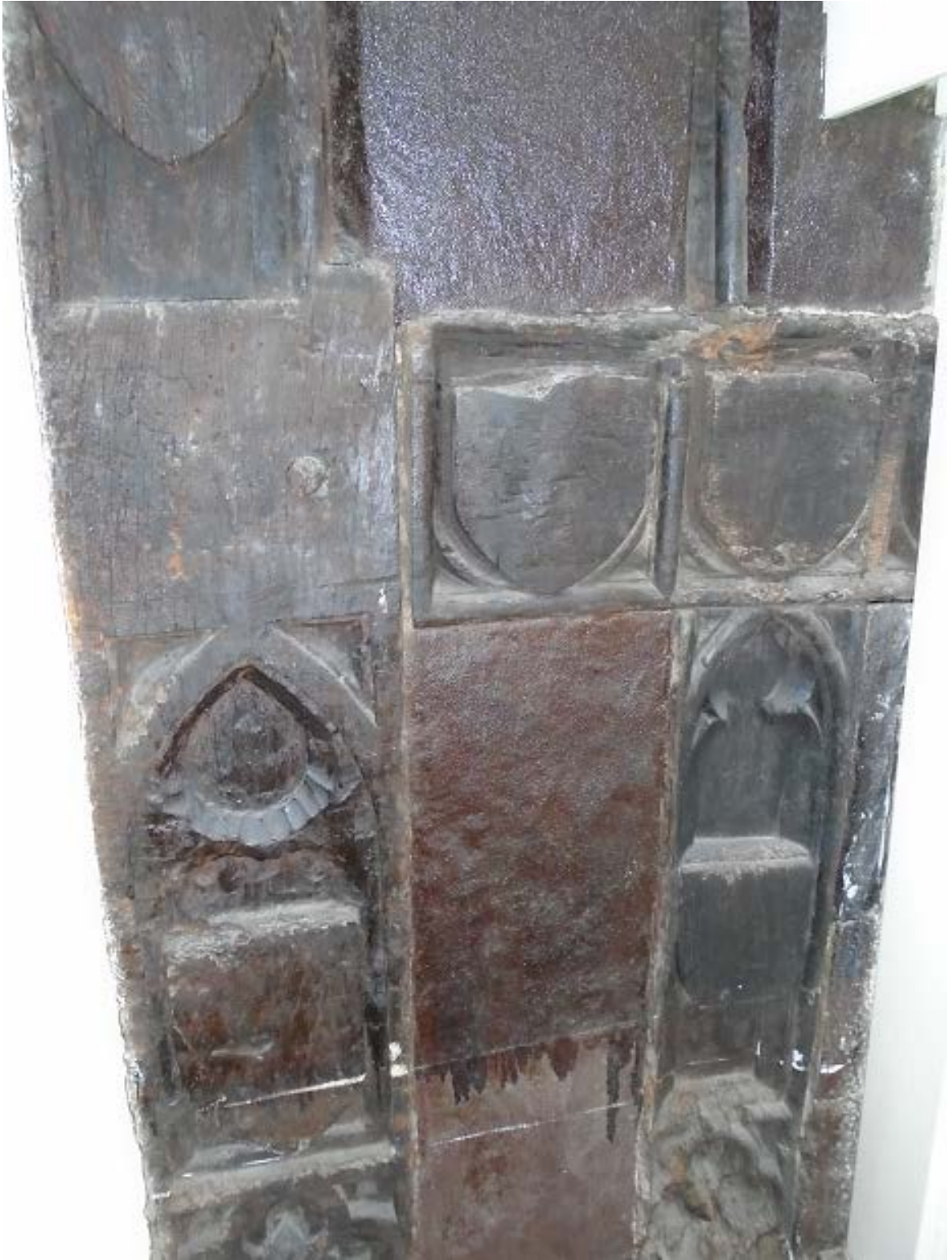
Figure 8: View of a section of the east wall of number 46 which was originally exposed to Lamb Alley. This wall was hidden when 45 High Street was built, and sections of it are now only partially visible behind wall panels in the upstairs rooms of number 45 (photograph Robert Howard).
