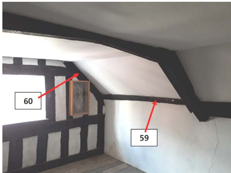
Figure 15f/g: Annotated photographs of the roof space of 41 High Street looking east to west (EXT-M56–EXT-M58; top) and west to east (EXT-M59 and EXT-M60; bottom) to help identify sampled timbers (photographs Robert Howard)
