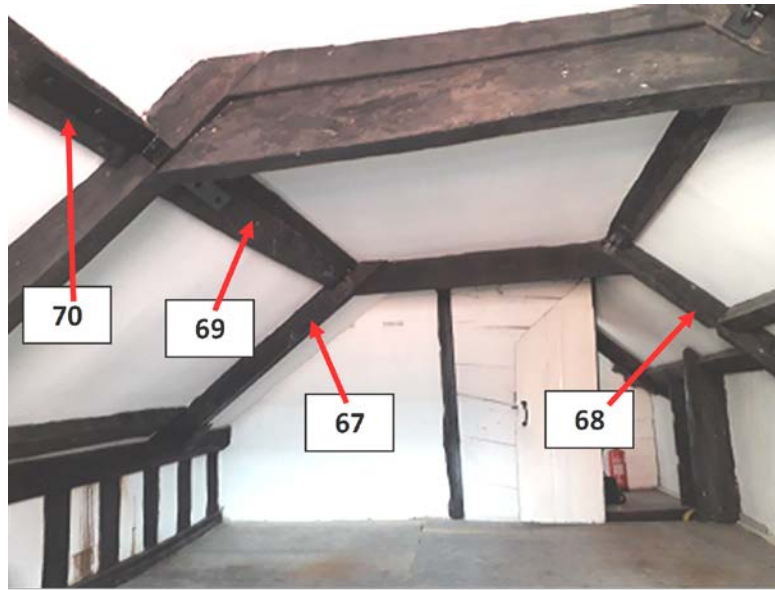
Figure 15l: Annotated photograph of the roof space of 42 High Street looking west to east to help identify sampled timbers (EXT-M67–EXT-M70)(photograph Robert Howard)
