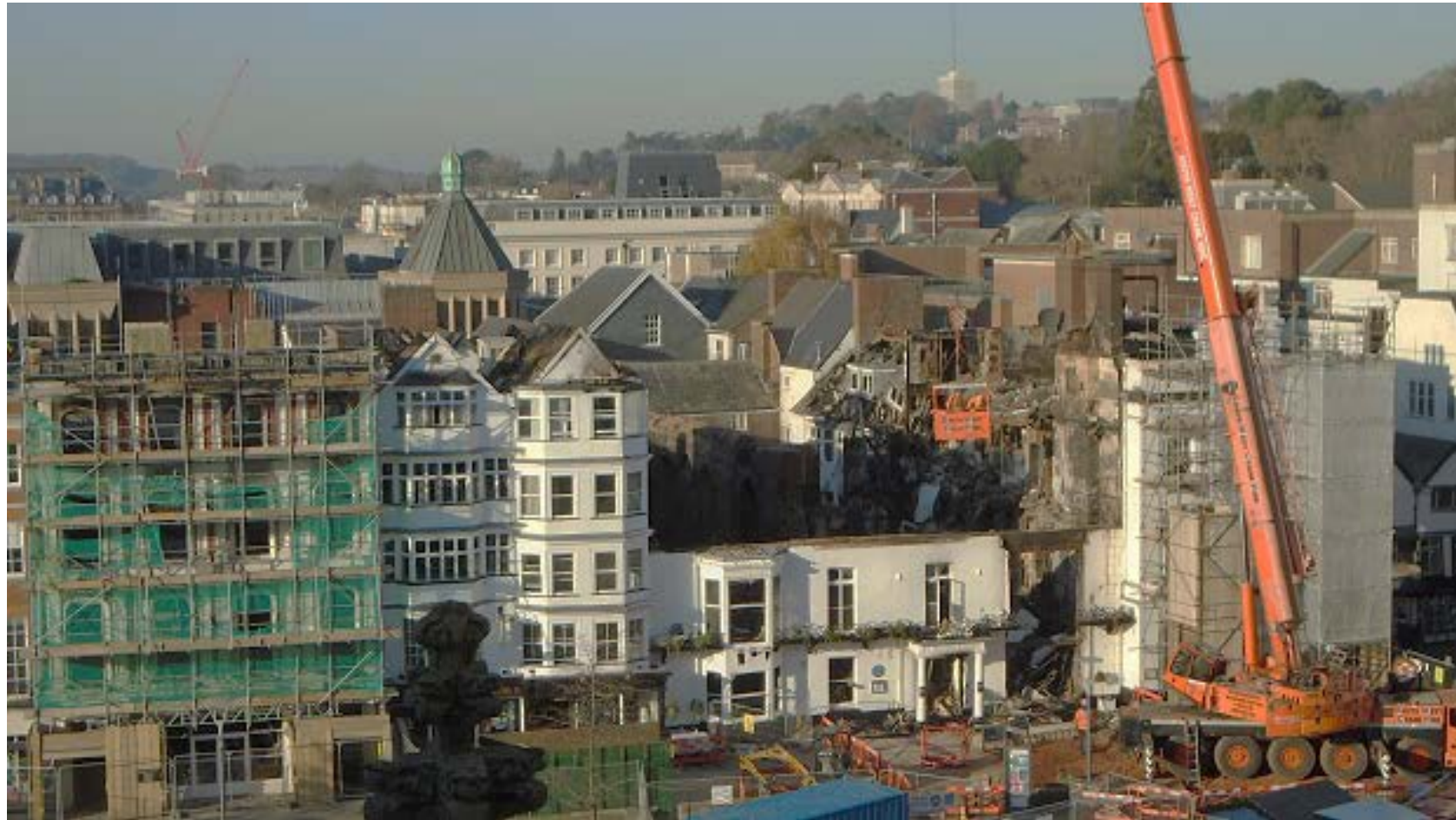
Figure 2: General view of the Royal Clarence Hotel and 16–17 Cathedral Yard (The Well House Tavern) looking west from Cathedral Yard. Only the ground- and first-floor frontage of the Royal Clarence Hotel remain in place, with the five-storey, double bay-fronted Well House Tavern to its left (photograph Robert Howard)
