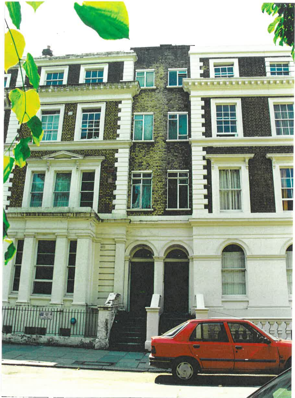
Fig. 32 The space between the uppers stages of Nos. 11 and 12 Albert Square was blocked, perhaps in the 1960s, to create new room space.
