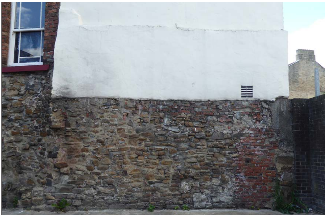
Figure 95: Nos. 6-7 North Bondgate, east elevation showing rough stone rubble to the lower section of wall; viewed from the east (© Historic England, photograph taken by Clare Howard, 2019)
