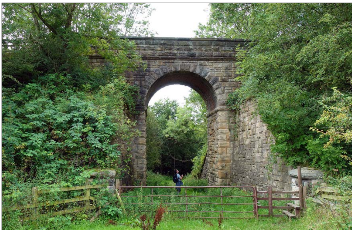
Figure 65: The eastern elevation of railway accommodation bridge no. BIF/9 (© Historic England, photograph taken by Rebecca Pullen, 2019)
