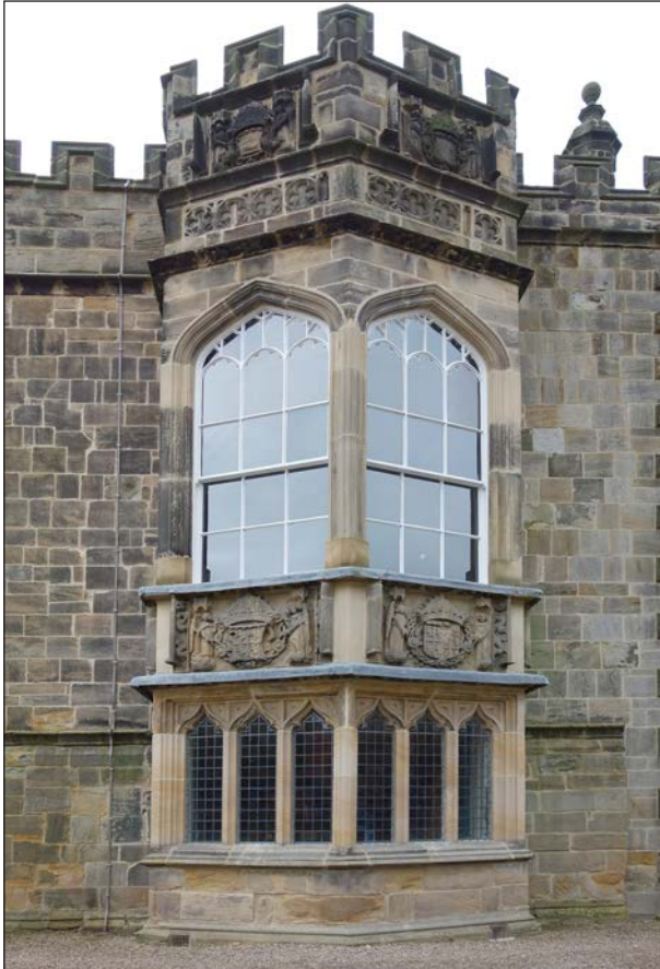
Figure 50: The canted bay window on the east side of the 16th-century extension, viewed from the east. The lower parts of the window are 16th century and retain the arms of Bishop Ruthall while its upper part and the walling of the first floor to the right of it has been replaced (© Historic England, photograph taken by Rebecca Pullen, 2019)
