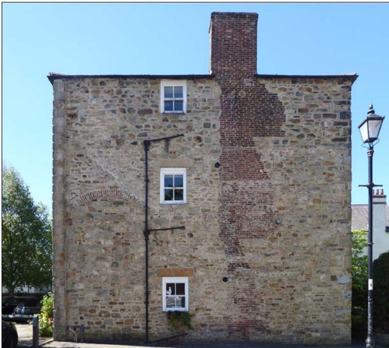
Figure 80: East elevation of no. 27 Market Place (The Elms), viewed from the east (© Historic England, photograph taken by Clare Howard, 2019)
