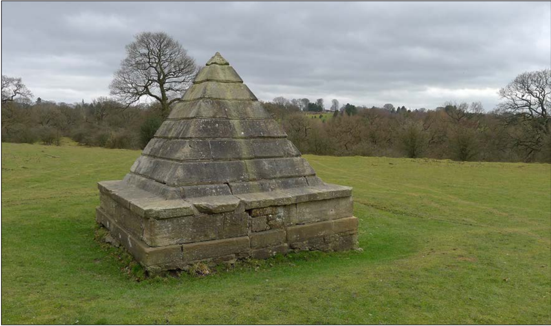
Figure 63: The pyramidal stone well head and one of the associated linear depressions denoting buried drains or pipes (right). Note the possible blocked inspection hatch within the plinth. Viewed from the north, with the golf course club house just visible on the far horizon indicating a key visual link with the highest point on High Plain (© Historic England, photograph taken by Rebecca Pullen, 2019)
