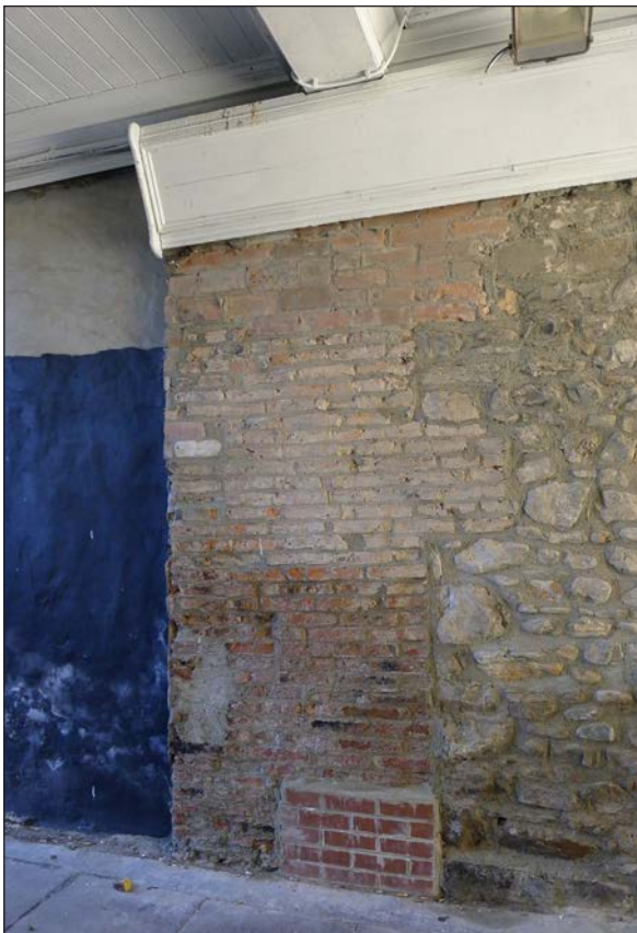
Figure 128: The north elevation of no. 73 Newgate Street showing the remnants of an earlier party wall perhaps in part belonging to the former Three Blue Bells Inn which stood on this site; viewed from the north (© Historic England, photograph taken by Hilary Gould, 2019)
