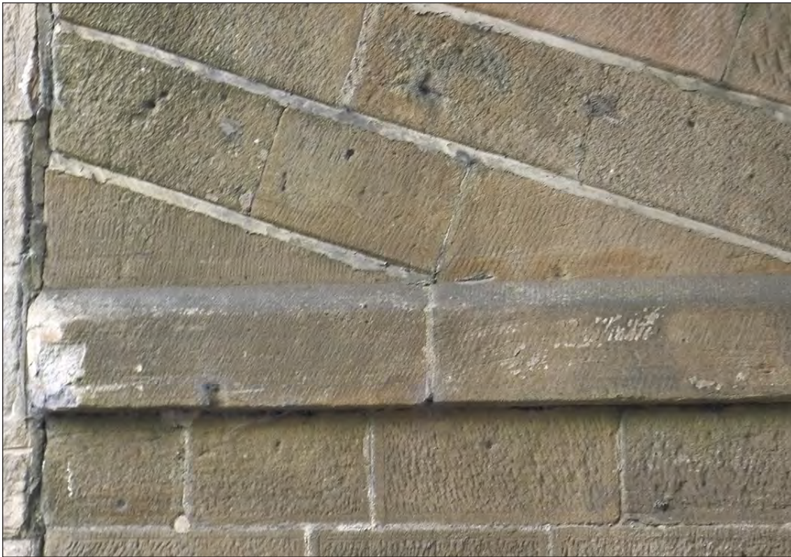
Fig 54. Detail of the impost banding and helicoidal coursing of the phase-1 arch barrel of railway underbridge DAE2/4 (High St, Coundon Grange). Note that the stones forming the first course of the barrel are integral with those in the impost banding beneath. Note also the butt joint with the masonry of the phase-2 widening just visible at left of frame. (© Historic England/Marcus Jecock)
