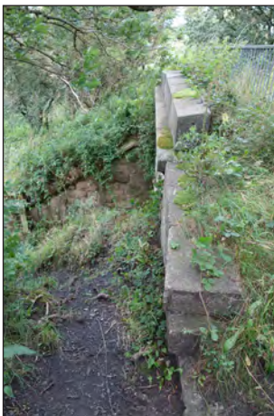
Fig 41. Detail of dislodged/missing stones in the eastern parapet of railway accommodation bridge BIF/10. (© Historic England/Rebecca Pullen)
