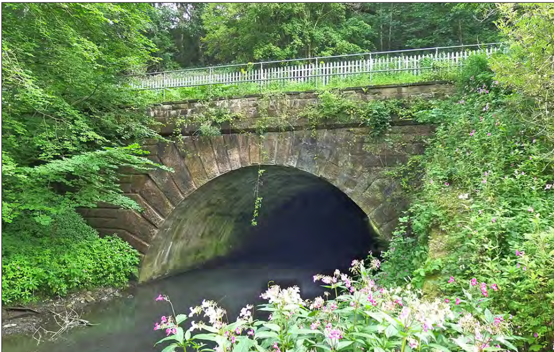
Fig 64. The northern portal of railway bridge DAE2/8 over the River Gaunless. Note the low parapet wall above the coping, probably added before 1896 to retain extra embankment material when the railway was widened. (© Historic England/Marcus Jecock)
