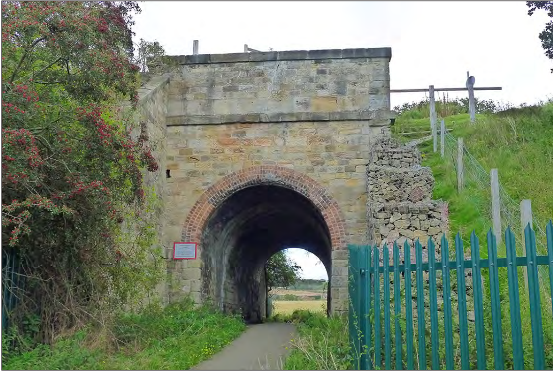
Fig 58. The western, phase-2, elevation of railway accommodation underbridge DAE2/6 ('Shepherds'). (© Historic England/Marcus Jecock)
