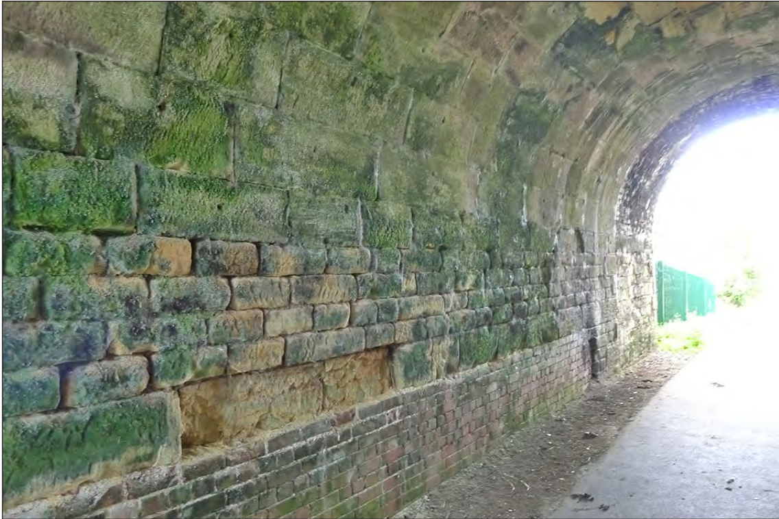
Fig 57. The southern face of the phase-1, abutment of railway accommodation underbridge DAE2/6 ('Shepherds'). Note the repeating rhythm of the original stonework: four narrow courses followed by one course of larger stones, all now deteriorating and heavily patched in brick. The stone arch barrel contrasts with the brick arch barrel of the phase-2 western extension which can just be made out at right of frame. (© Historic England/Marcus Jecock)
