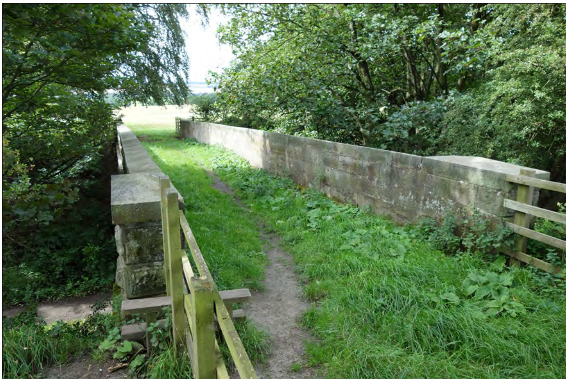
Fig 48. View west along deck of railway accommodation bridge BIF/12, showing parapets and end piers. (© Historic England/Rebecca Pullen)
