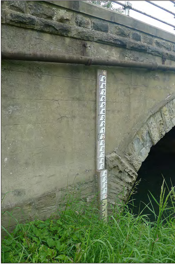
Fig 23. Detail of the western abutment of the phase-1 B6282 bridge over the River Gaunless at South Church, showing the difference in the form of the voussoirs and the exposed masonry in the causeway. (© Historic England/Marcus Jecock)
