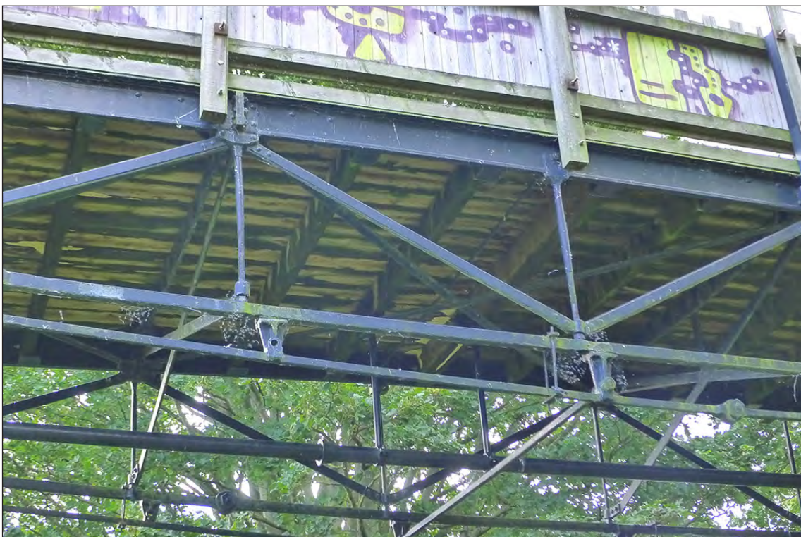
Fig 75. Detail of the chords, truss structure and cross-bracing of railway accommodation overbridge DAE2/12 (lenticular truss). (© Historic England/Marcus Jecock)
