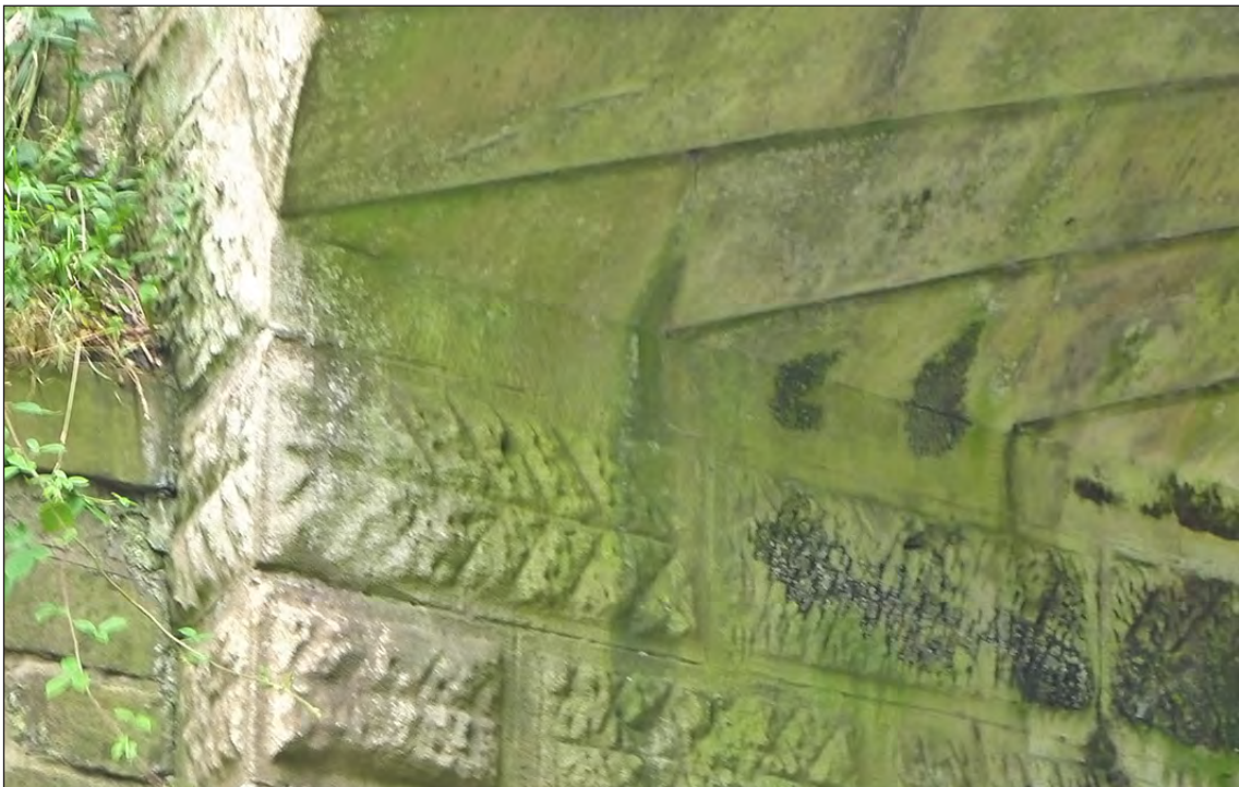
Fig 60. Detail of the arch springing on railway underbridge DAE2/7 (Bone Mill Bank). Note the stones forming the first course of the arch barrel are integral with the abutment coursing, and the distinctive way the stones of the abutment have been dressed using incised chevrons. (© Historic England/Marcus Jecock)
