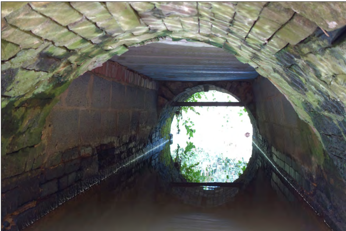
Fig 81. Detail looking through the arch barrel of 'Bishop Trevor's' culvert for the Coundon Burn in Auckland Park, showing the central section rebuilt and re-decked in modern materials. (© Historic England/Rebecca Pullen)
