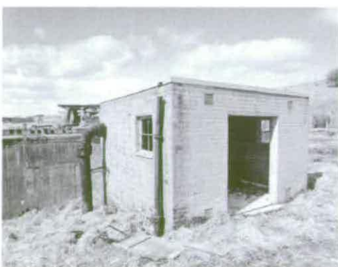
Figure 239 Pump House to the east of Effluent Lagoon C31.3 © Crown copyright NMR (AA94/2033)
