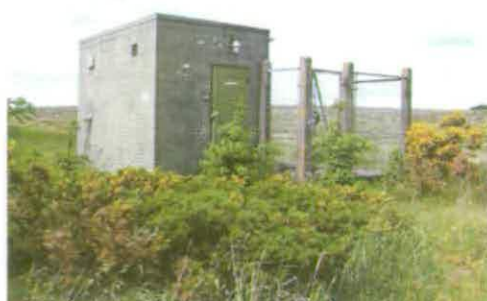
Figure 180 Electricity Sub-Station A10.4 © English Heritage (AF00134/A10.4)
