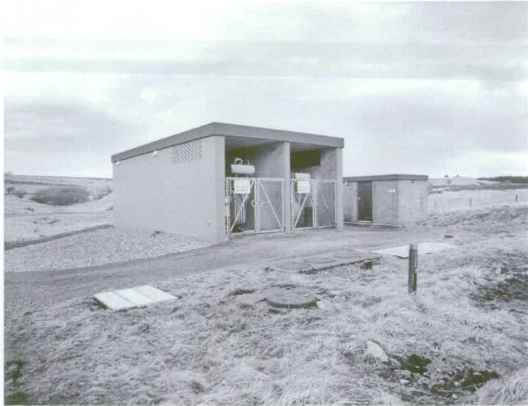
Figure 227 Electrical Sub-Station C5.4 © Crown copyright NMR (AA94/1989)
