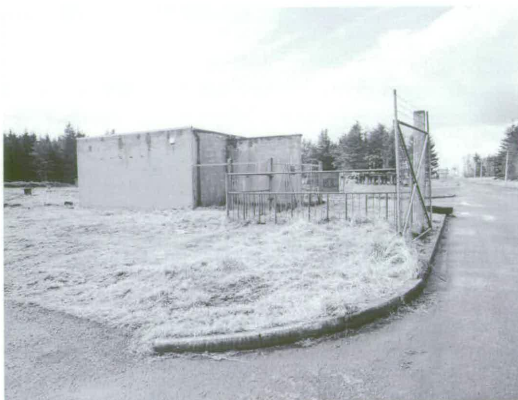
Figure 91 Sub-station D10 © Crown copyright NMR (AA94/2902)
