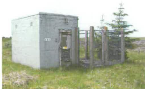
Figure 178 Electricity Sub-Station A10.2 © English Heritage (AF00134/A10.2)
