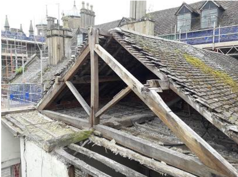
Figure 3a/b: Views of the ground-floor ceiling beams to the (top), and roof truss to the agricultural wing (bottom) (photographs Robert Howard)
