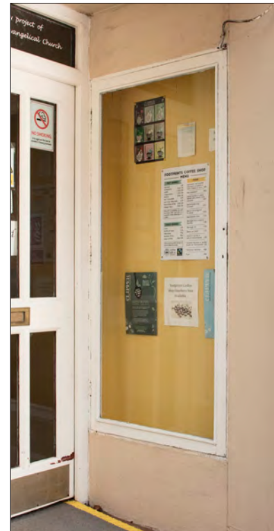
Figure 31 (right). 38B High Street, a plain shopfront with a simple wooden frame, large plate-glass window and deep splayed lobby with shallow display case. © Historic England, DP247558
