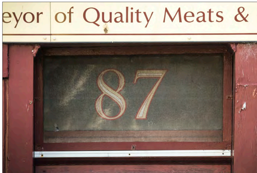
Figure 86. The hand-painted number within the fanlight of 87 High Street; the later mesh screen suggests the fanlight opened for ventilation. © Historic England DP236858
