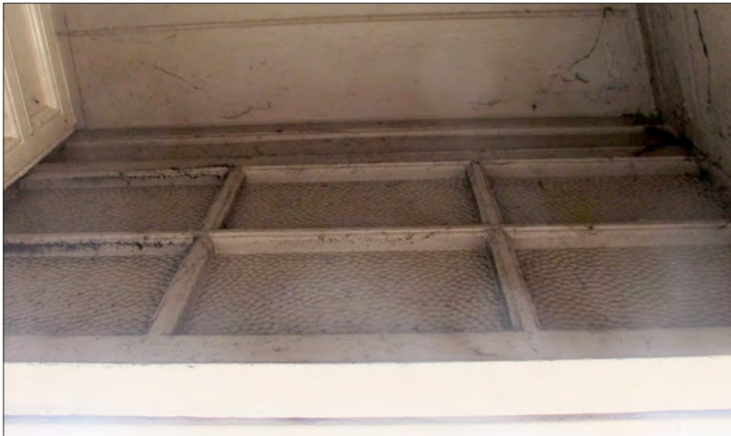
Figure 63. Behind the modern shop sign of 66 High Street, a six-pane transom light with hammered glass survives above the lobby. © Historic England, Katie Carmichael
