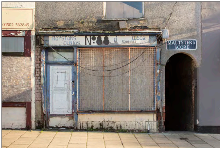
Figure 87. 88 High Street, a potentially mid-Victorian shopfront (with later alterations), currently in a very poor state of repair. © Historic England DP236859
