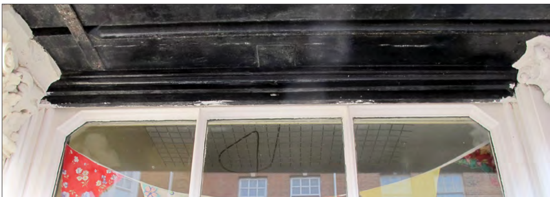
Figure 29. Wooden roller shutters appear to survive at 36 High Street – the base of a shutter is just visible above the window, set within shutter grooves. © Historic England, Katie Carmichael
