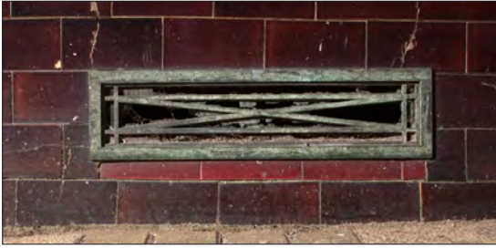
Figure 153. Geometric bronze ventilation grilles are set into ox-blood red tiled stallrisers at 144 High Street. © Historic England DP236921
