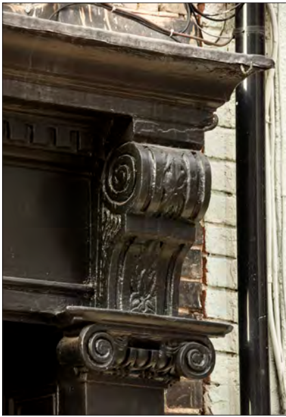
Figure 147. Classically inspired Ionic capitals and scrolled consoles at 139 High Street. © Historic England DP236916
