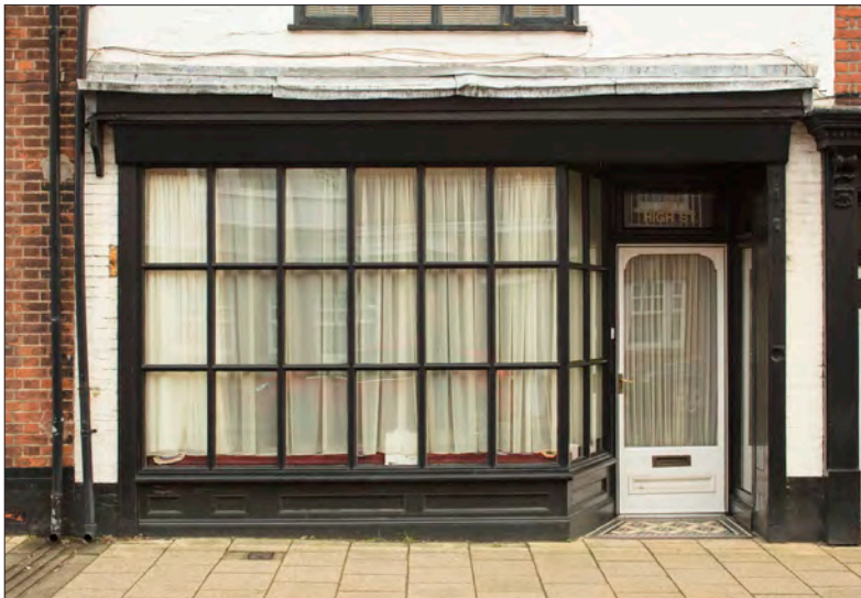
Figure 22. The early Victorian-style glazing of 31 High Street was installed in c.2002 and is set within an original Victorian framework. © Historic England DP247550
