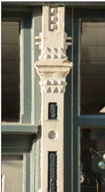
Figure 131. Elaborately carved mullions help to frame the display windows of the c.1869 shopfront at 127-129 High Street. © Historic England DP236900
