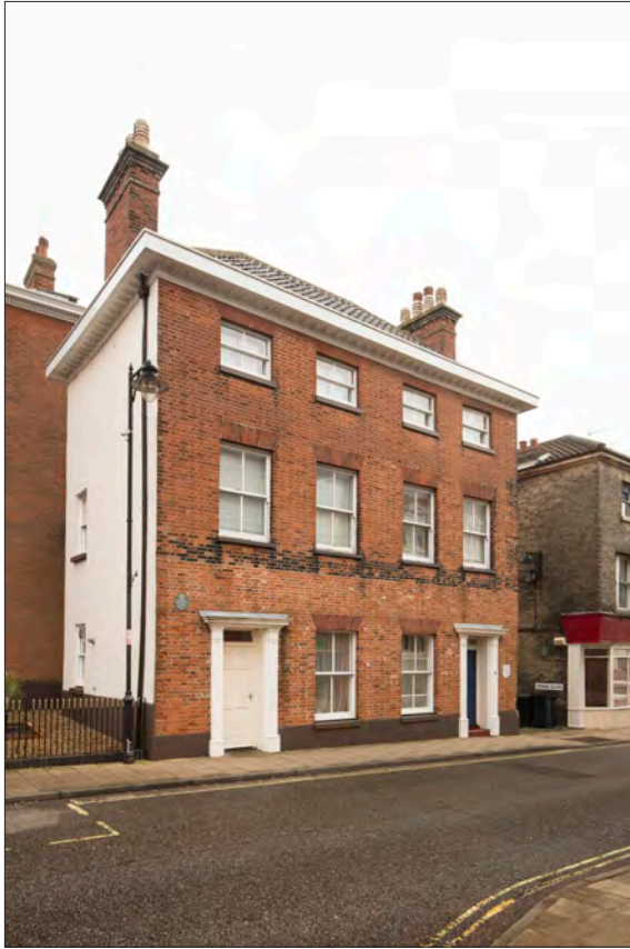
Figure 44. 50 High Street – the change in the brickwork between the ground and first floors following the removal of shopfronts is clearly visible. © Historic England DP247566
