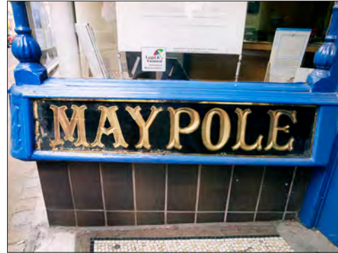
Figure 73. Maypole branding on the stallboard of 15 High Street, Leominster – a Maypole shopfront which still retains its mirrored pilasters, carved spandrels and ventilator strip. © Historic England AA009183
