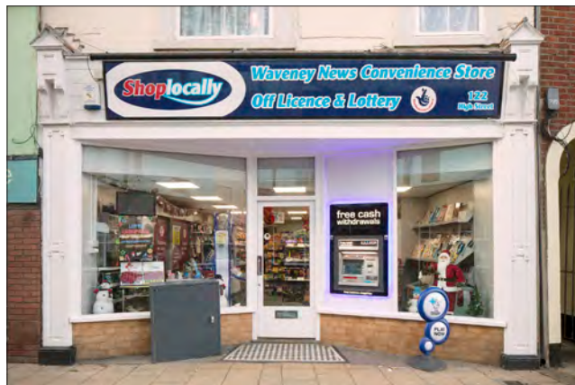
Figure 125. 122 High Street – the consoles and framework of a c.1902 shopfront survive, but the entrance and glazing date to c.1980. © Historic England DP236892
