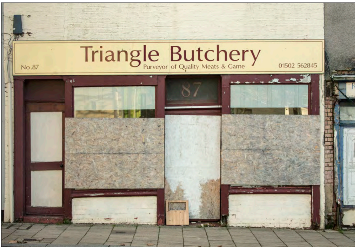
Figure 85. 87 High Street – a former butchers', now in a poor state of repair. The simple frame, where visible, suggests a date of c.1900 or a little later. © Historic England DP236857
