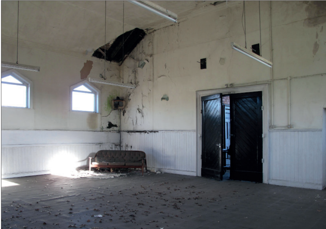
Figure 299: Poor state of repair, including partial collapse of the ceiling
