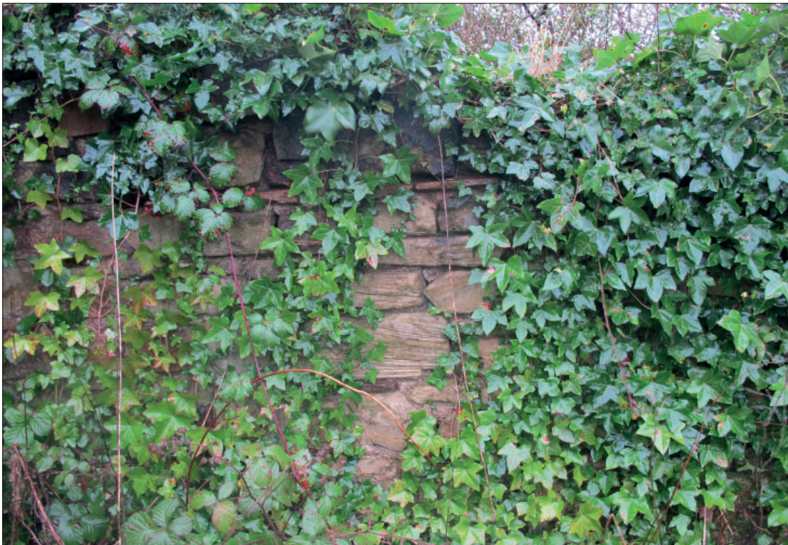
Figure 125: Heavily overgrown north boundary wall, internal view
