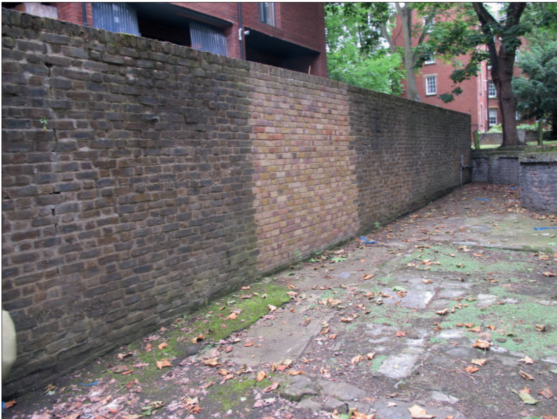
Figure 156: Blocked gap in the east boundary wall
