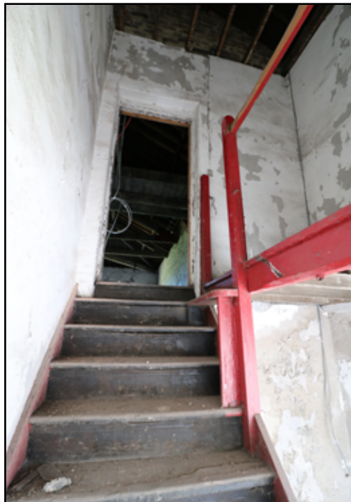
Figure 35. Staircase looking towards S2; the line of a handrail runs across the landing joist to the right with timber step providing access onto the landing.
