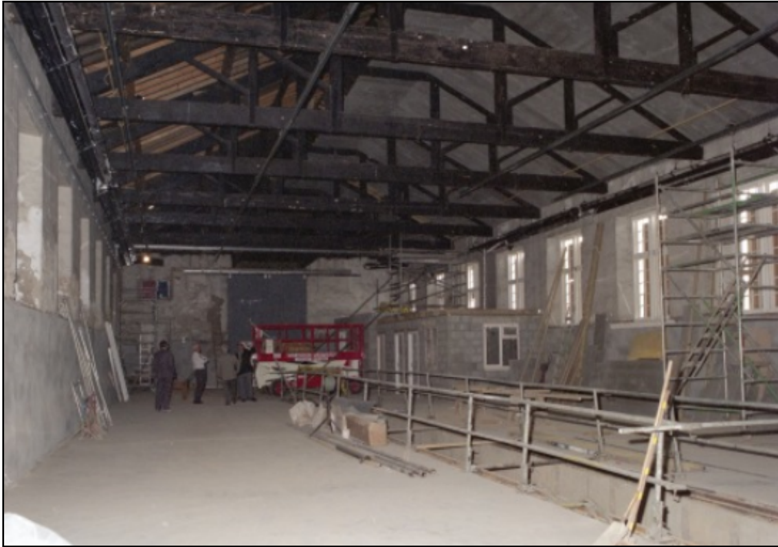
Figure 54. Photograph of 1997 the southern workshop, looking south, showing restoration in progress ( https://www.a1steam.com/darlington-locomotive-works/ ).
