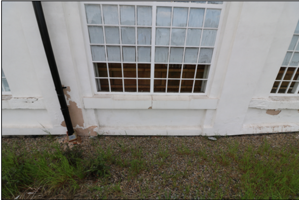
Figure 16. East elevation of the north workshop. Former doorway with modern cill and interrupted plinth below.
