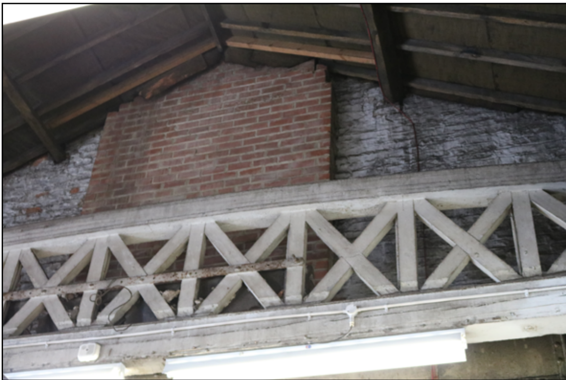
Figure 27. Chimney stack above G2 rebuilt but the original is likely to have served a fireplace to the ground floor workshop and one in S2.
