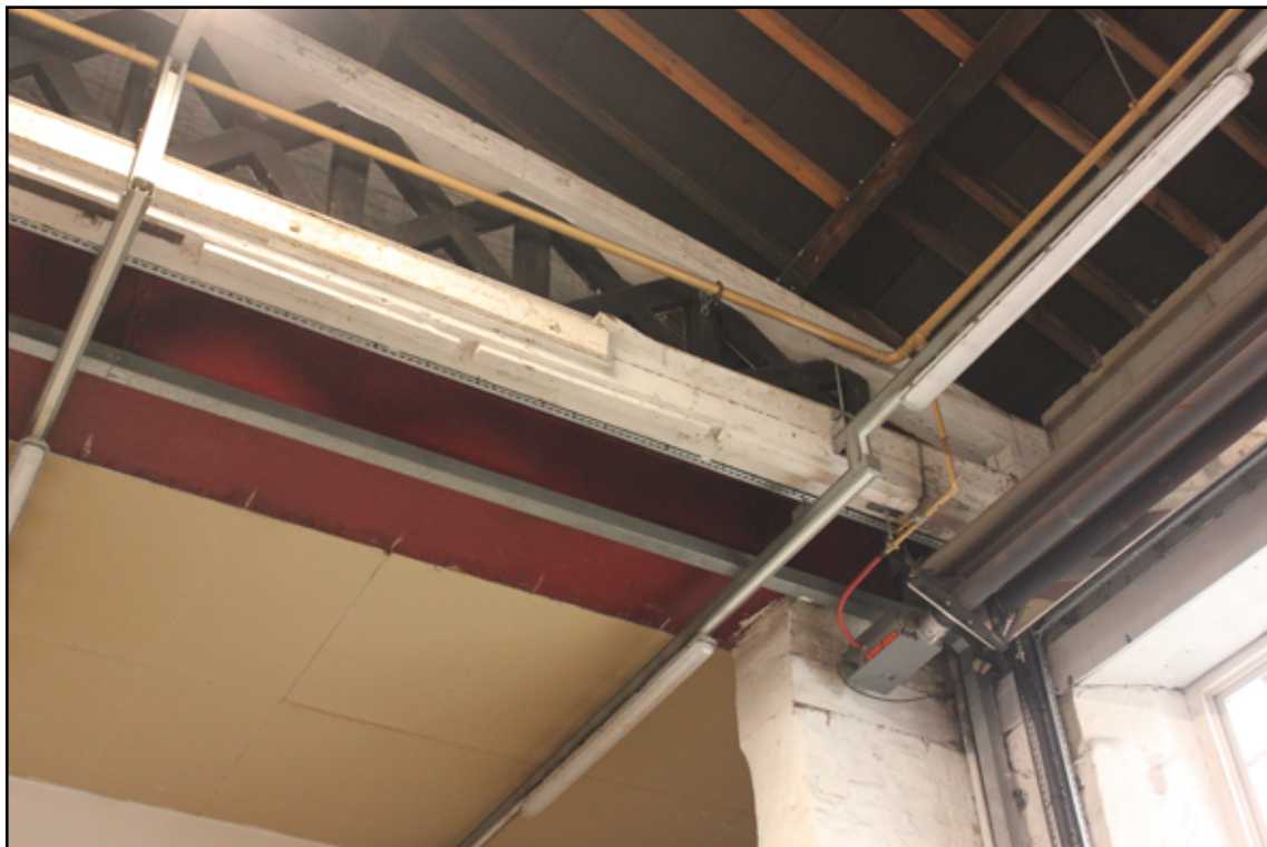
Figure 45. The bow-string truss showing the iron rail and timber stop on its outward face.
