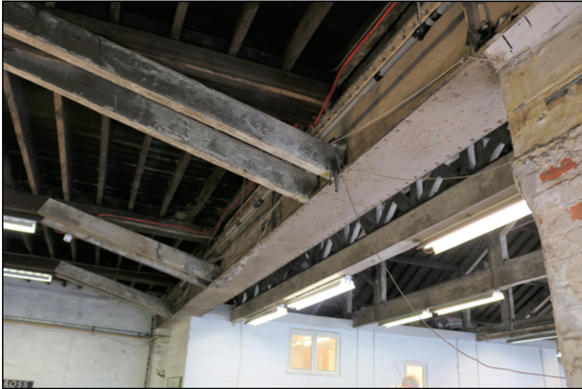
Figure 43. Box-beam in the north workshop. The timber struts support the trussed timber girder of the floor of S2.
