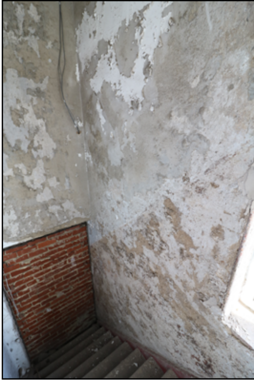
Figure 36. Bricked up doorway which formerly led into the workshops. Note the line of a wainscot or dado to the external wall to the right.
