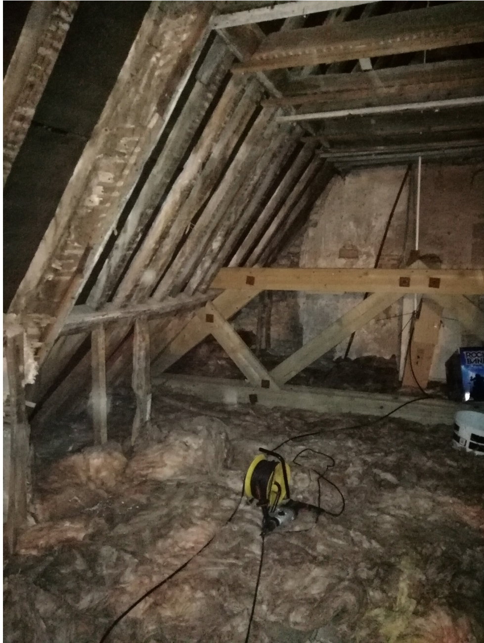
Figure 3: View of the east end of the roof (looking east) showing the form of the old roof, and a later strengthening framework (photograph Martin Bridge)
