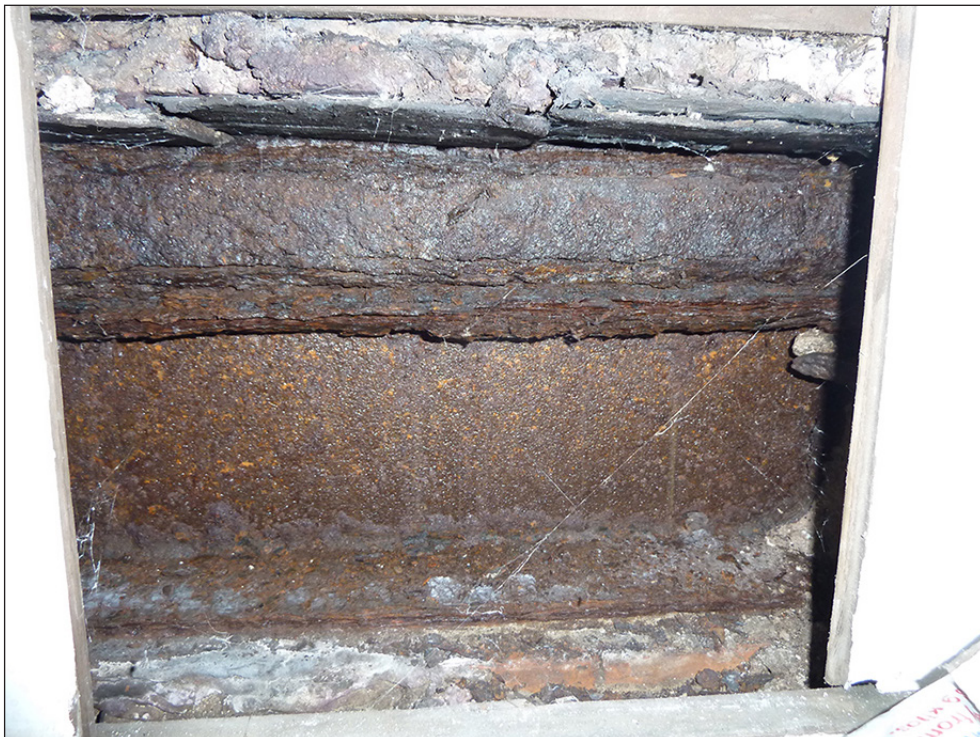
Figure 45: Rusted I-beam under the westernmost first-floor window in the south-east elevation of the market house. [Johanna Roethe]
