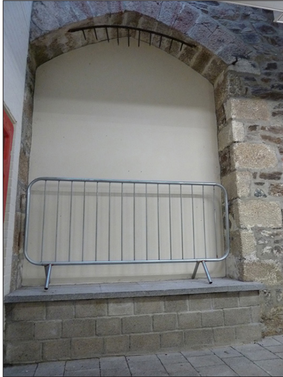
Figure 32: The blocked east arch in the south-east elevation of the meat market. [Johanna Roethe]
