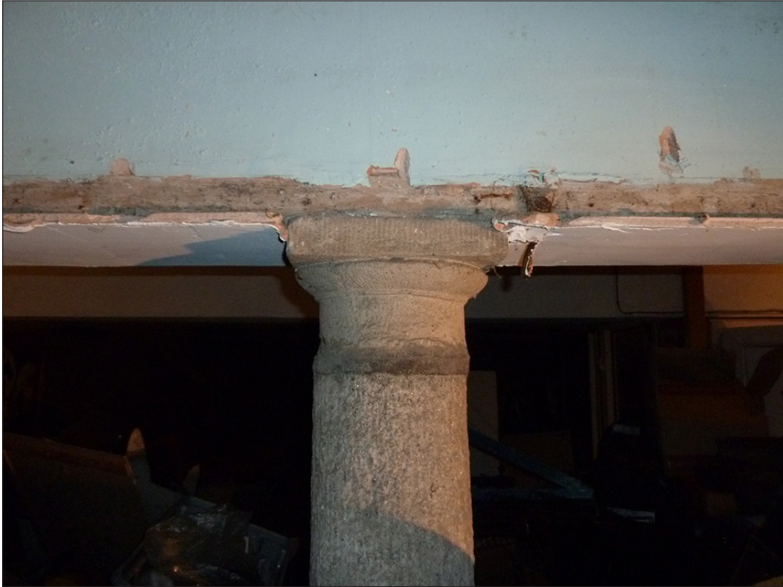
Figure 21: Granite column and capital on the lower ground floor of the Mining Exchange. [Johanna Roethe]
