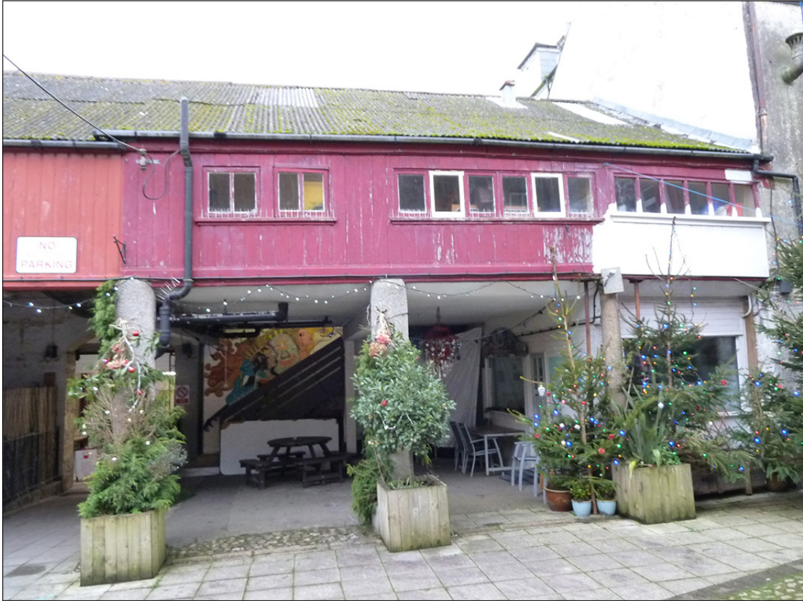
Figure 46: The first-floor offices in the north-west range with the two late-20th-century pillars to the left. [Johanna Roethe]
