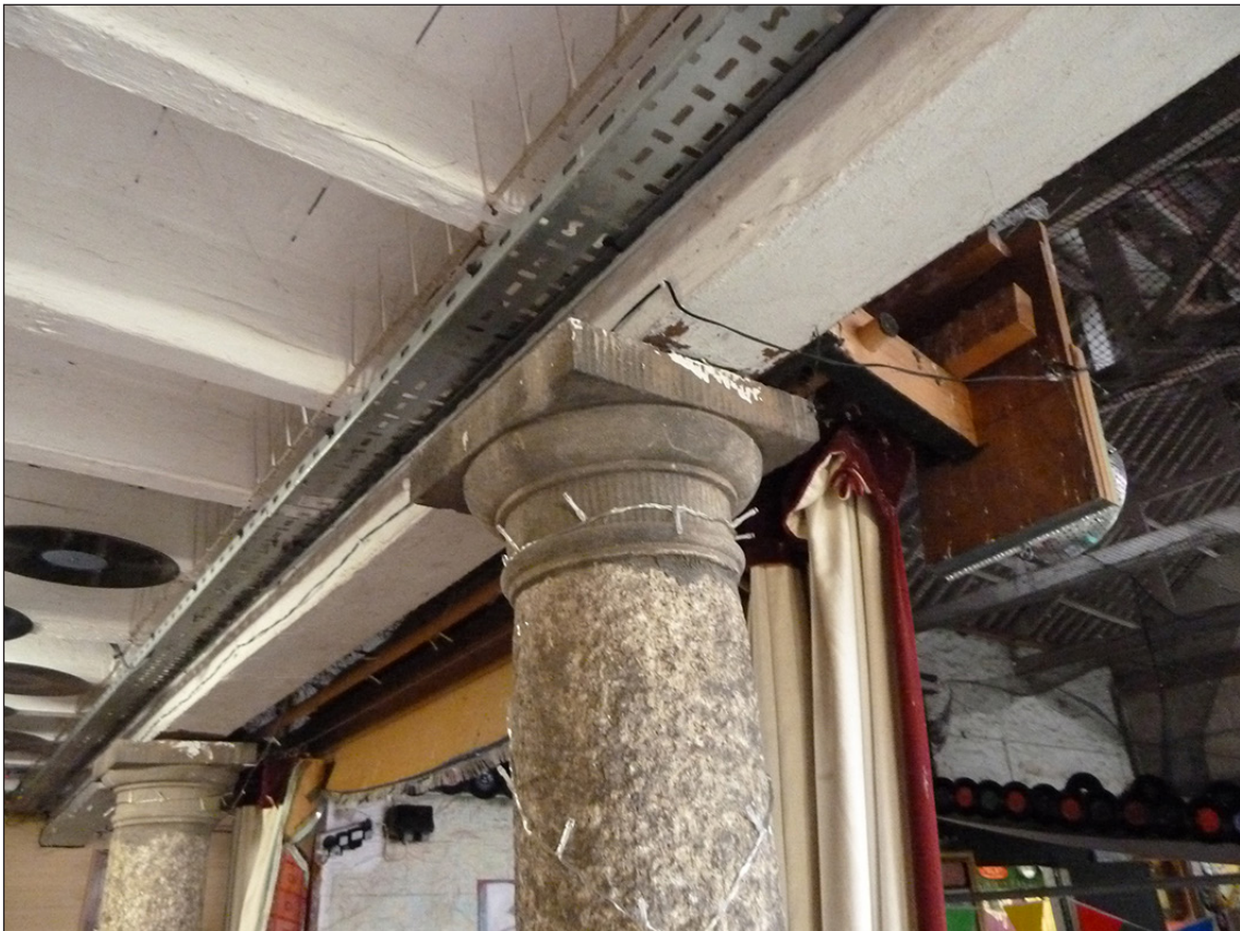
Figure 26: Two 1820s columns with mid-19th-century capitals at the north end of the south-west courtyard range. [Johanna Roethe]
