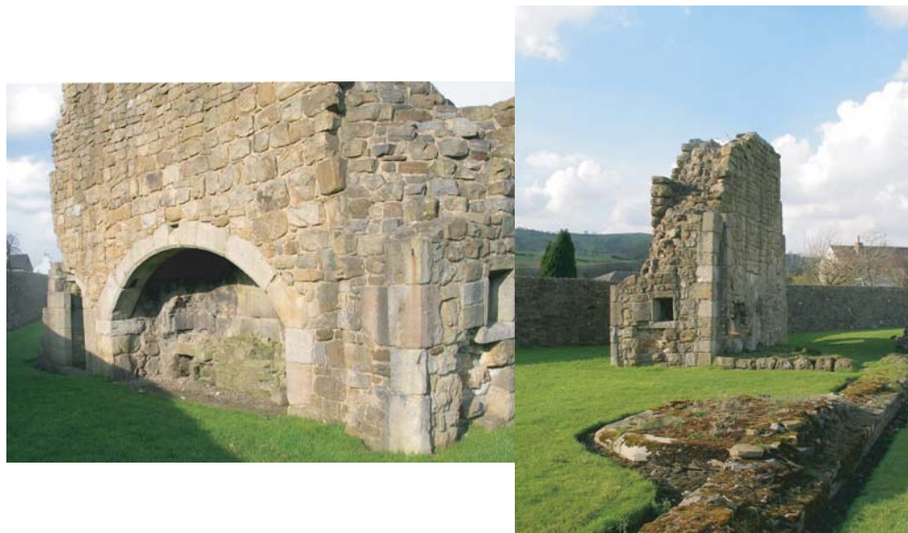
Figure 25 Photographs showing the remains of the fireplace and chimney adjacent to the western range of the cloister.
