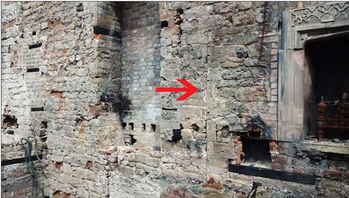
Figure 14 Straight joint visible in the north wall of the south wing, west of the first-floor fireplace (Drone survey image © Historic England)
