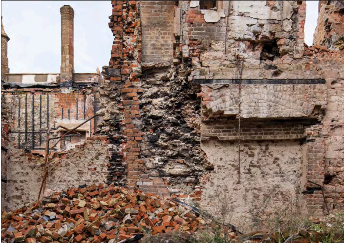
Appendix Two Figure 121: Interior, south wing, north elevation, detail of collapsed wall between south wing and dining room, looking north (DP276011)
