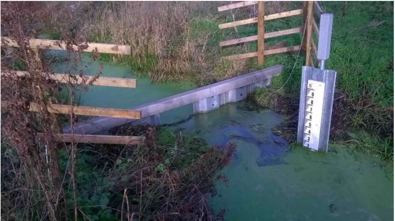
Figure 95 The new water control structure and gauge board at the northern end of the ditch on the west side of the site
