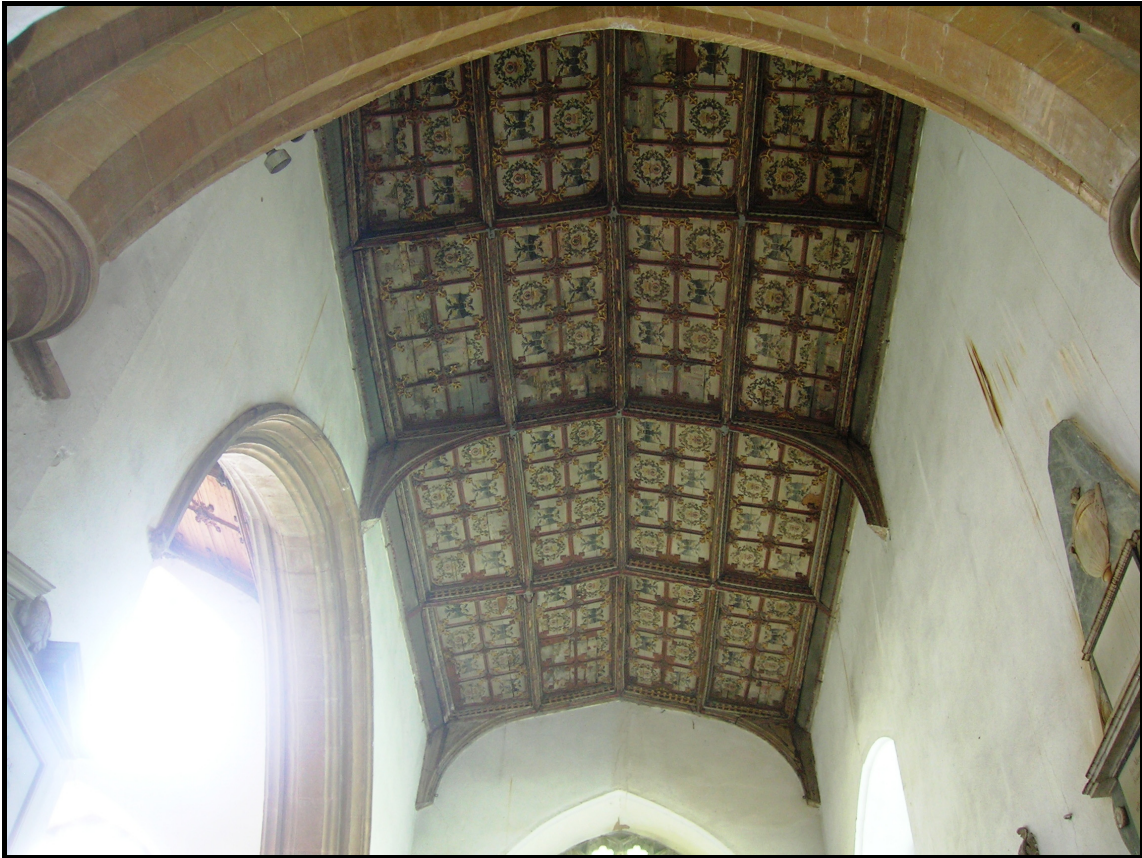
Figure 6: North chapel ceiling (as viewed from below) with north transept to the left
