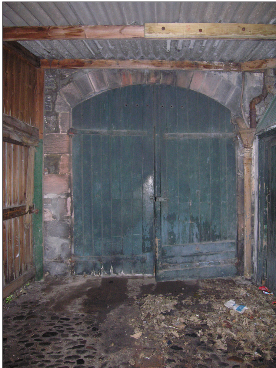
Fig. 44: The carriage house arch in the western end of the southern wall of the granary. © English Heritage
