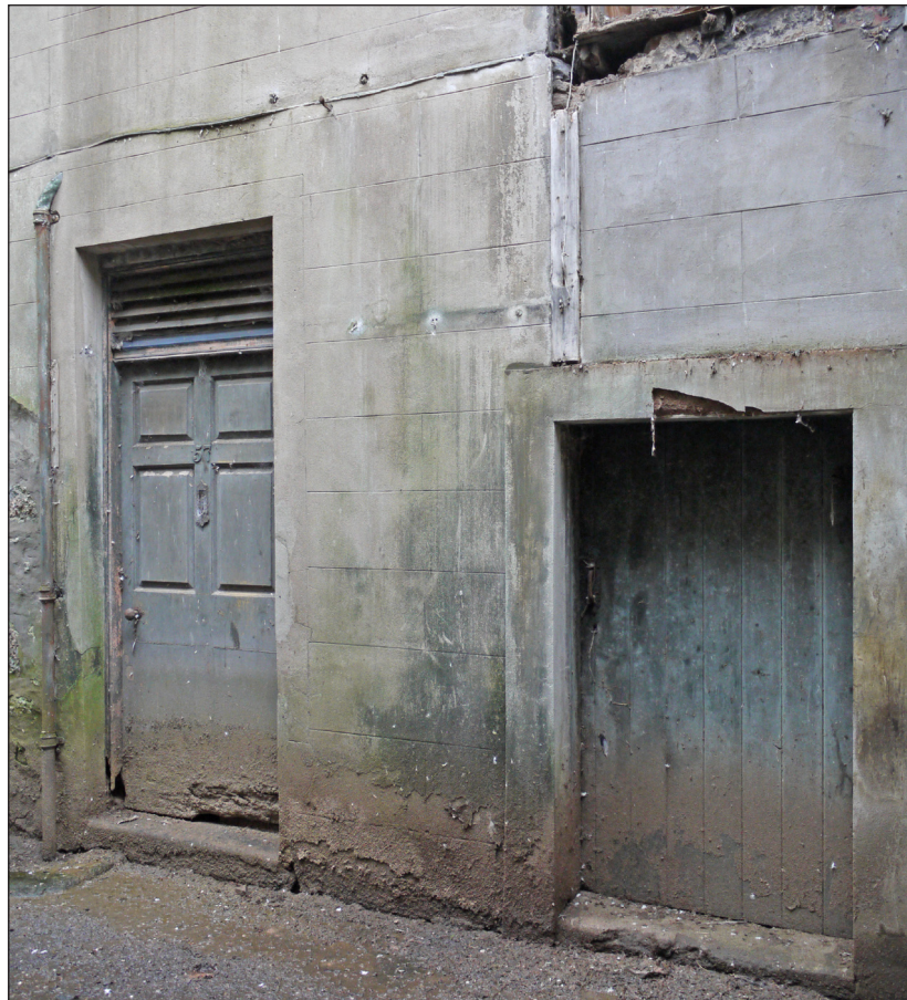
Fig. 41 (right): The lower doorway, seen from the yard of 2 Love Lane / 64 West Street, with its raised stone surround belongs to the original stable and coach house. © English Heritage
