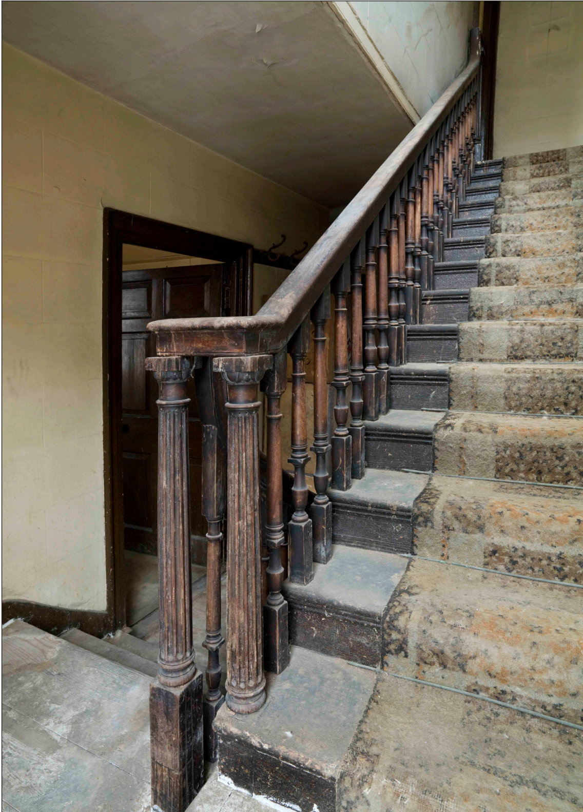
Fig. 67: The main stair, with its column newels and two balusters per tread, in the principal range of 57 West Street / 64-66 Bridge Street. The lower flight has been shortened by one step, and the corresponding newel lengthened, to maintain headroom when the second-floor west room was extended into the stair compartment. DP065374 © English Heritage
