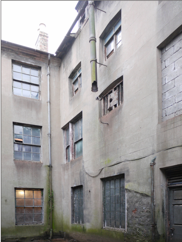
Fig. 50 (left): Altered fenestration in the south wall of the granary, including a paired sash window on the first floor. © English Heritage
