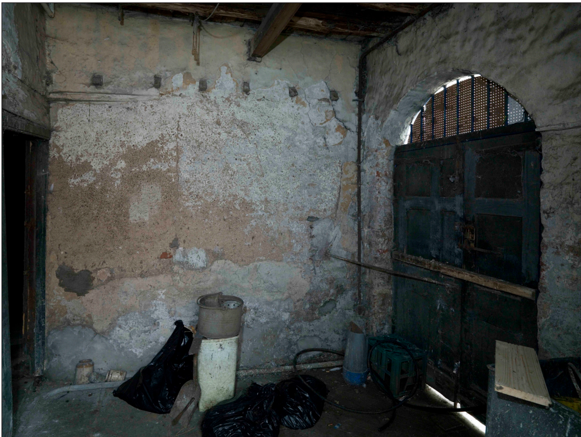
Fig. 76: The yard entrance at the side of 57 West Street / 64-66 Bridge Street, looking south-west. The rafter ends of a former pent roof are visible a little below the ceiling of the added rear range. DP065402 © English Heritage
