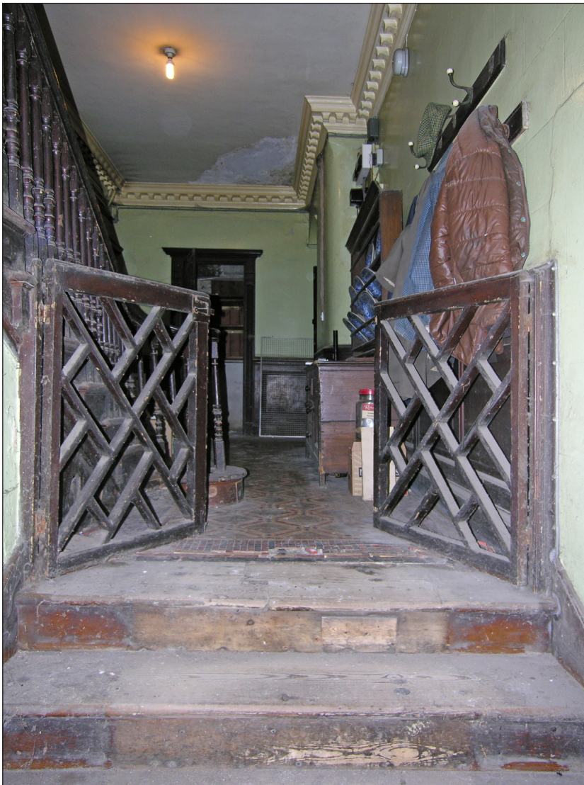
Fig. 18: The 18th-century dog-gate in the stair hall of 2 Love Lane / 64 West Street. © English Heritage
