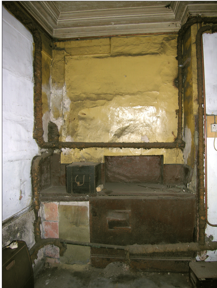
Fig. 19: The original dining room, complete with high-status cornice, later used as a kitchen at 2 Love Lane / 64 West Street. The chimney breast projects to the right. © English Heritage
