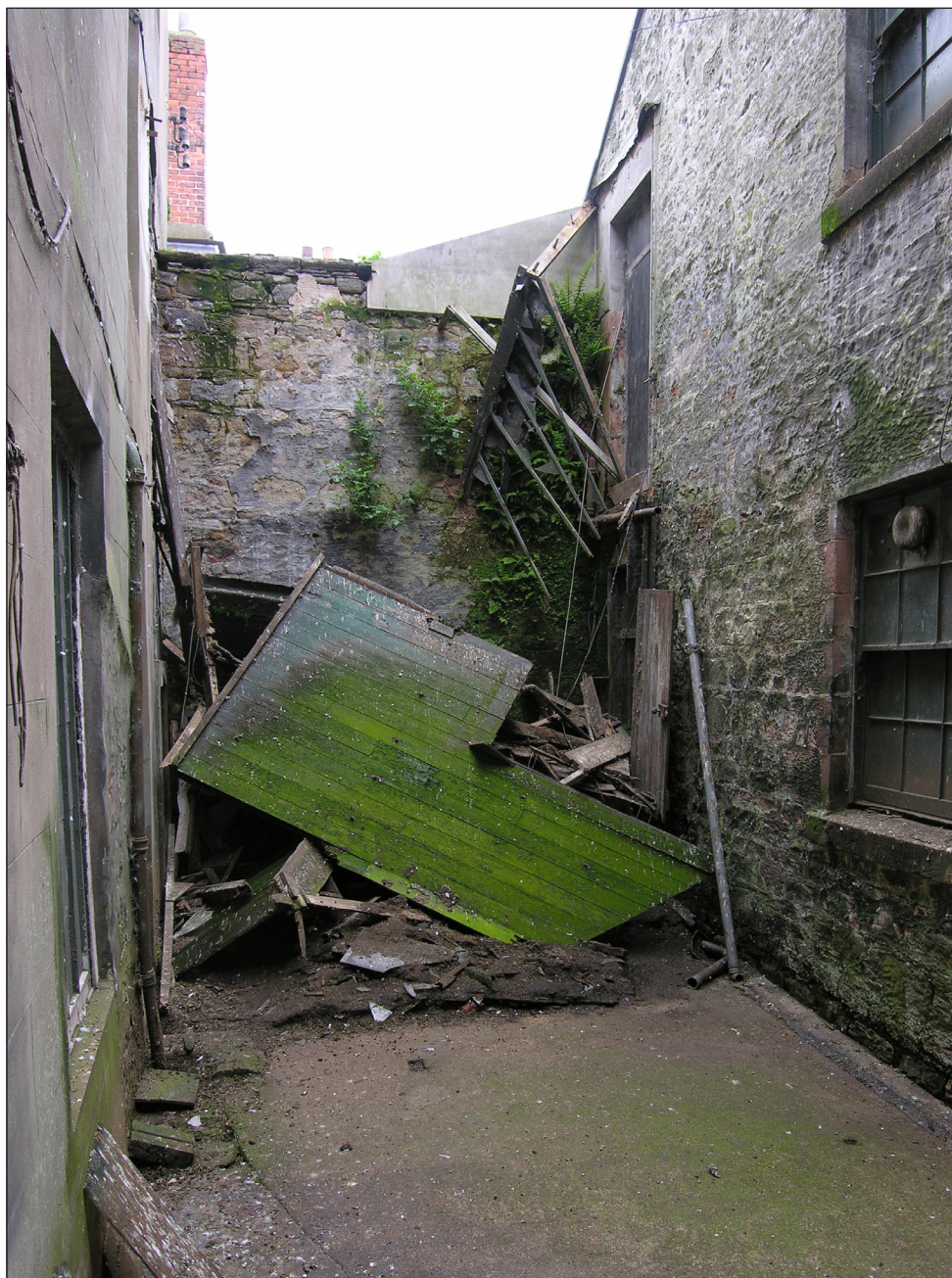
Fig. 53: The collapsed timber corridor which crossed the internal yard between 2 Love Lane / 64 West Street and the granary (60 West Street). © English Heritage
