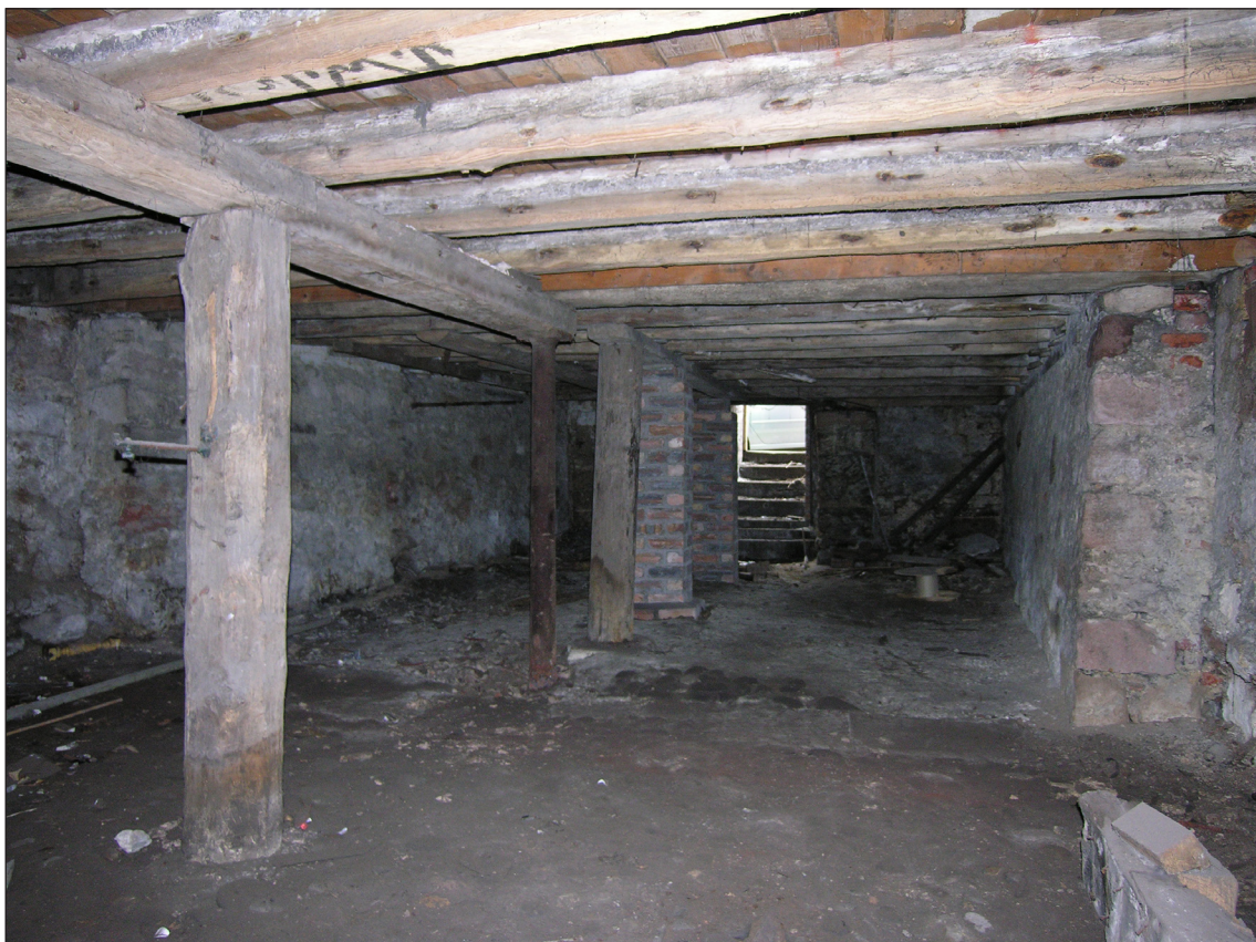
Fig. 38: The cellar of 2 Love Lane / 64 West Street, looking west. The ceiling bears a series of painted inscriptions, including J Wilson's name on a joist and the date 1887 (not visible) on plaster. The supporting axial beam and Samson posts are more characteristic of 18th- and early 19th- century warehouses and granaries. © English Heritage
