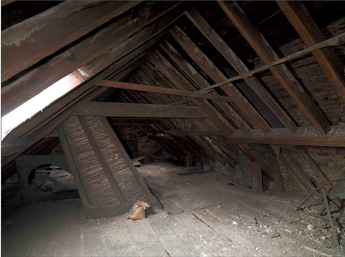
Fig. 27: The roof of the front range of 2 Love Lane / 64 West Street. The boxed-in skylight illuminates the stair serving the western first-floor room. DP065340 © English Heritage
