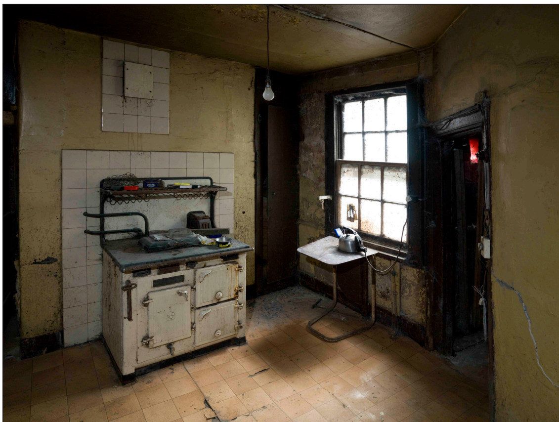
Fig. 66: The kitchen, at the rear of 57 West Street / 64-66 Bridge Street. DP065400 © English Heritage
