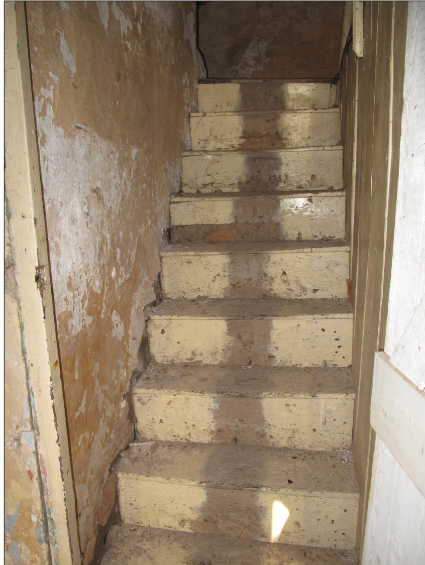
Figure 60 The current stair, probably in the location of an earlier stair arrangement, looking north [© Historic England Rebecca Lane]
