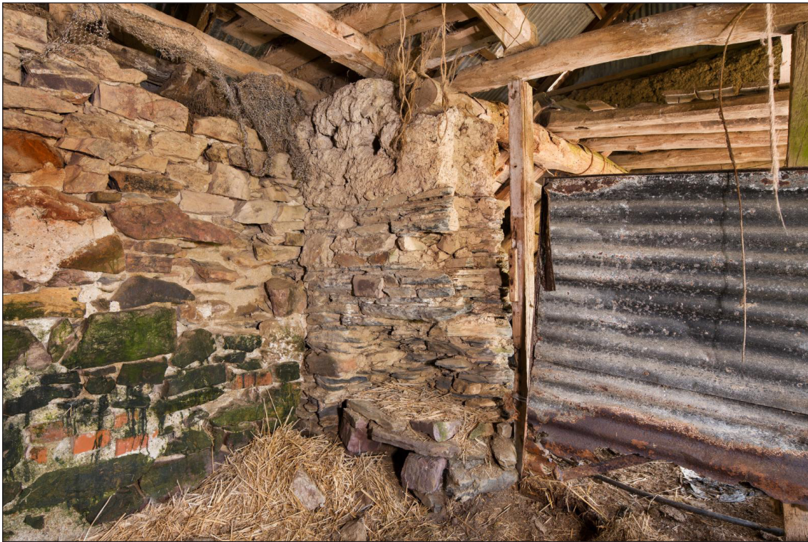
Figure 47 Former west wall of the linhay, looking north east. The west wall is on the right-hand side of this photograph, with the spine beam of the linhay resting in the upper cob section. The stone walling on the left-hand side of the photograph is a later insertion [DP220526]
