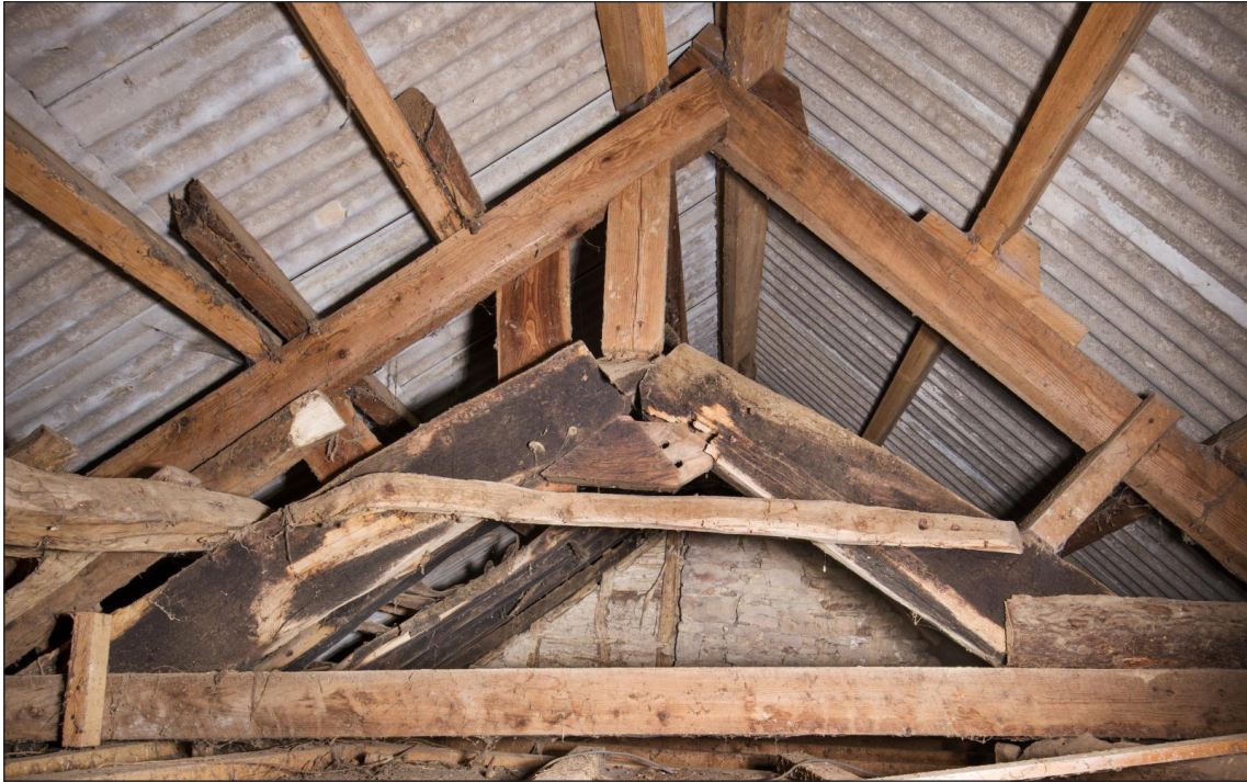
Figure 20 Apex of the eastern side of truss C-C1 as viewed from the linhay looking west, showing the yoke which joined the two blades together. The original truss is distinguished from the later timber by the surviving smoke blackening on the timbers. Also visible are smoke-blackened common rafters on the southern side of the roof [DP220553]
