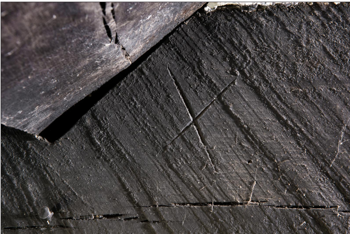
Figure 17 Scratch carpenter's mark on the eastern side of the southern principal rafter of truss A-A1, looking west [DP220566]
