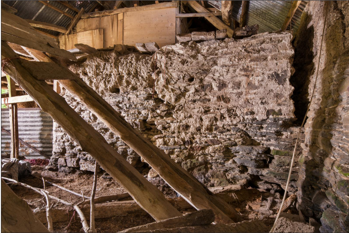
Figure 45 View of the former west wall of the linhay, looking west. The section to the south (left-hand side) appears to be formed of stone and cob, with the section further north formed of stone, the upper part of this is probably a later reconstruction [DP220520]
