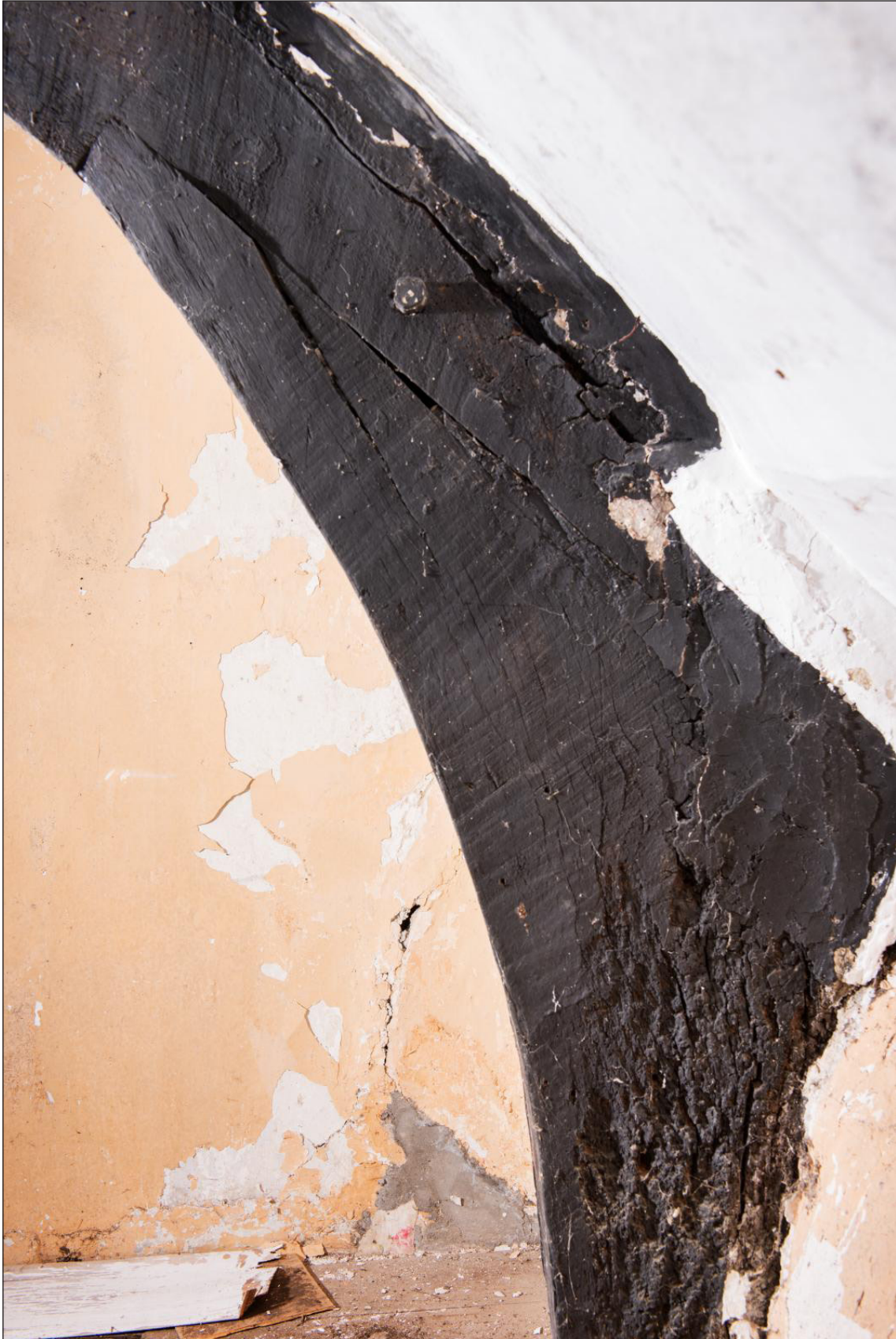
Figure 19 Western side of the southern cruck blade of truss B-B1, looking east, showing the junction of the two parts of the blade and the side pegging [DP220562]
