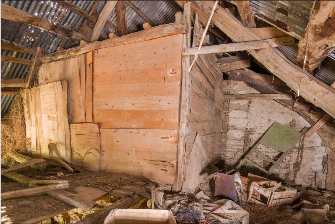
Figure 32 Partition between the former east first-floor room and the cross passage, looking west. Note the plaster visible on the eastern side of the partition wall immediately adjacent to the original northern cruck blade, on the right-hand side of this photograph [DP220519]
