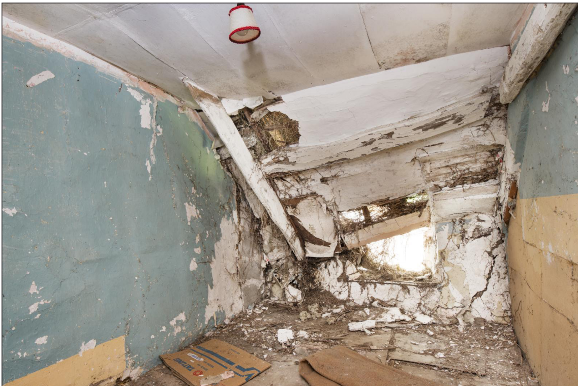
Figure 23 First-floor eastern room, looking south east, showing southern purlin which may be part of the original roof structure, with other later timbers [DP220551]
