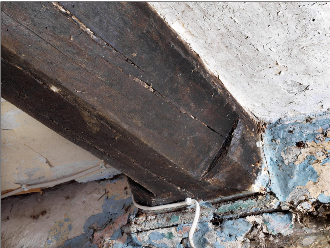
Figure 37 Southern end of the central cross beam in the hall, showing the keel chamfer stop, looking south east [DP220753]
