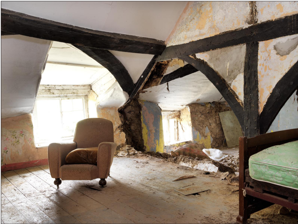
Figure 22 Upper part of hall, looking south west towards truss A-A1, showing purlin and wind brace arrangement to either side of the truss [DP220757]
