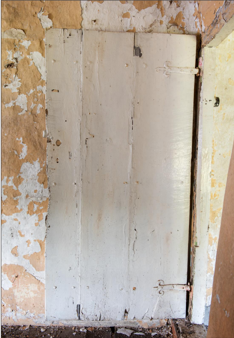
Figure 40 Door between the first-floor landing and the room over the hall [DP220569]
