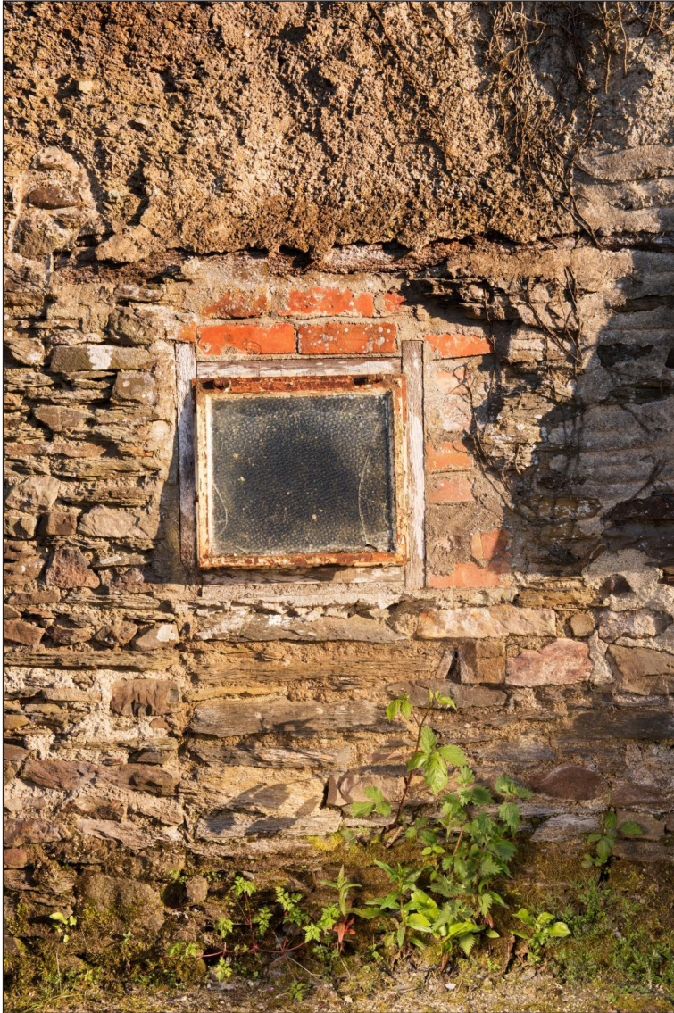
Figure 9 North elevation, showing bathroom window inserted into the former north doorway of the cross passage, looking south [DP220572]
