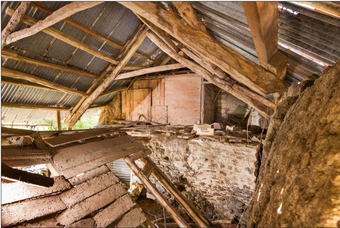
Figure 53 Interior of the linhay, looking south west. Note the former west wall of the linhay has been reduced to the height of the tallet, to allow the extension of the hay loft over the former low end of the farmhouse [DP220515]
