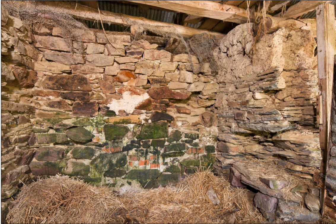
Figure 58 Rebuilt section of walling abutting the former west wall of the linhay, showing inclusions of bright red brick at low level, looking north east [DP220525]
