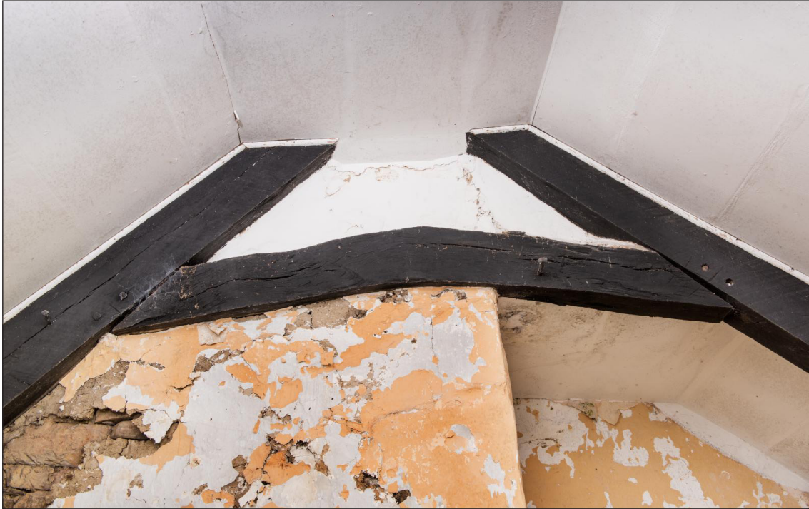
Figure 18 Upper part of truss B-B1, looking east, partially built into the later chimney breast [DP220564]
