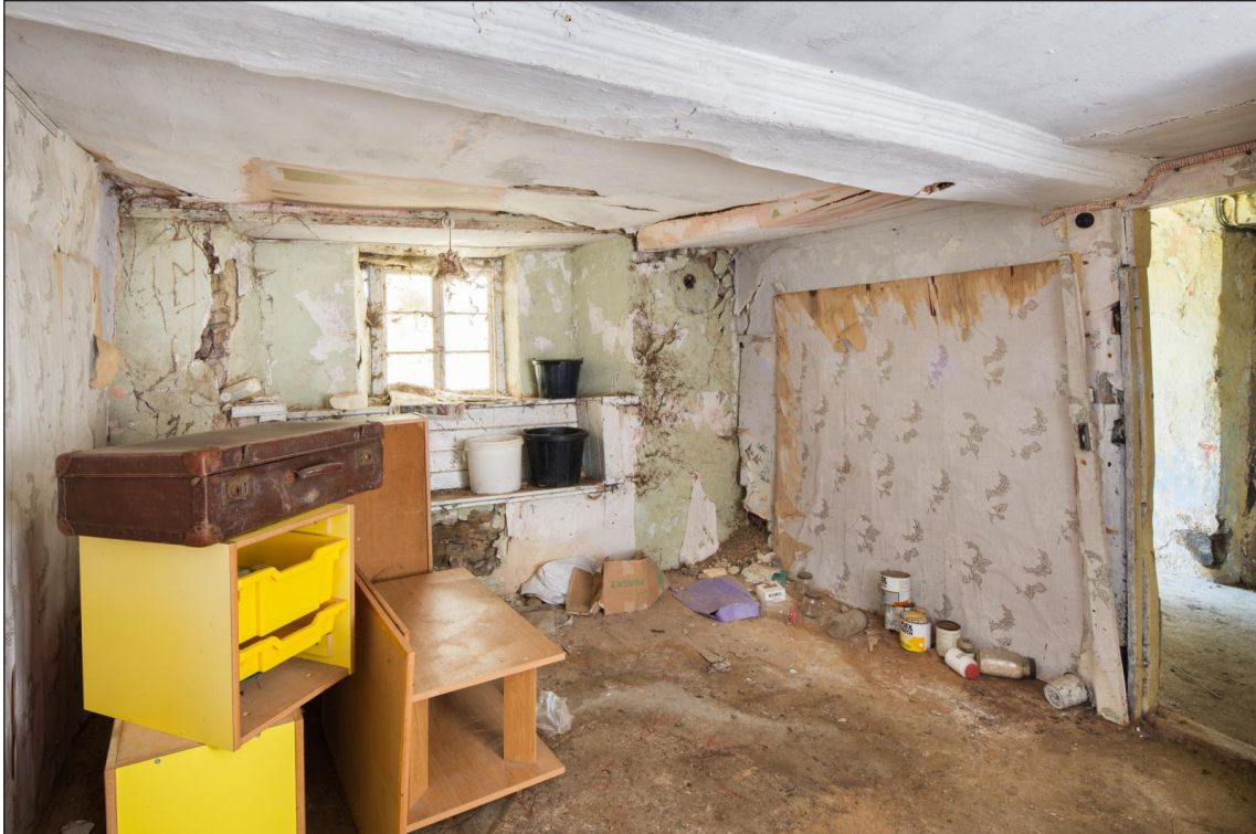
Figure 21 Ground-floor eastern room, looking south west, showing the profile of the post surviving in the partition between the room and the cross passage, adjacent to the current doorway [DP220542]
