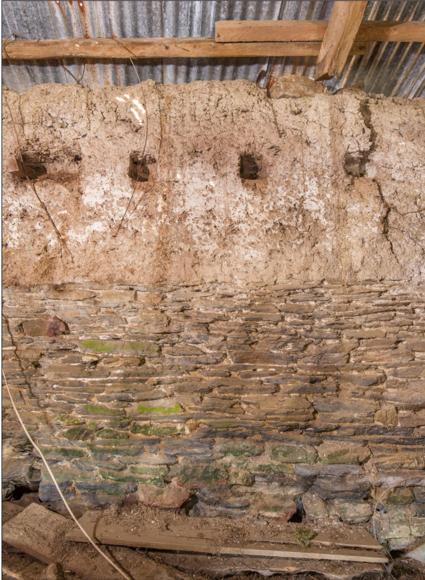
Figure 50 North wall of the linhay showing the sockets for the joists of the tallet (DP220517).
