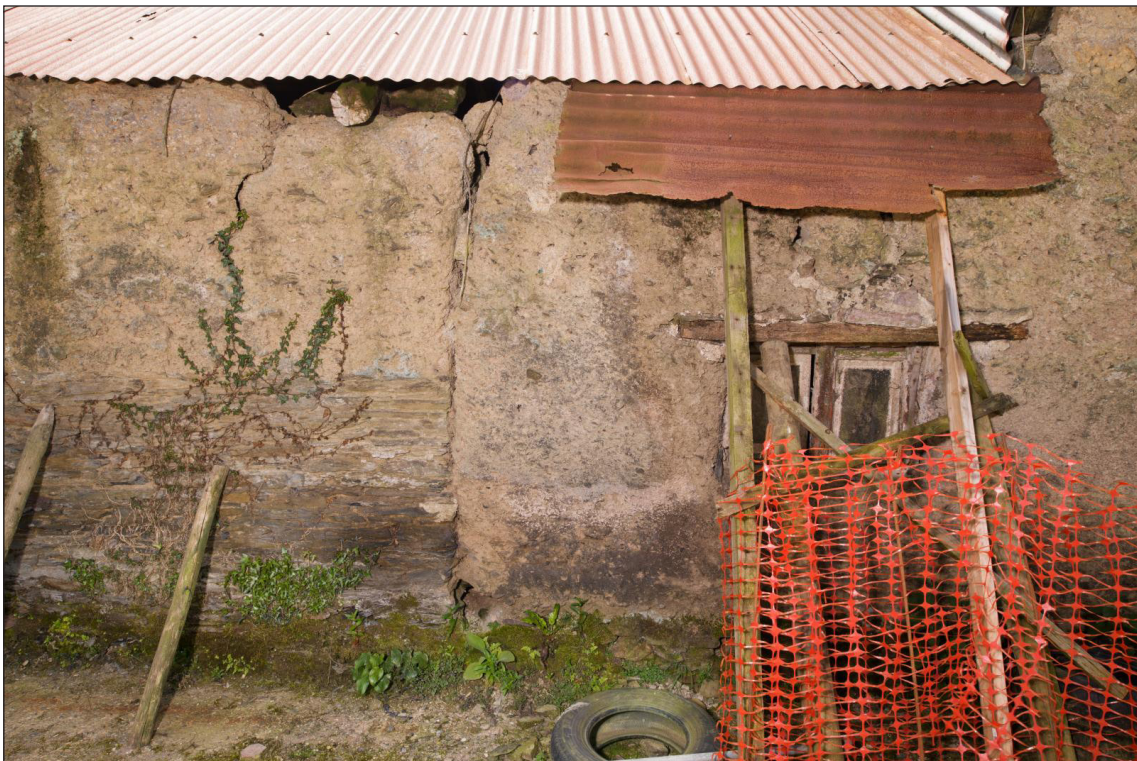
Figure 46 The north elevation of the linhay and farmhouse, looking south. Note the straight joint between the wall of the linhay and the wall of the farmhouse, and the significant difference in the height of the stone plinth between the two [DP220511]
