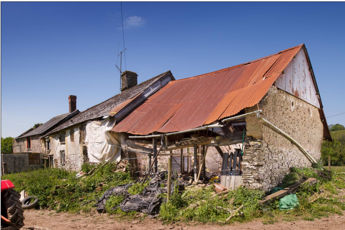
Figure 43 The south and east elevations of the linhay, looking north west [DP220513]
