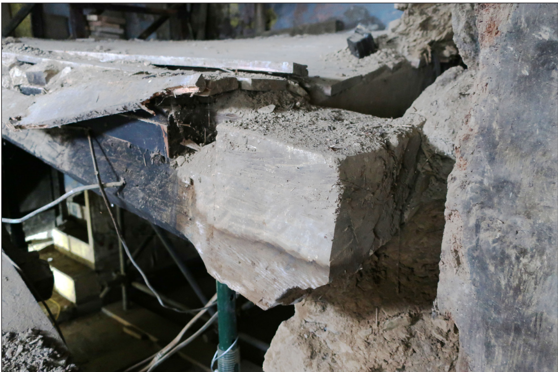
Figure 26 Detail of the east end of the inserted spine beam visible due to the collapse of the inserted cob wall, looking north west [© Historic England Rebecca Lane]
