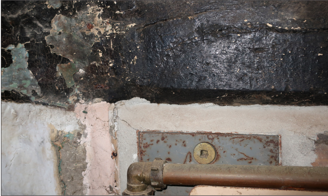
Figure 28 Detail of the chamfer and associated chamfer stop on the bressumer of the fireplace in the ground-floor west room [© Historic England Rebecca Lane]
