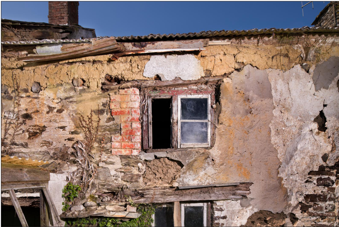
Figure 57 Window of the first-floor western room, looking north. Note the rebuilt western jamb in red brick with bull-nose profile [DP220528]
