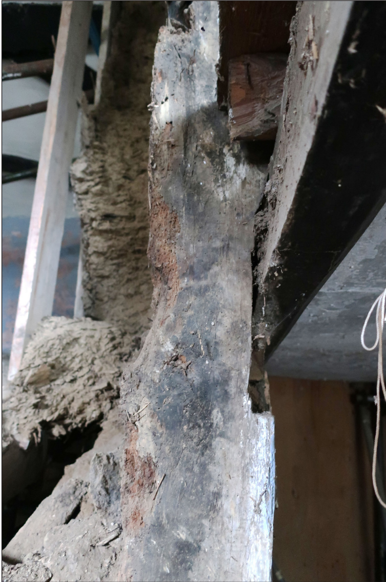
Figure 14 View of the southern side of the central post of the partition under truss A-A1, looking north, showing the joint for an original mid-rail with a smaller, later timber now in the same position [© Historic England Rebecca Lane]
