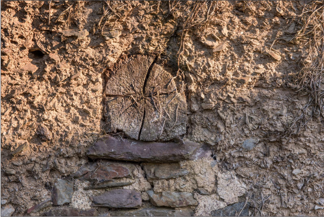
Figure 36 Northern end of the central cross beam inserted into the hall, visible externally in the north elevation, looking south [DP220537]
