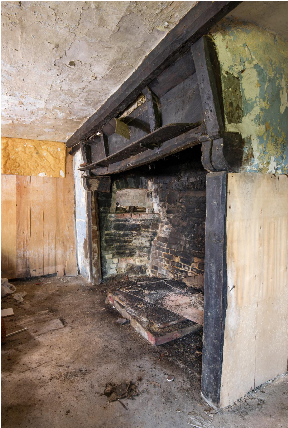
Figure 38 The early 16th-century fireplace, with later cross beam supported on timber brackets attached to the bressumer, looking north east [DP220537]
