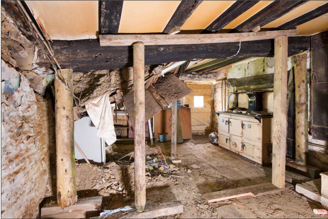
Figure 25 Ground-floor west room, showing the floor inserted as part of Phase Two, looking south [DP220539]
