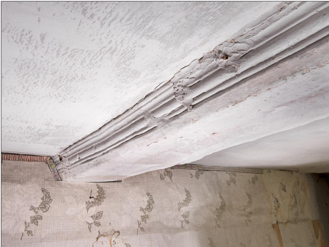
Figure 34 Encased spine beam in the eastern ground-floor room, looking south east. Note the residual plasterwork on its northern face [DP220560]
