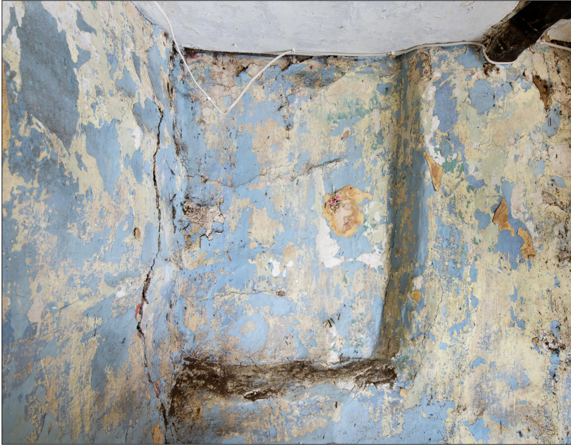
Figure 10 Recess visible in the south elevation in the hall, possibly an original window opening, looking south [DP220535]
