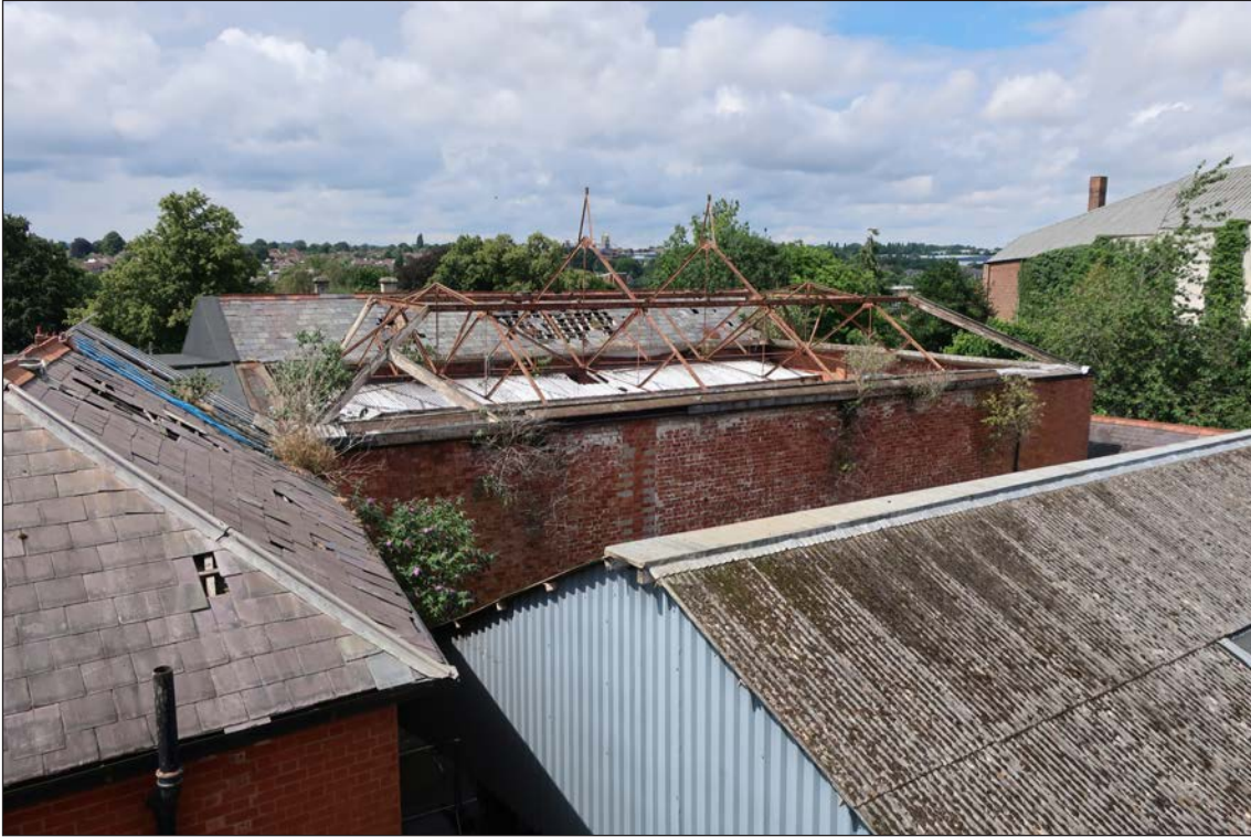
Figure 55: Roofs over the courtyard, viewed from the hotel fire escape.[© Historic England, Aimee Henderson]
