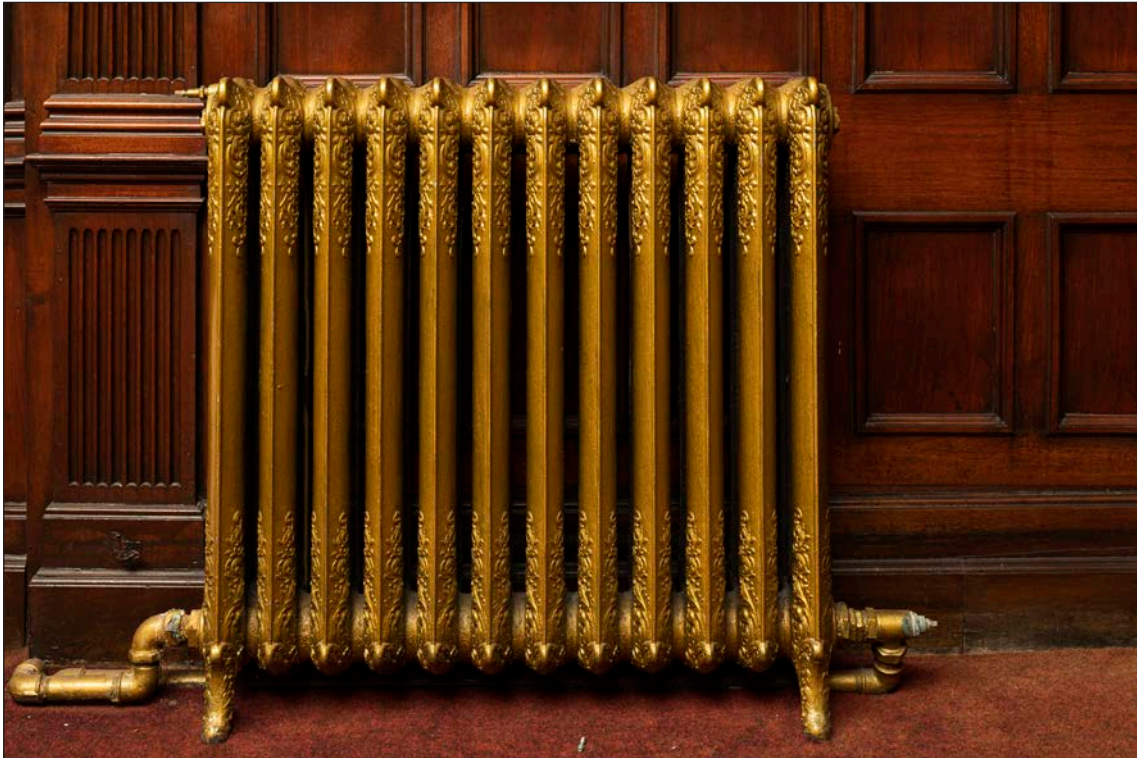
Figure 38: Cast iron 'Beeston Decorated' radiator, example from the restaurant, [DP311973]
