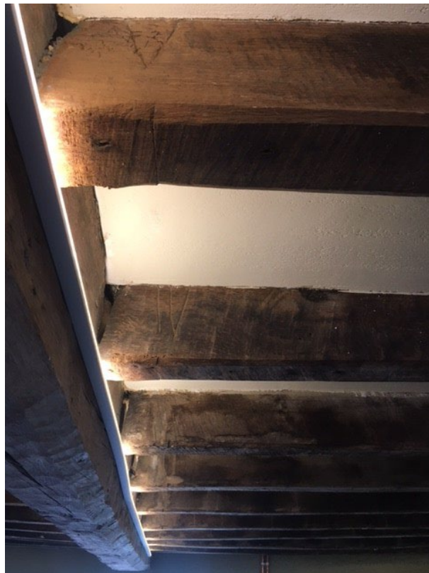
Figure 5: Chamfered and stopped joists in bay 3, photograph taken from the east (Alison Arnold)
