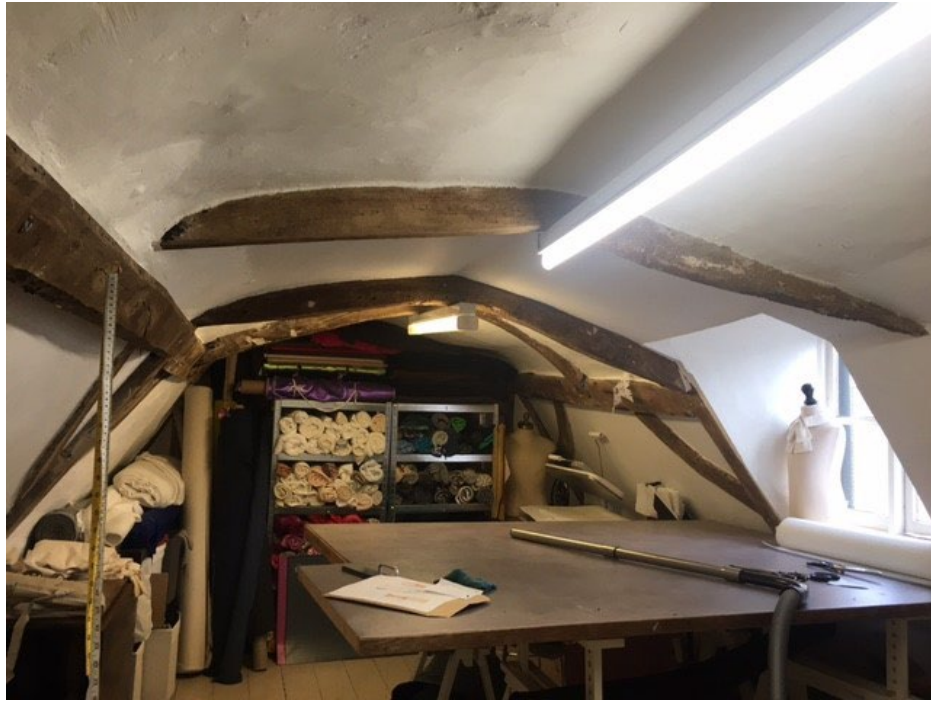
Figure 2: Roof (No 26), truss 5 and one of the intermediary collars in the foreground, photograph taken from the south (Alison Arnold)
