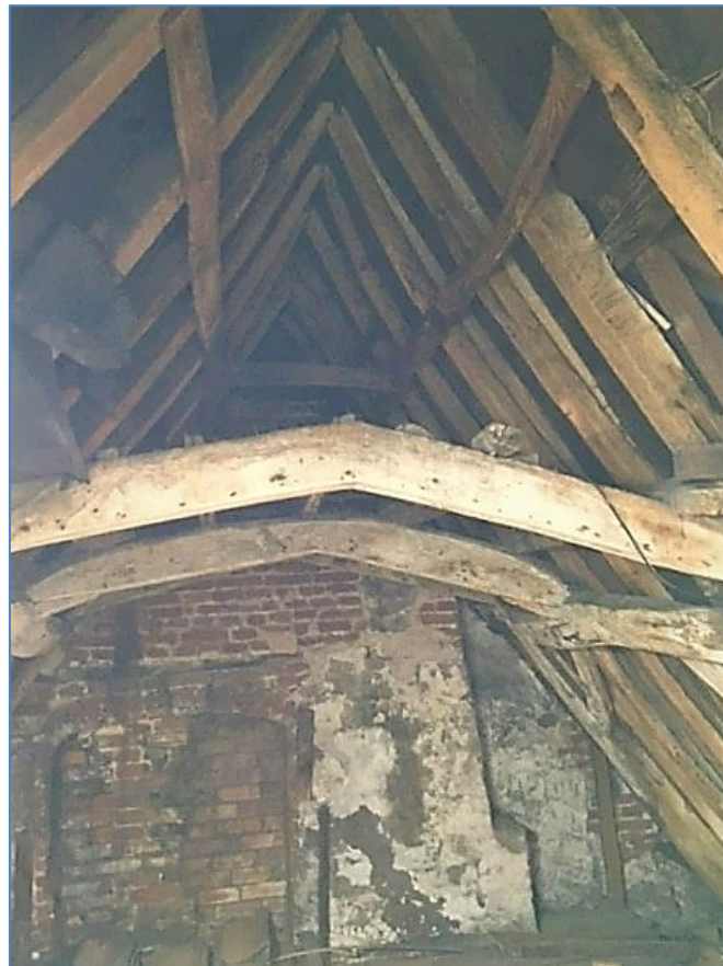
Figure 3: Roof (No 27), truss 2 in foreground, photograph taken from the south (Alison Arnold)
