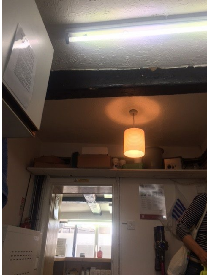
Figure 6: Ground-floor ceiling beam (No 27), the chamfered beams can be seen in the background, photograph taken from the west (Alison Arnold)
