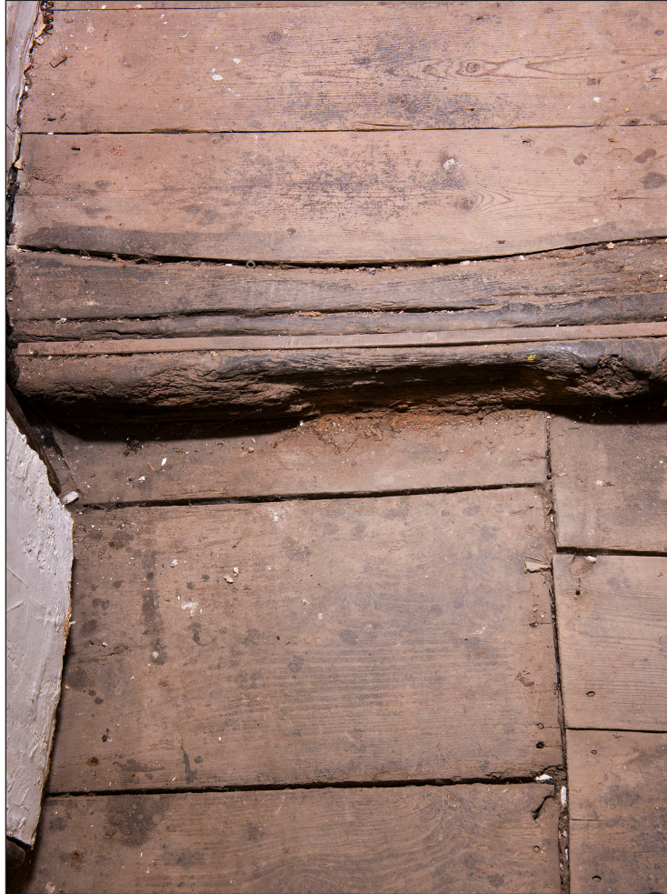
Figure 31 Interior, first floor, north room, detail of transverse partition running through the building. [DP219902]
