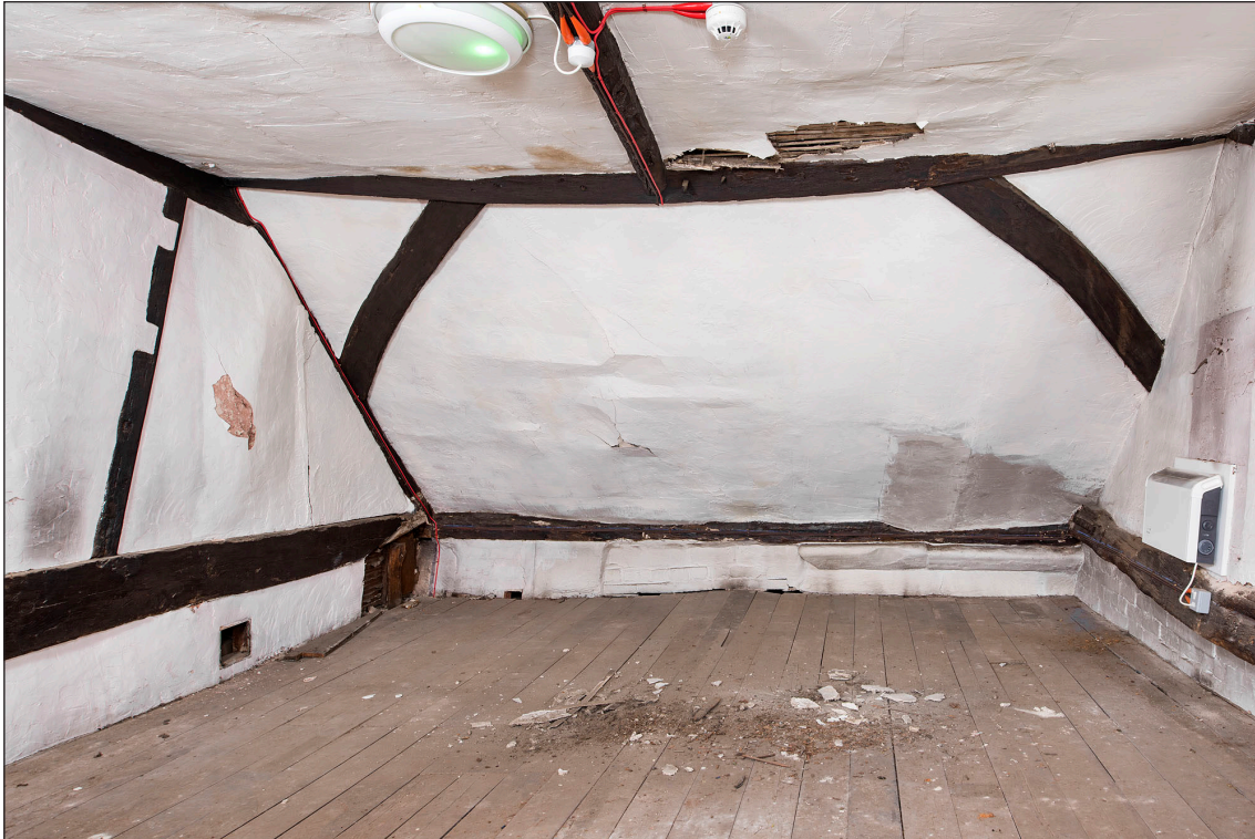
Figure 18 Interior, west elevation, second floor, north room, showing projecting stonework towards the north of the elevation. [DP219893]
