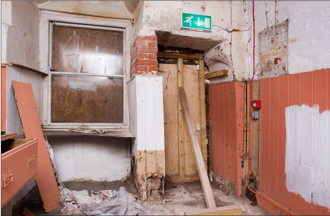
Figure 13 Interior, west elevation, ground floor, south room showing southern doorway arrangement. [DP219913]
