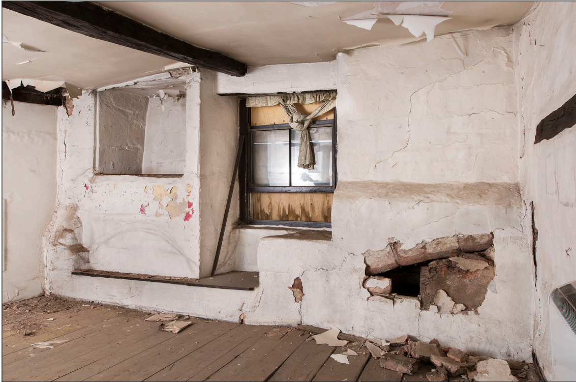
Figure 14 Interior, west elevation, first floor, south room. Note the remains of the eastern side of the principal arch exposed on the right-hand side of the photograph. [DP219907]
