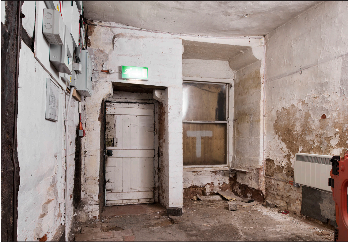
Figure 12 Interior, west elevation, ground floor, north room showing north doorway arrangement. [DP219917]
