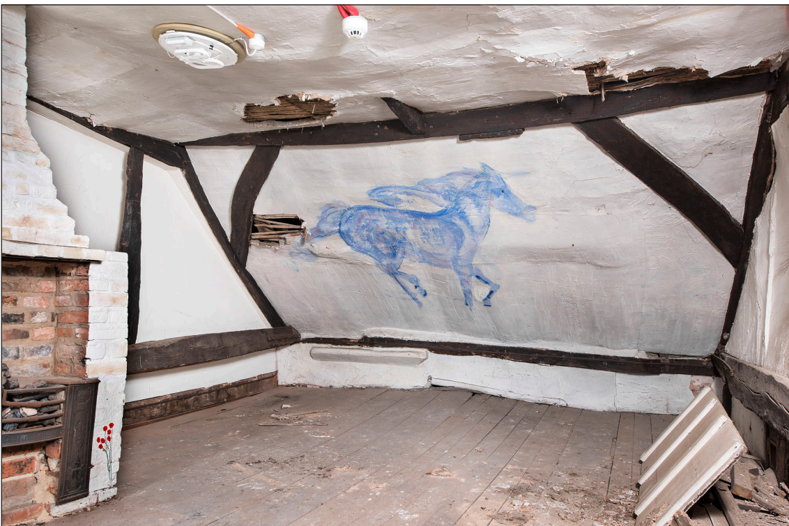
Figure 17 Interior, west elevation, second floor, south room showing projecting stonework towards the southern end of the elevation. [DP219891]
