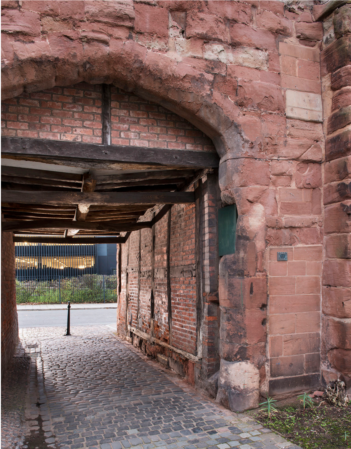
Figure 22 Exterior, east elevation, showing window opening cut through gateway arch jamb and the blocked doorway opening and intermediate window opening above. [DP219942]
