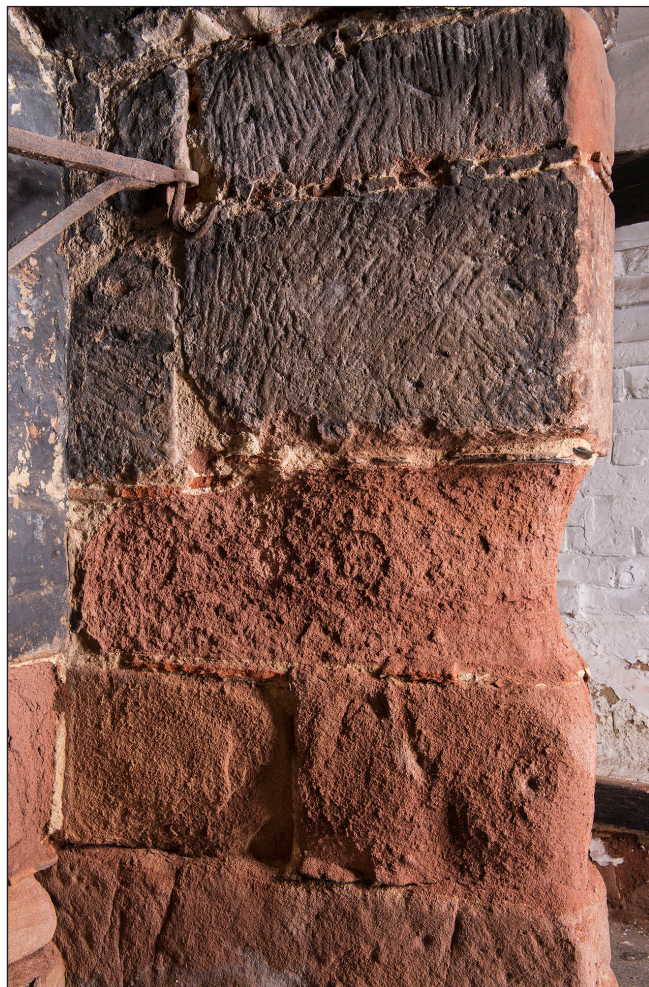
Figure 29 Interior, ground floor, north room, detail of south jamb showing small sections of brick and other ceramic building material used during construction. [DP219922]
