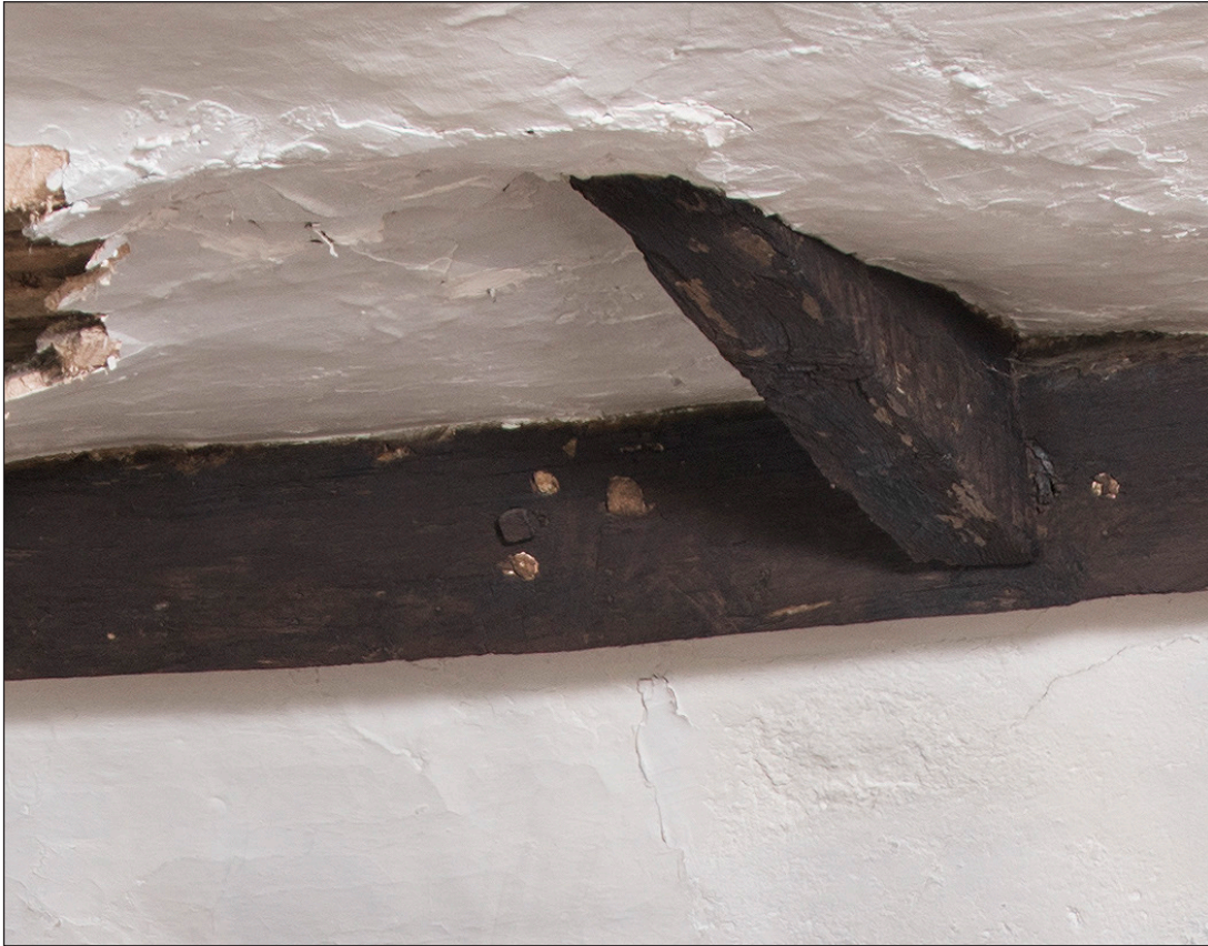
Figure 35 Interior, second floor, detail of purlin on south side, showing redundant peg holes. [DP219891 crop]
