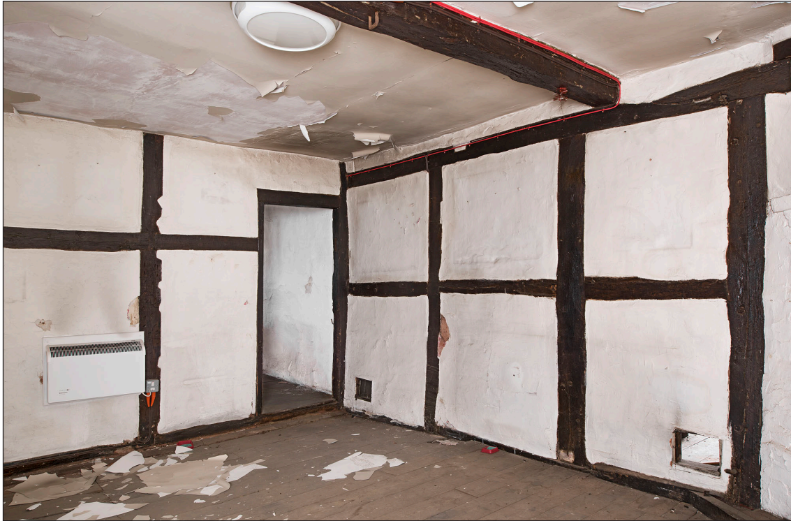
Figure 36 Interior, first floor, south room, showing detail of lateral partition running east to west through the building on the right, with later framing in the left-hand wall. [DP219909]
