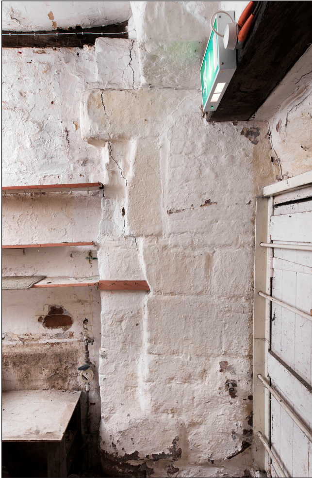
Figure 19 Interior, east elevation, ground floor, south room, showing jamb of doorway and brick blocking. [DP219915]
