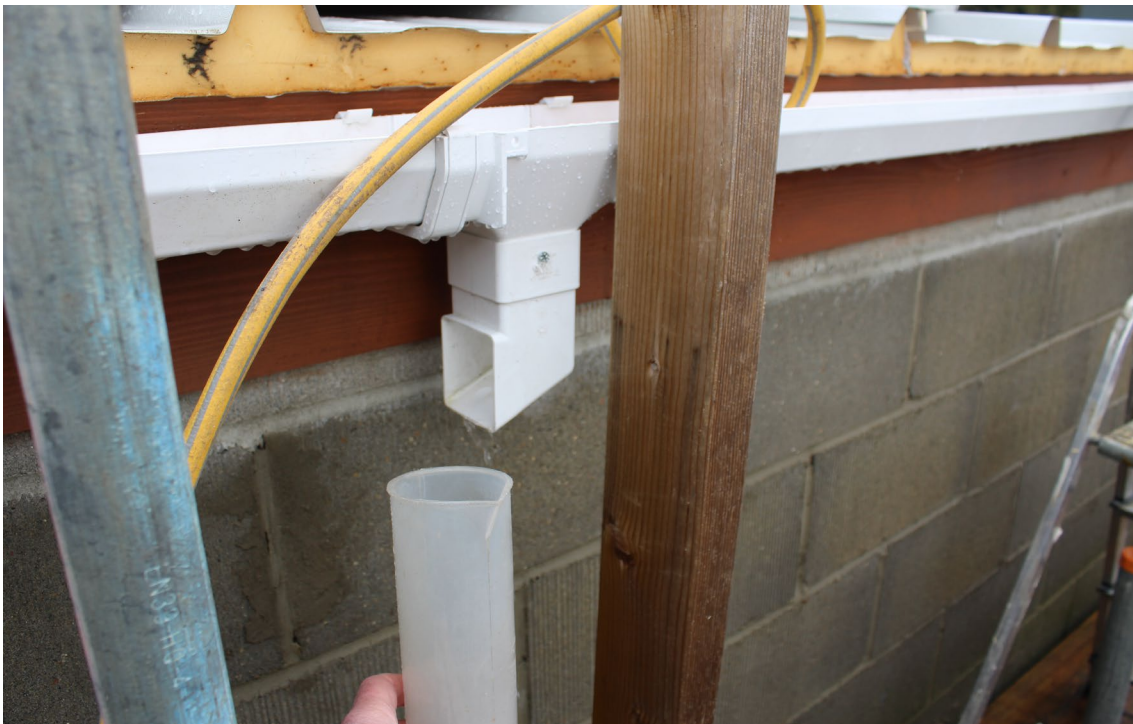
Photo B6: Rate of water flow is checked by collecting water as it drains from test room gutter
