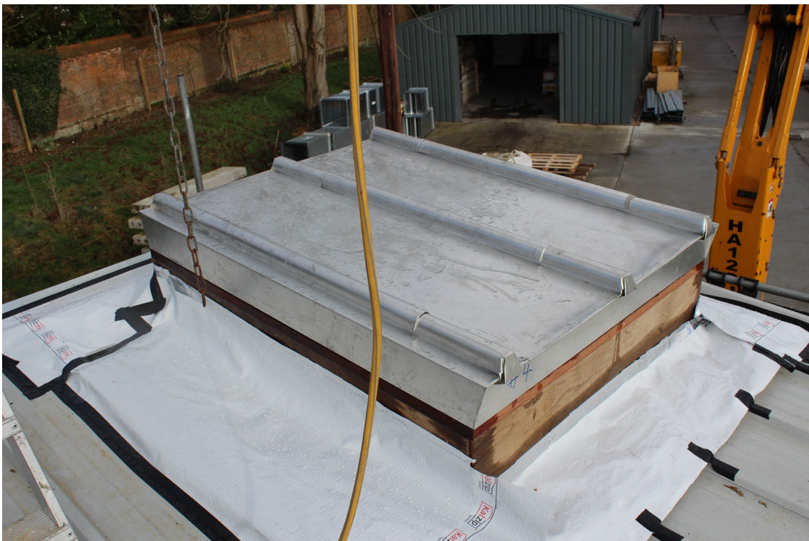
Photo B8: Follow-on roof sample, ready for testing on 19 February 2021
