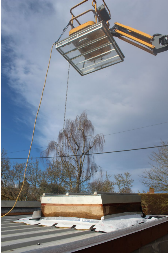
Photo B5: Water tank suspended 3.5m above roof sample, water supplied by hosepipe
