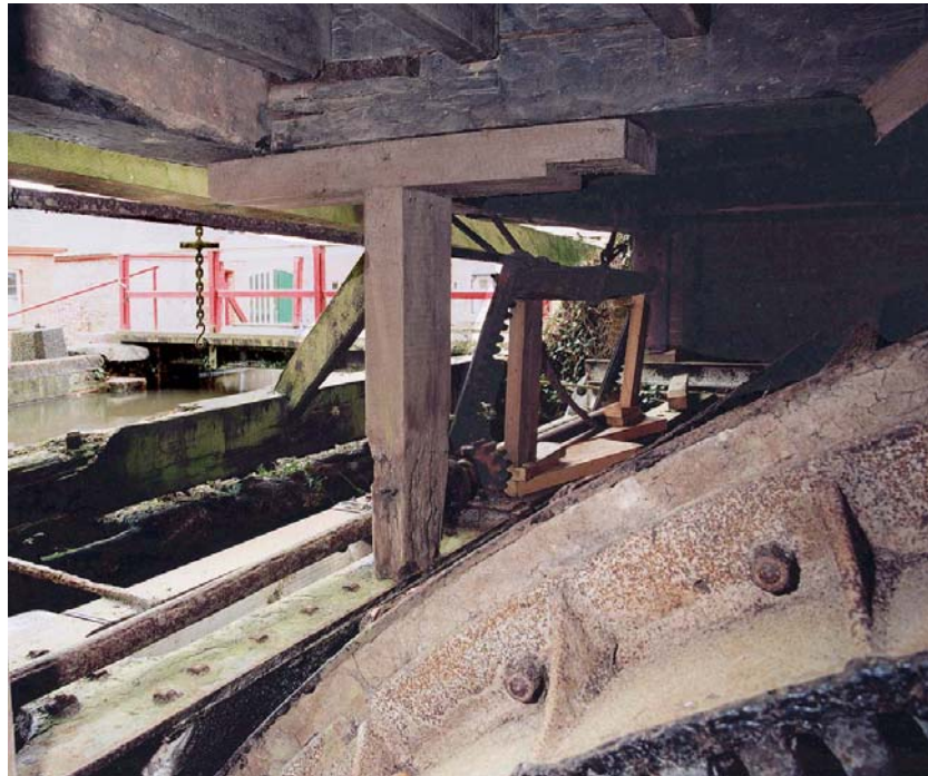
Fig 12. West shroud of the wheel, showing the rack and pinion mechanism of the penstock.
