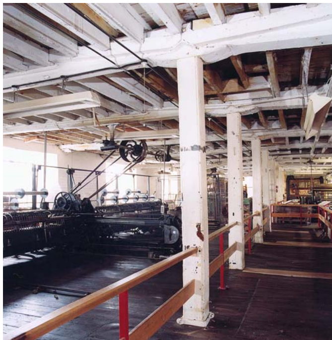
Fig 8. The first floor, showing original timber props and top pads with later reinforcement to beams and joists.
