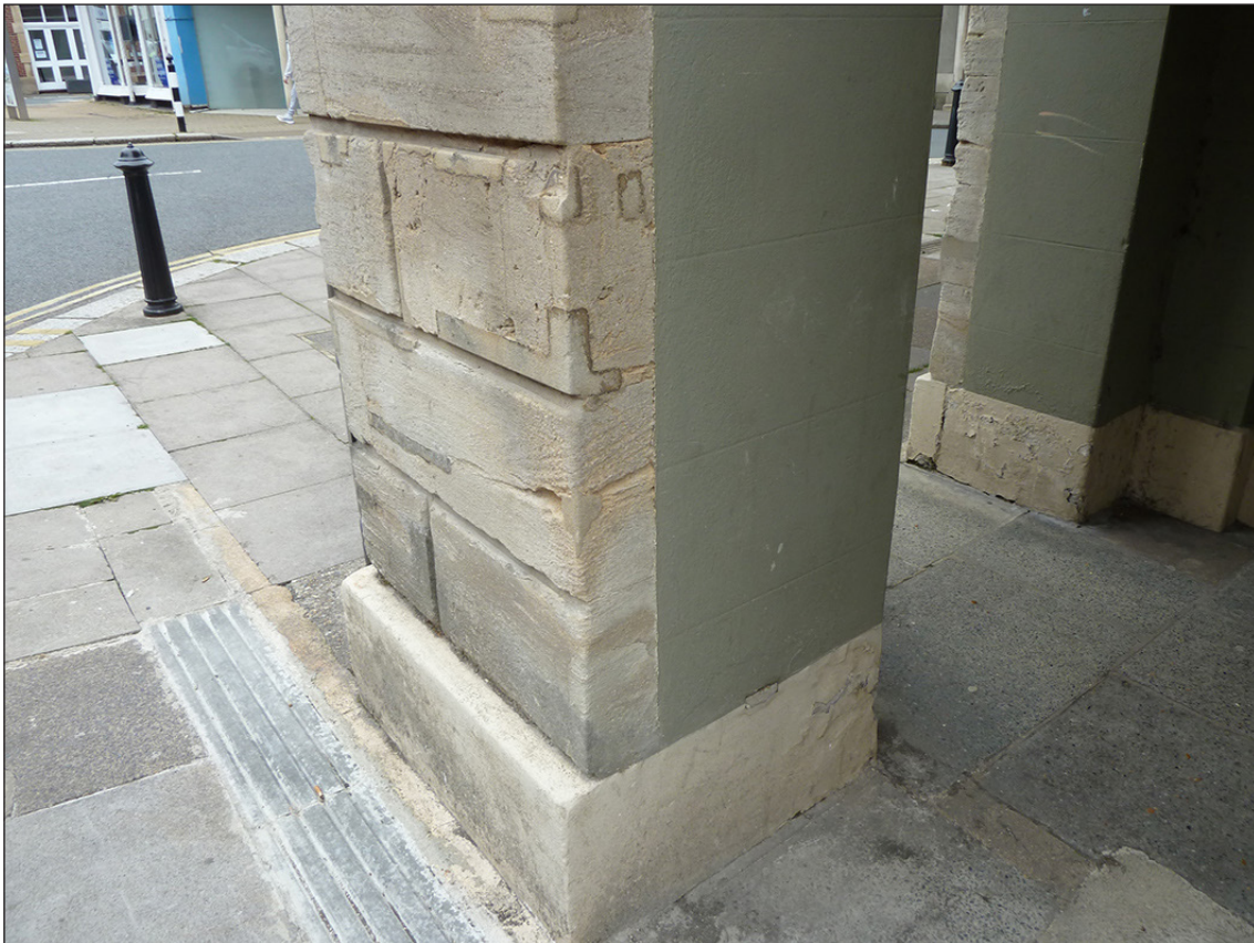
Figure 20: The south-west corner, showing the skin of Bath stone which was applied as part of the 1887-8 clock tower.
