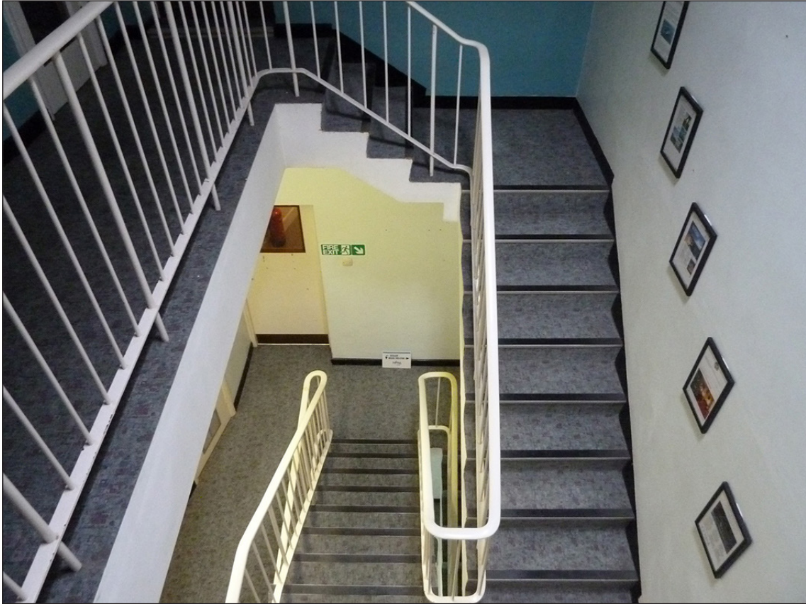
Figure 41: The staircase in the 1960s extension, looking down from the second floor.
