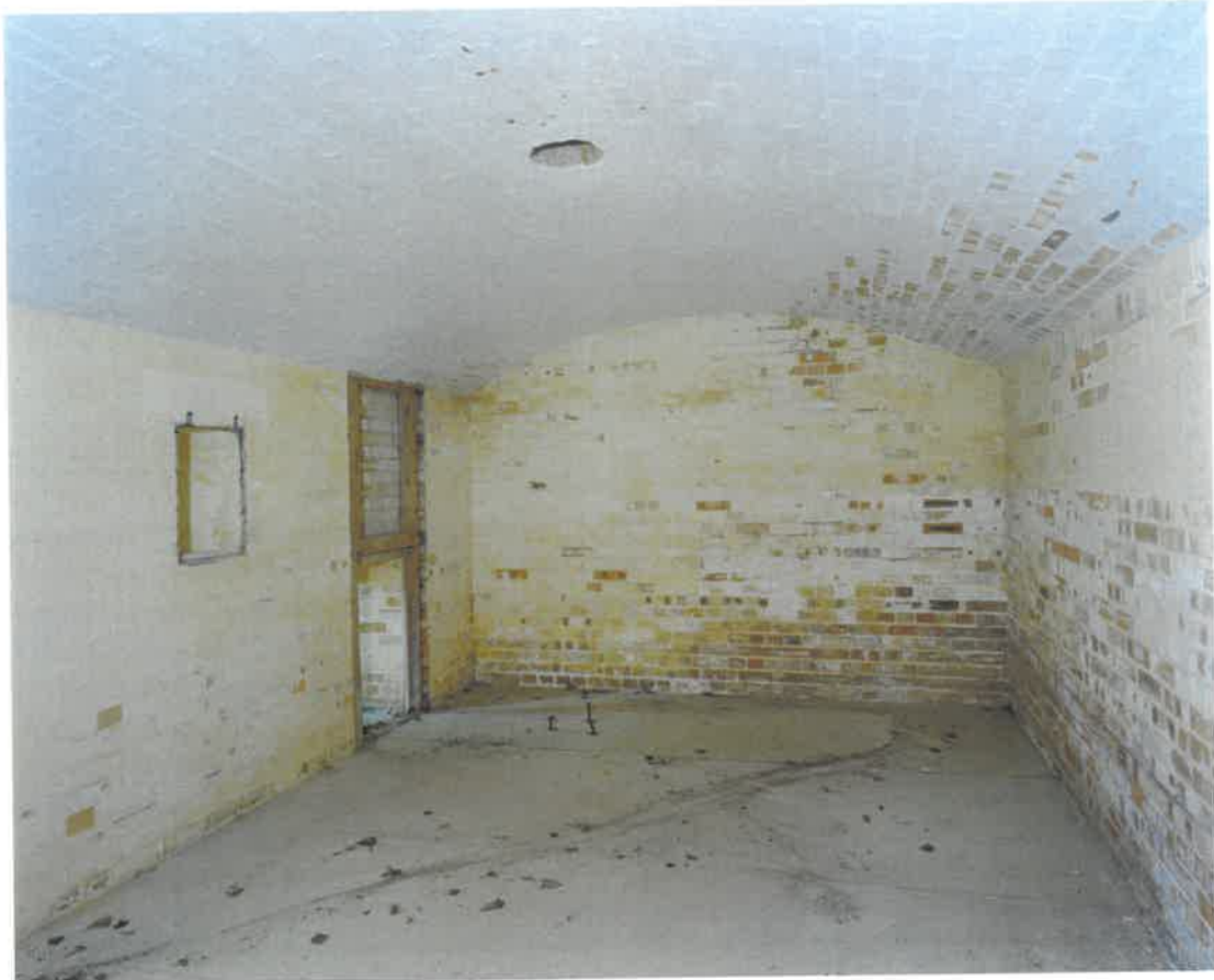
Figure 48 6-inch Magazine: cartridge store 2, showing (at left) a lamp recess and the larger aperture for the issue hatch. A solitary vent pierces the vault (NMR: AA051411)
