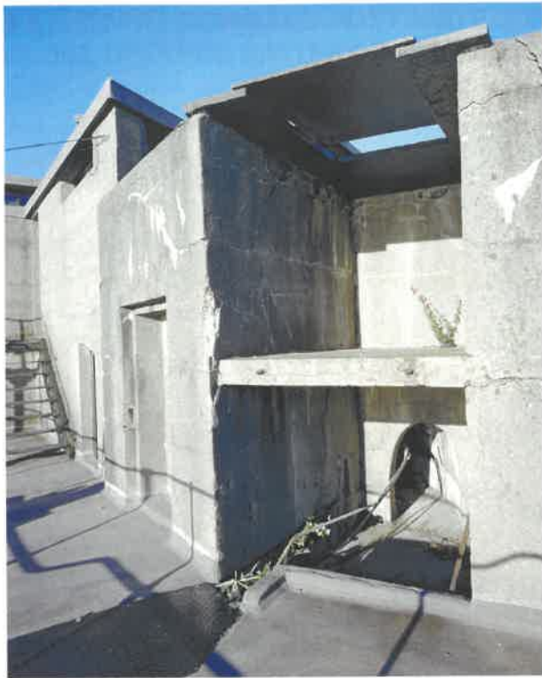
Figure 55 No III gun: recess for the hydraulic accumulator, later converted into a shelter for signallers (see section 3.5); the recess in the angled face just to the left was for battery and dials equipment (NMR: AA051418)
