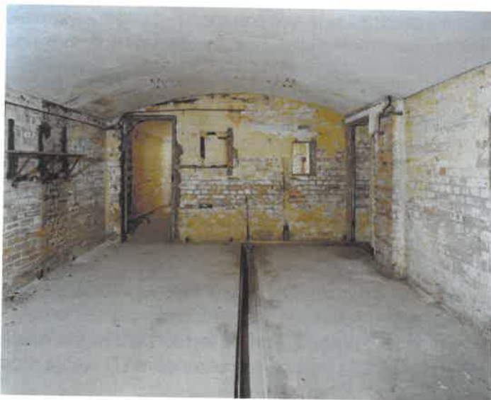
Figure 72 10-inch Magazine: the cartridge store (later Battery Plotting Room) showing the remains of the shifting lobby at the far end: note the scars where the dividing wall has been removed (NMR: AA051415)
