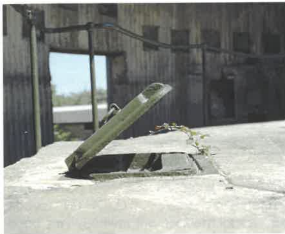
Figure 24 No II gun: the top of the ladder lift on the gun floor (NMR: AA051386)
