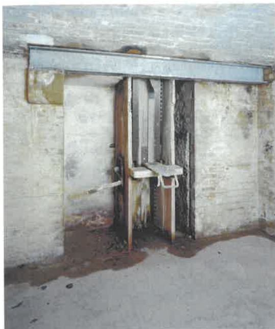
Figure 46 6-inch Magazine: ammunition lifts in shell store 2. The band lift transported cartridges (left), while the ladder lift transported shells (right) (NMR: AA051407/ AA051408)
