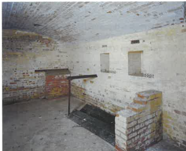
Figure 45 6-inch Magazine: Shell store 2 at the north-eastern end of the magazine complex. The brick and metal piers supported the shelf where shells were stored before being taken to the gun (NMR: AA051410)
