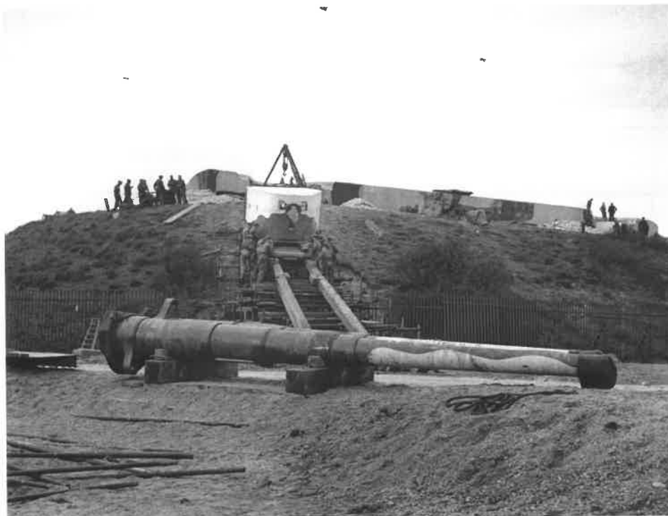
Figure 14 No 1 gun: the 10-ton shield being removed in 1943; note the painted camouflage on the gun barrel and casemates (IWM: H28714; reproduced with the permission of the Imperial War Museum)
