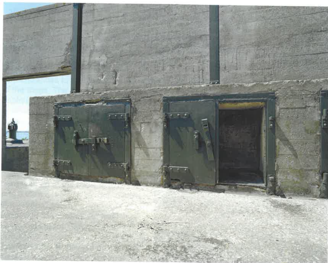
Figure 81 Second World War no 2 gun: ammunition recesses along the rear wall of the gunhouse, many of which still have their heavy metal doors (NMR: AA051398)
