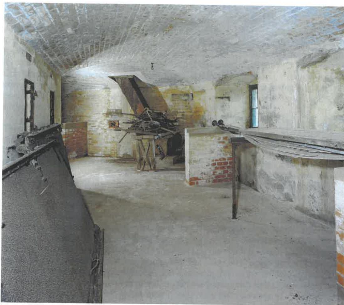
Figure 49 6-inch Magazine: shell store 1, with the remains of a shelf along the right-hand wall and the ladder lift at the far end of the room (NMR: AA051405)
