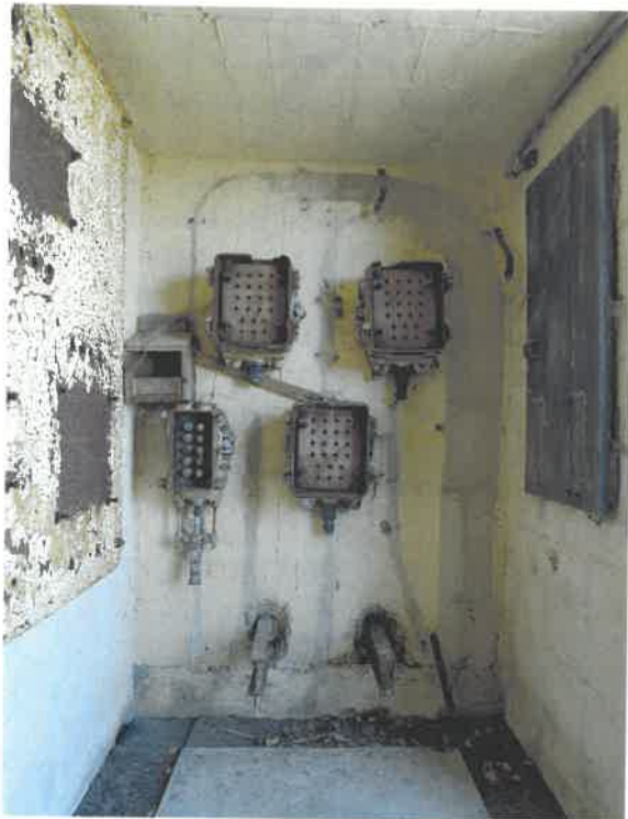
Figure 82 Second World War no 2 gun: the interior of the switch room, showing the electrical equipment (NMR: AA051400)
