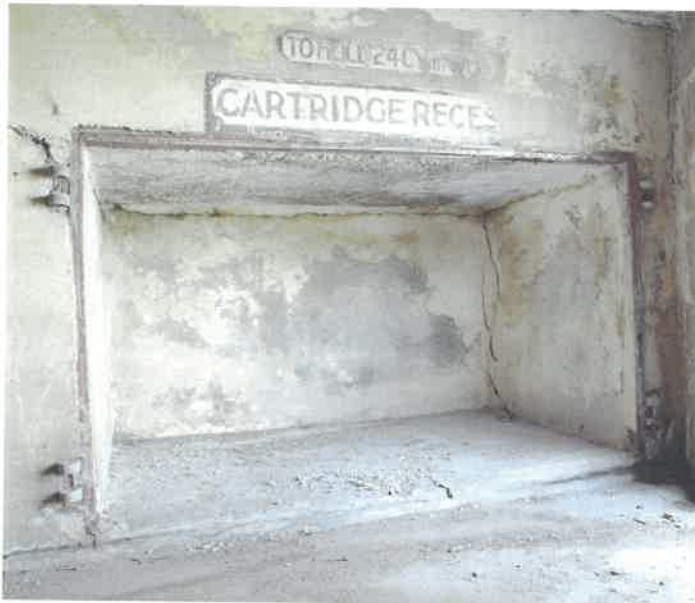
Figure 53 No III gun: recess to hold cartridges for the 10-inch gun. Noth the metal frame and hinges for the heavy metal doors (NMR: AA051414)
