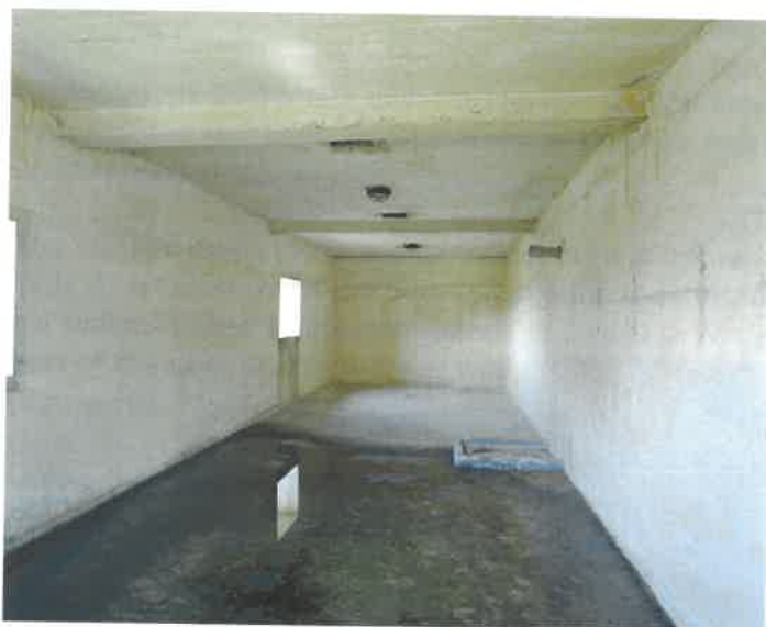
Figure 84 Second World War no 2 gun: the interior of the War Shelter for the crew; there were shelves along the right-hand wall flanking the stove position (NMR: AA051435)
