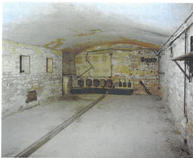
Figure 73 10-inch Magazine: the cartridge store, later Battery Plotting Room, showing the arrangements for electrical cabling at the far end (NMR: AA051416)
