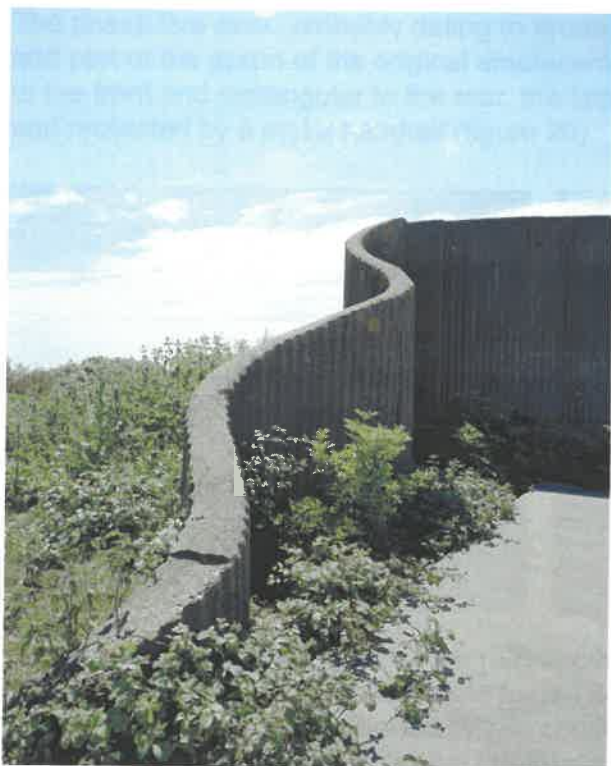
Figure 27 No II gun: the sinuous concrete wall was an attempt to camouflage the otherwise straight lines of the casemate (NMR: AA051443)
