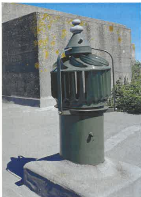
Figure 18 An example of one of the Howarth ventilators which helped to draw damp air through the magazines and other rooms at the rear of the trace (NMR: AA051402)
