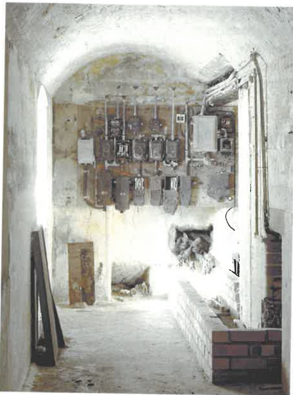
Figure 71 10-inch Magazine: detail of the end of the corridor, showing the array of fuse boxes installed during conversion of the magazine into a battery plotting room in 1943, and the brick channel which guided cables (extract from NMR: AA051440)
