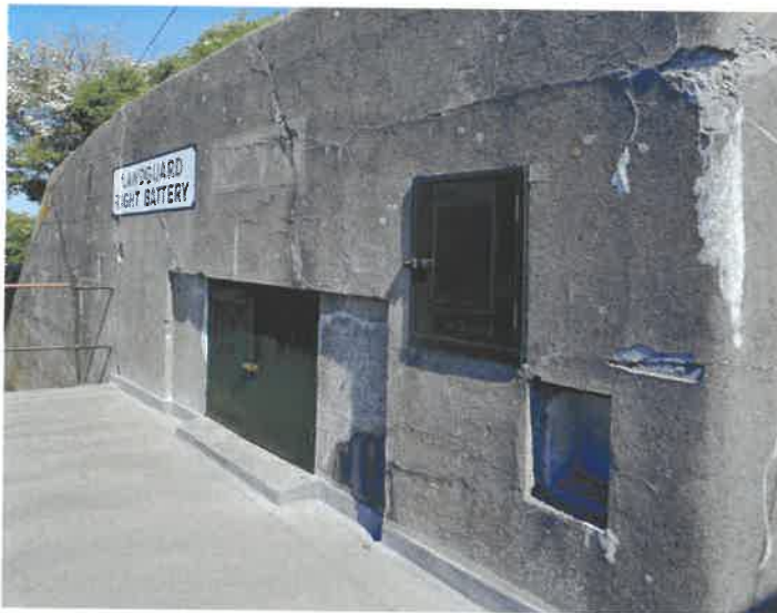
Figure 54 No III gun: the flanking wing wall of the 10-inch emplacement, with openings for (left to right) the ammunition lift and group and fuse stores (NMR: AA051427)
