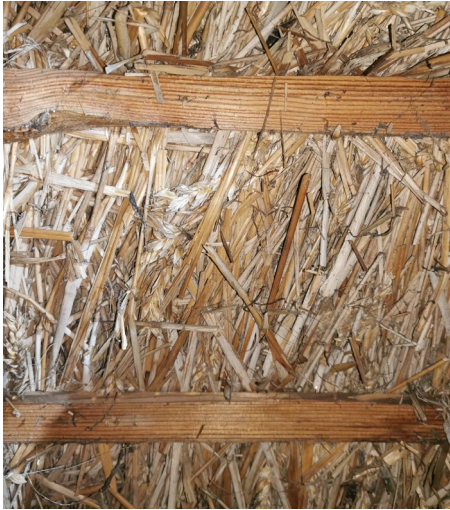
Figure 2 Visible ears of wheat and crushed straw laid in random fashion seen in the phase 1 roof in Room 2.
