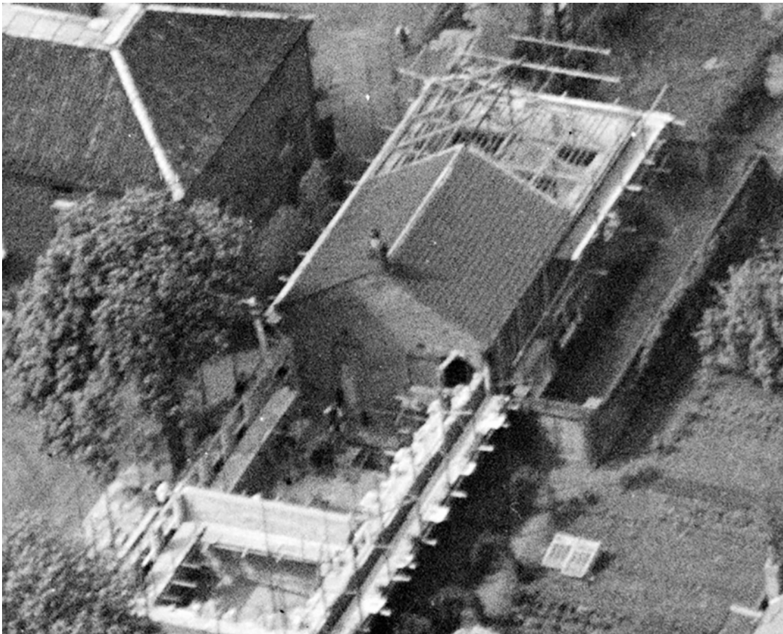
Fig 82: Extensions to a school building, seen from the south-east in 1928. Detail of EPW021290 MAY 1928 © Historic England (Aerofilms Collection).
