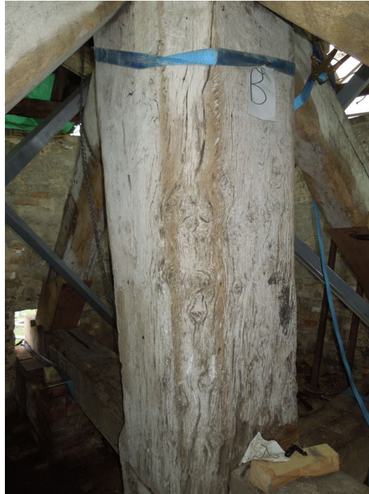
Figure 9: View of the main post below the quarter bars showing the weathered painted surface and knotty nature of the timber (photograph by Martin Bridge)
