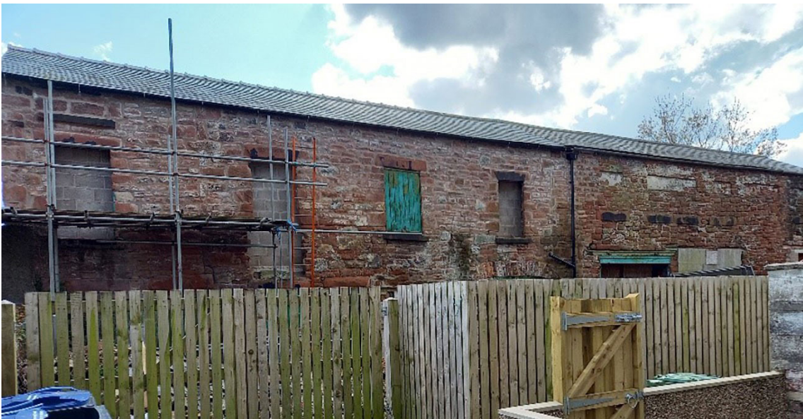
Figure 52: Former range of small houses to the rear of Nos. 61 to 71 Eaglesfield Street (© Historic England, photograph: Fiona Wooler, 2021)
