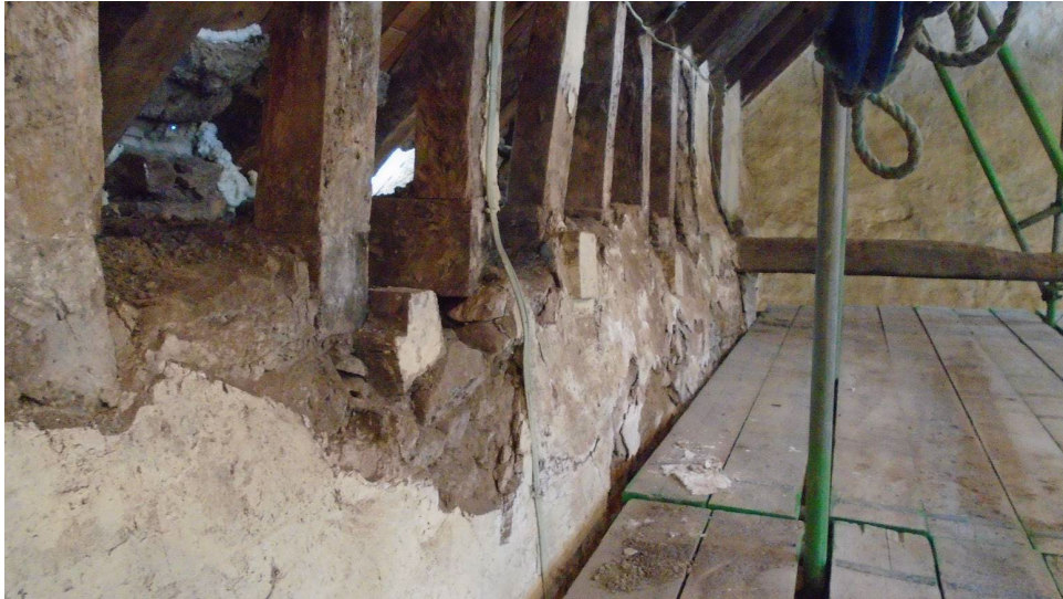
Figure 3: Earlier nave roof from the east, with intact tiebeam in background and the southern end of truncated tiebeams or sole-plates to the left (photograph Alison Arnold)
