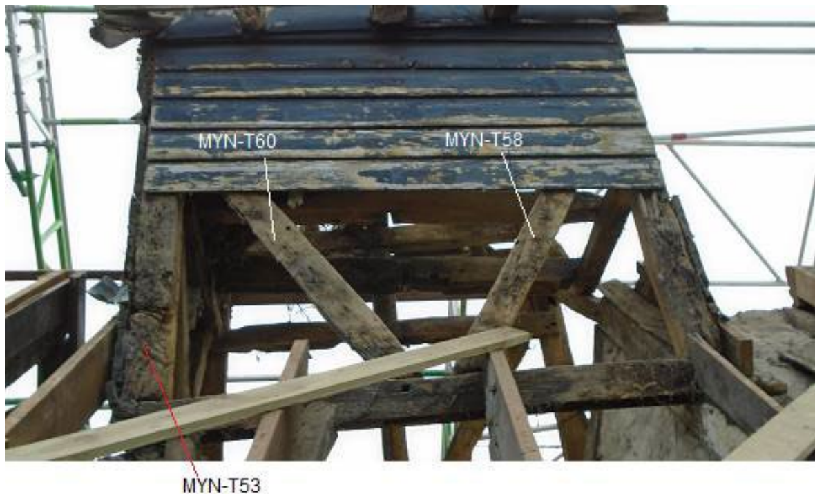
Figure 25: Bell-cote, showing sampled timbers MYN-T53, MYN-T58, and MYN-T60, from the north (photograph Robert Howard)
