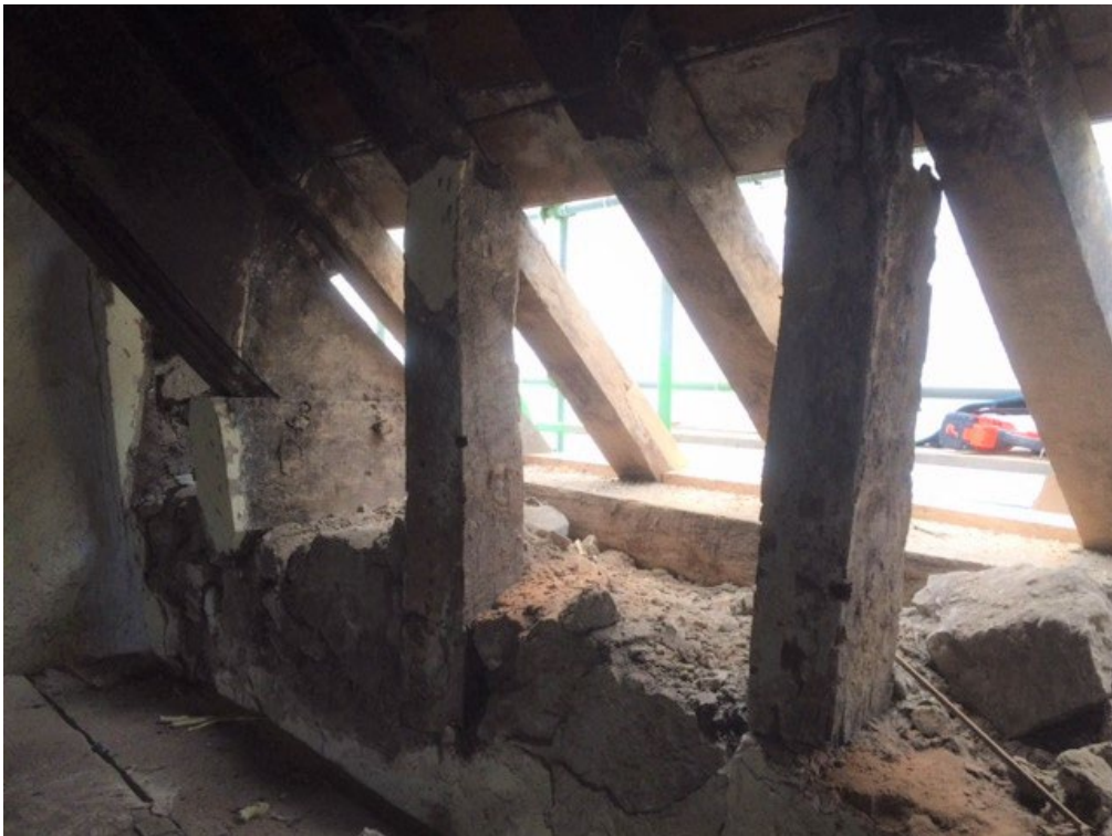
Figure 6: Remnants of an earlier chancel roof, from the north-west (photograph Alison Arnold)
