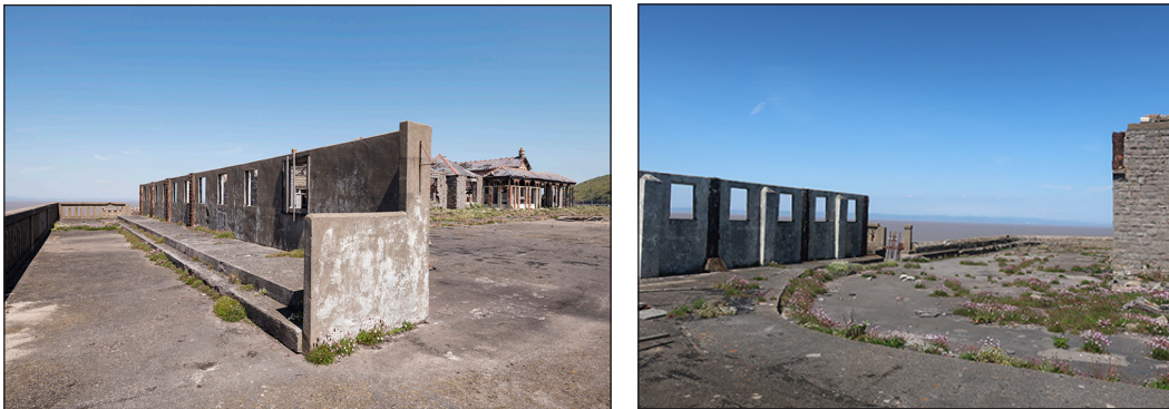
Figure 60: Left: the shelter from the south-west in 2018 [Steven Baker © Historic England Archive, DP218694]; right: the north end from the south-east. [Allan Brodie © Historic England]
