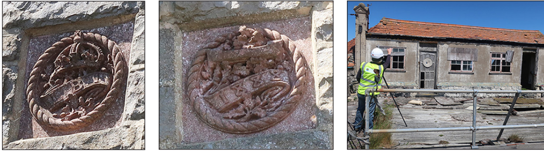
Figure 46: Left and centre: plaques on either side of the oriel on the east elevation in 2018. [Johanna Roethe © Historic England] Right: south elevation in 2018. [Allan Brodie © Historic England]
