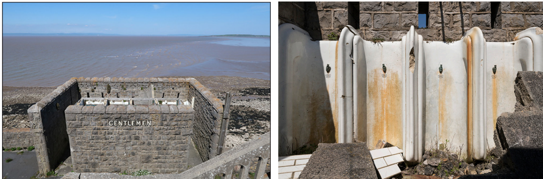
Figure 64: Left: the gents' lavatories in 2018, seen from the viewing deck stair [Johanna Roethe © Historic England]; right: a detail of the urinals, in 2018. [Steven Baker © Historic England Archive, DP218703]
