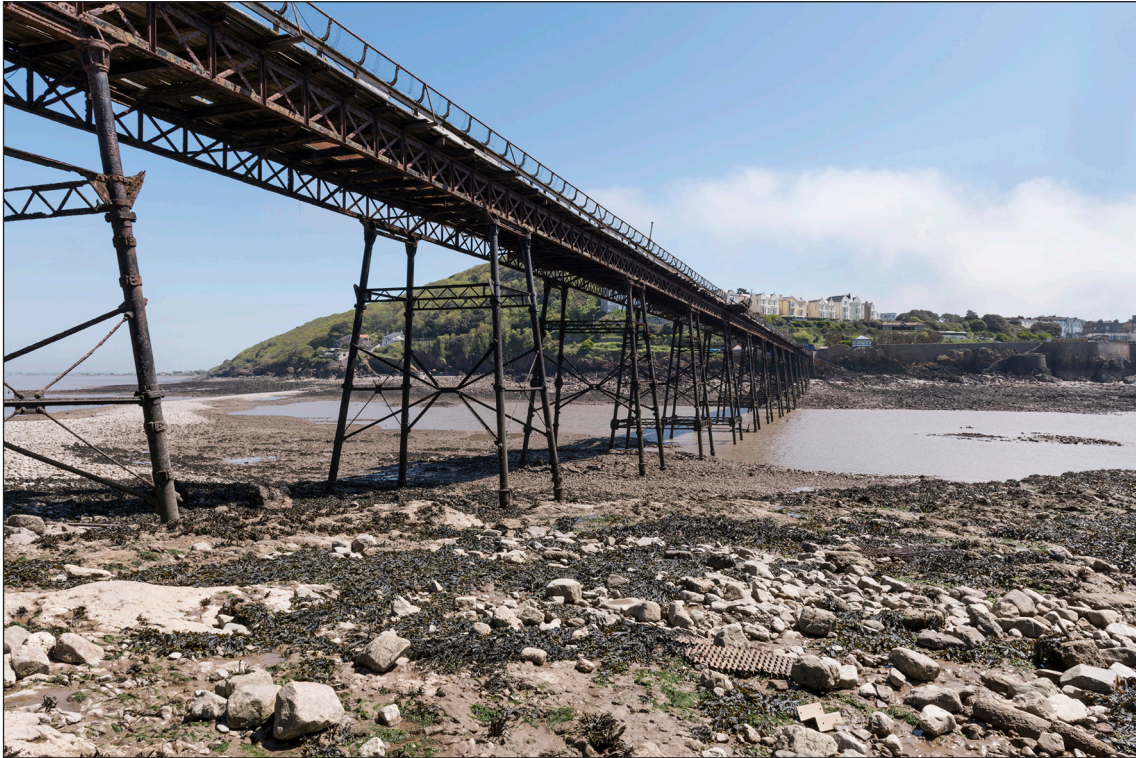
Figure 6: Birnbeck Pier's support structure in 2018, looking eastwards [Steven Baker © Historic England Archive, DP218668]
