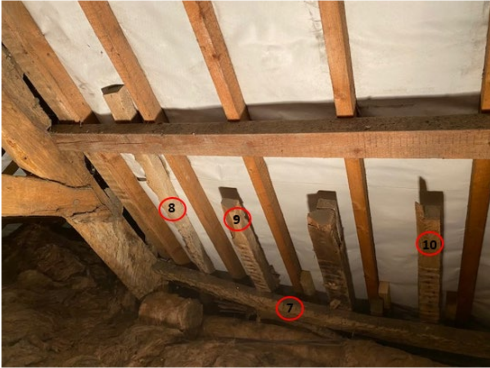
Figure 3c: Roof bay 1 viewed looking north to help identify sampled timbers (photograph Robert Howard)
