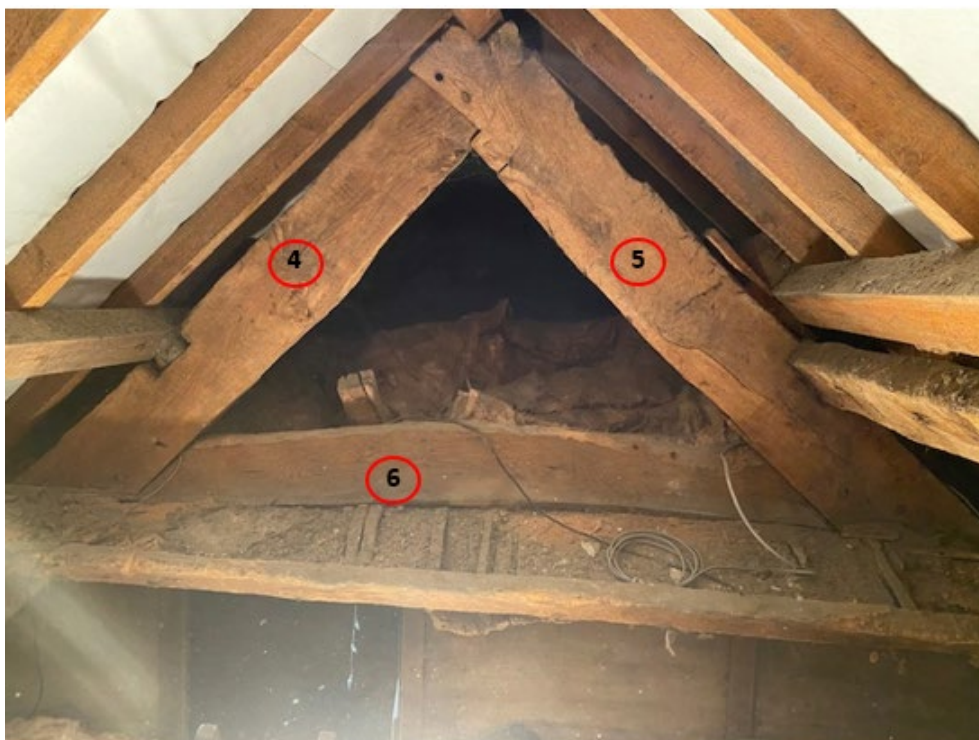
Figure 3b: Roof truss 2 viewed looking east to help identify sampled timbers (photograph Robert Howard)
