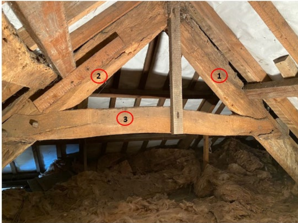
Figure 3a: Roof truss 1 viewed looking west to help identify sampled timbers (photograph Robert Howard)
