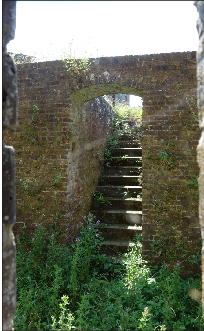
Figure 55 View of sally port opening in counterscarp of redan ditch, with steps to Spur flank [Geraint Franklin © Historic England HE0129/P9]
