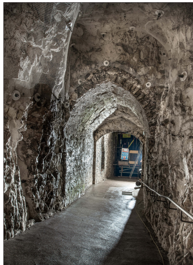
Figure 23 Tunnel immediately south of St John's Tower. Note the junction between the foreground section of tunnel, which has been hewn out of the surrounding rock, and the constructed section beyond. [DP289569]
