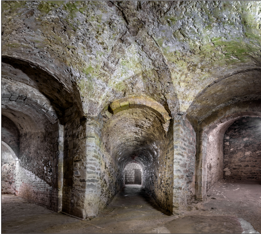
Figure 49 The three tunnels trifurcating from a vaulted central crossing. To the left, the original incline of the north east tunnel can be seen in the wall, underbuilt in later brick. [DP289570]
