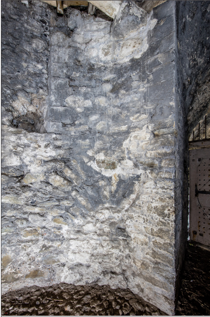
Figure 36 Ground-floor southern reveal of west opening showing change in character of stone. Visible top left is the jamb to a blocked opening. [Courtesy of English Heritage]
