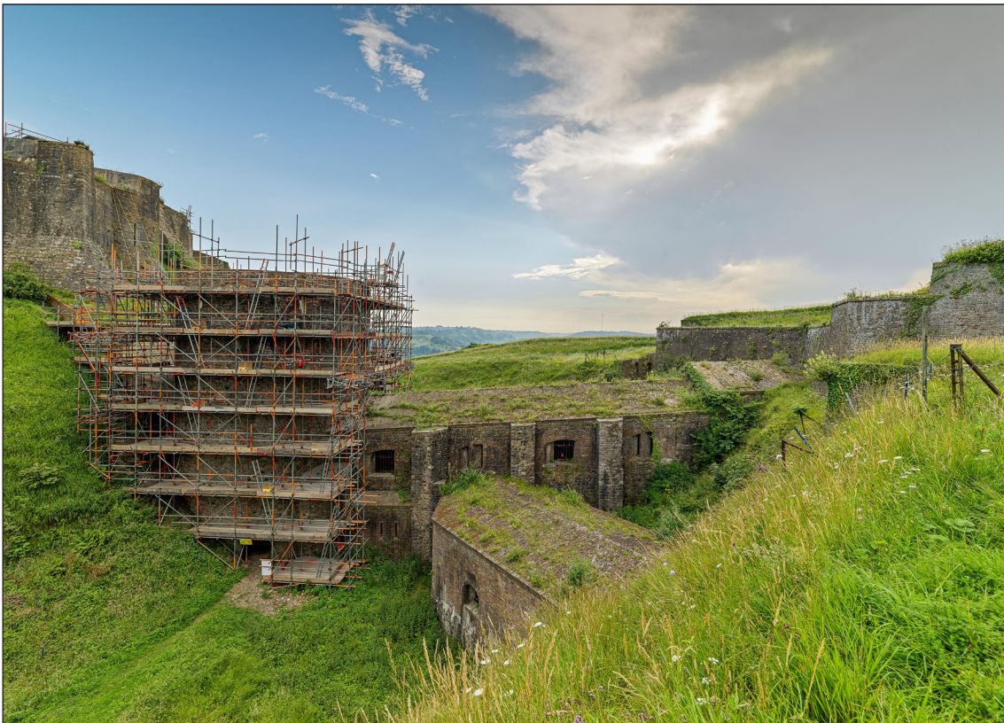
Figure 44 General view of St John's Tower and caponier, taken from the east flank of the Spur during the conservation works of 2021. Note the buttresses to the caponier and the casemated wing caponiers. [DP289564]
