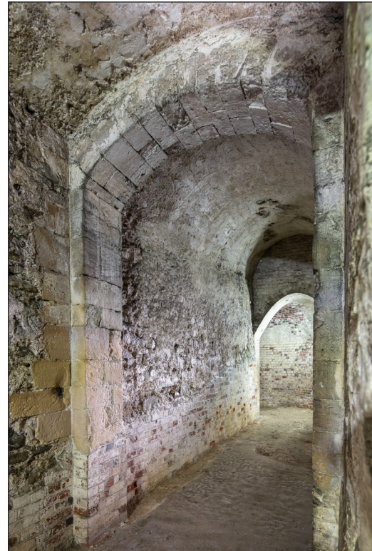
Figure 51 West face of north-west tunnel, retaining evidence for original floor sloping upwards. [DP289572]
