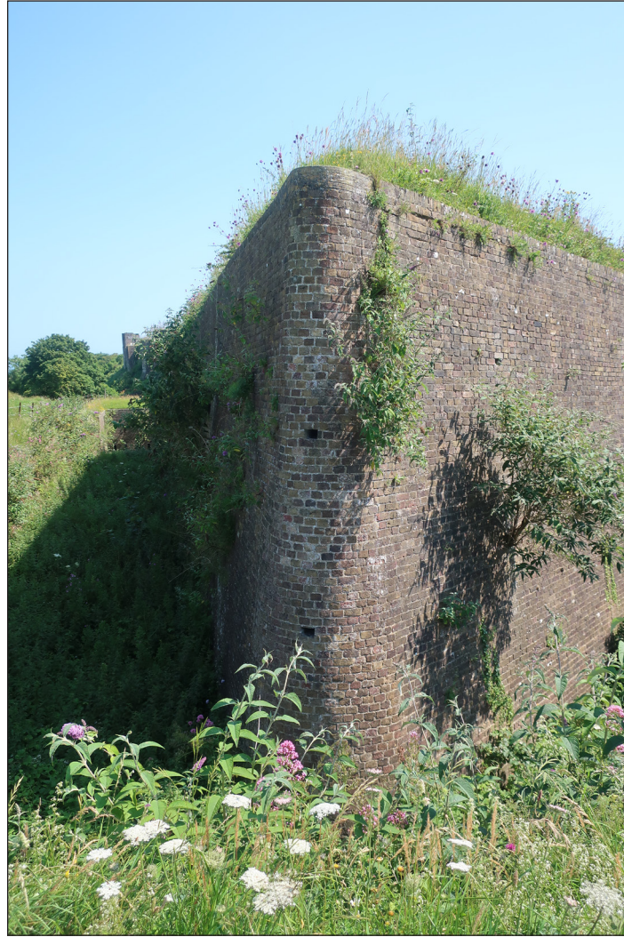
Figure 47 North tip of revetted redan, looking south eaSt [Geraint Franklin © Historic England HE0129/P6]
