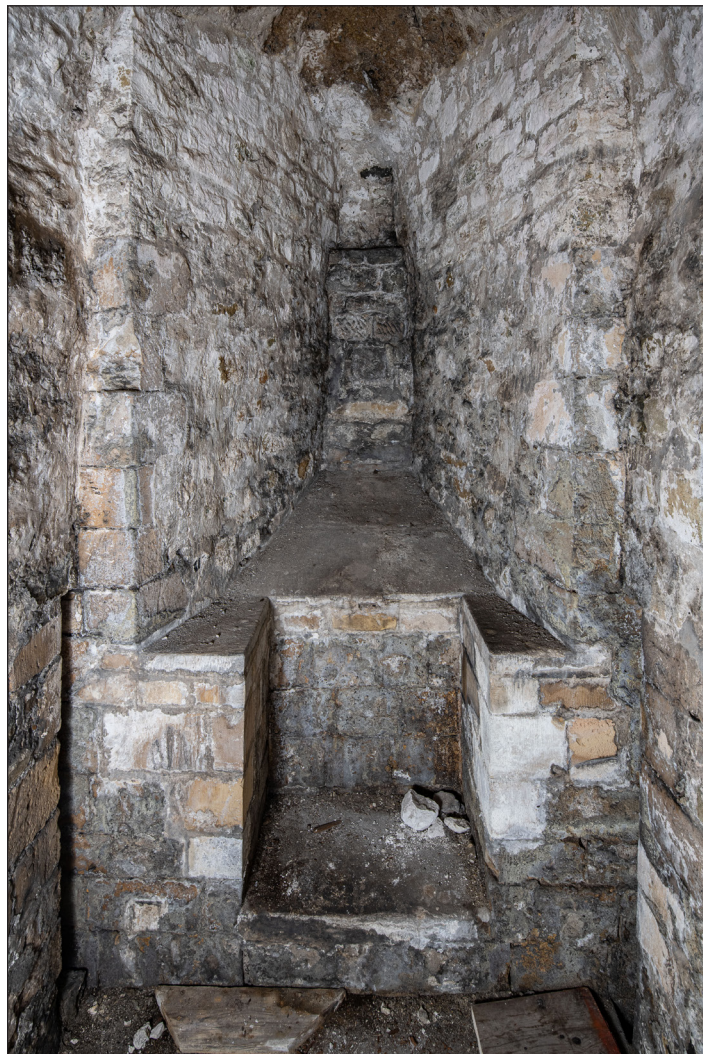
Figure 37 Firing position at second-floor level in north face of St John's Tower [DP289575]
