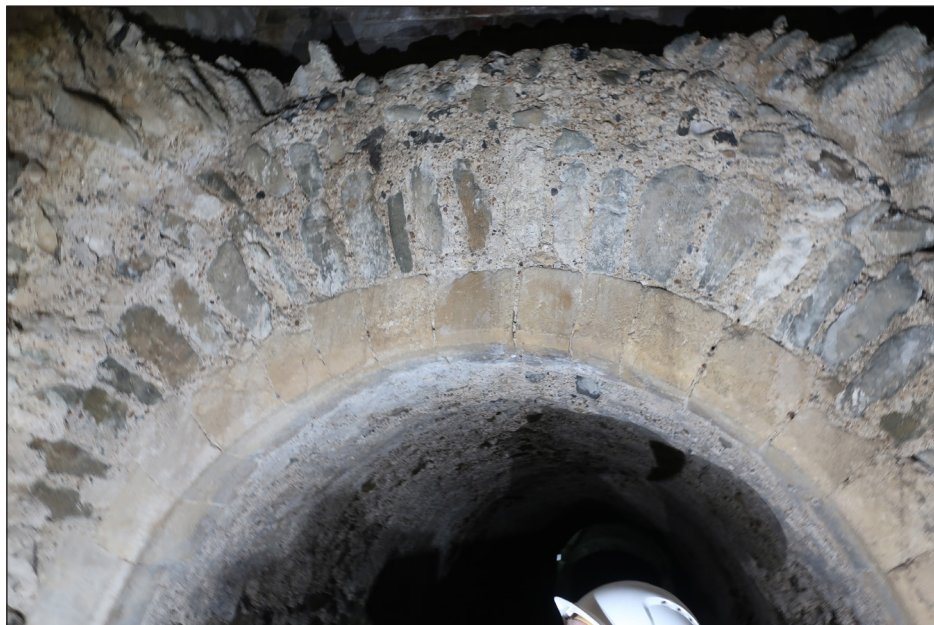
Figure 52 Rubble-walled chamber at end of northern or central branch tunnel. Note chamfered arch to tunnel and scar of barrel vault above. [Geraint Franklin © Historic England HE0129/P8]
