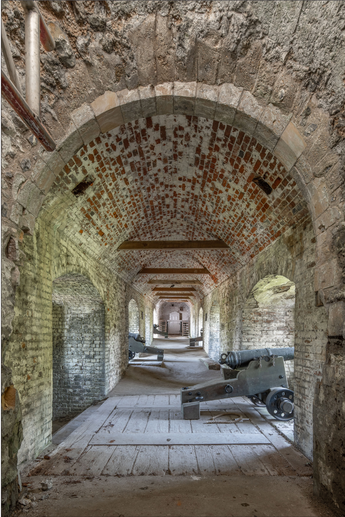
Figure 46 View of upper gallery of the caponier from the north entrance of St John's Tower. Note the plank floor over the former drawbridge pit, modelled floor surface and gun embrasures. [DP289565]
