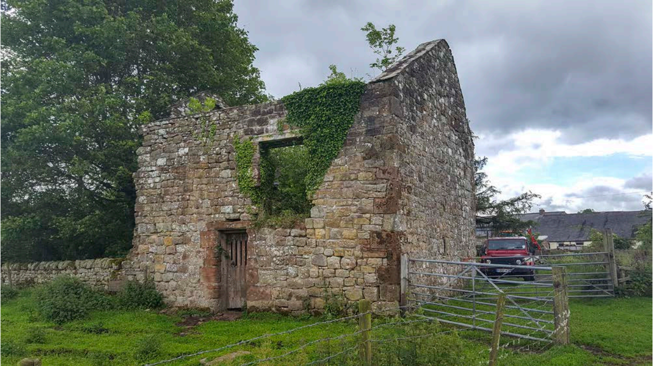
Figure 53: The bastle at Upper Denton is derelict and ruinous. It is the most complete example still standing in the project area. Looking south-east. June 2017 © Historic England.
