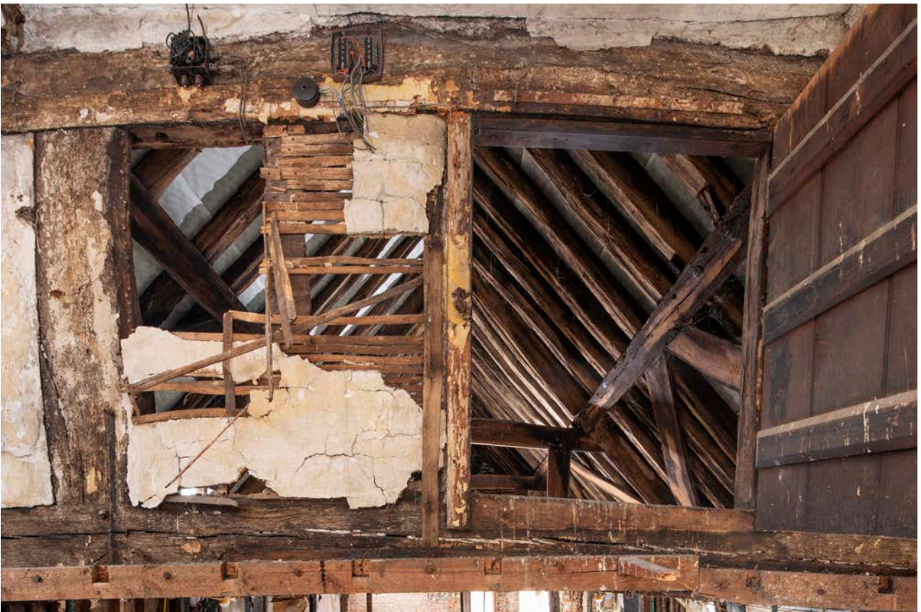
Figure 59: The central part of the truss of frame IV, looking south, showing the original stave positions on the underside of the collar. [James O. Davies © HEA DP435636]
