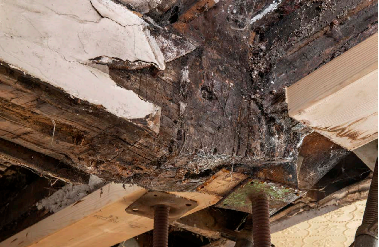
Figure 44: The western post of frame III, cut off below the cross beam, looking south-west. [James O. Davies © HEA DP435643]
