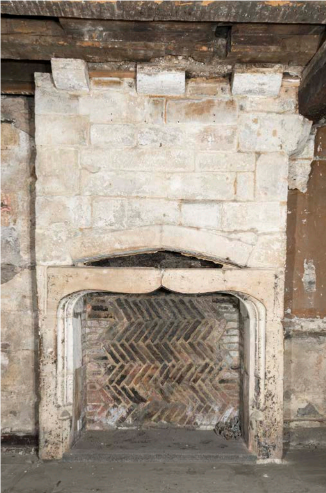
Figure 143: The stone chimney stack and fireplace inserted into the central ground-floor room of the great inn range, possibly also around 1919, looking east. [Steve Baker © HEA DP325623]
