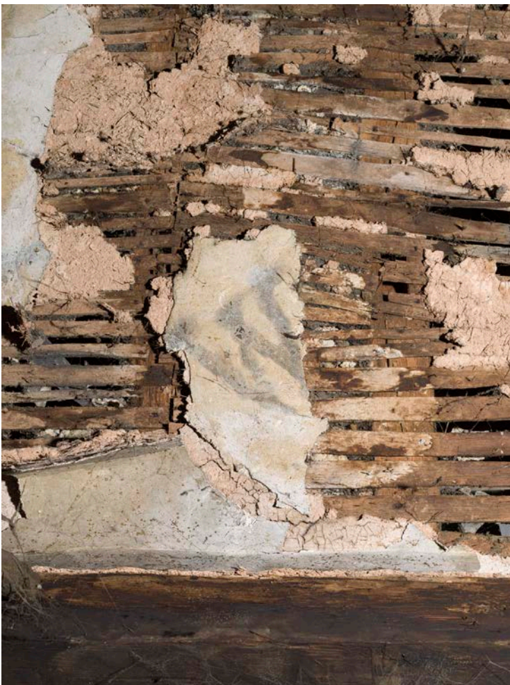
Figure 127: A fragment of the plaster ceiling over the northern first-floor room of the great inn range, showing a possible candle-marked 'W' (or 'M'). [Steve Baker © HEA DP325670]
