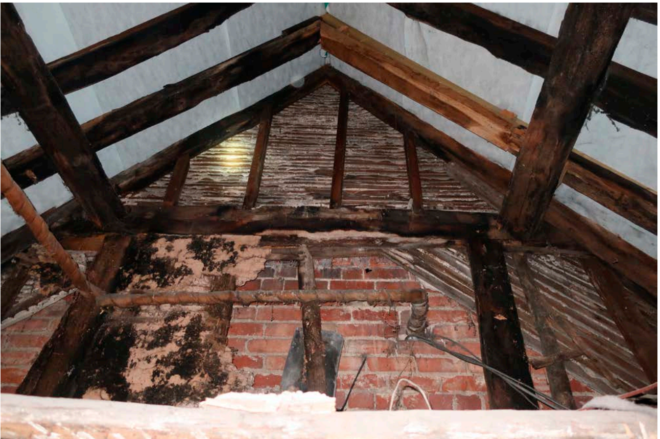
Figure 104: The roof truss of frame IIII, showing smoke blackening, and later stud infill above the collar. [Rebecca Lane © Historic England]
