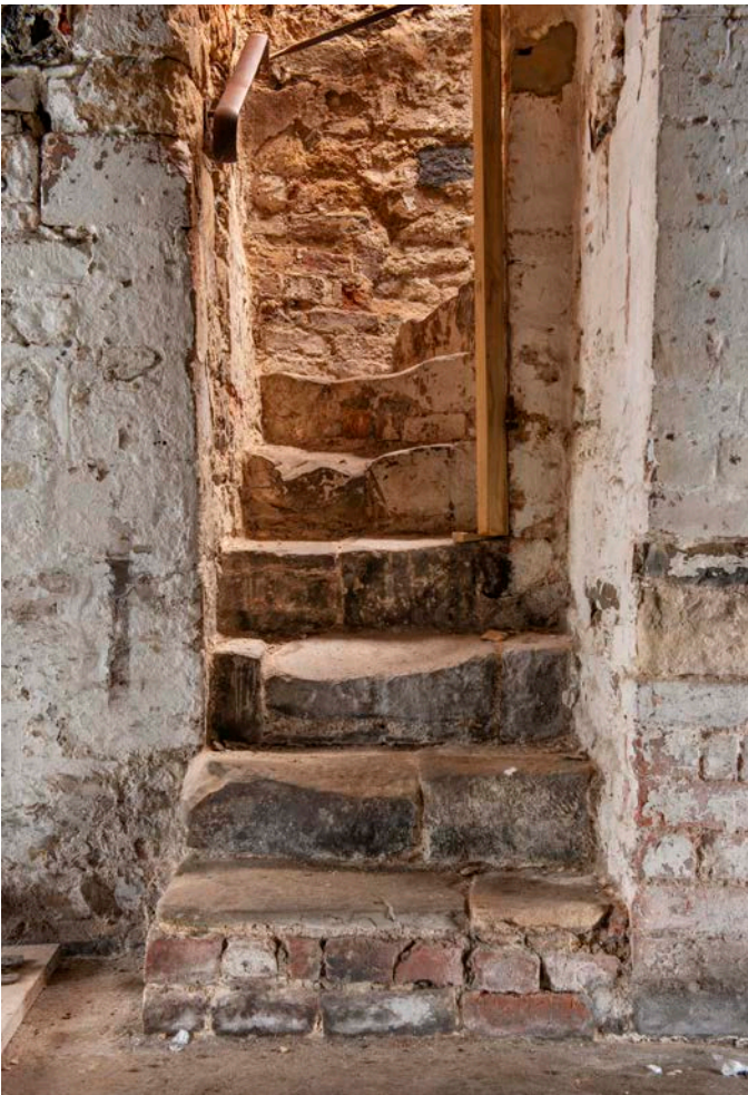
Figure 132: Inserted internal stair from the undercroft to the ground-floor level in the great inn range, looking east. [James O. Davies © HEA DP435619]
