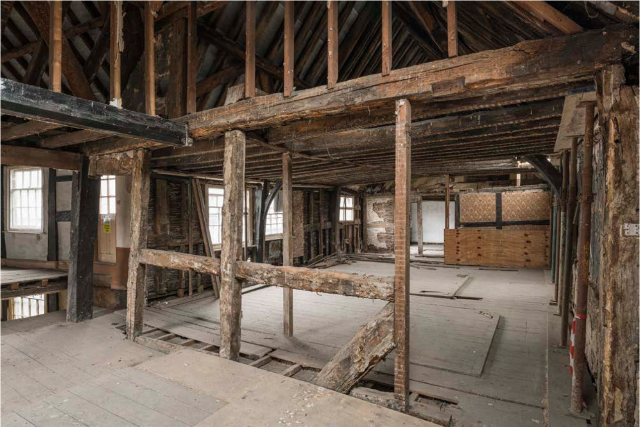
Figure 123: The south bay of the great inn range at first-floor level, looking north-west, showing the earlier partition with the later lap joint adjacent to the inserted doorway at the east end of the partition (the right-hand side of the photograph). [Steve Baker © HEA DP325594]
