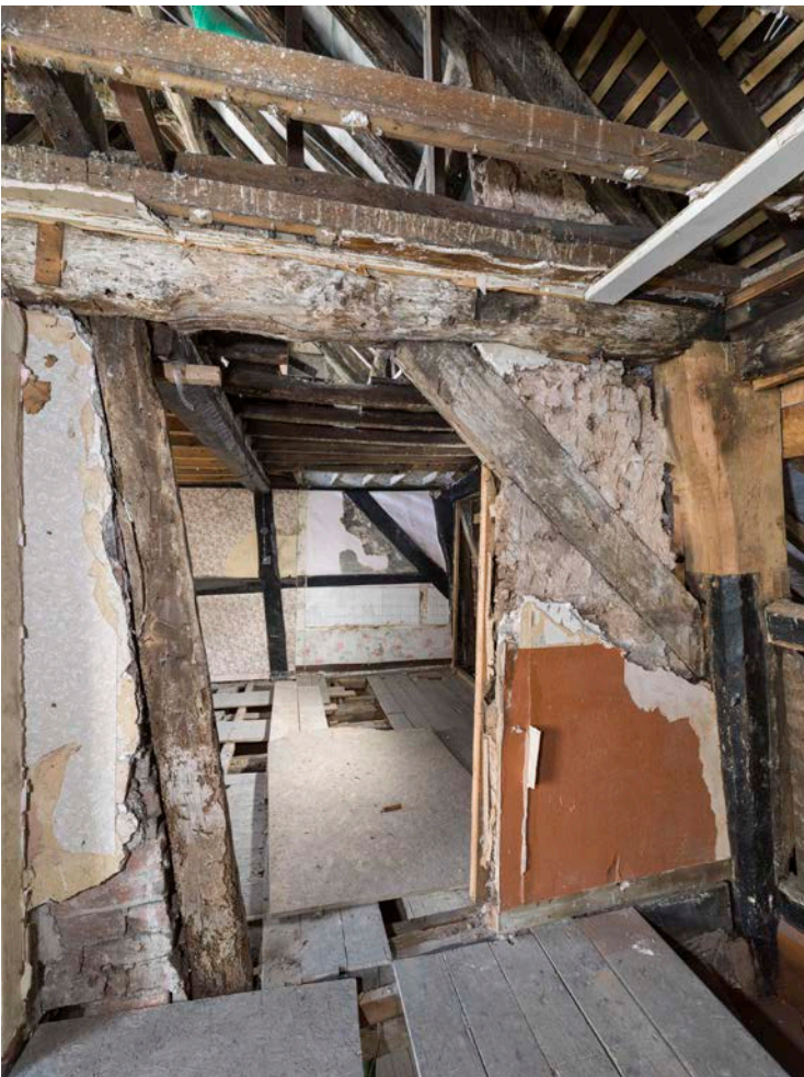
Figure 91: Frames III and V at second-floor level, looking east, showing the pattern of framing in the partitions. [Steve Baker © HEA 325636]
