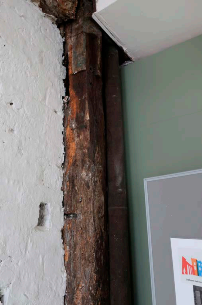
Figure 79: South post of frame V, now visible in the shop at ground-floor level in No. 21 (bay E), looking south-east. [Rebecca Lane © Historic England]
