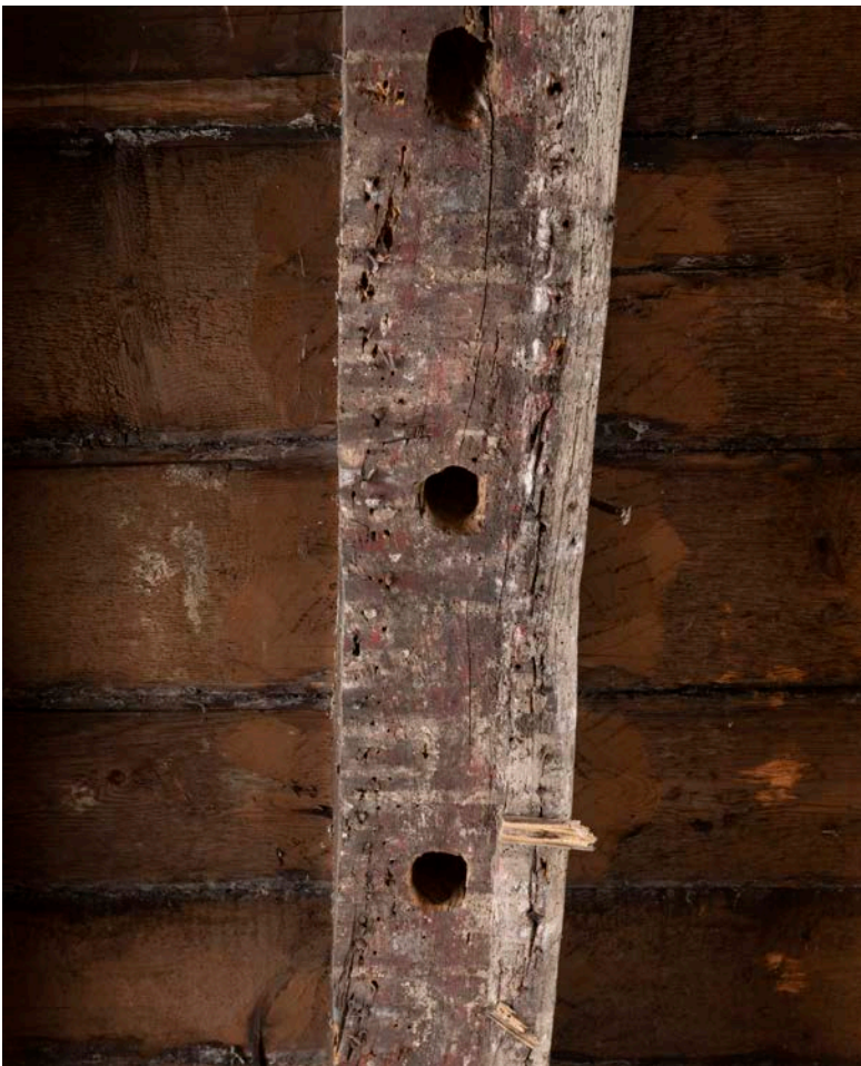
Figure 119: Evidence for an inserted partition in the south bay of the great inn range at ground-floor level, with stave holes inserted into an earlier joist. [James O. Davies © HEA DP435626]
