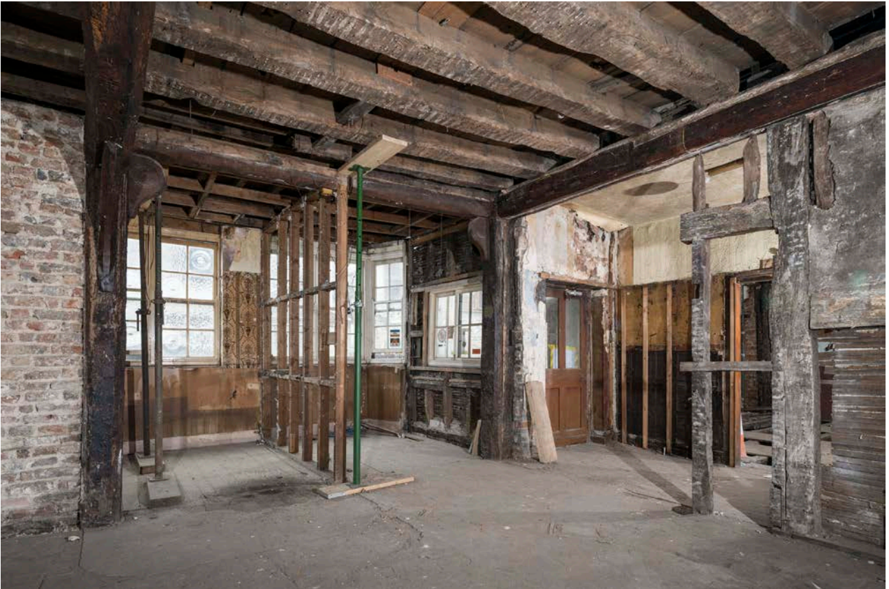
Figure 136: Inserted bay window in the central room at ground-floor level in the great inn range, looking north-west. [Steve Baker © HEA DP325603]
