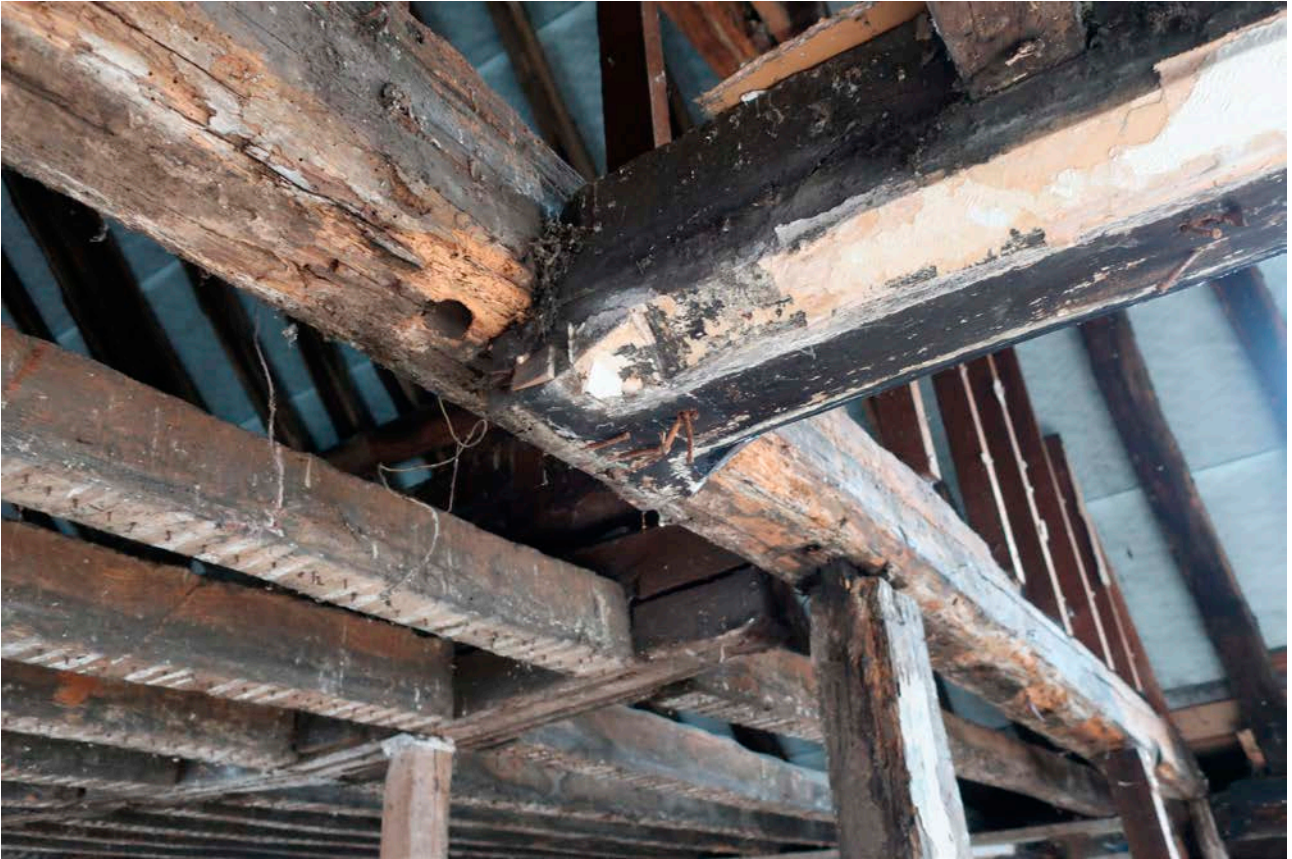
Figure 121: The northern end of the inserted beam in the south bay, looking north-east, showing the bar chamfer stop. [Rebecca Lane © Historic England]
