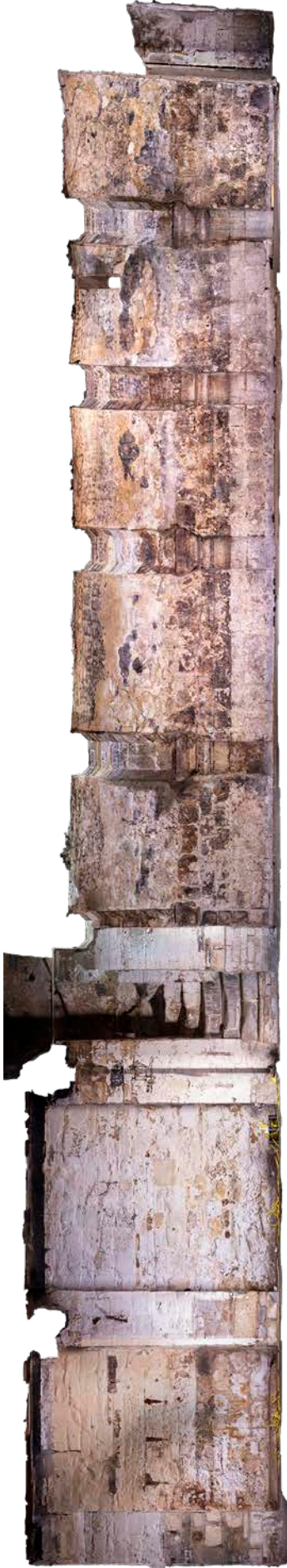
Figure 30: Rectified photograph of the east elevation of the undercroft. [Geospatial Survey © HEA DP364811]
