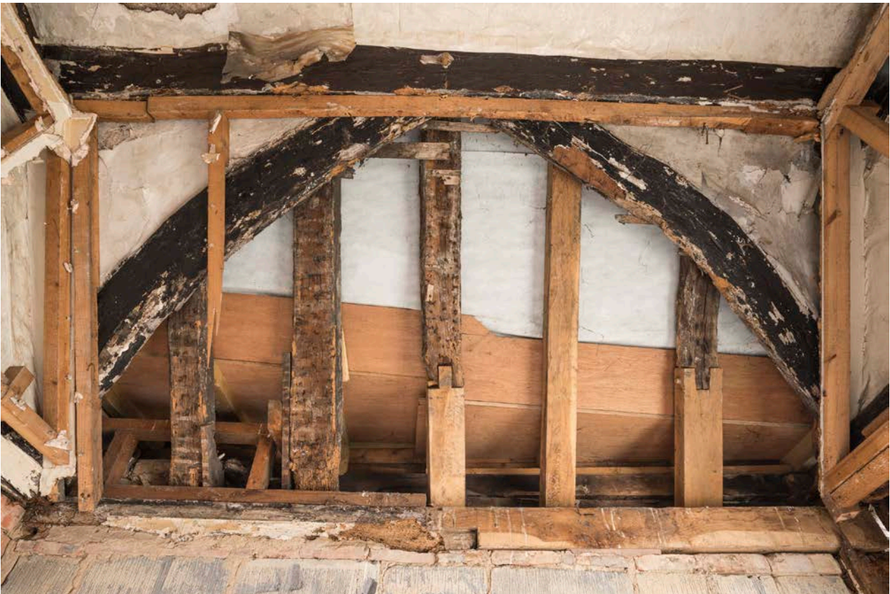
Figure 110: The eastern part of the roof structure of the north-east corner bay, looking east, showing the curved wind braces and original rafters. [Steve Baker © HEA DP325684]
