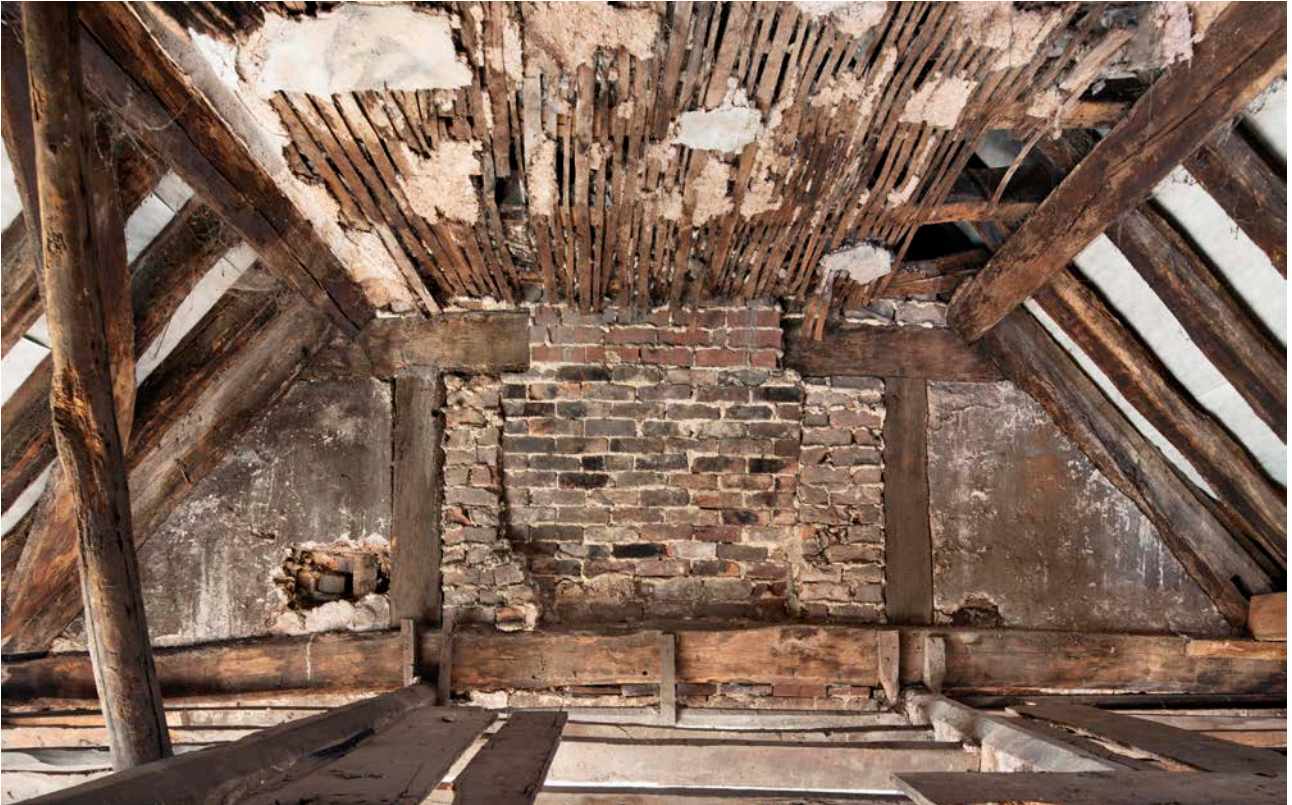
Figure 55: The upper part of frame II, looking north, showing the form of the original timber truss with later brick infill. [James O. Davies © HEA DP435635]
