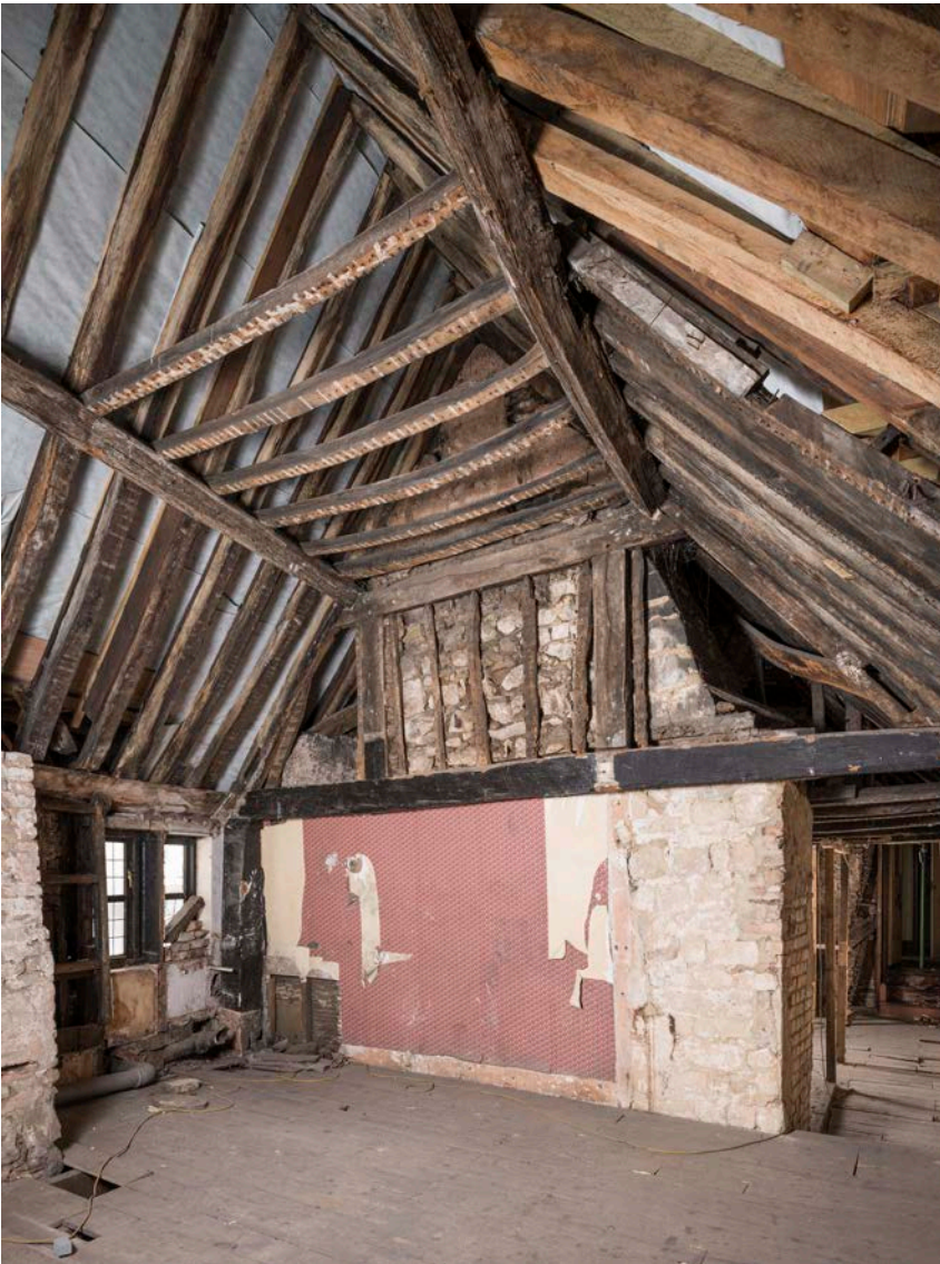
Figure 99: The northern face of frame II of the west range, looking south-east, with the stonework of the inserted chimney sitting against the southern side. [Steve Baker © HEA DP325613]
