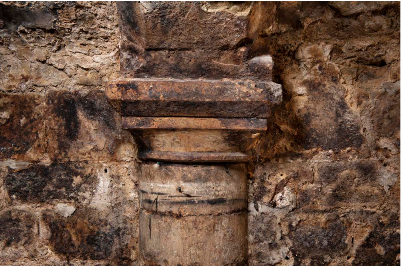
Figure 29: The capital of one of the engaged columns in the undercroft, looking east. [James O.Davies © HEA DP435621]
