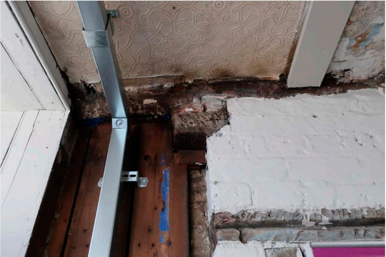
Figure 80: East wall of No. 21 (bay E), looking east, showing the cut off jetty plate adjacent to frame V. [Rebecca Lane © Historic England]
