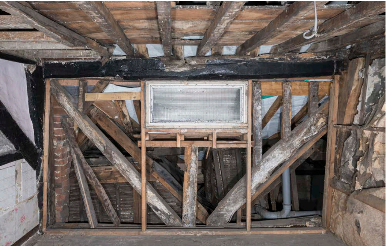
Figure 93: South elevation of bay D (No. 19A) at second-floor level showing the original timber framing, looking south, including curved brace to the west (right-hand) side and later inserted straight brace on the east (left-hand) side. [Steve Baker © HEA DP325641]
