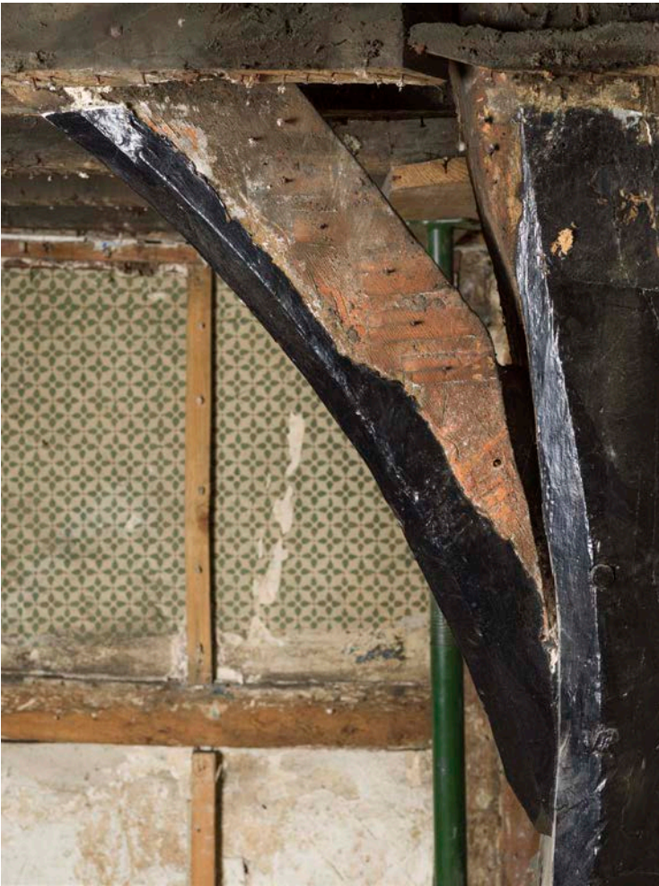
Figure 57: The up-brace and western post of frame III, looking south, showing surviving fragments of a red paint. [Steve Baker © HEA DP325669]
