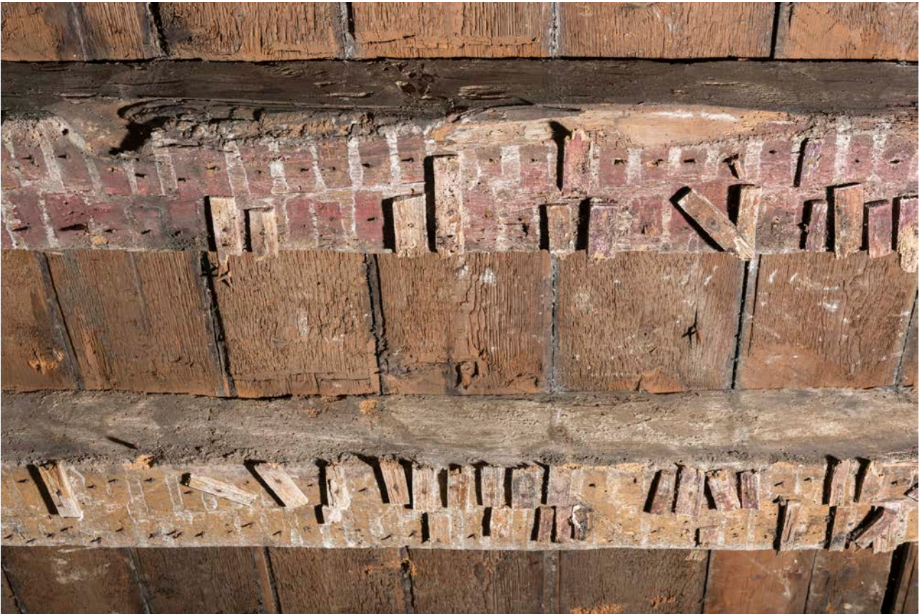
Figure 112: The ground-floor southern bay (bay F) of the great inn range, showing the possible use of alternating red and yellow paint on the ceiling joists. [Steve Baker © HEA DP325692]
