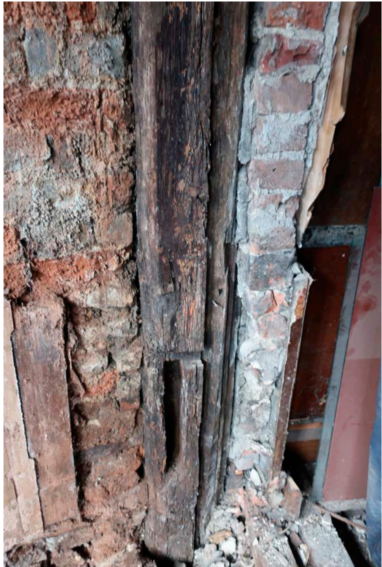
Figure 43: Lower part of the west post of frame II showing the mortice and slot which indicate the base of the oriel window, looking north. [Rebecca Lane © Historic England]
