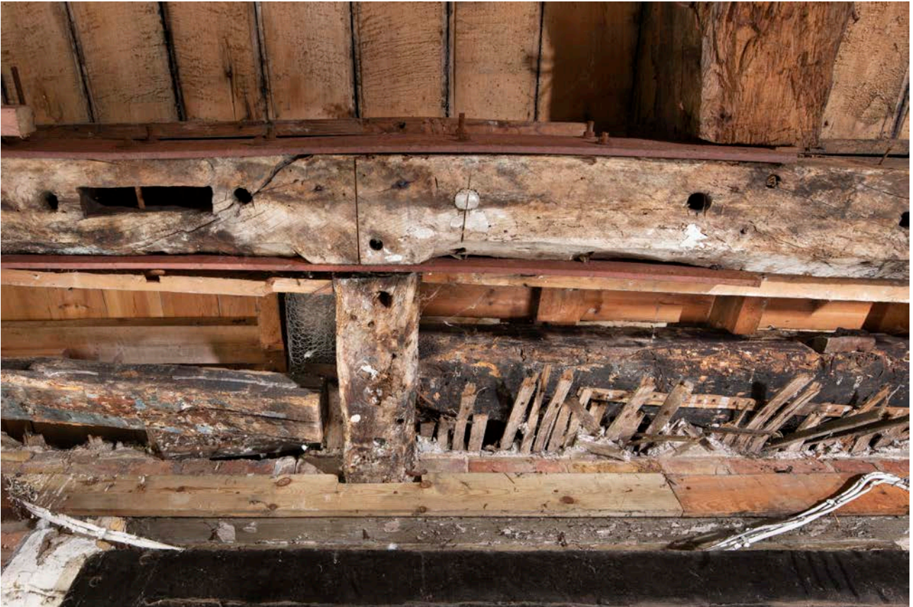
Figure 78: The underside of the central part of the cross beam of frame III, now visible in the passageway through the street-front range, showing the empty mortices for the original partition. [James O. Davies © HEA DP435637]
