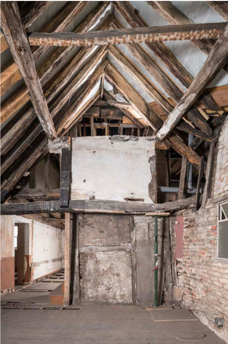
Figure 97: The southern side of frame I of the west range, looking north-west. [Steve Baker © HEA DP325611]
