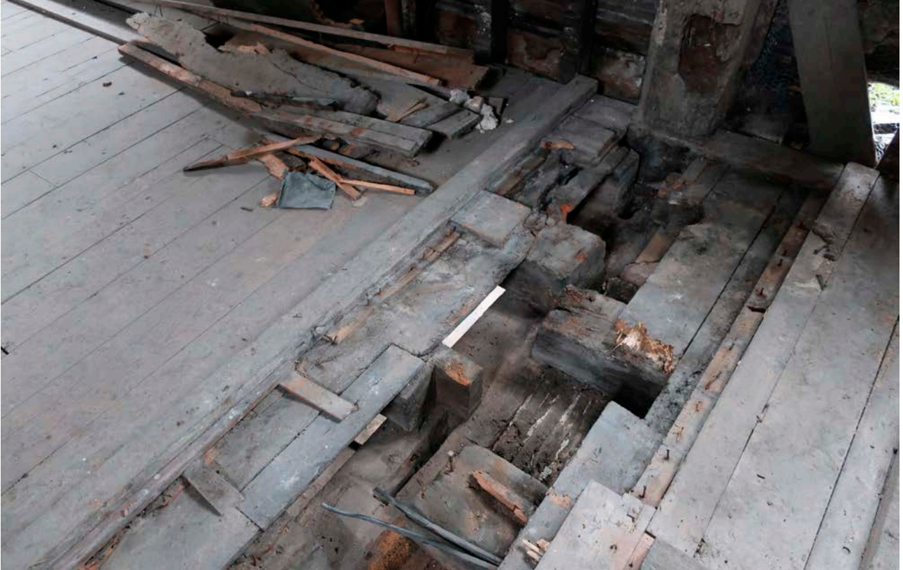
Figure 58: The upper edge of the cross beam in frame IV, looking south-west, showing empty mortices for the partition at first-floor level and the floor joists resting on top of the beam. [Rebecca Lane © Historic England]
