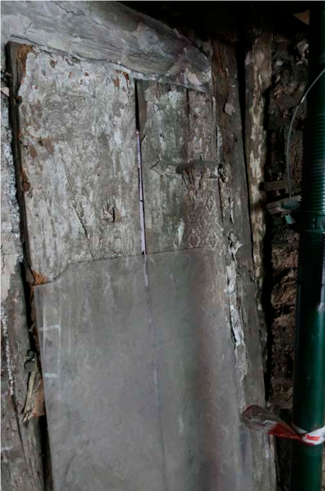
Figure 128: Detail of the inserted door in the south elevation of the street-front range at first-floor level, leading into the first floor of the west range, showing a 17th-century strapwork hinge, looking north-west. [Rebecca Lane © Historic England]
