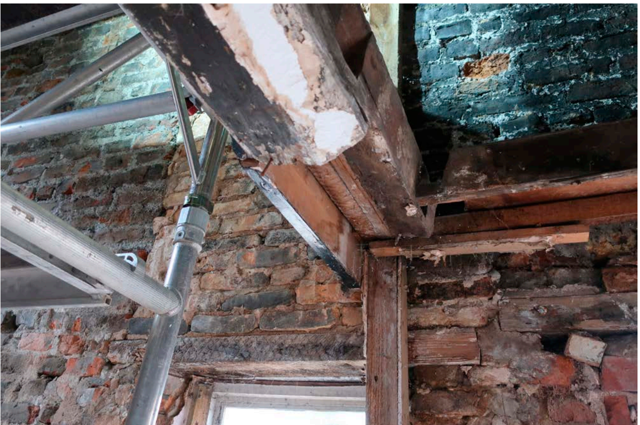
Figure 122: The southern end of the inserted beam in the south bay, looking south, showing the off set in the beam for the former chimney position. [Rebecca Lane © Historic England]
