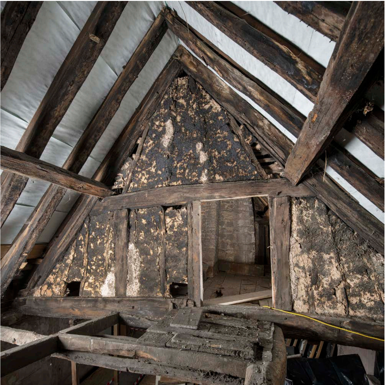
Figure 101: The southern face of the roof truss of frame III, looking north-west, showing the smoke blackening on the in situ wattle and daub panels and the timber frame. [Steve Baker © HEA DP325677]
