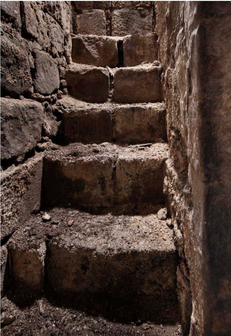
Figure 33: The original intra-mural stair in the south wall of the undercroft, looking west. [James O. Davies © HEA DP435615].
