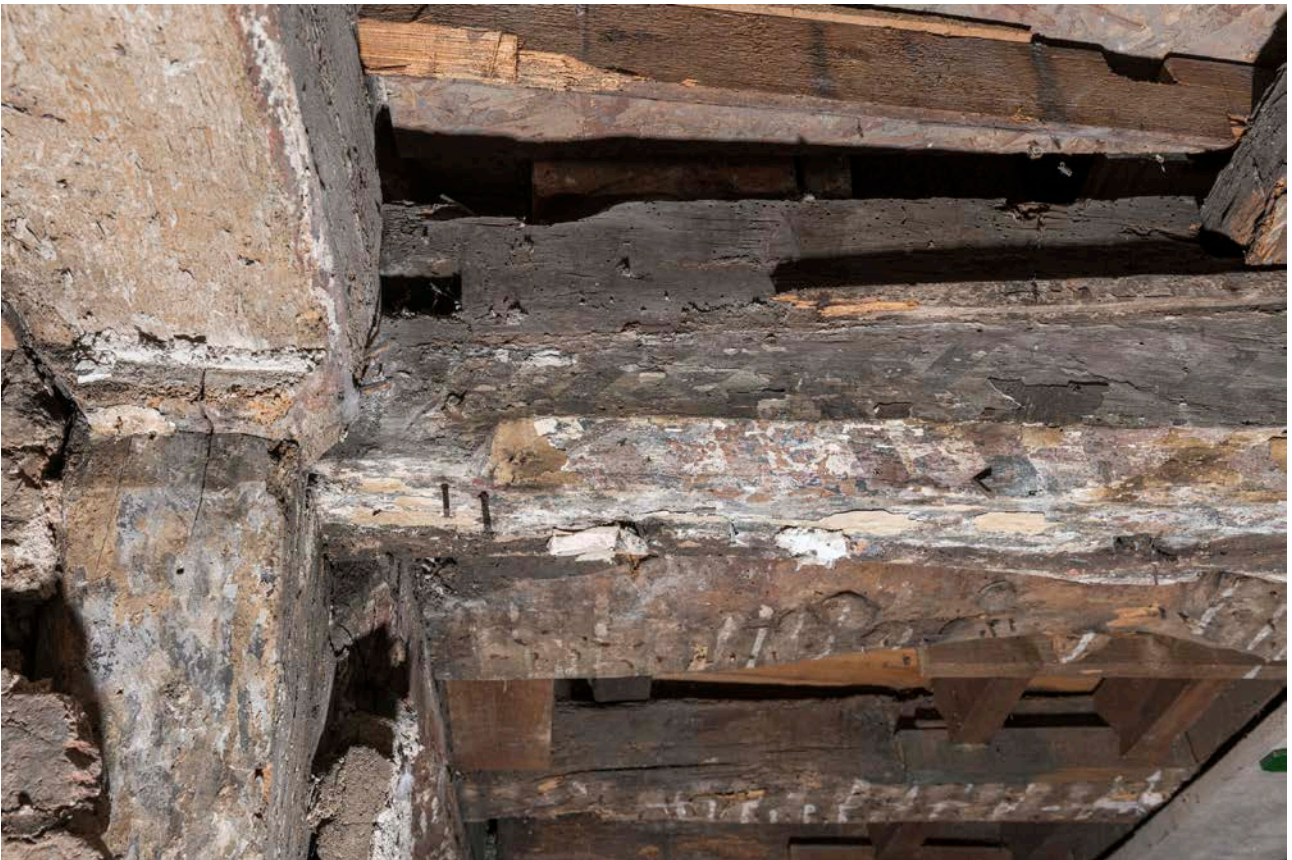
Figure 134: Black and white chevron pattern faintly visible on the timber beam and post of frame V, in bay E (No. 21), possibly applied at the same time as the pattern at ground-floor level, looking east. [Steve Baker © HEA DP325646]
