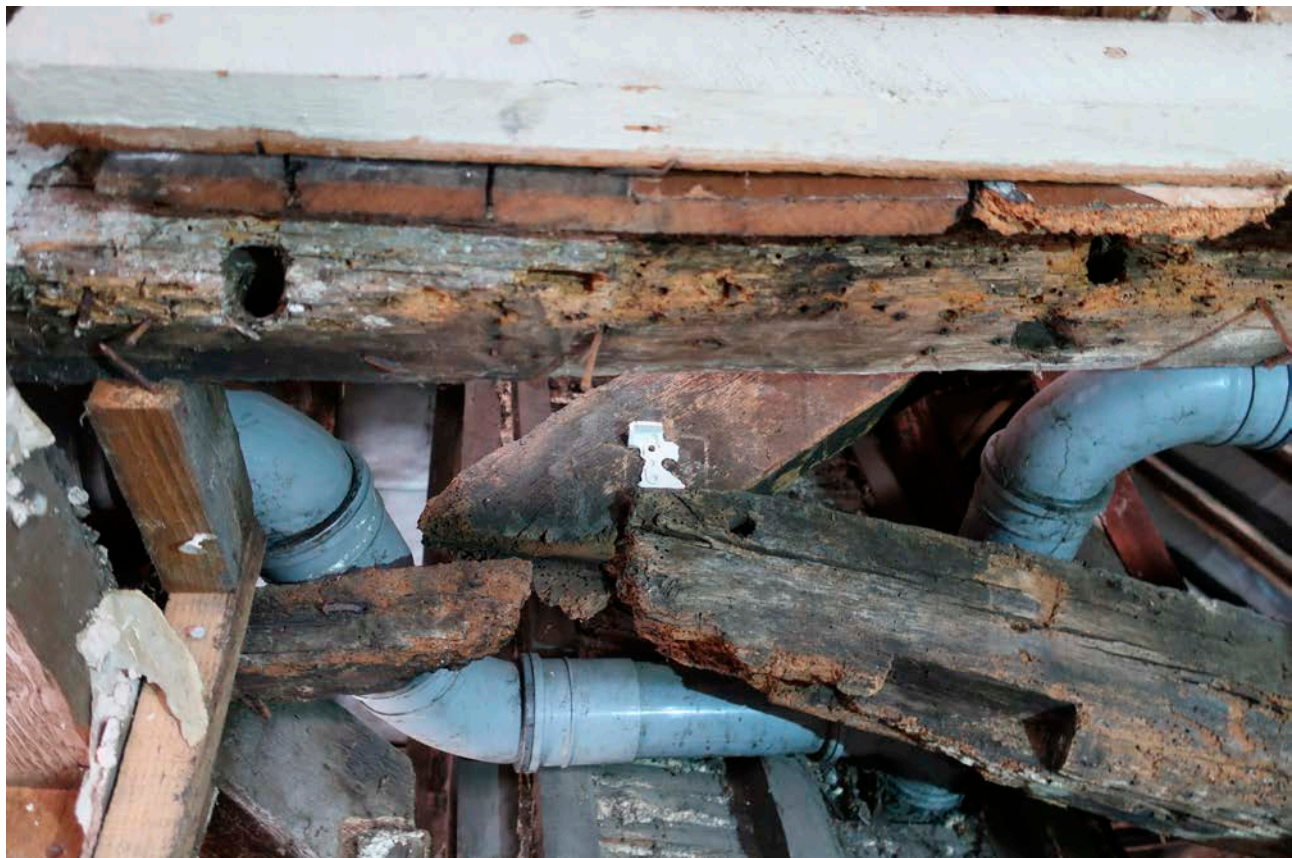
Figure 84: Girding beam in the south elevation of bay D (No. 19A) showing peg holes which may indicate the position of a window opening. [Rebecca Lane © Historic England]
