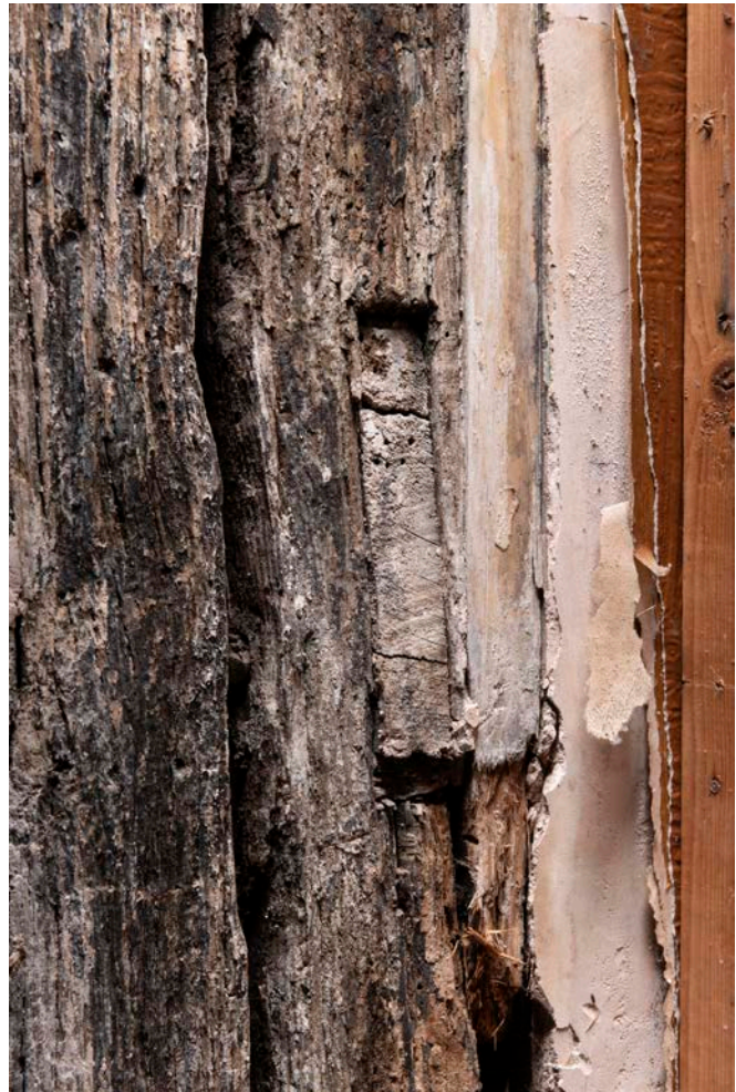
Figure 72: Detail of the mortice on the outer (western) face of the west post of frame VII, looking east, possibly indicating some form of structure originally attached to western side of the range. [James O. Davies © HEA DP435651]
