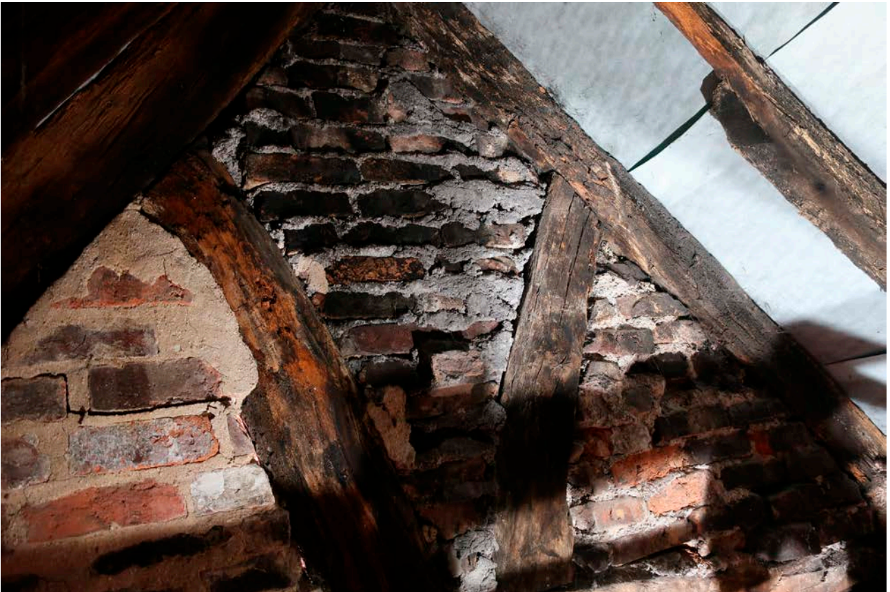
Figure 71: Upper part of the truss of frame VII, looking south-west, showing curved struts running from the collar to the principal rafters. [Rebecca Lane © Historic England]
