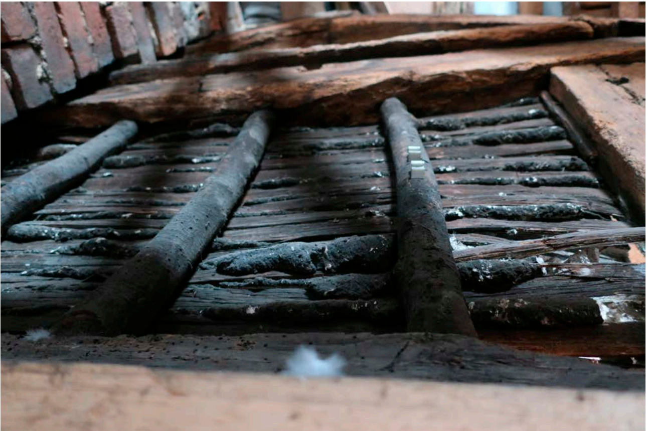
Figure 95: The north frame of the north-east corner bay, showing the northern (outer) face with the original staves with no indication of any original plaster on this side of the truss. [Rebecca Lane © Historic England]
