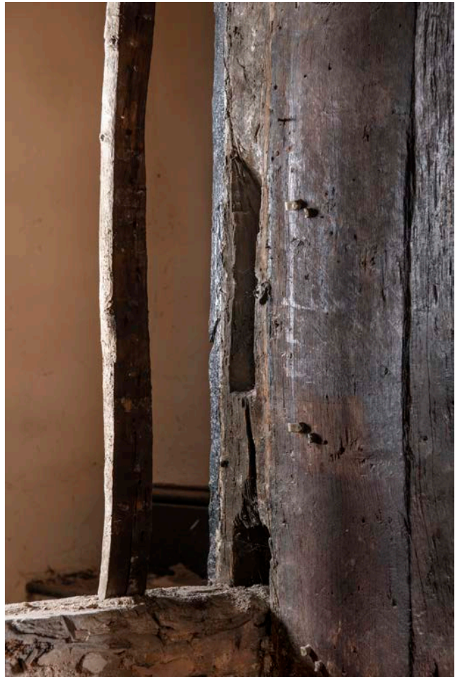
Figure 51: The west post of frame VI, looking north-west, showing the empty mortice for an up-brace. [James O. Davies © HEA DP435641]
