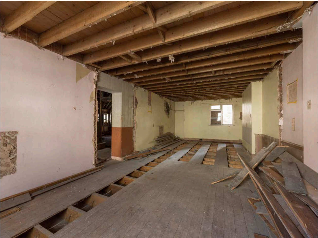
Figure 148: The first floor of No. 23, looking south-east, with floor levels as reconstructed in the 1970s. [Steve Baker © HEA DP325649]
