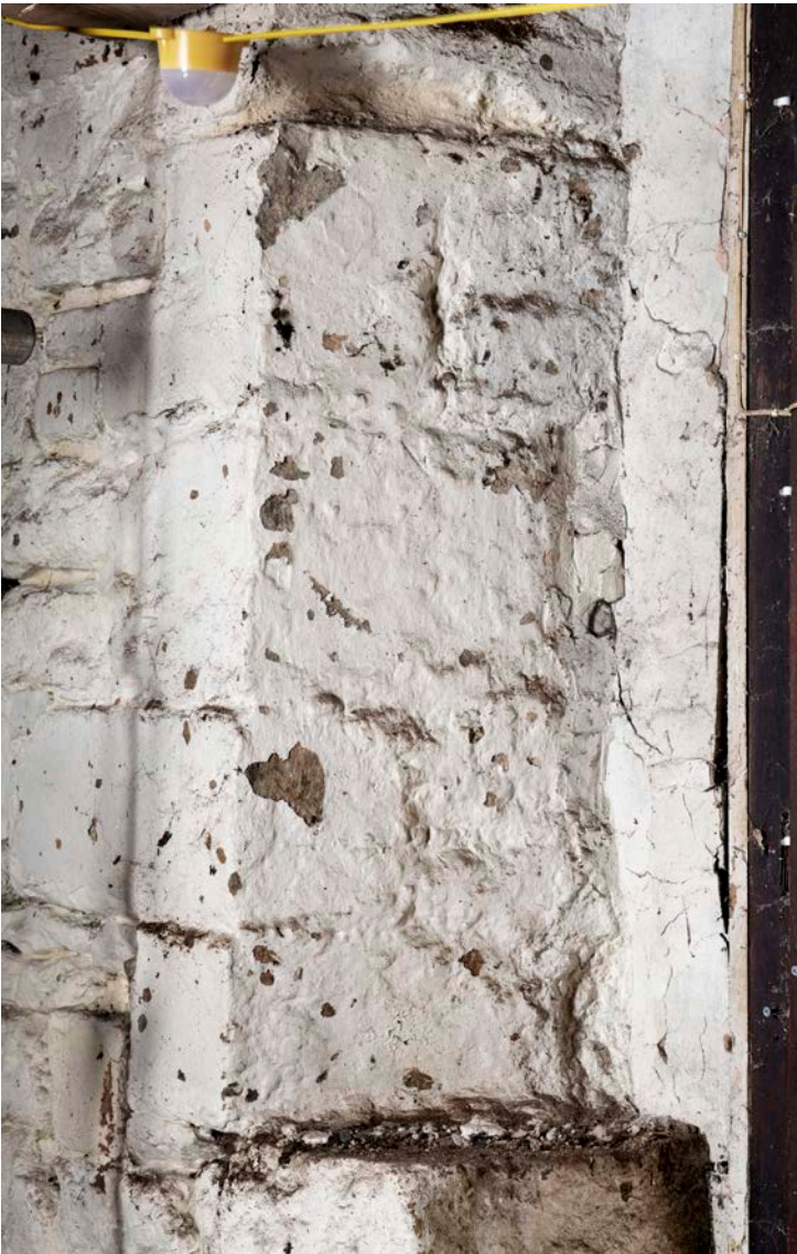
Figure 38: Splayed window opening in the north end of the undercroft, looking south-west, possibly dating from the 15th century. [James O. Davies © HEA DP435624]
