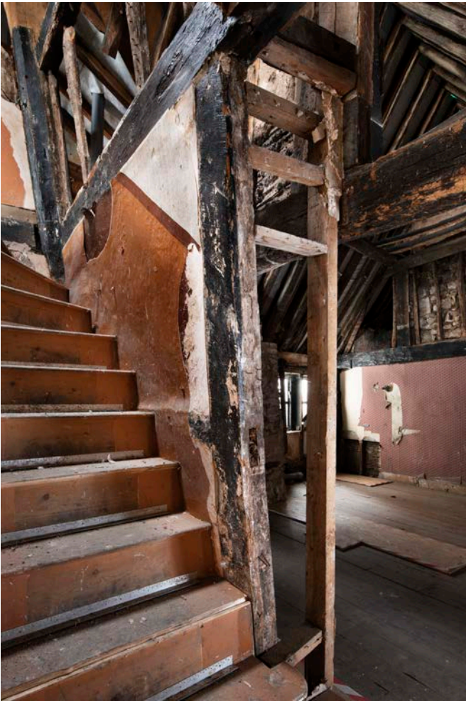
Figure 89: South elevation of the street-front range in bay E (No. 21), looking south east, showing the girding beam, stud and infill of the elevation at first-floor level. [James O. Davies © HEA DP435637]
