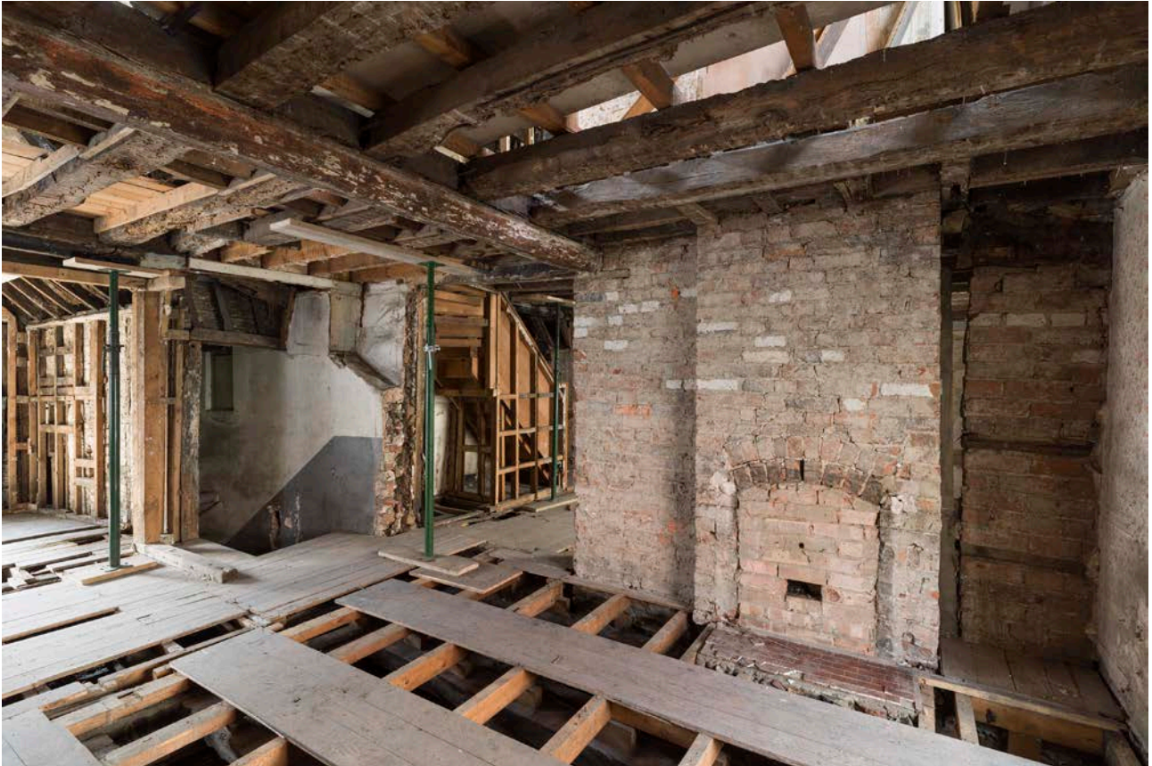
Figure 83: Bay D (No. 19A) at first-floor level, looking south-west, showing the surviving girding beam of the south wall towards the left-hand side. [Steve Baker © HEA DP325631]
