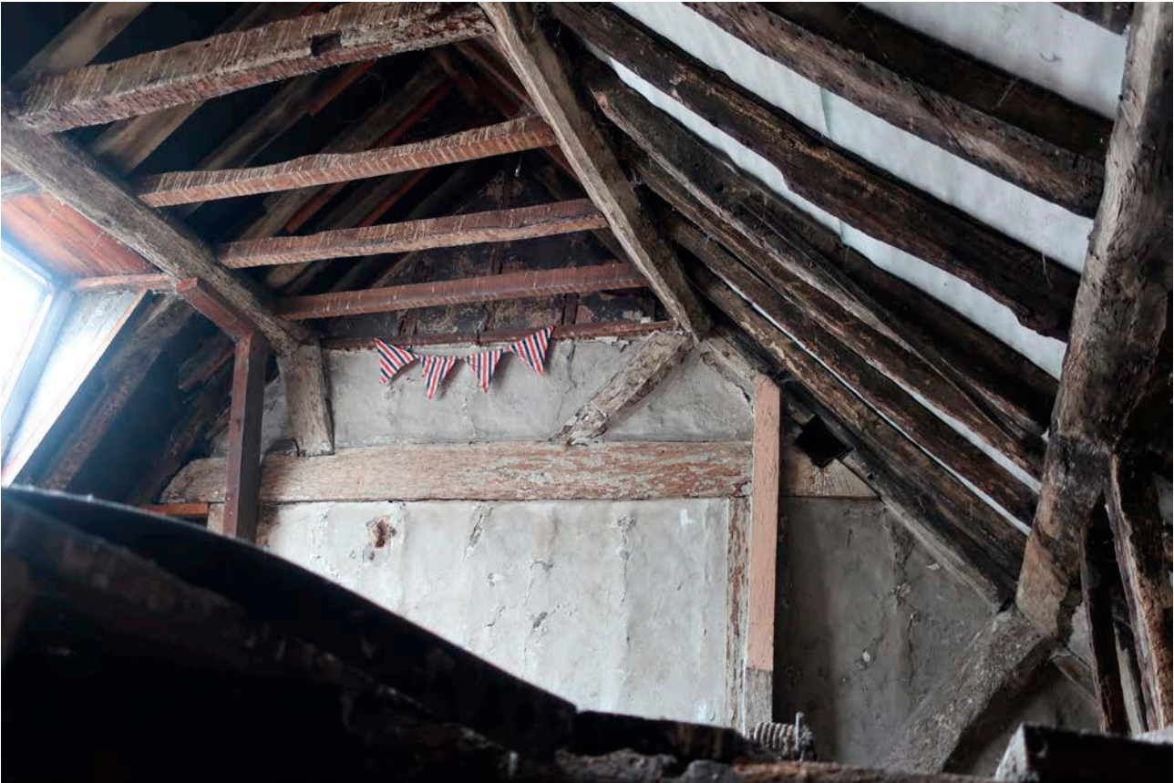
Figure 92: Frame IIII at roof level, looking north-east, showing the surviving elements of the roof truss, looking north east. [Rebecca Lane © Historic England]
