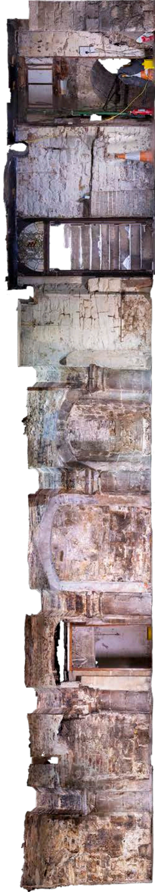
Figure 31: Rectified photograph of the west elevation of the undercroft. [Geospatial Survey © HEA DP364810]
