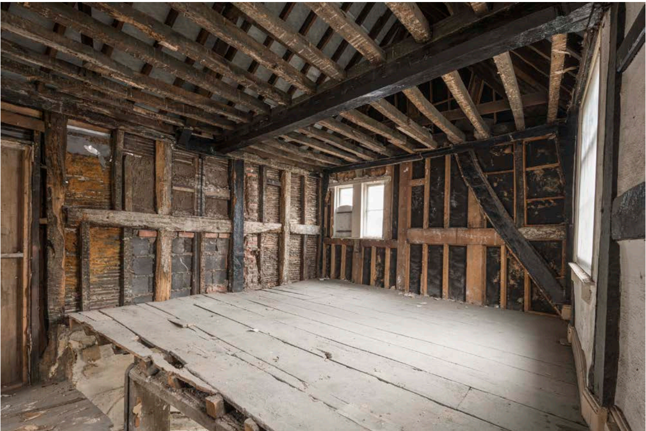
Figure 115: The south-west wing of the great inn range, internal arrangement at first-floor level, looking south-west. [Steve Baker © HEA DP325592]
