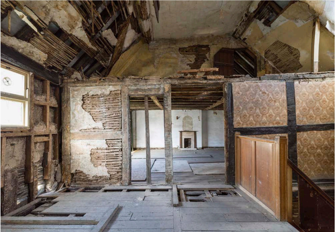
Figure 126: The ceiling inserted at collar level over the northern first-floor room of the great inn range, looking north, with the ceiling and the rafters plastered over. The partition shown below is part of the late 18th-century alterations at the site. [Steve Baker © HEA DP325625]
