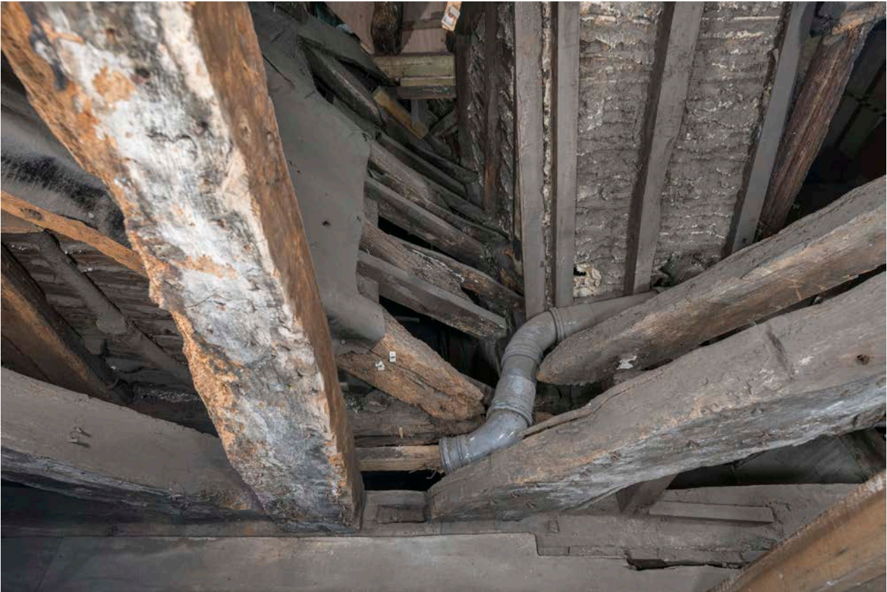
Figure 105: The junction between the main west range and the north-east corner bay, showing the rafters of both running down to the shared wall plate. [Steve Baker © HEA DP325643]
