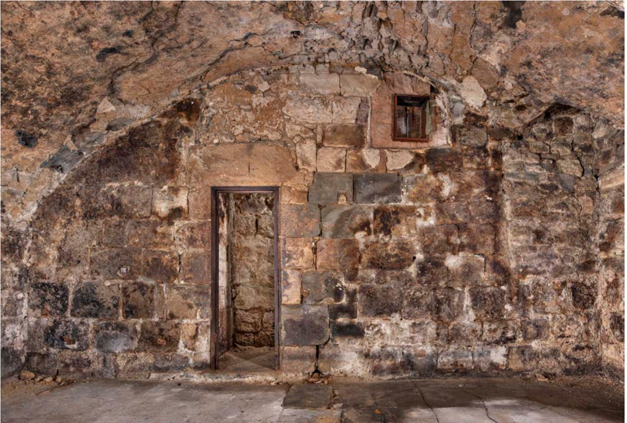
Figure 32: The south elevation of the undercroft, looking south, showing the original doorway to the intra-mural stair. [James O. Davies © HEA DP435614].
