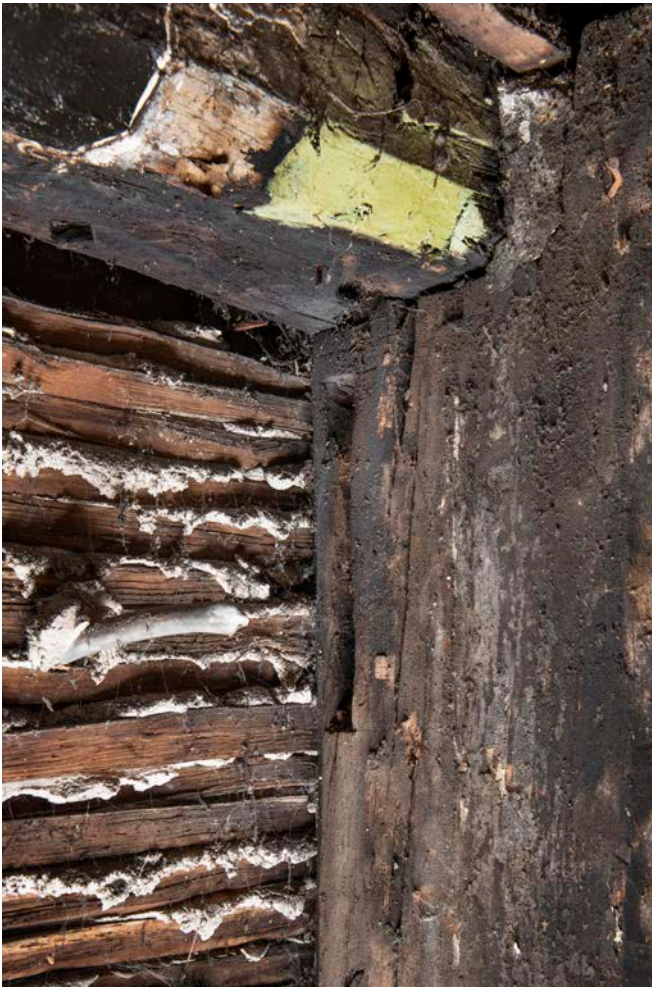
Figure 62: The west post of frame IV and the framing in bay D, looking north-west, showing the mortice for a window head and the diamond-shaped hole in the wall plate for an iron bar. [James O. Davies © HEA DP435629]
