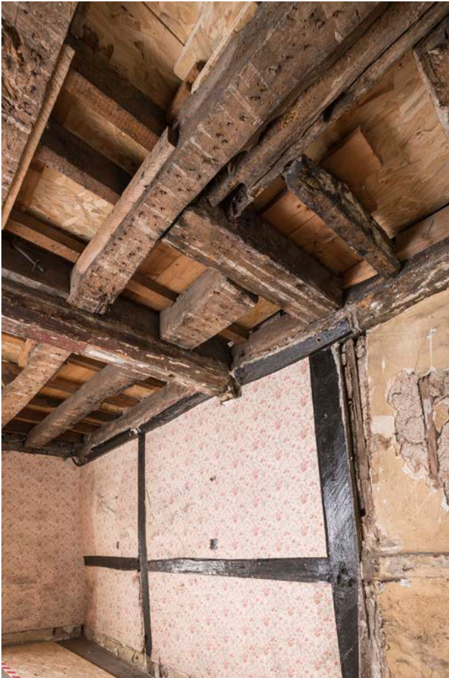
Figure 85: Ceiling at first-floor level in bay D (No. 19A), looking north-east, showing the position of a partial partition running along the central lateral beam, partly indicated by the paintwork pattern. [Steve Baker © HEA DP325686]
