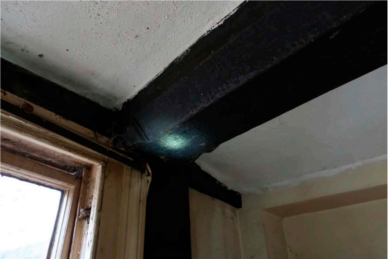
Figure 117: The cross beam at first-floor level in the south-west wing of the great inn range, looking north-east, showing chamfer stop detail. [Rebecca Lane © Historic England]
