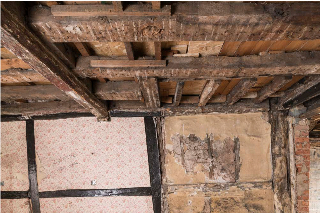
Figure 86: Ceiling at first-floor level in bay D (No. 19A), looking east, showing the stair trimmer indicating the position of the stair in the south-east corner of the bay. [Steve Baker © HEA DP325687]
