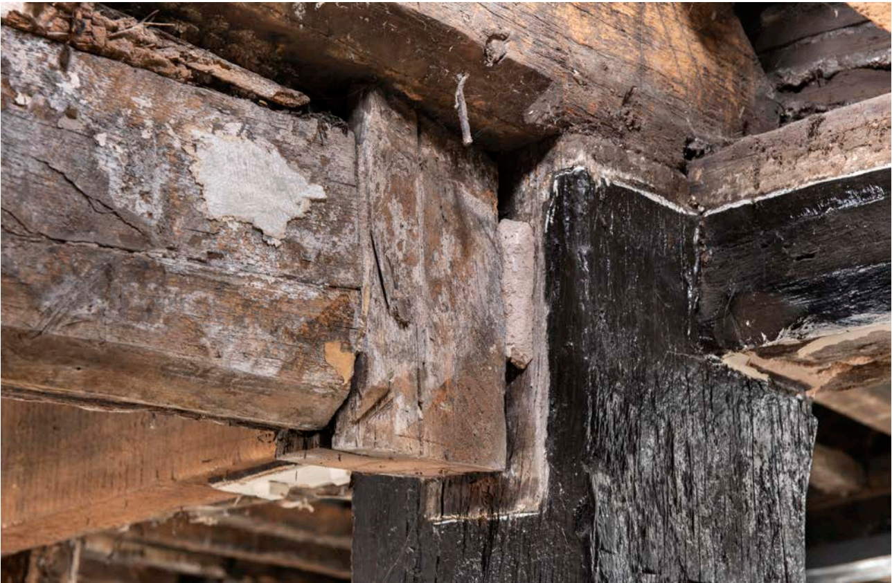
Figure 65: Detail of doorhead in frame VI, showing the chamfered lintel and the cut off jamb, looking south-west. [James O. Davies © HEA DP435646]
