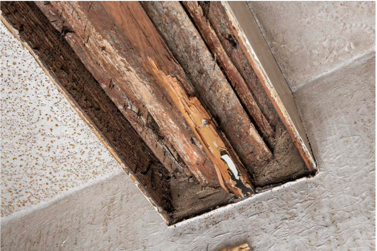
Figure 41: The cross beam of frame III, looking north-east, showing the moulding on the underside of the beam. [James O. Davies © HEA DP435628]
