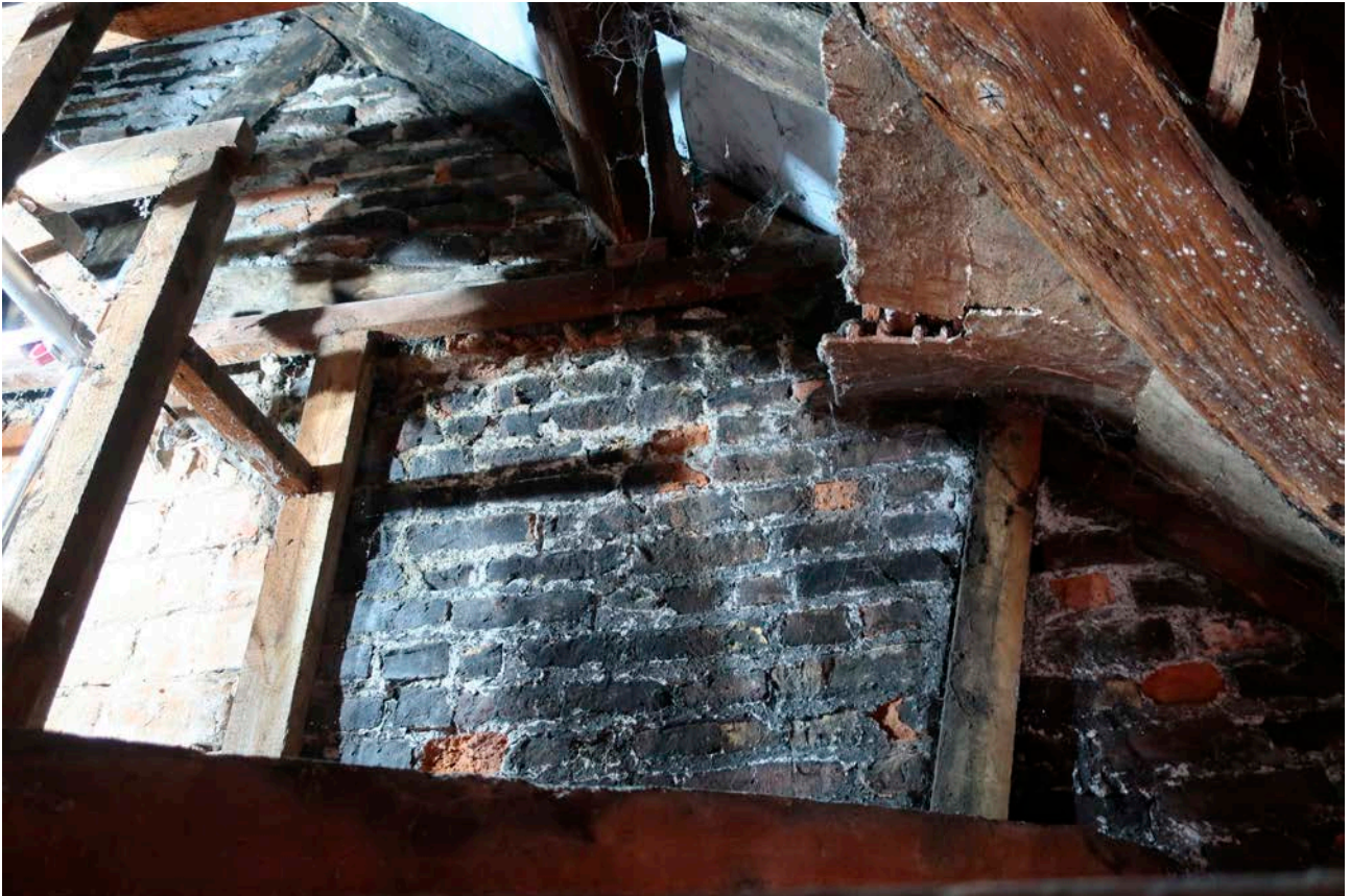
Figure 124: The south elevation of the great inn range at roof level, looking south, showing place bricks inserted around the original timber frame, blackened by soot from the adjacent chimney position. [Rebecca Lane © Historic England]
