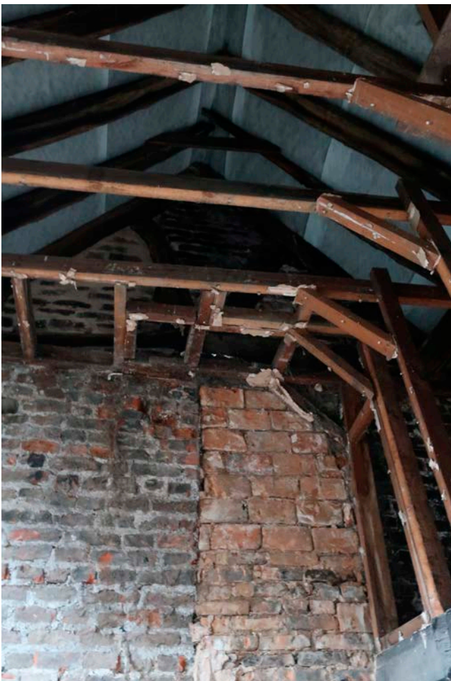
Figure 125: The south elevation of the great inn range at roof level, looking south-west showing the place bricks inserted into the eastern part of the elevation. [Rebecca Lane © Historic England]
