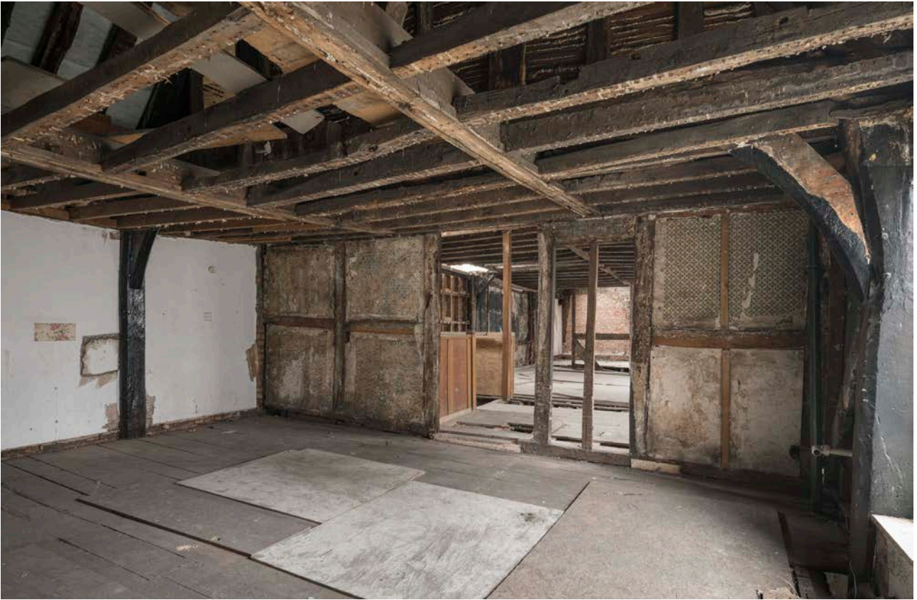
Figure 131: The inserted partition at the north end of the first-floor level in the great inn range, showing early wall paper on its northern face, looking south. [Steve Baker © HEA DP325596]
