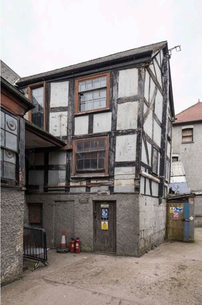
Figure 116: The south-west wing of the great inn range, north elevation, looking south. [Steve Baker © HEA DP325654]
