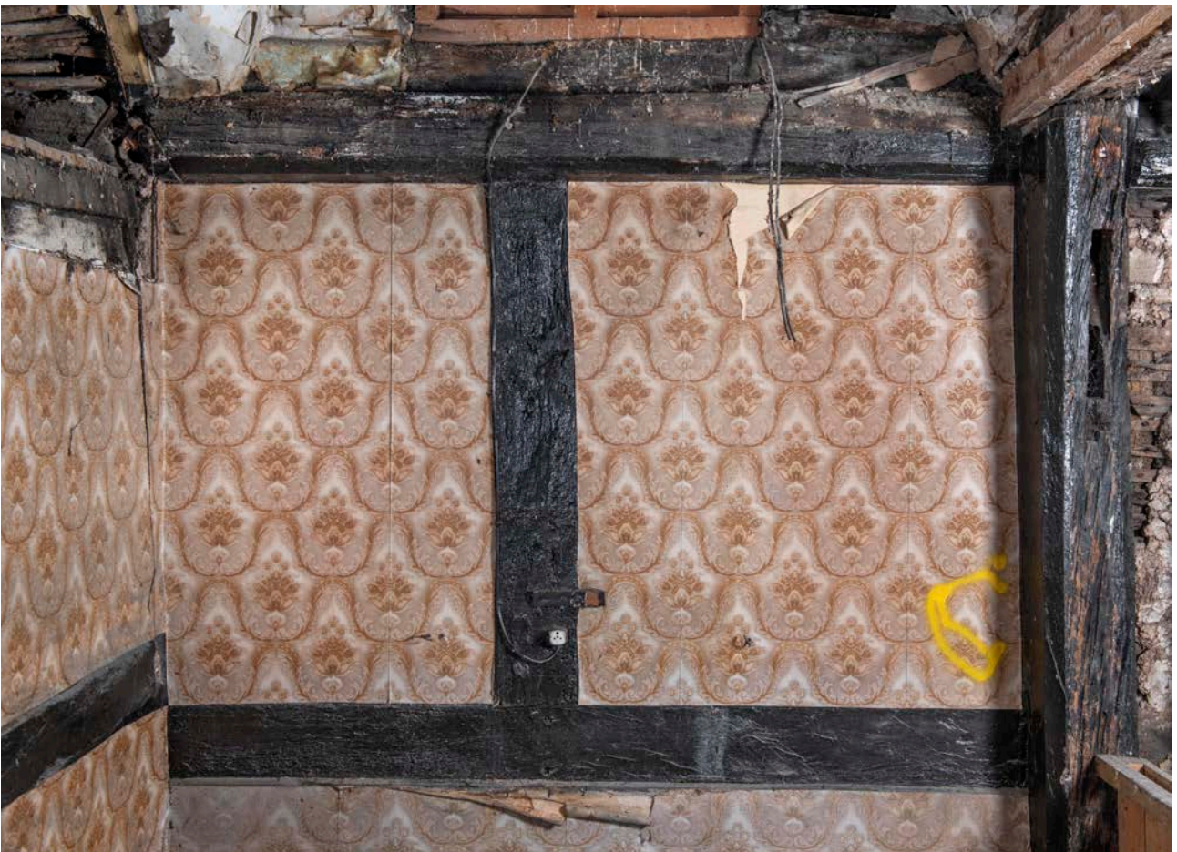
Figure 56: The timber framing of the east elevation of bay C, looking east, showing the mid-rail and stud arrangement. [James O. Davies © HEA DP435653]
