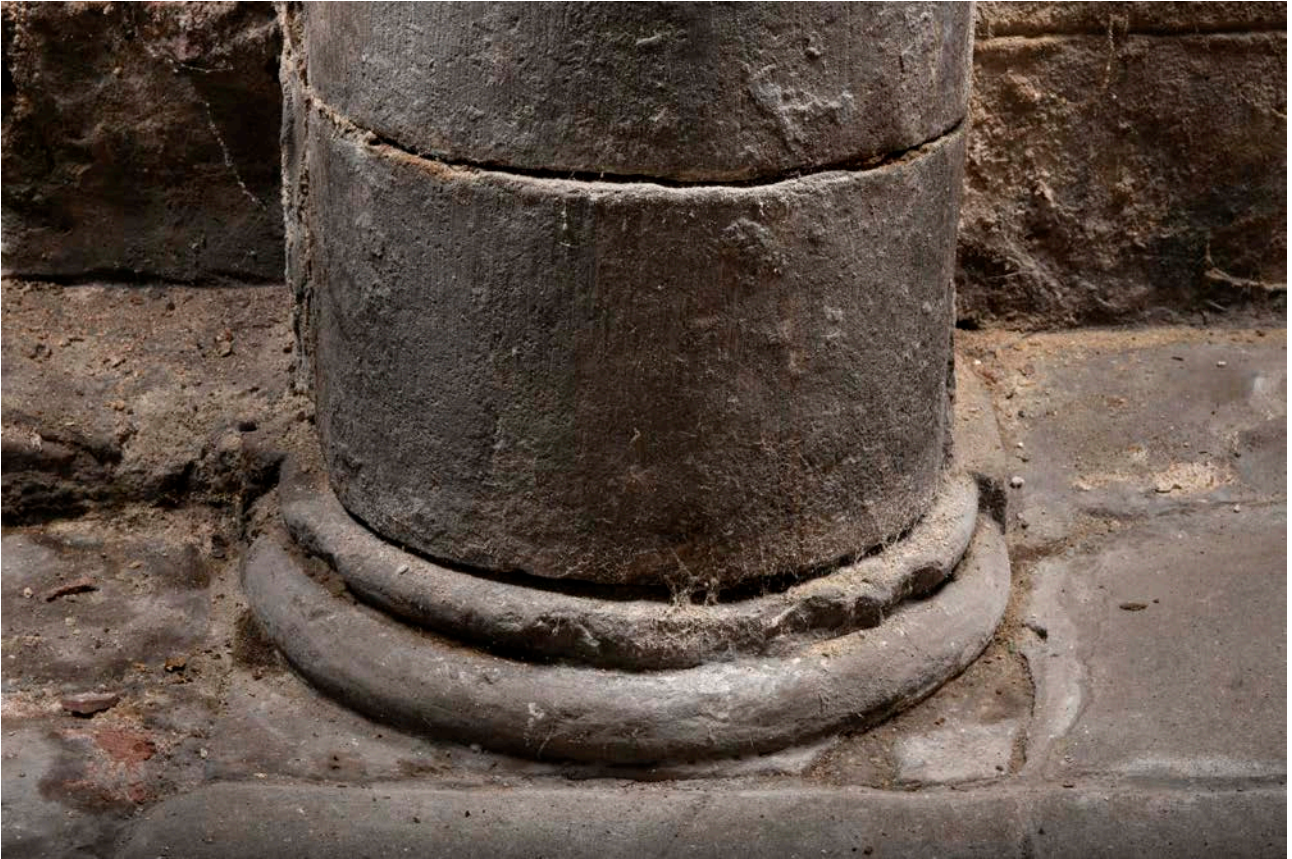
Figure 28: The base of one of the engaged columns in the undercroft, looking west. [James O.Davies © HEA DP435623]
