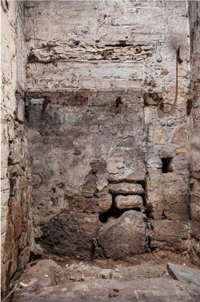
Figure 129: Inserted stone and brickwork at the north end of the undercroft of the great inn range, with the position of a doorway visible, with later stone infill, looking north. [James O. Davies © HEA DP435613]
