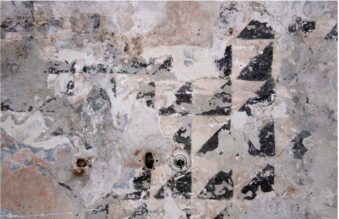
Figure 133: Diamond pattern decoration on the ground-floor ceiling of bay E (No. 21), possibly applied in the 18th century. [James O. Davies © HEA DP435655]
