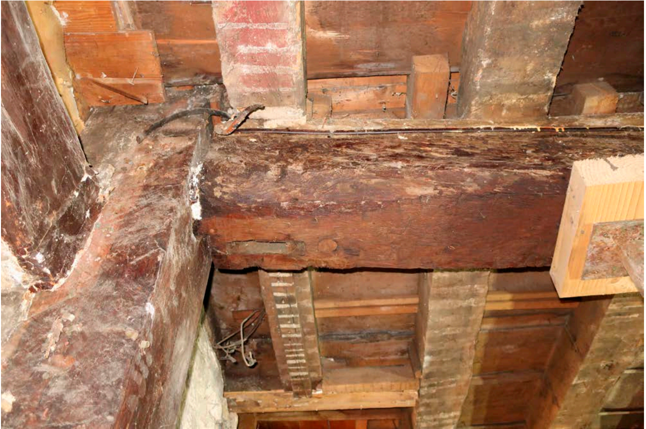
Figure 49: The cross beam of frame VI, looking north, showing the mortice for the western jamb of the doorway. [Rebecca Lane © Historic England]
