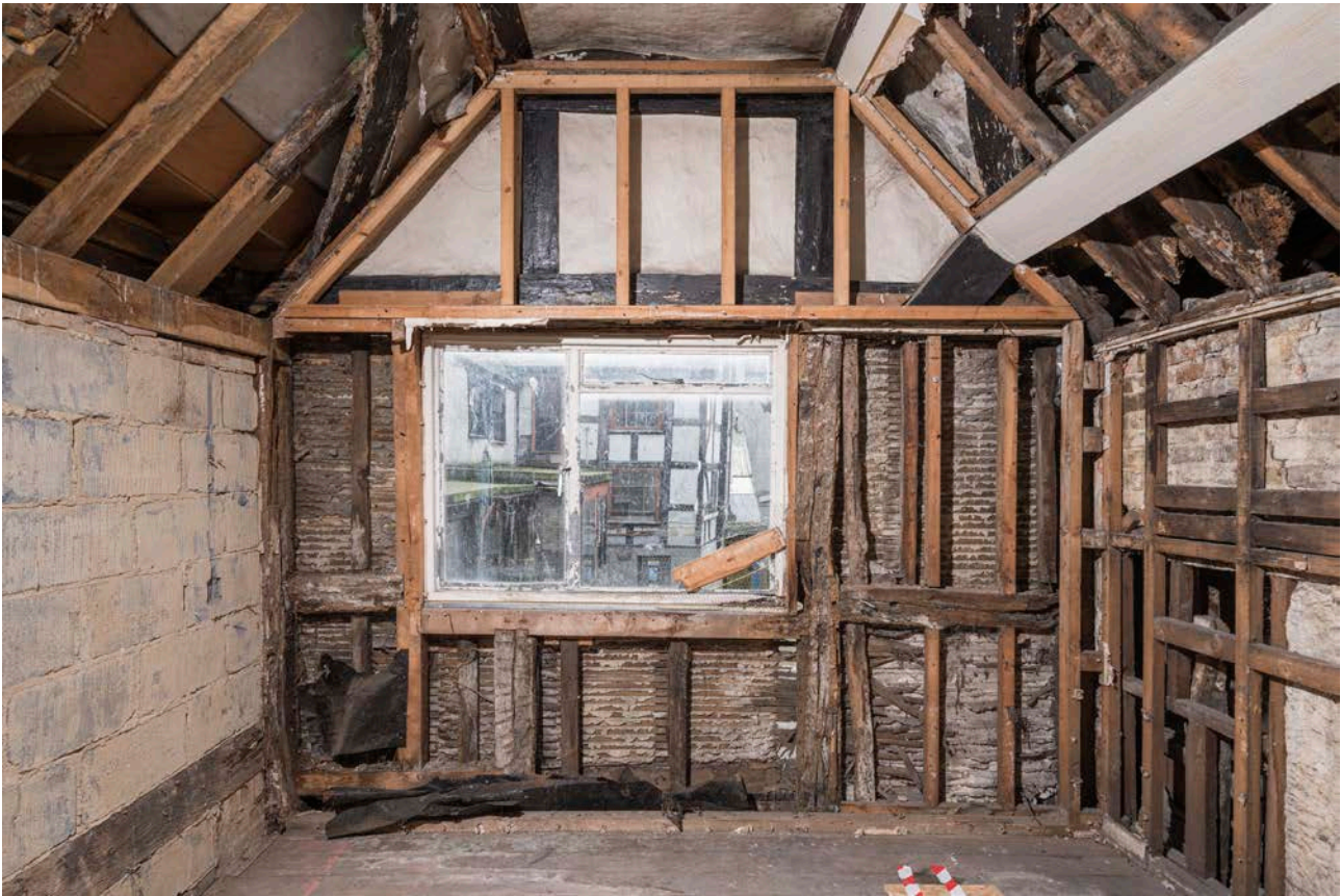
Figure 109: The first-floor room of the north-east corner bay, looking south, showing the framing of the south elevation. [Steve Baker © HEA DP325678]
