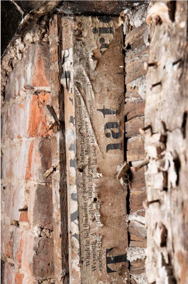
Figure 137: Inserted timber stud in the west elevation of the great inn range, with a section of a paper playbill attached to the side showing the date 1802. [James O. Davies © HEA DP435631]
