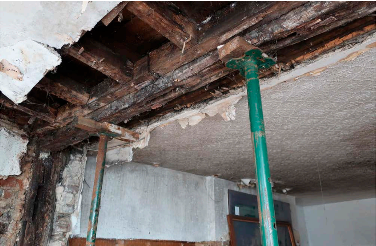
Figure 39: Girding beam forming part of the west elevation of the great inn range, looking north-east, with empty mortices showing the position of studs and window openings. [Rebecca Lane © Historic England]
