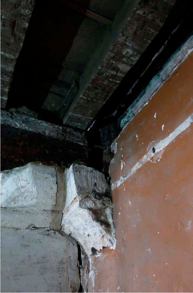
Figure 135: Inserted stone corbel with a sunk chamfer decoration on the side, supporting the earlier cross beam of frame V at ground-floor level in the great inn range, looking north-east. [Rebecca Lane © Historic England]
