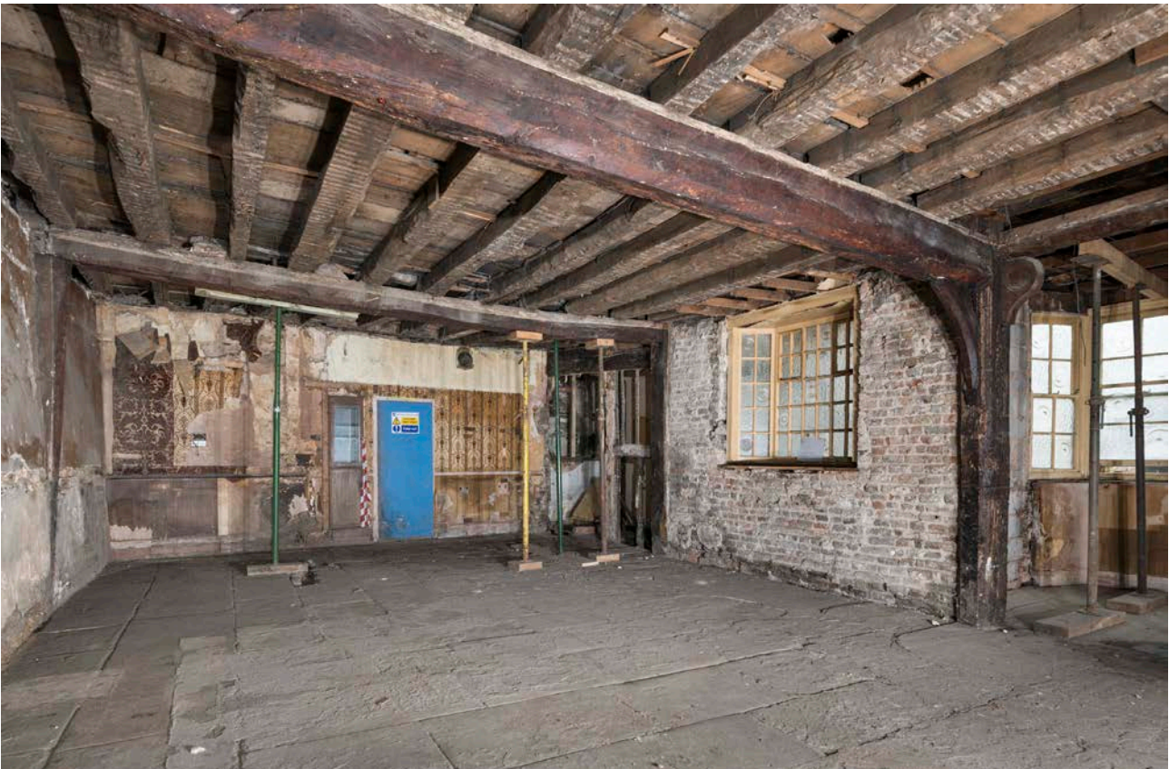
Figure 47: The southern part of the ground-floor area of the great inn range, looking south-west. [Steve Baker © HEA DP325600]
