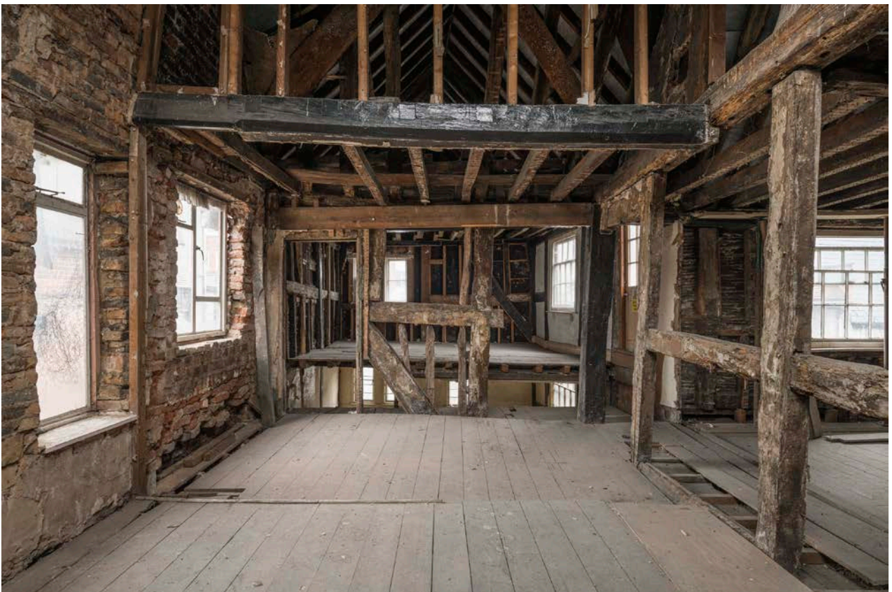
Figure 120: The inserted beam in the south bay of the great inn range at first-floor level, lapped onto the earlier partition to the north (right), looking west. Also showing the positions of the joists for the section of the ceiling which was later removed. [Steve Baker © HEA DP325590]
