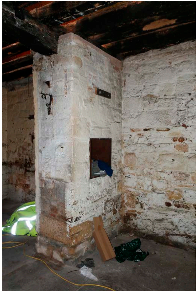
Figure 113: The undercroft in the great inn range, looking north-east, showing the inserted stone piers and timber beams of the raised floor at the northern end of the building. [Rebecca Lane © Historic England]
