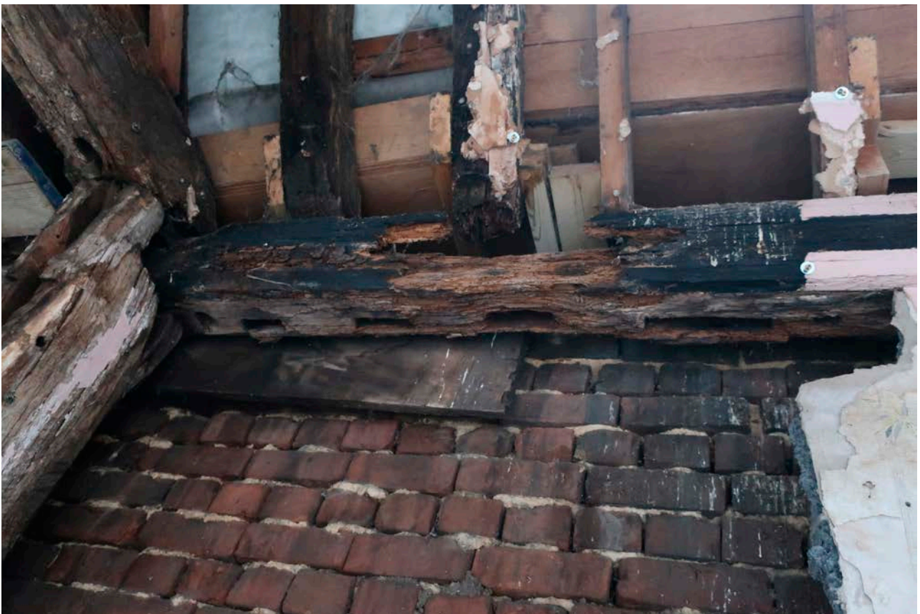
Figure 67: Underside of the wall plate of the eastern elevation in the south bay (bay E), looking north-east showing the mortice for a window position. [Rebecca Lane © Historic England]
