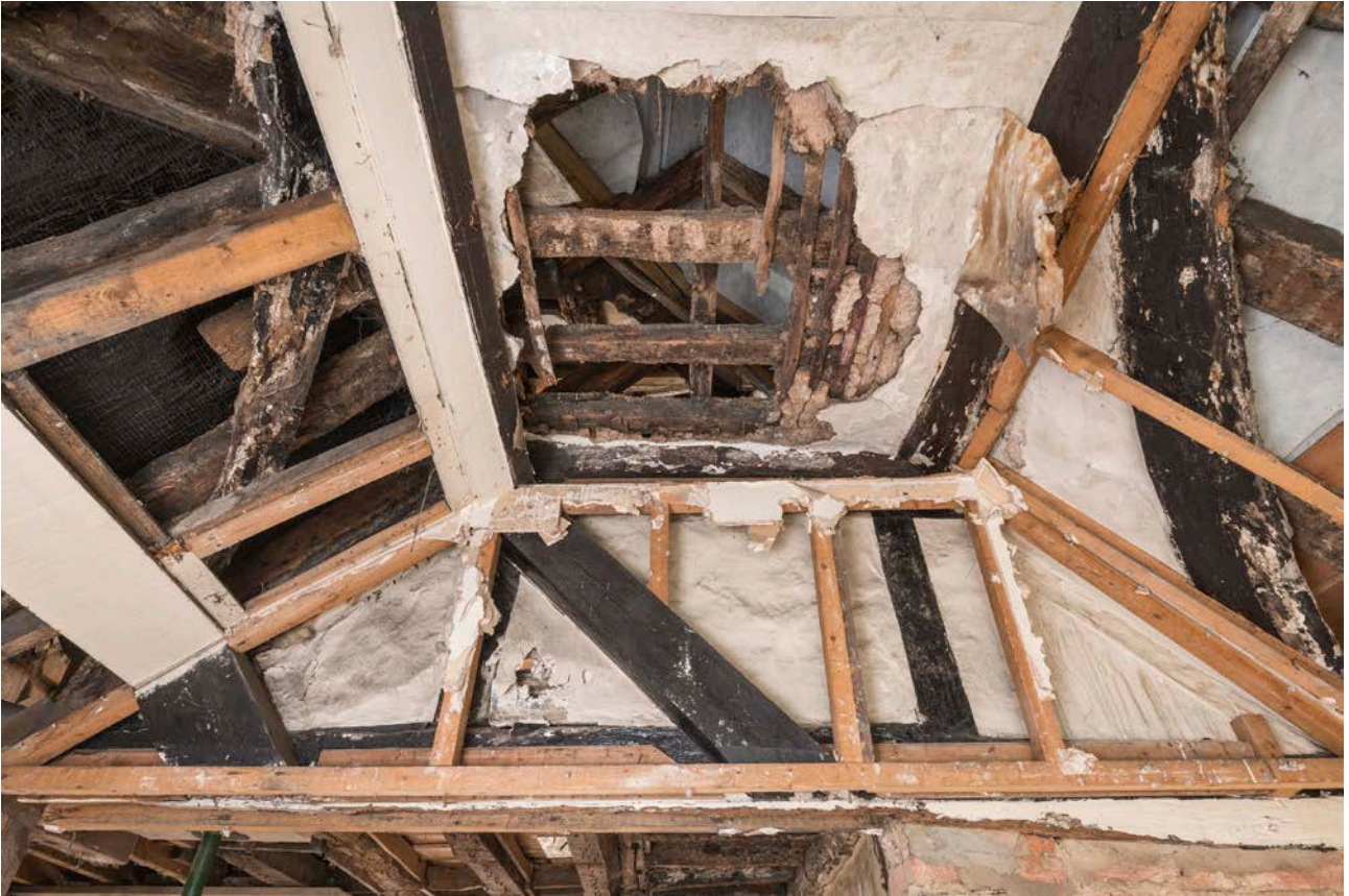
Figure 108: The roof truss arrangement of the northern frame of the north-east corner bay, looking north, with later timber and plaster ceiling inserted. [Steve Baker © HEA DP325683]
