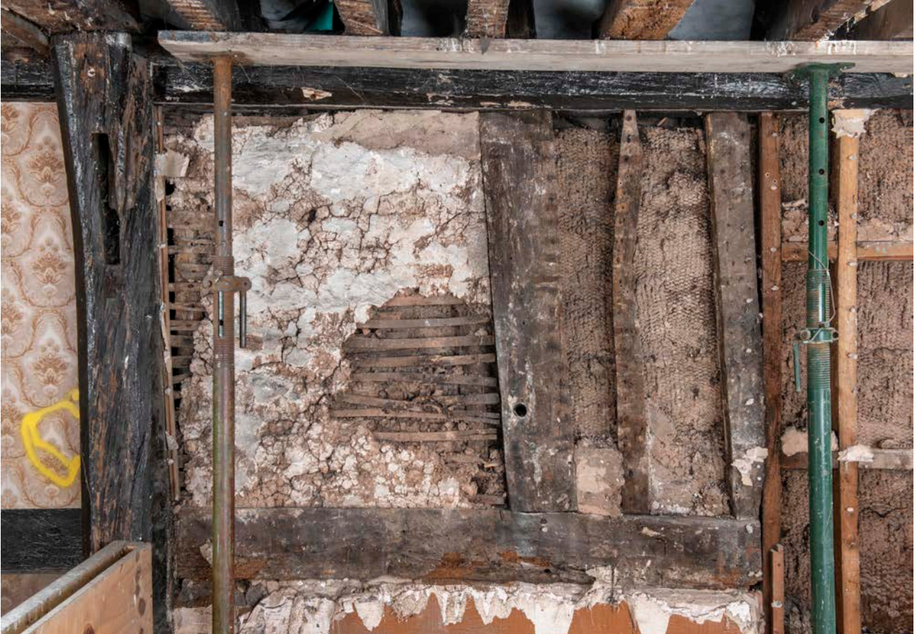
Figure 61: Surviving framing of the east elevation of bay D, looking east, with surviving wattle and daub infill. [James O. Davies © HEA DP435652]
