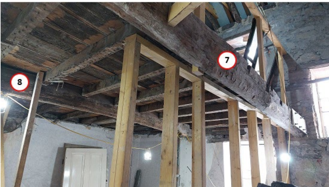
Figure 6: 2nd floor, south-west room, annotated photograph (looking south) to help identify sampled timbers (photograph Robert Howard)
