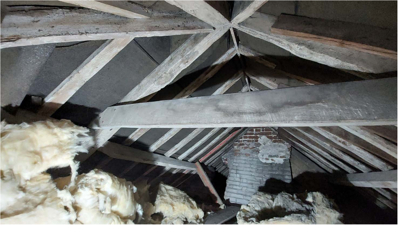
Figure 3: The roof over the primary part of the building with the oak principal rafters in the foreground, photograph taken from the south-west (Alison Arnold)
