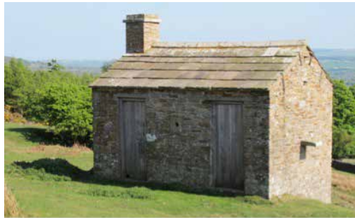
Figure 10.10 The Com-mandants/observation post of the Wensleydale Volunteers Rifle Range reroofed with grant aid from the Yorkshire Dales National Park Authority in 1995
