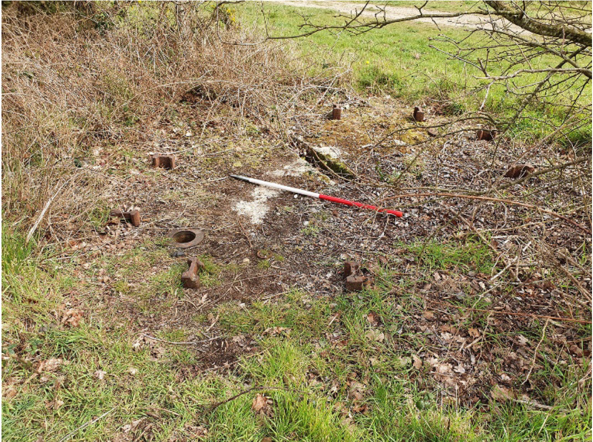
Figure 50: The surviving remains of the southern-most gun position (No.4 on fig 64) of the Browdown Second World War HAA battery. Beneath the grass and moss is the circular reinforced concrete base pad with the radial cable duct (top) and embedded with the recesses for the gun holdfast bolts and an outer ring of steel column sections. Photograph © Fiona Small 01-April-2021
