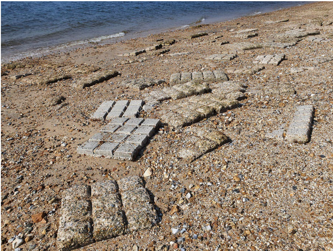
Figure 58: Dislocated fragments of the precast sections of ‘chocolate block’ concrete matting from G1 embarkation hard scattered across the shingle beach at Stokes Bay. 21-MAY-2021. (Photograph © Fiona Small).
