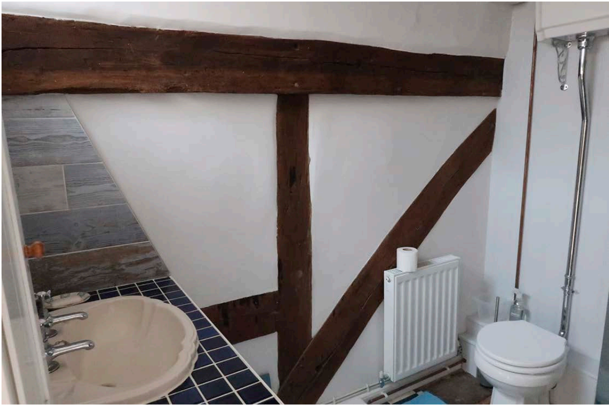
Figure 33: The west brace of the north truss of the middle bay, seen from the north. [Johanna Roethe © Historic England]
