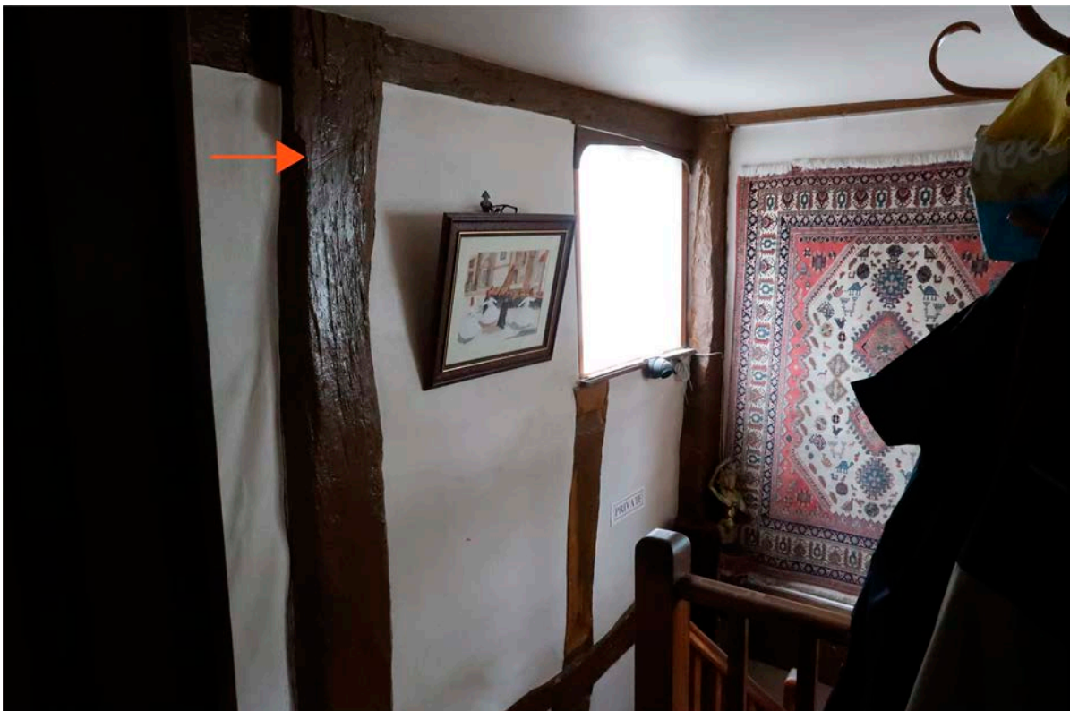
Figure 20: The south-east corner of the rear bay at first-floor level, with an arrow indicating the location of one of the carpenters' marks on the full-height stud. [Johanna Roethe © Historic England]
