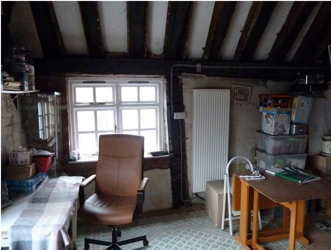
Figure 22: The west wall of the second floor of the south bay. [Johanna Roethe © Historic England]
