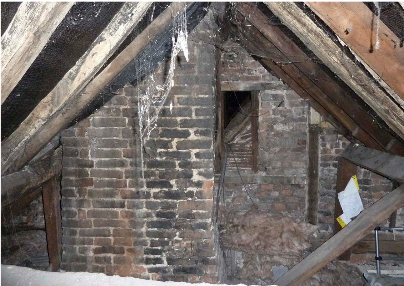
Figure 40: The chimneystack at the north end of the roofspace of the middle bay. [Johanna Roethe © Historic England]
