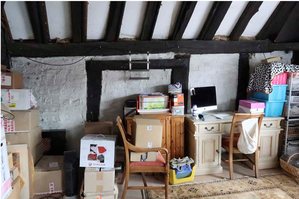
Figure 21: The east wall of the attic of the south bay, showing the three studs and wall plate (with a later horizontal timber lapped onto the inner side of two of the studs). [Johanna Roethe © Historic England]
