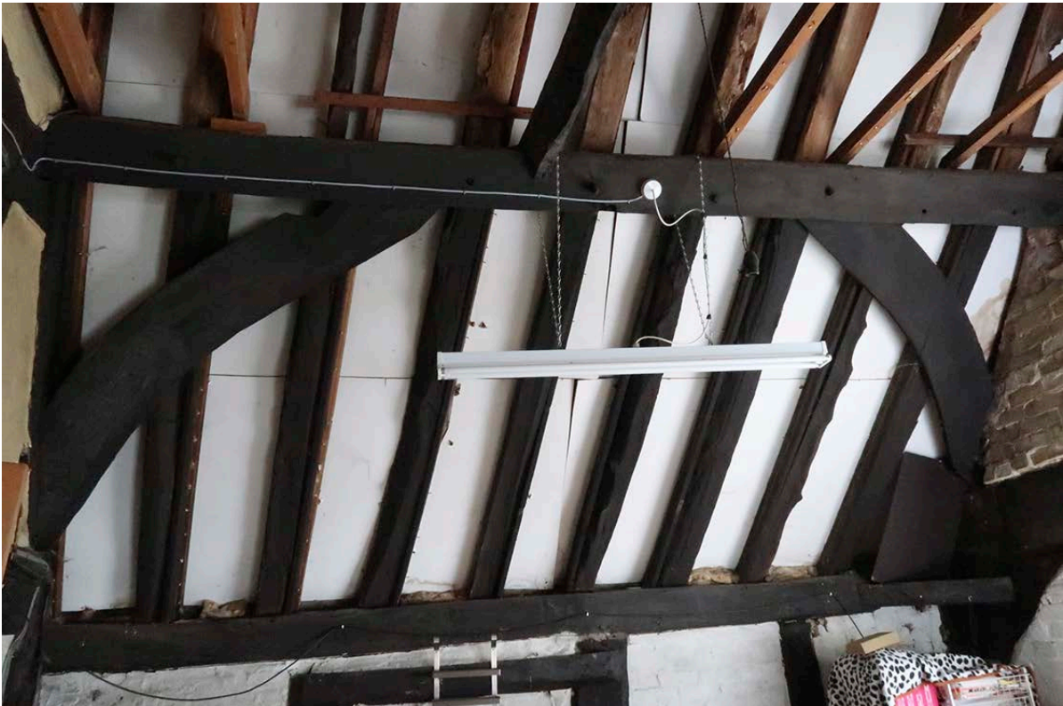
Figure 28: The windbraces on the east side of the south roof. [Johanna Roethe © Historic England]
