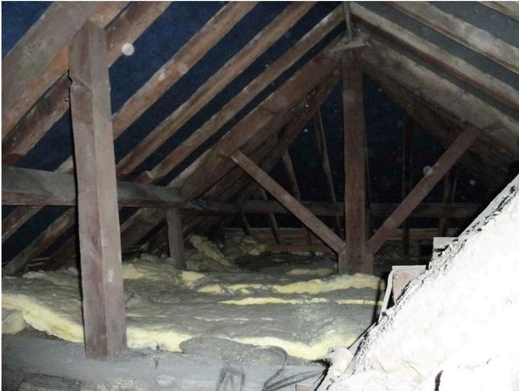
Figure 43: The king-post truss in the roof of the north bay, looking north. [Johanna Roethe © Historic England]
