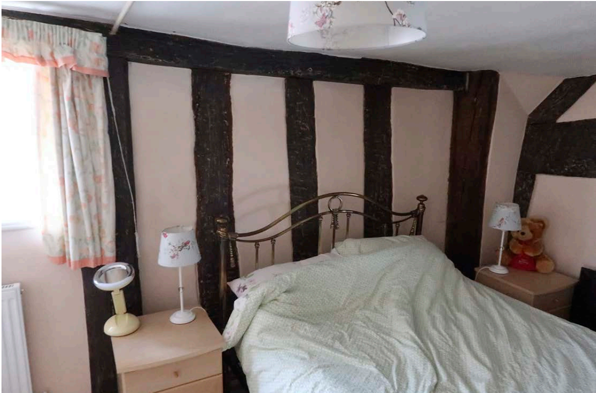
Figure 32: Close studding in the west wall of the middle bay at second-floor level. [Johanna Roethe © Historic England]
