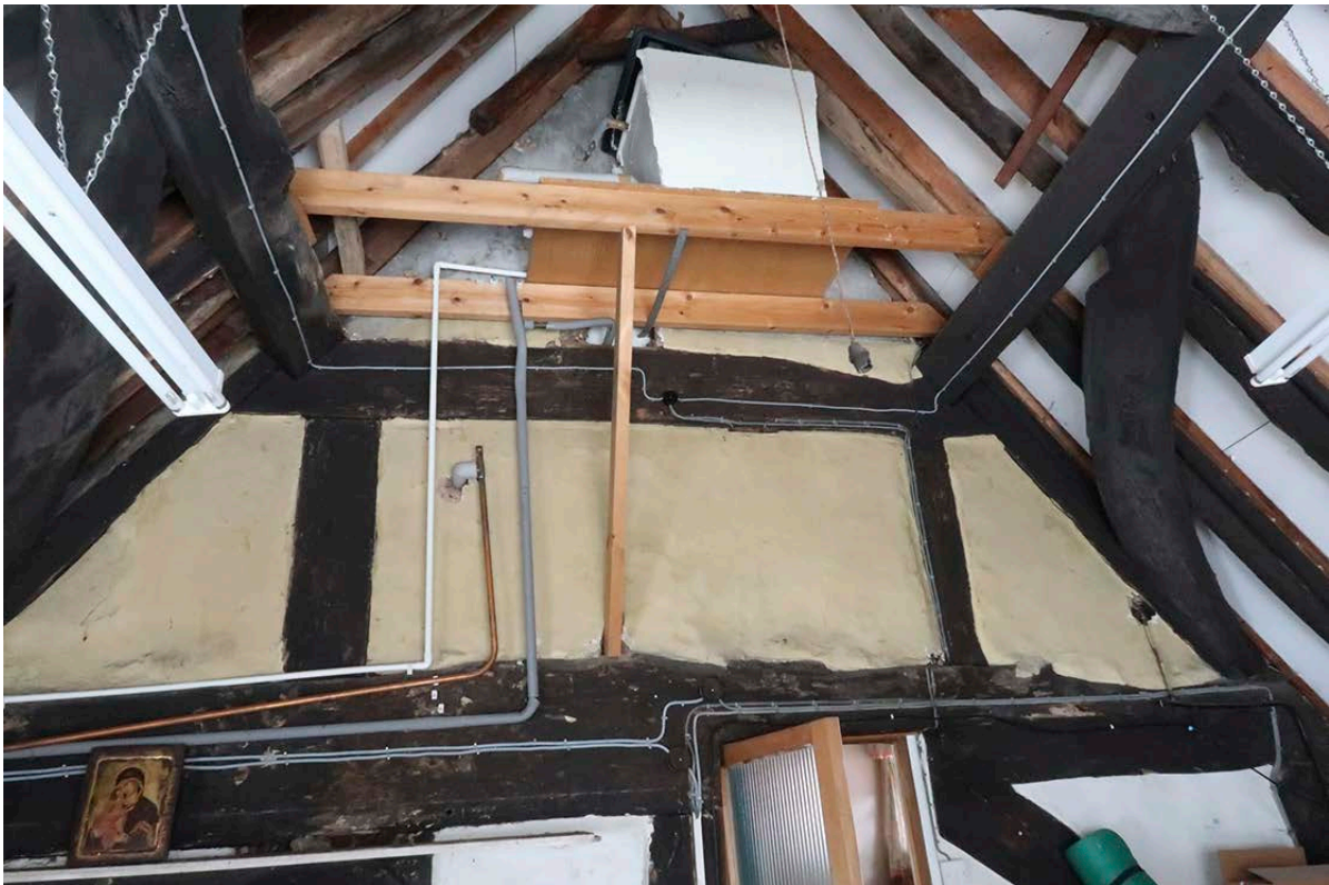
Figure 24: The upper part of the north truss of the south bay, seen from the south. [Johanna Roethe © Historic England]
