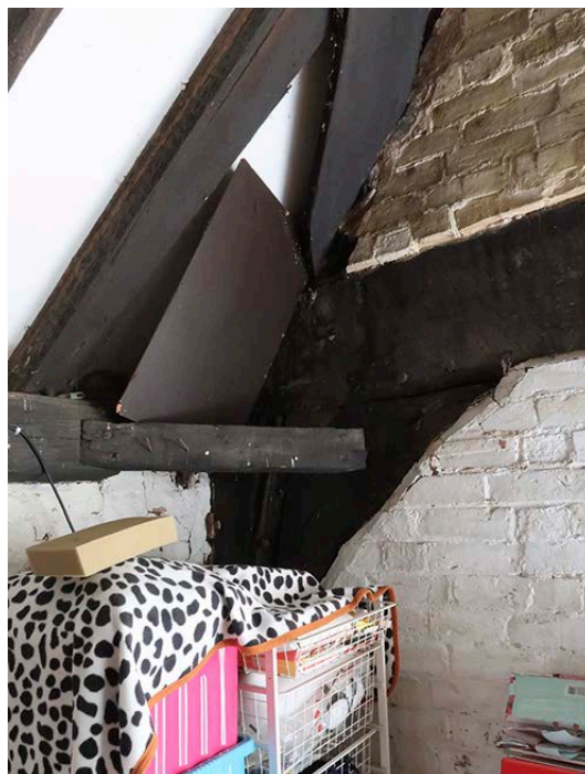
Figure 27: The knee brace in the south-east corner of the south bay (with a later timber infilling the corner between the brace, the post and the tie beam, and a further later timber spanning the corner between the wall plate and the brace). [Johanna Roethe © Historic England]
