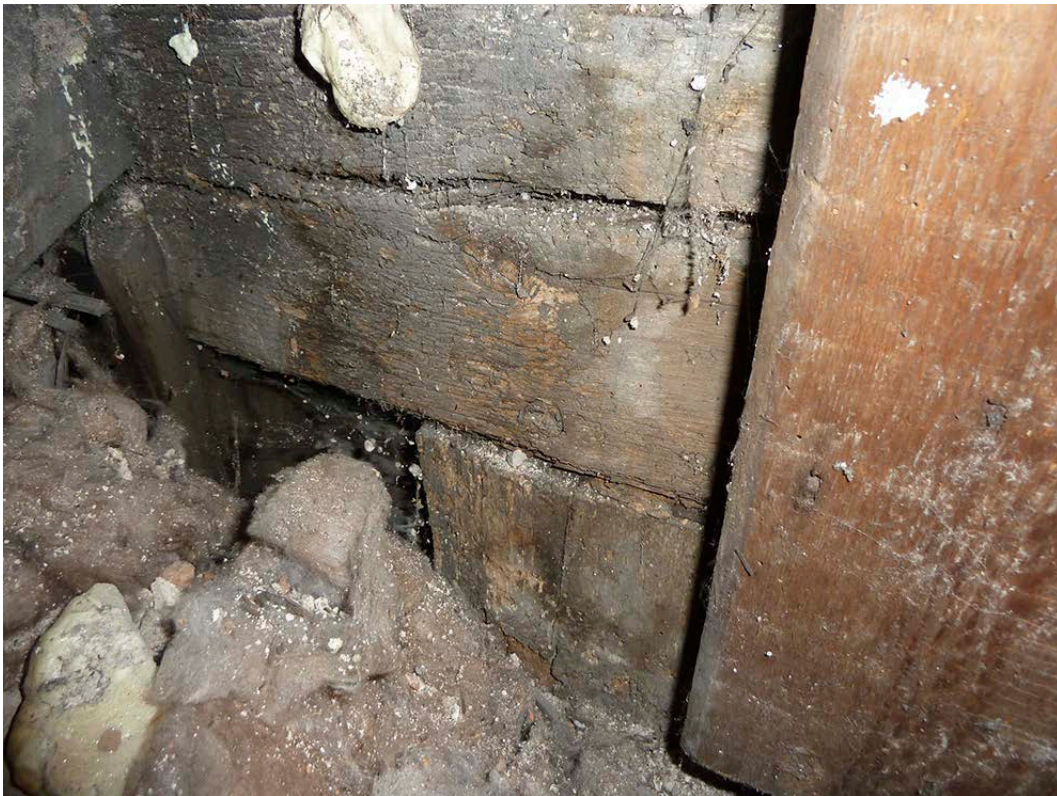
Figure 35: A pegged timber (centre bottom) below the tiebeam of the north truss of the middle bay. [Johanna Roethe © Historic England]
