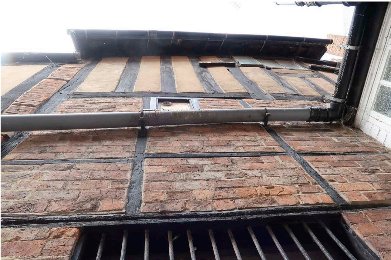
Figure 31: The close studding of the second floor of the middle bay. [Johanna Roethe © Historic England]
