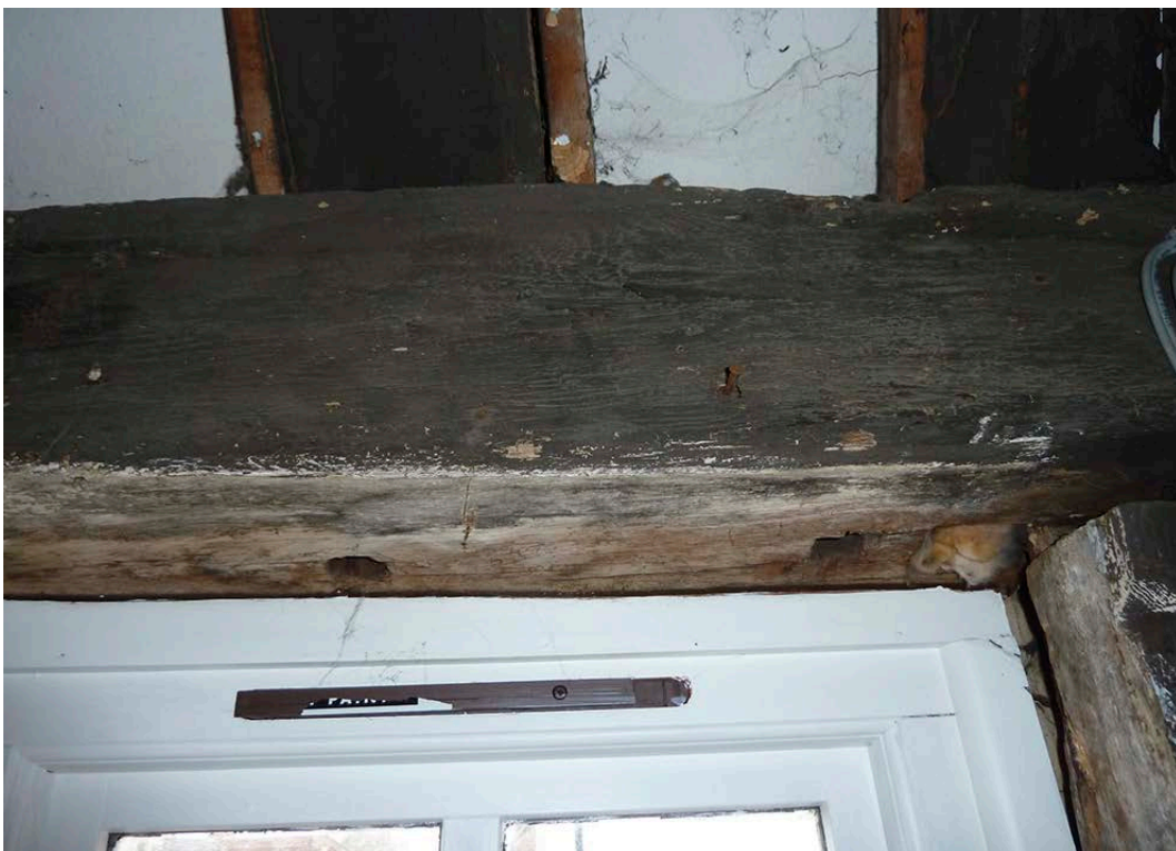
Figure 23: The underside of the wallplate in the west wall with the stave holes and the top chamfer of the adjacent stud (right). [Johanna Roethe © Historic England]
