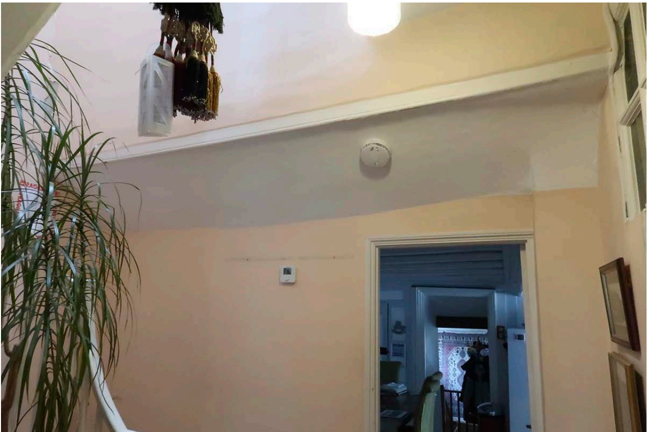
Figure 42: The truncated north end of the floor structure of the middle bay, seen from the stairwell in the front bay at first-floor level. [Johanna Roethe © Historic England]
