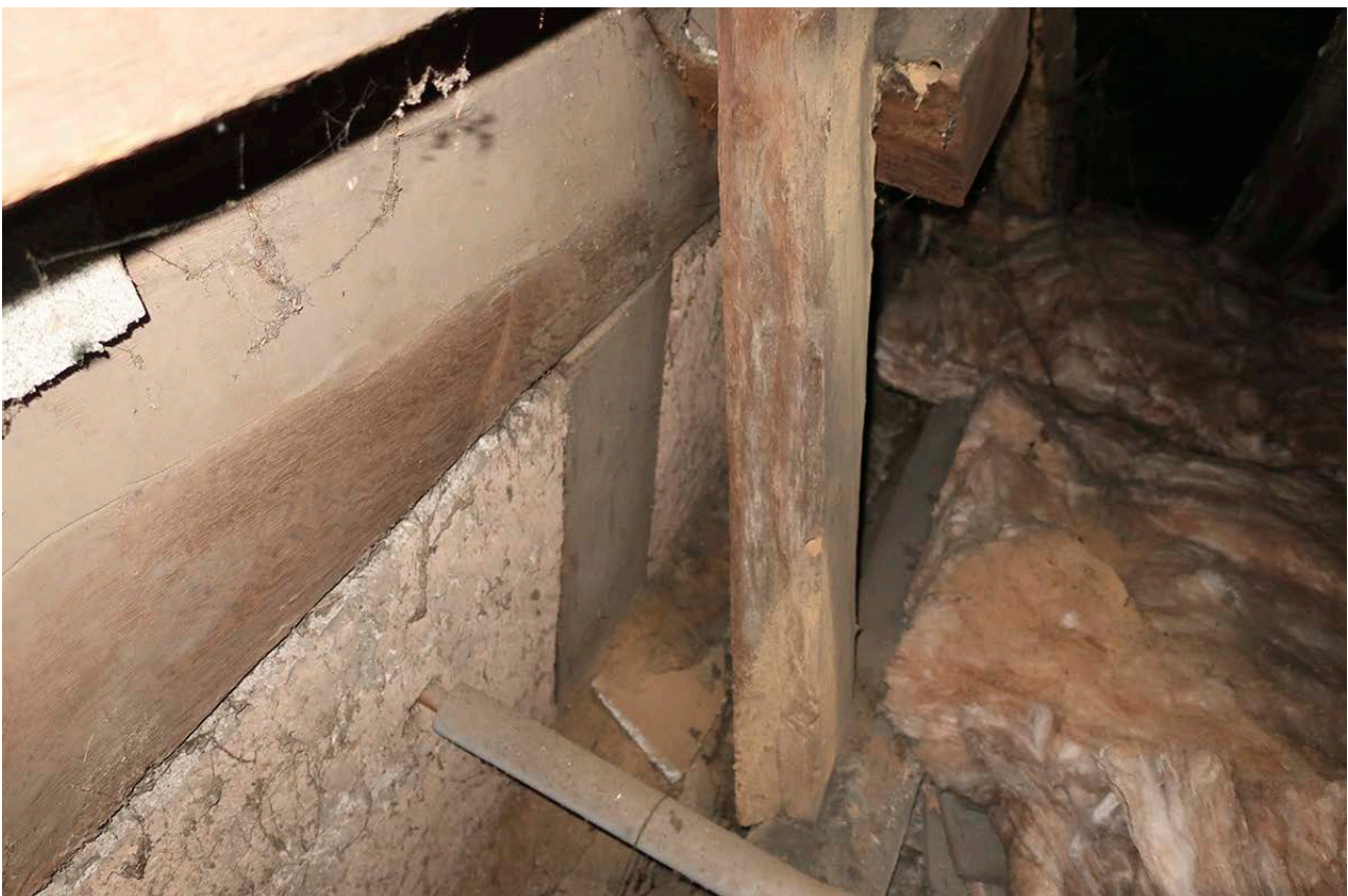
Figure 37: The west strut of the south truss of the middle bay. [Rebecca Lane © Historic England]
