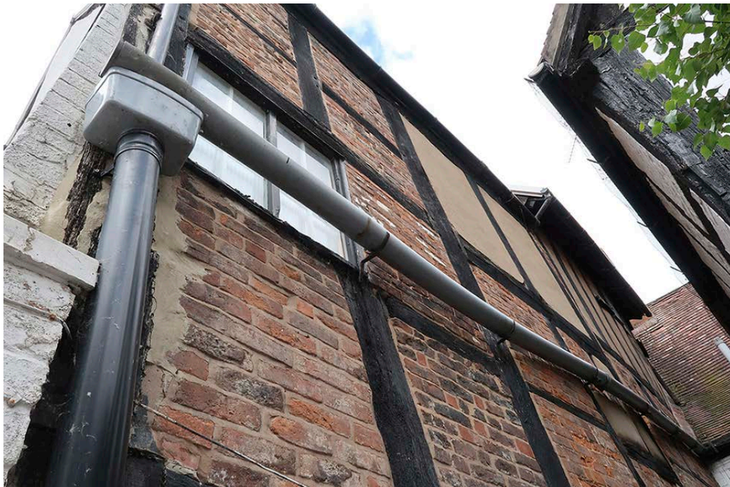
Figure 15: The east elevation of the south bay from Lilley's Alley. [Johanna Roethe © Historic England]
