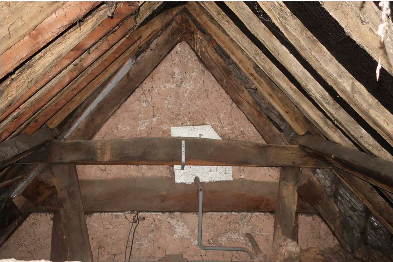
Figure 30: The closed north truss of the south bay seen from the north, with the open south truss of the middle bay in front of it. [Rebecca Lane © Historic England]
