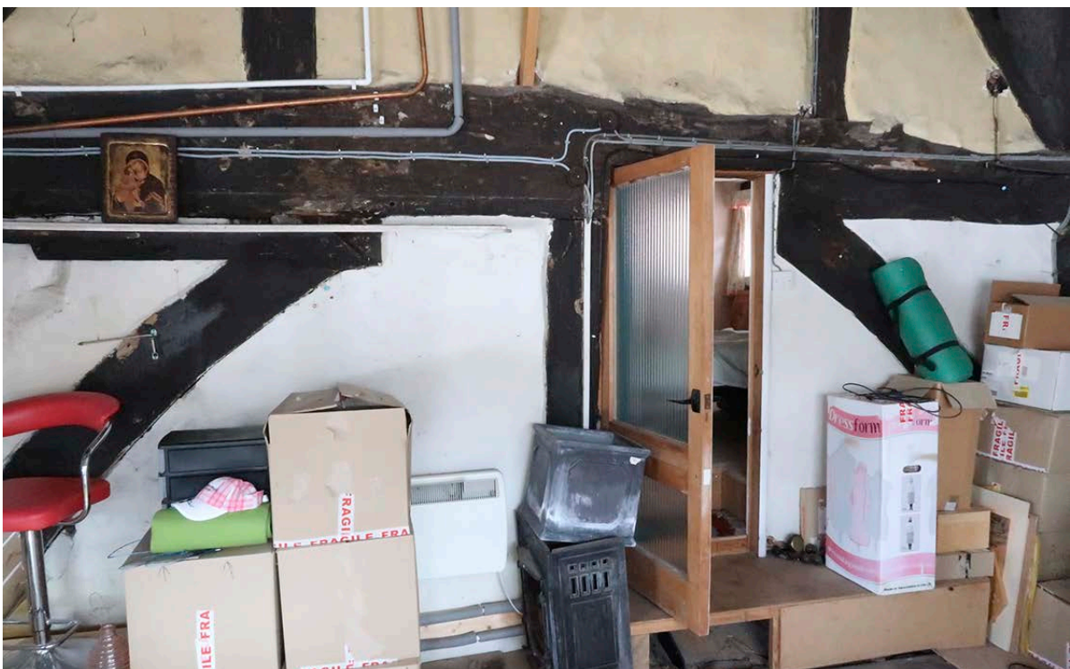
Figure 25: The lower part of the north frame of the south bay, seen from the south. [Johanna Roethe © Historic England]
