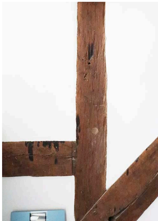
Figure 36: The taper burn marks on the north truss of the middle bay. [Johanna Roethe © Historic England]
