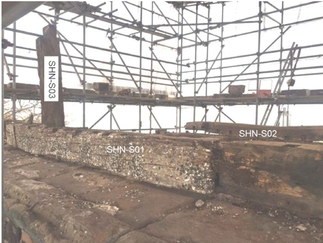
Figure 2: Floor/roof beams, north beam with in-situ joist (standing upright) in foreground; samples SHN-S01–SHN-S03 (samples SHN-S04 and SHN-S05 cut off tenons not shown), photograph taken from the north-west (Photograph: Alison Arnold)
