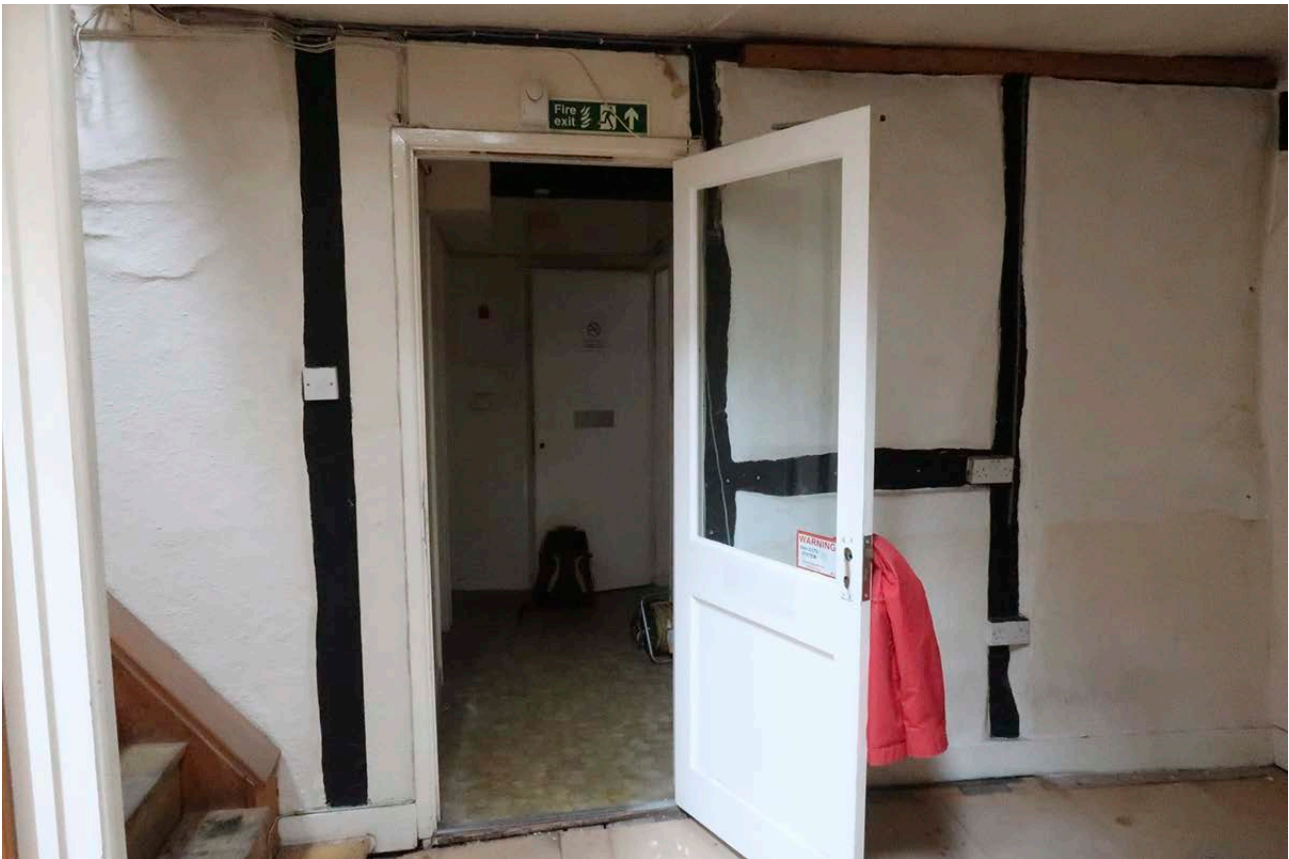
Figure 84: East side of the timber-framed partition in Bay A. [Johanna Roethe © Historic England]
