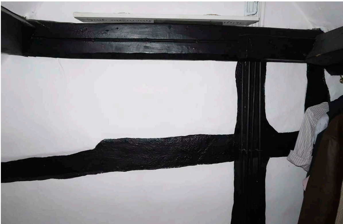
Figure 80: The west truss in the attic of the front range. [Johanna Roethe © Historic England]
