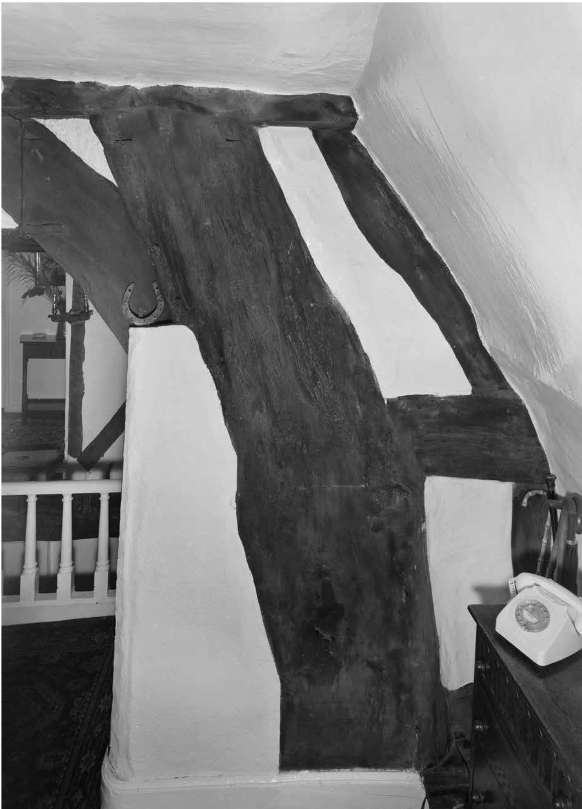
Figure Appendix 3.10: The north side of the west blade of the main range's frame 1, seen from the first floor of the front range. [© Crown Copyright. Historic England Archive, bb72/00616]
