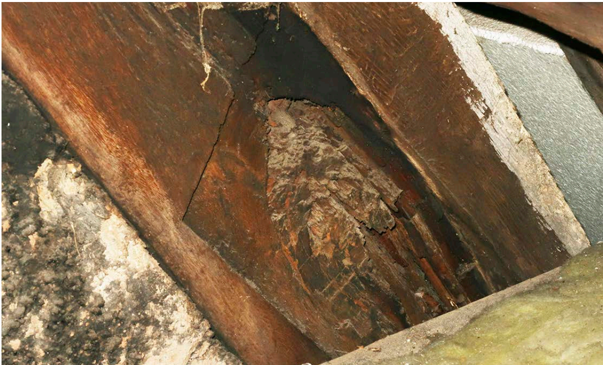
Figure 41: The missing patch infill in the east blade of frame 1 near the apex. [Johanna Roethe © Historic England]
