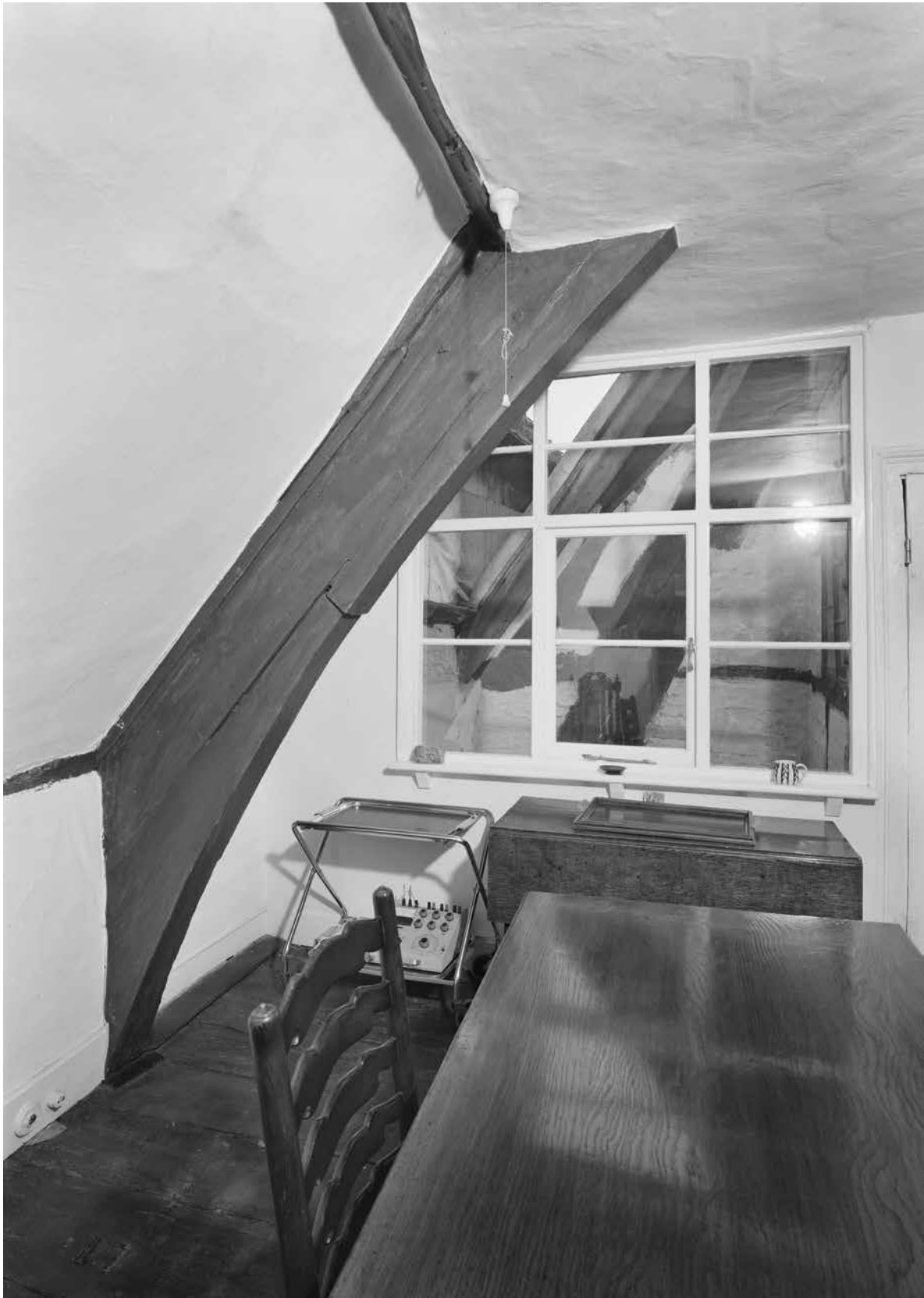
Figure Appendix 3.14: The north side of the east blade of the main range's frame 2, at first-floor level. Behind (south of) the frame is the 18th-century lightwell and frame 3. [© Crown Copyright. Historic England Archive, bb72/00620]
