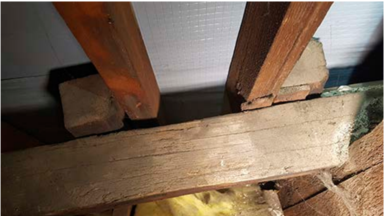
Figure 69: Two truncated common rafters on the west side of bay A, just south of frame 1 (right), with the upper purlin in the foreground and modern rafters behind. [Abigail Lloyd © Historic England]
