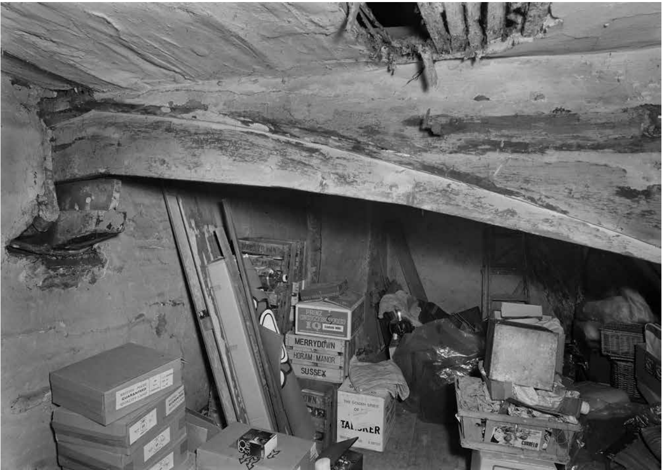
Figure Appendix 3.16: The west end of the collar of frame 2 (south side), at what was then attic level and is now the second floor. The surviving arch brace is embedded in the later wall to the left. [© Crown Copyright. Historic England Archive, bb72/00629]
