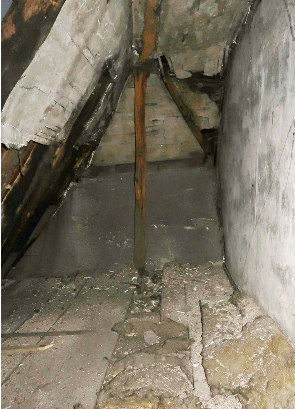
Figure 68: The inside of the additional roof space above the east end of the front range, looking north. The flat plaster wall to the right is the side of the adjoining building, 78-80 Barton Street. [Johanna Roethe © Historic England]
