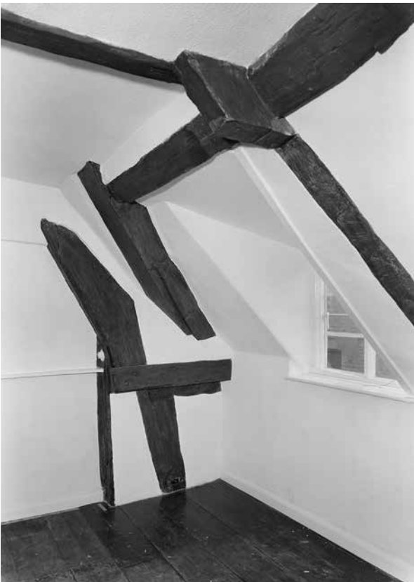
Figure 56: The west side of bays C and D at first-floor level in 1971 with frame 5 at centre left, with a windbrace rising from it, and the truncated inner rafter of frame 4 at centre top. [© Crown Copyright. Historic England Archive, BB72/00624]
