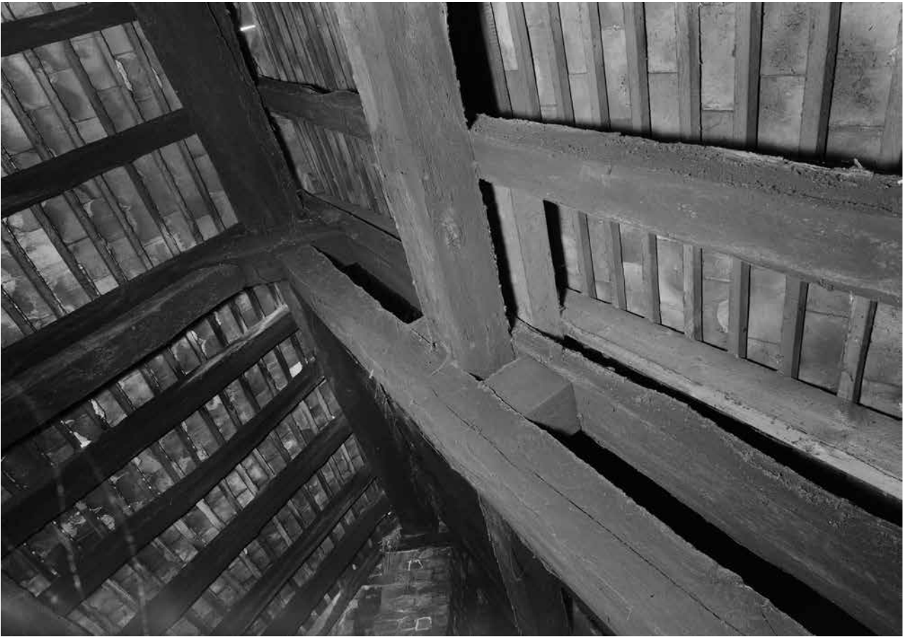
Figure Appendix 3.19: The north side of the main range's frame 2 in the roof space, looking south. In the background is the chimneystack set against frame 3. [© Crown Copyright. Historic England Archive, bb72/00632]
