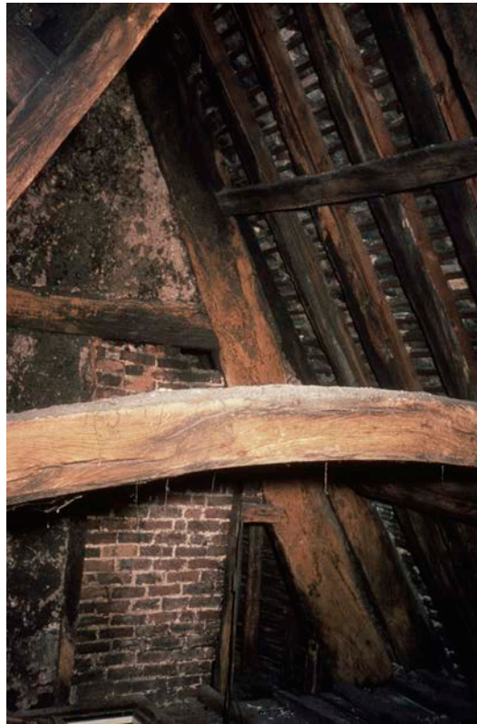
Figure 14: 1960s photograph by Stanley R. Jones showing the smoke-blackened south face of the partition between the hall and solar (frame 3) with the collar of the open frame over the solar (frame 4) in the foreground. The brick is part of a later chimneystack. [© Historic England Archive, SJC01/03/0006]
