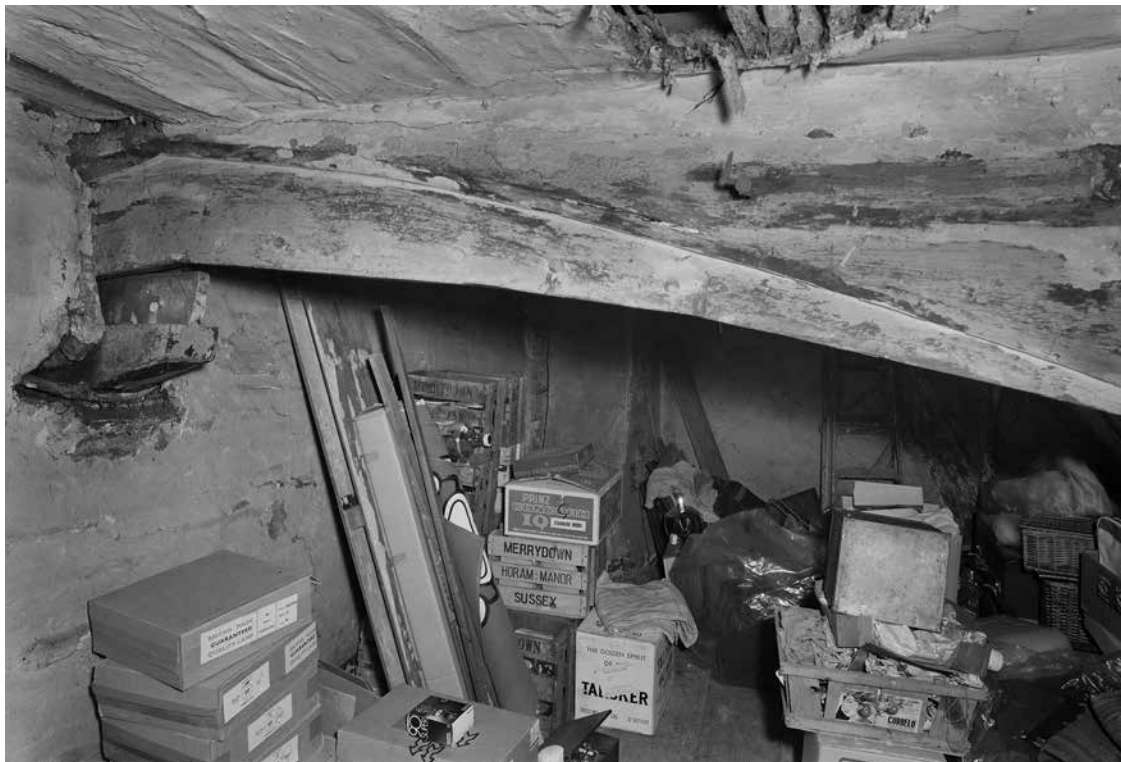
Figure 22: The collar of frame 2 with the partially-surviving arch brace to the east (left), photographed by Dennis Evans in December 1971. [© Crown Copyright. Historic England Archive, BB72/00629]
