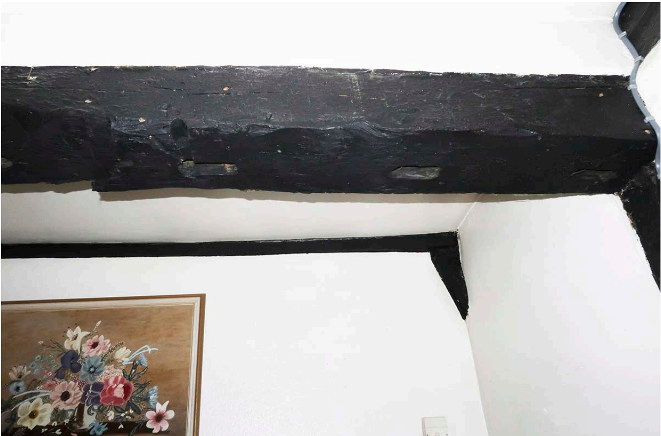
Figure 71: The former wall plate at the rear (south) of the east bay at first-floor level. The timber behind may be part of frame 1 of the main range. [Johanna Roethe © Historic England]
