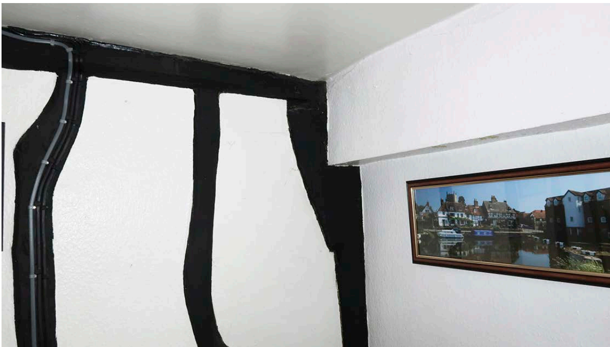
Figure 74: The north post and tiebeam of the central cross frame at first-floor level, now incorporated into a later partition. [Johanna Roethe © Historic England]
