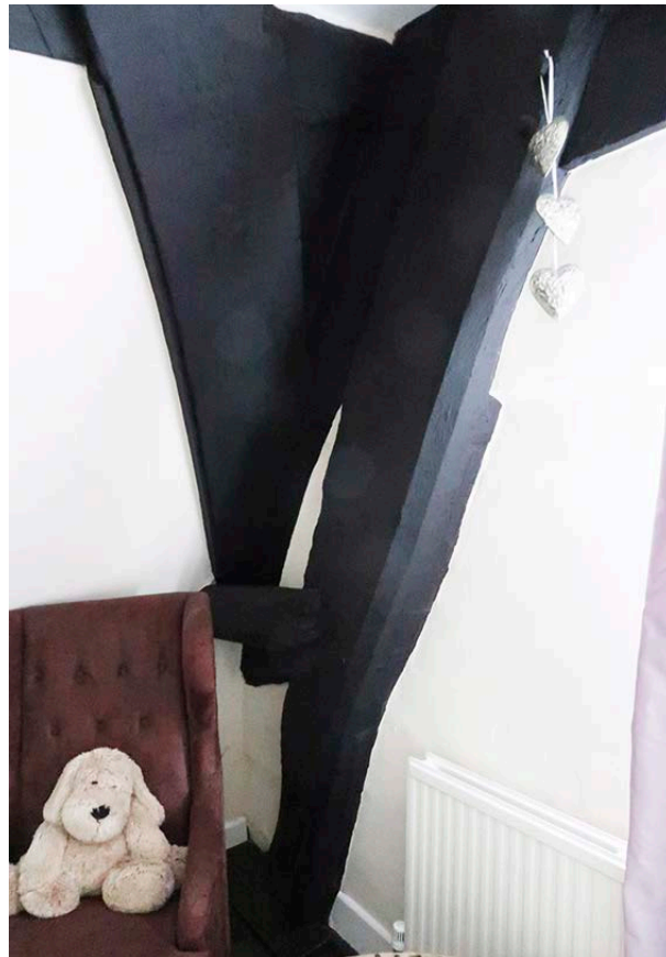
Figure 60: The east side of frame 5 at wall plate level, showing the springing of the windbrace and the chamfered cruck blade. A small piece of timber was later fixed to both windbrace and cruck blade, half-obscuring the cruck spur. [Johanna Roethe © Historic England]
