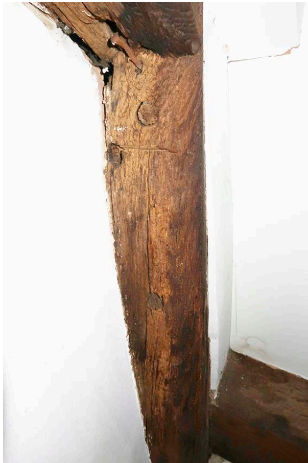
Figure 67: Three peg holes in the west cruck blade, two immediately below the collar and a further hole approximately 30cm below this. [Johanna Roethe © Historic England]
