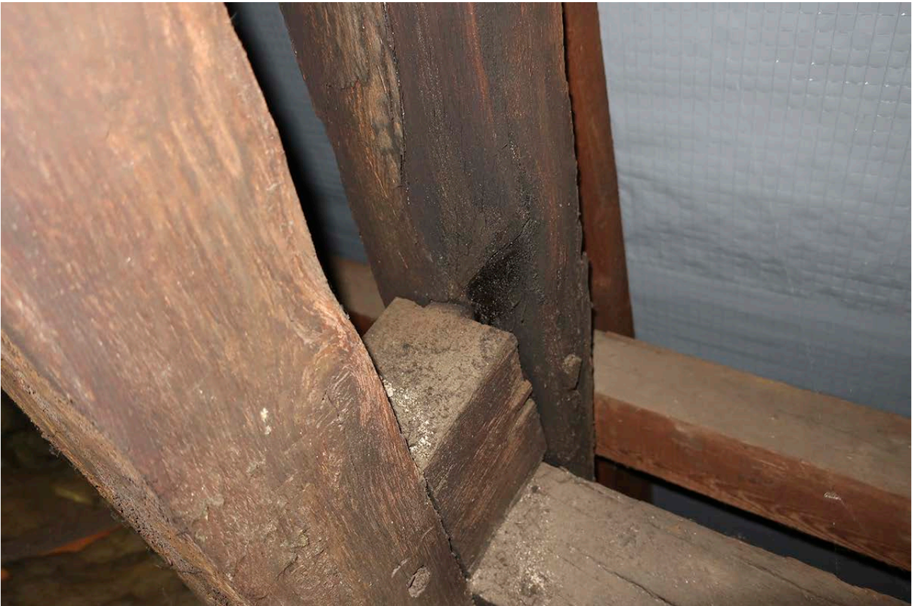
Figure 45: Detail of frame 2, showing the pegged spacer above the upper purlin. [Rebecca Lane © Historic England]
