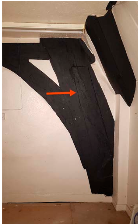
Figure 39: The south side of the east blade of frame 1 at collar level (now first-floor level), with the shallow cut-out indicated by a red arrow. [Abigail Lloyd © Historic England]
