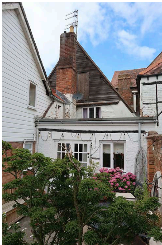
Figure 92: The flat-roofed, single-storey range to the south-east of the main range (centre) and to the left the 1970s rebuilding of the third 19th-century range. [Johanna Roethe © Historic England]
