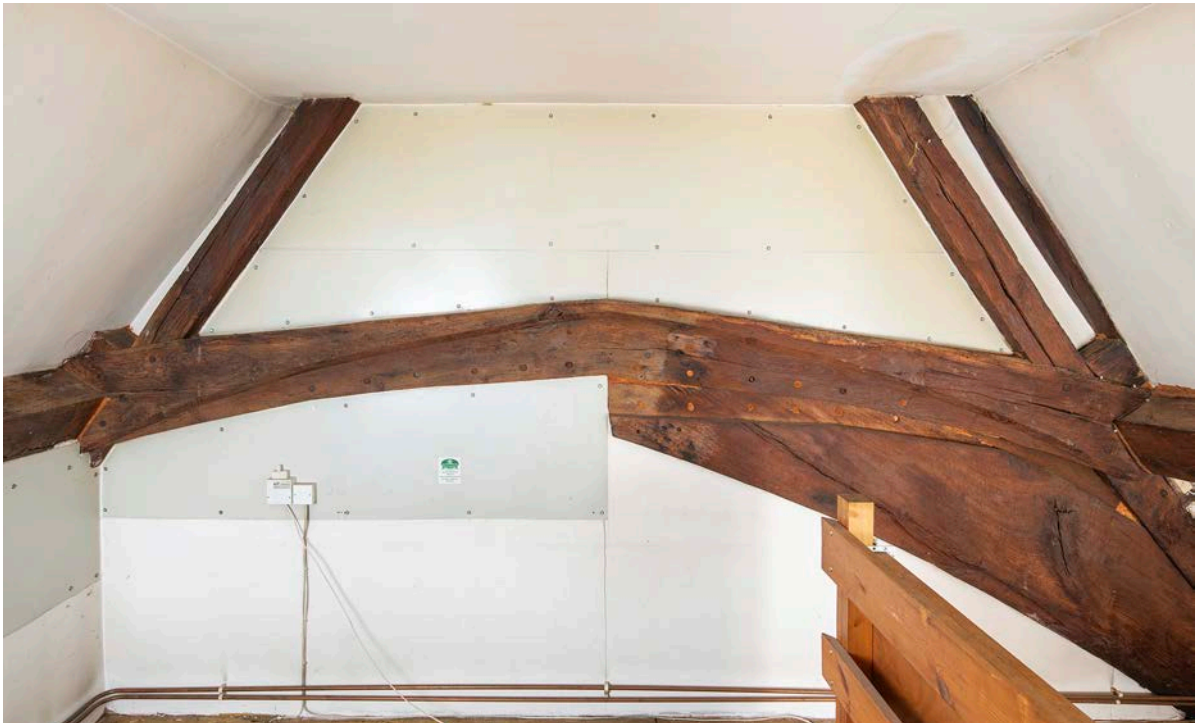
Figure 46: The south side of frame 2 at collar level (now second-floor level). [Steven Baker © Historic England Archive, DP325782]
