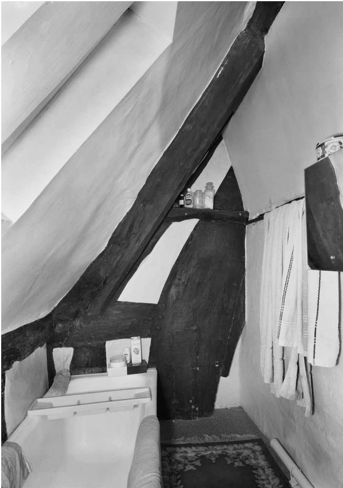
Figure Appendix 3.13: The south side of the west blade of the main range's frame 1, at first-floor level. [© Crown Copyright. Historic England Archive, bb72/00622]
