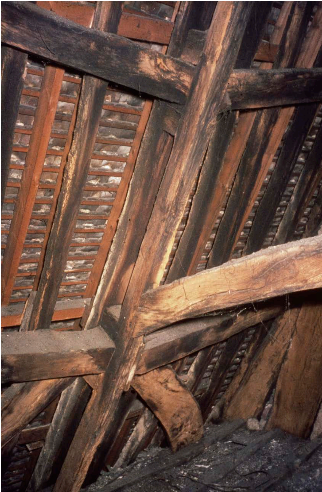
Figure Appendix 1.10: The collar of frame 4 (centre right) and the western central purlin and windbraces in bays C and D. [© Historic England Archive, SJC01/03/0008]
