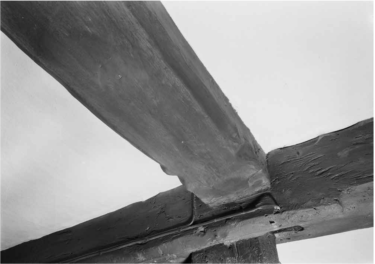
Figure Appendix 3.8: Detail of the chamfer stops of the axial beam in the west bay of the front range at first-floor level. [© Crown Copyright. Historic England Archive, bb72/00619]
