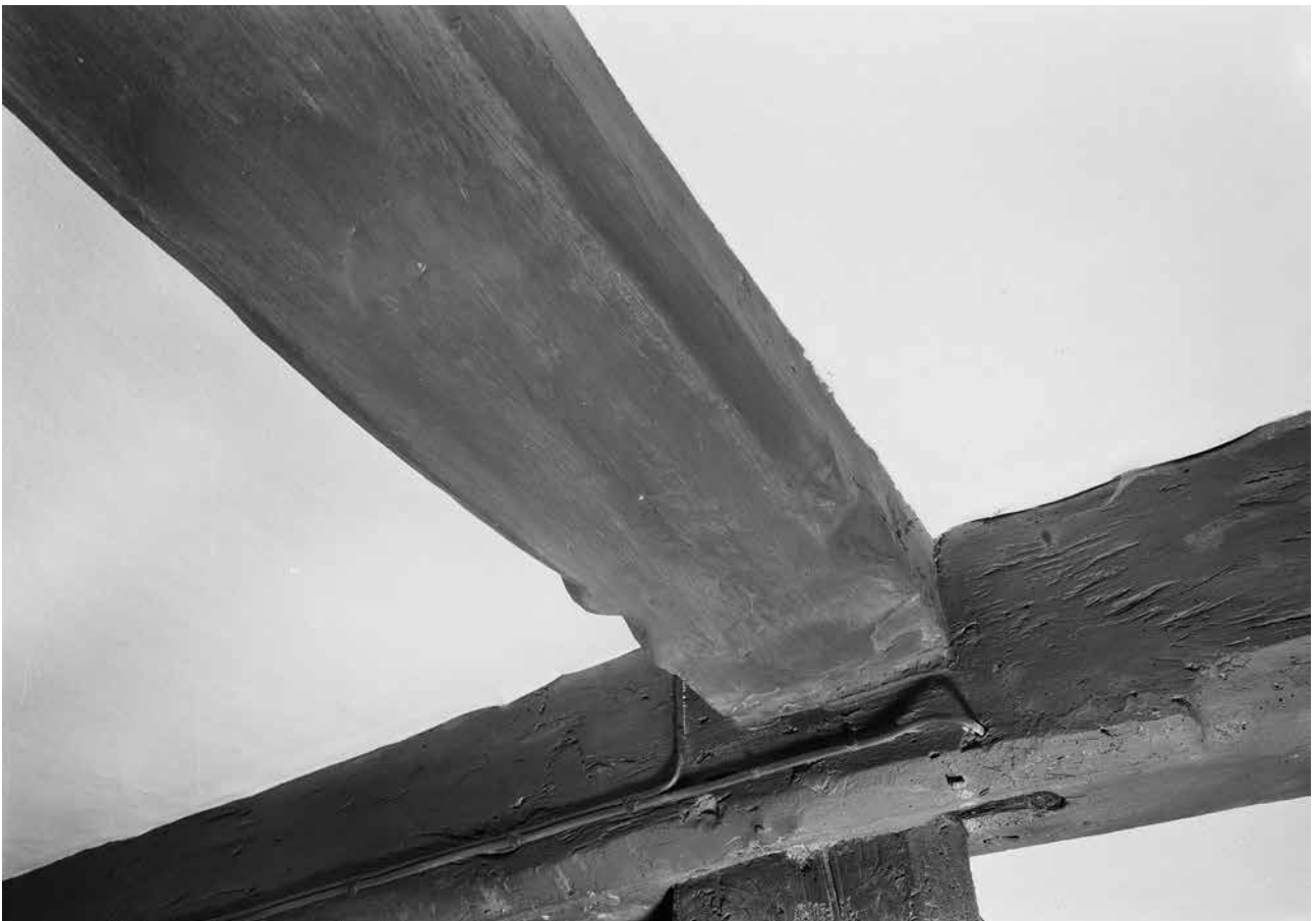
Figure 83: The ceiling beam in the west bay with a jewel stop and the large mortice for the original central stud, with later infill (bottom) in 1971. [© Crown Copyright. Historic England Archive, bb72/00619]
