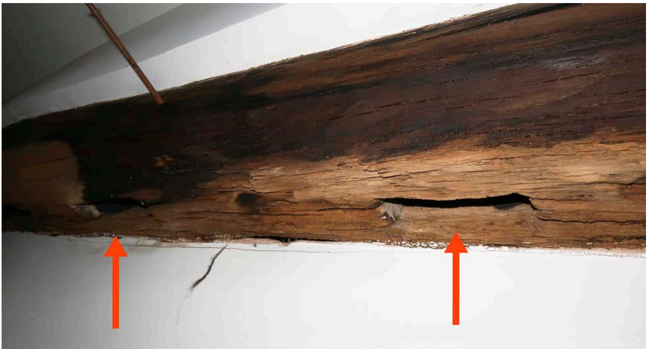
Figure 66: Two empty mortices (indicated by red arrows) for staves in the upper collar of frame 5. [Johanna Roethe © Historic England]
