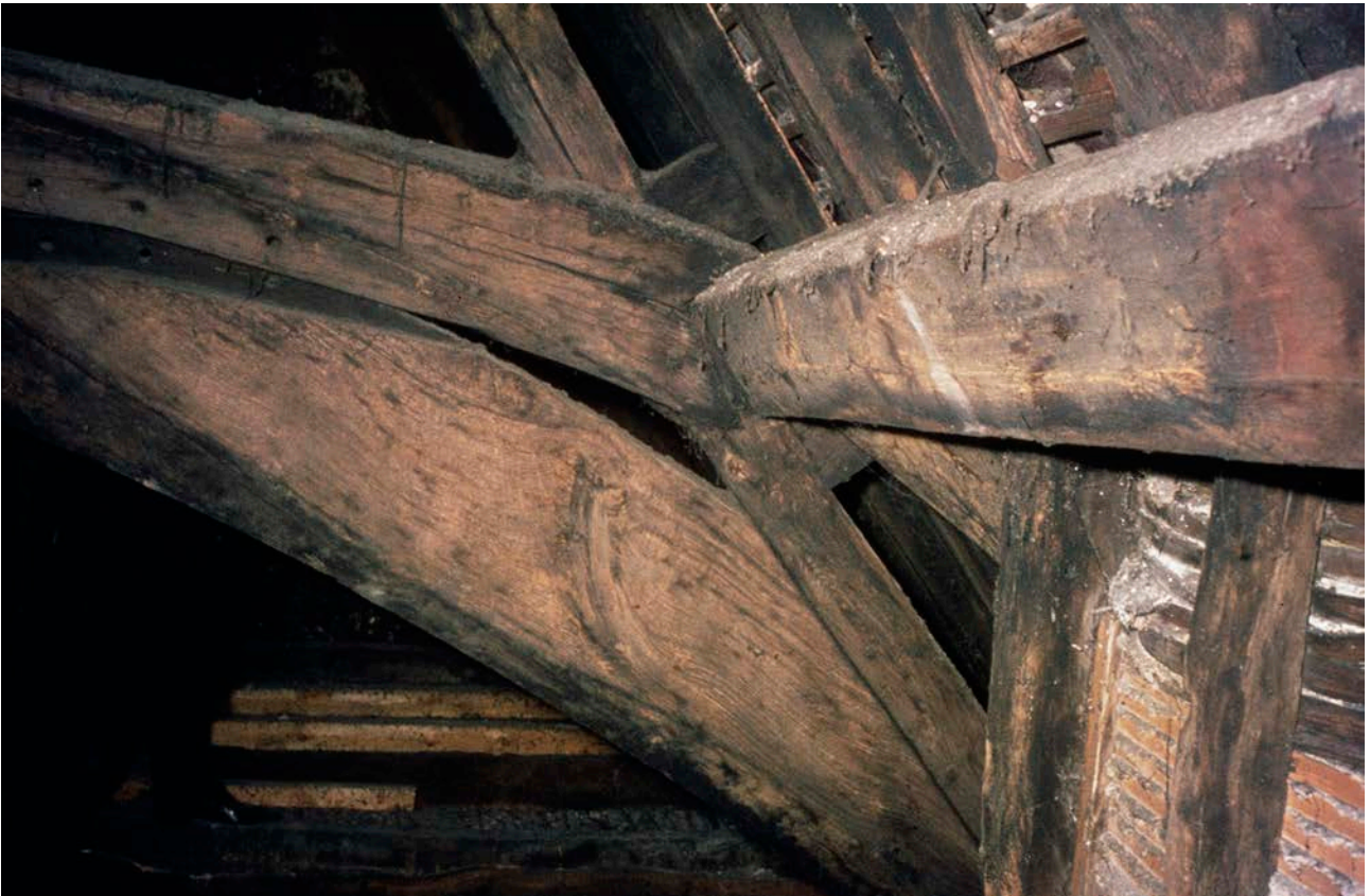
Figure Appendix 1.7: Detail of the birdsmouth joint of the collar and eastern central purlin of frame 2. [© Historic England Archive, SJC01/03/0005]
