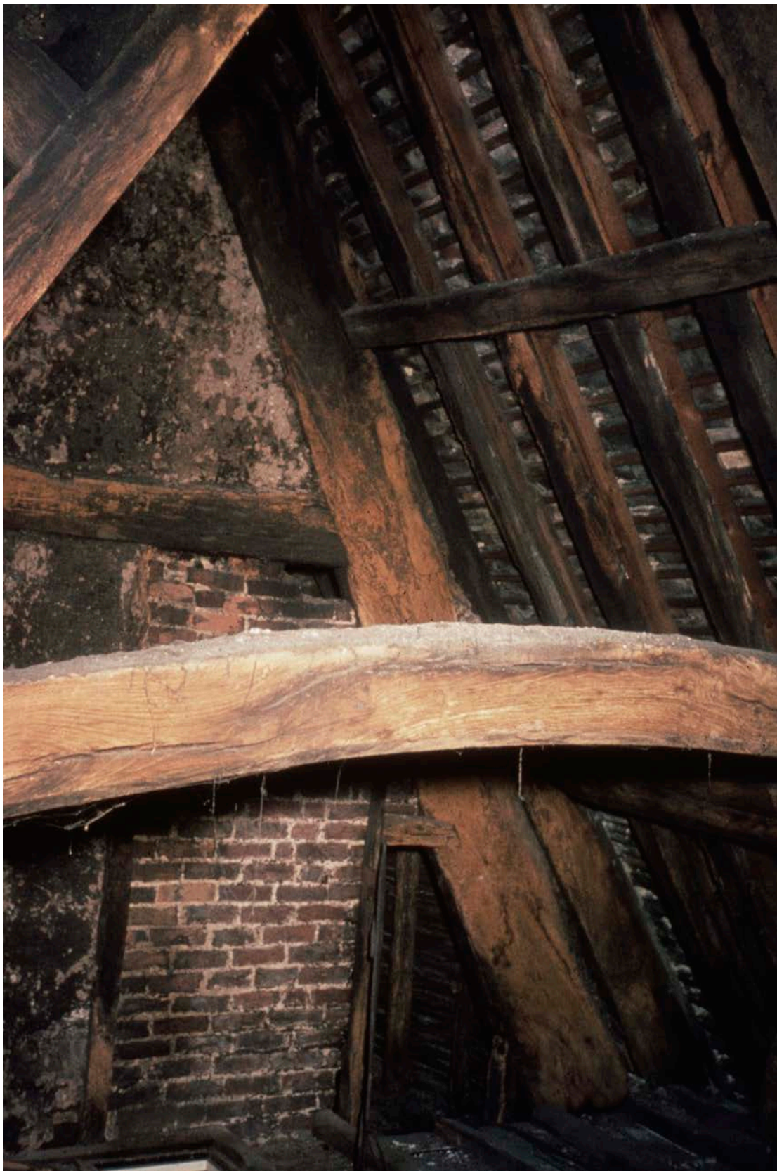
Figure Appendix 1.8: The collar of frame 4 in the foreground and the south side of frame 3 in the background. [© Historic England Archive, SJC01/03/0008]
