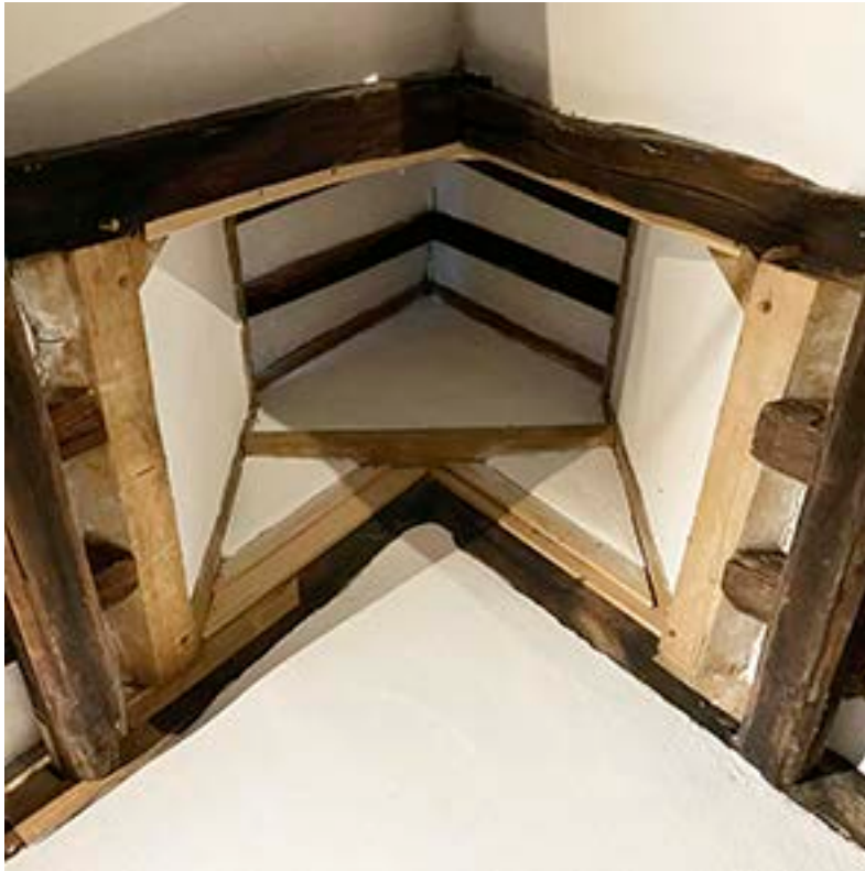
Figure 70: The reconstructed smoke louvre in a rear wing of the Royal Hop Pole Hotel in Tewkesbury. [Rebecca Lane © Historic England]
