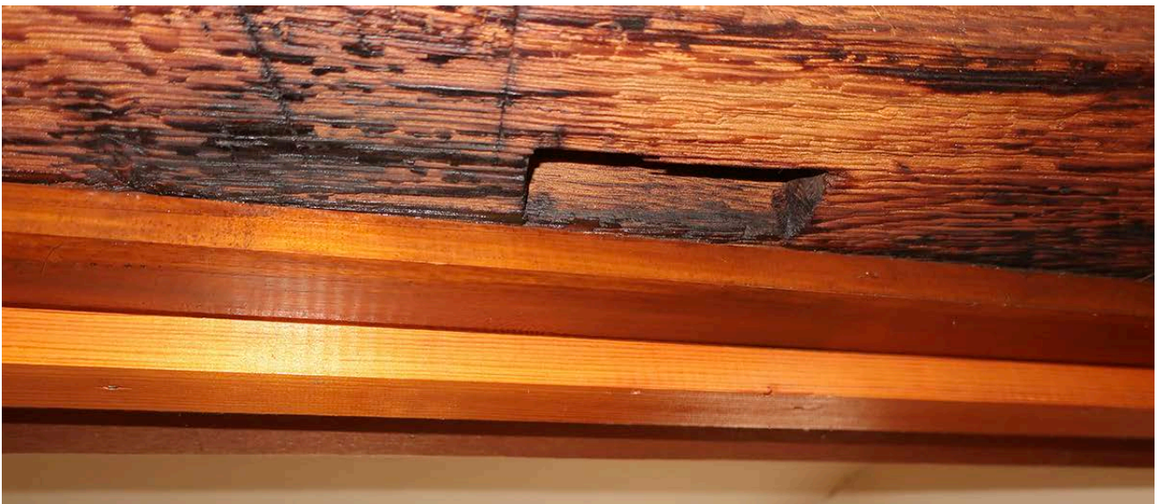
Figure 52: The empty mortise in the upper collar of frame 3 for a stud next to possible scribed marks. [Rebecca Lane © Historic England]
