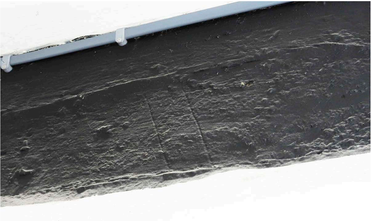
Figure 78: A scribed carpenter's mark (II for two) on the central tiebeam at the present first-floor level. [Johanna Roethe © Historic England]
