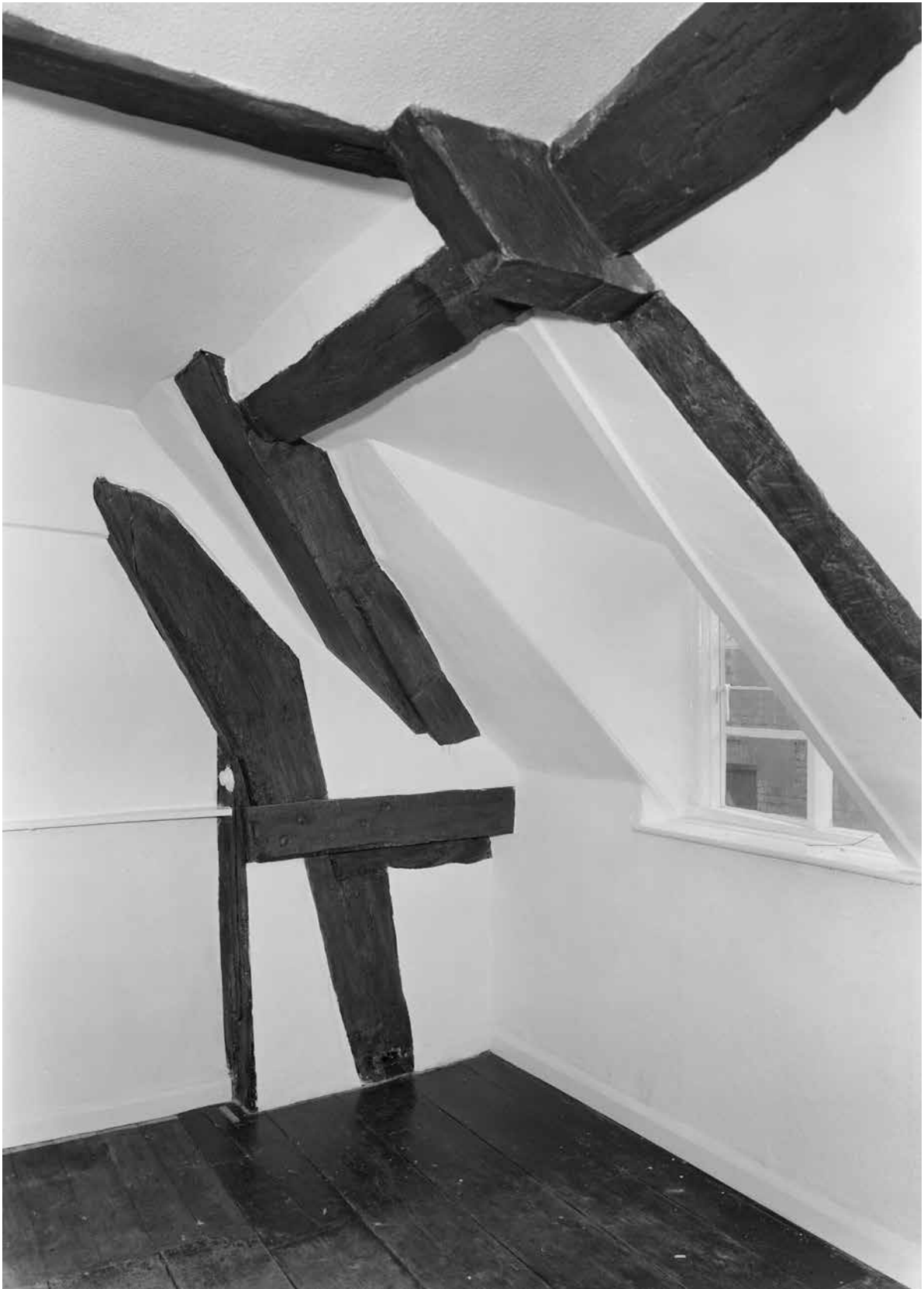
Figure Appendix 3.21: The west side of frames 4 (right) and 5 (left) at first-floor level and looking south. [© Crown Copyright. Historic England Archive, bb72/00624]
