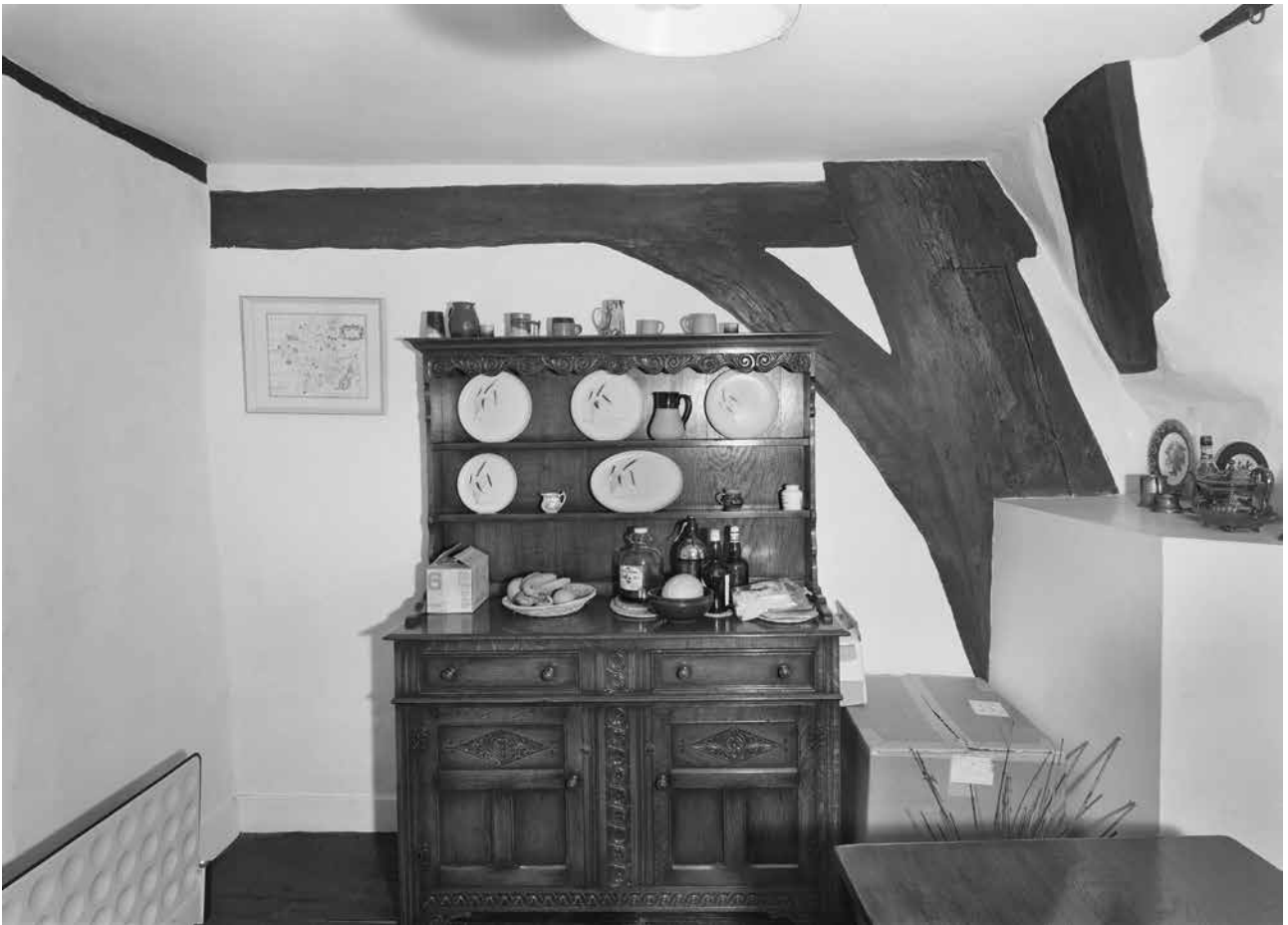
Figure Appendix 3.12: The south side of the east blade of the main range's frame 1, at first-floor level. [© Crown Copyright. Historic England Archive, bb72/00621]
