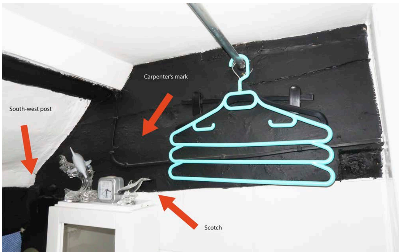
Figure 77: The south-west post and west tiebeam, annotated with the location of a carpenter's mark (III) and a scotch. [Johanna Roethe © Historic England]
