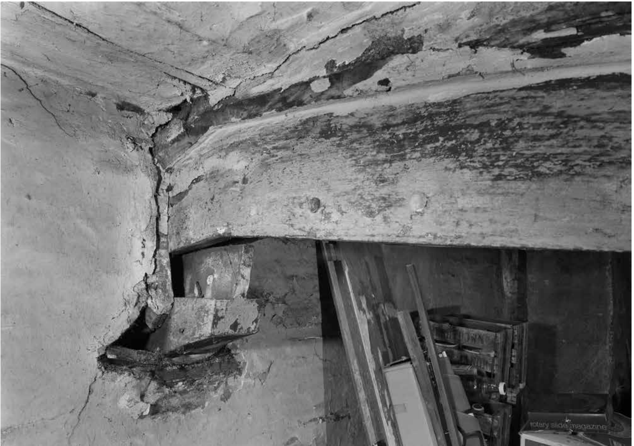
Figure Appendix 3.17: Close-up of the collar and surviving arch brace of frame 2. [© Crown Copyright. Historic England Archive, bb72/00630]
