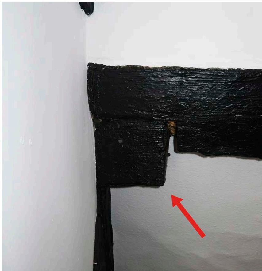
Figure 34: The north side of the west end of frame 1, seen from the second-floor flat in the later front range and looking west. The arrow indicates the projecting central purlin, with a later timber scarfed onto its northern end. [Johanna Roethe © Historic England]
