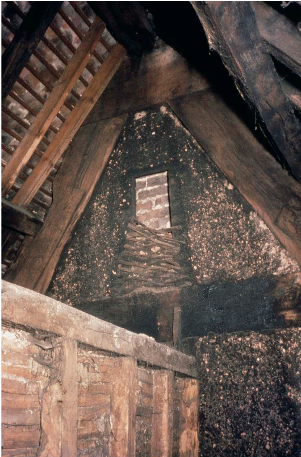
Figure 13: 1960s photograph by Stanley R. Jones showing the smoke-blackened south face of the northernmost frame (frame 1), with the lath-and-plaster attic in the foreground. [© Historic England Archive, SJC01/03/0008]
