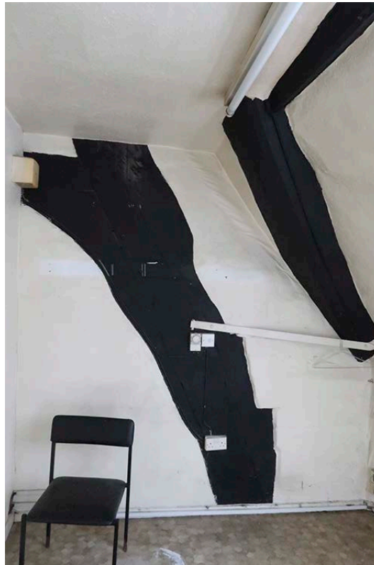
Figure 49: The north face of the west blade of frame 3, at the level of the lower collar (now first-floor level). [Johanna Roethe © Historic England]
