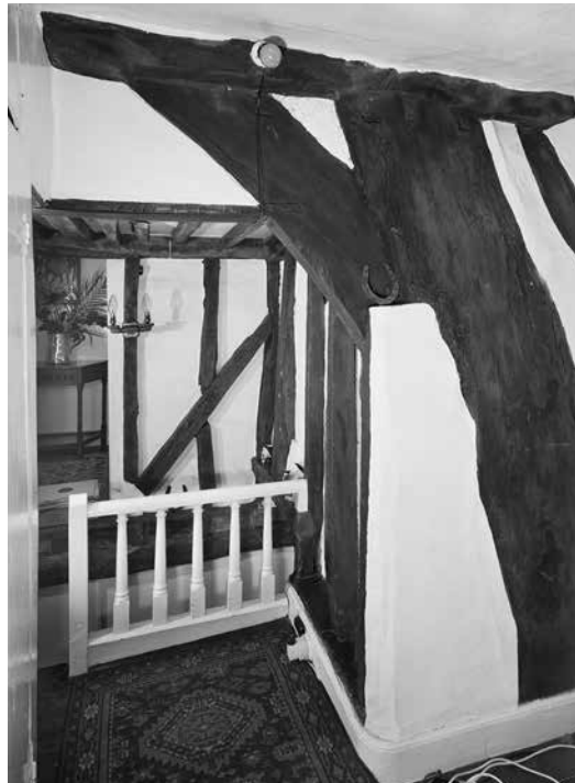
Figure 21: View from the front range at first-floor level with the north side of frame 1 of the main range in the foreground right. Photograph taken by Dennis Evans of December 1971. [© Crown Copyright. Historic England Archive, BB72/00615]
