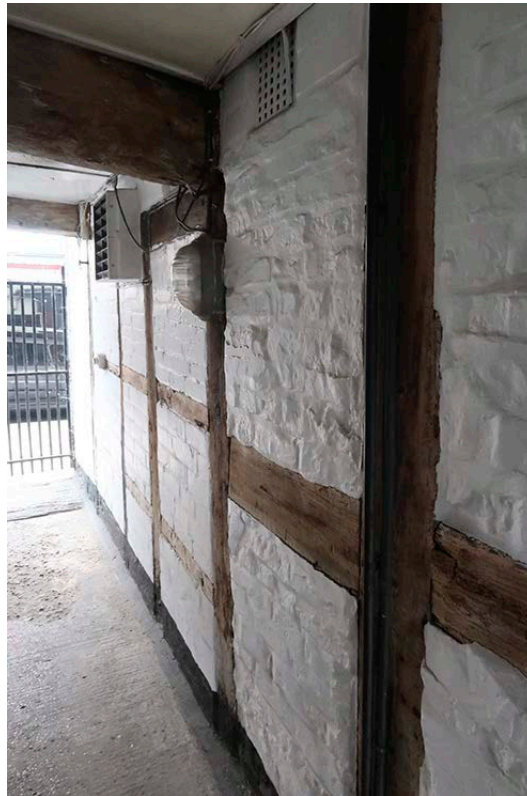
Figure 90: The west wall of the ground floor of the front range from Mason's Court, looking north-east. [Johanna Roethe © Historic England]
