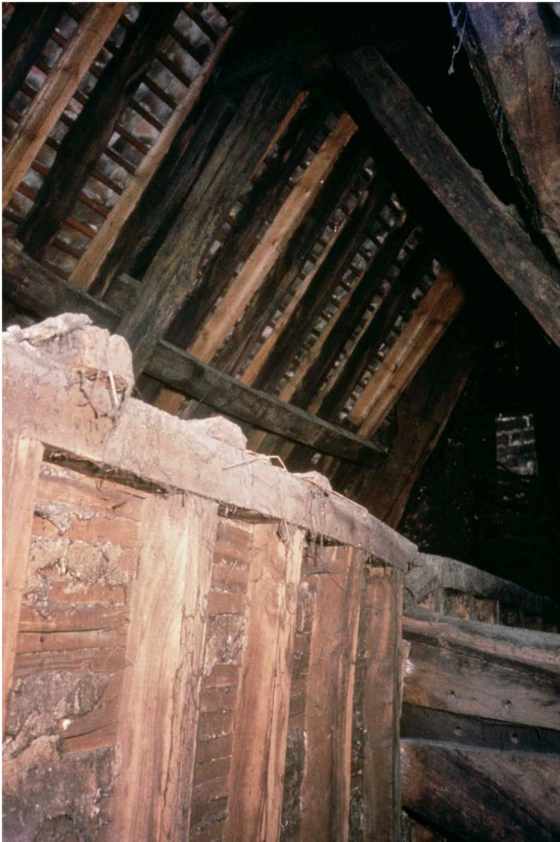
Figure Appendix 1.6: The south side of frame 2 in the middle distance, with frame 1 in the background. In the left foreground is the inserted partial attic. In the right foreground is the collar with arch brace of frame 2. [© Historic England Archive, SJC01/03/0007]
