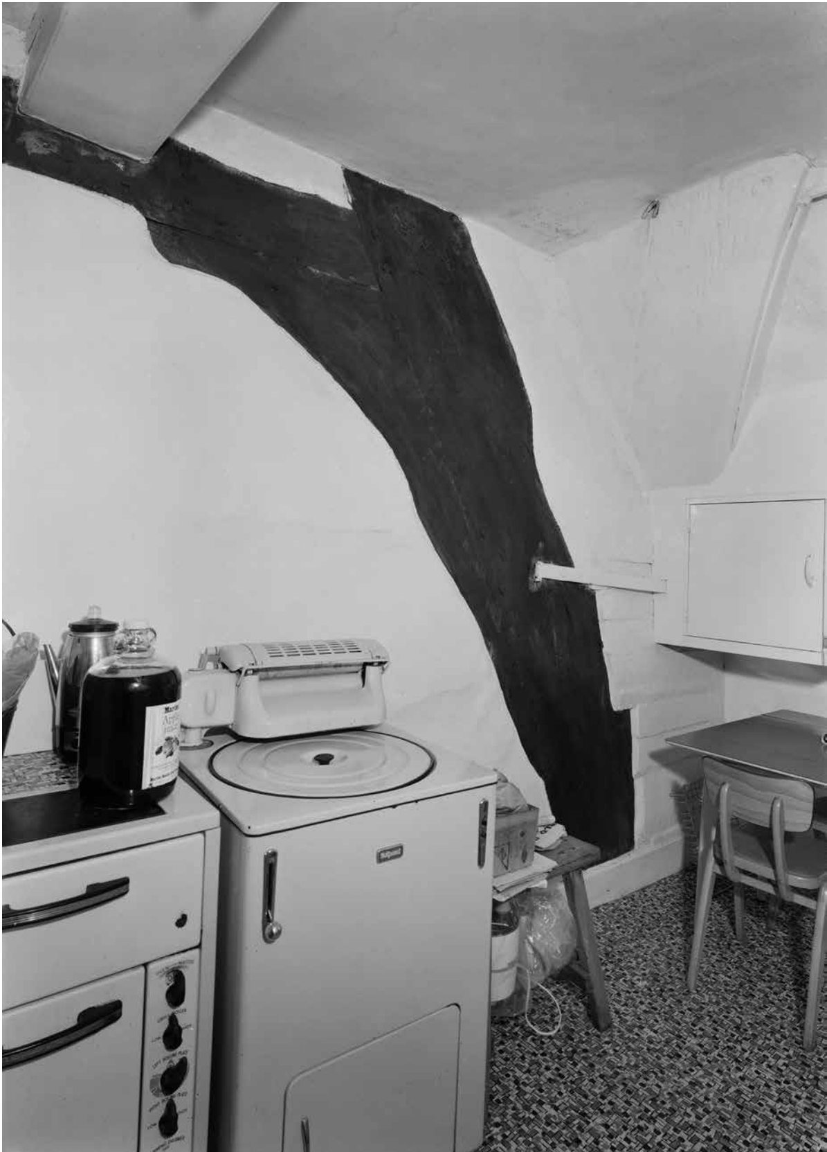
Figure Appendix 3.20: The north side of the west blade of the main range's frame 3, at first-floor level. [© Crown Copyright. Historic England Archive, bb72/00627]
