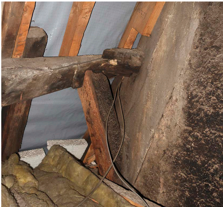
Figure 53: The splayed and tabled scarf joint in the upper purlin on the east side just north of frame 3 in bay B. [Rebecca Lane © Historic England]
