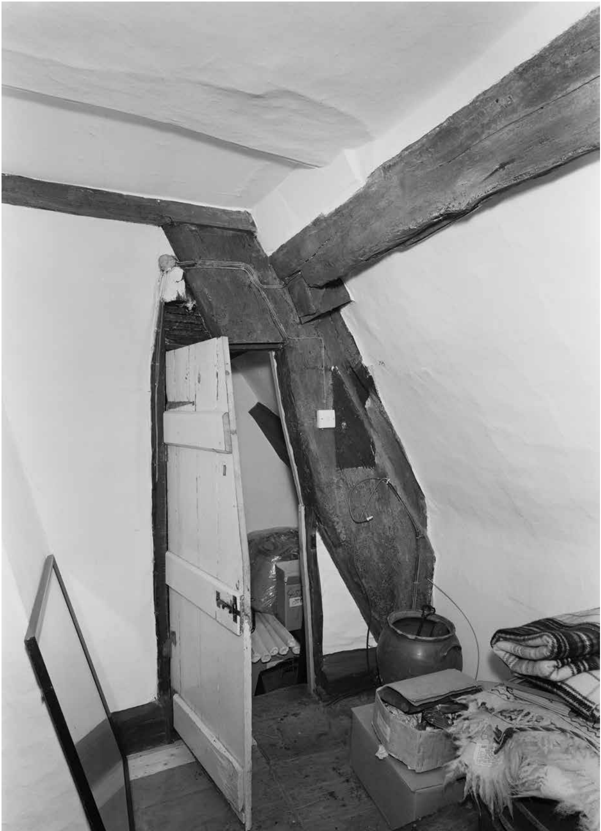
Figure Appendix 3.11: The north side of the west blade of the main range's frame 1, seen from the second floor of the front range. [© Crown Copyright. Historic England Archive, bb72/00628]
