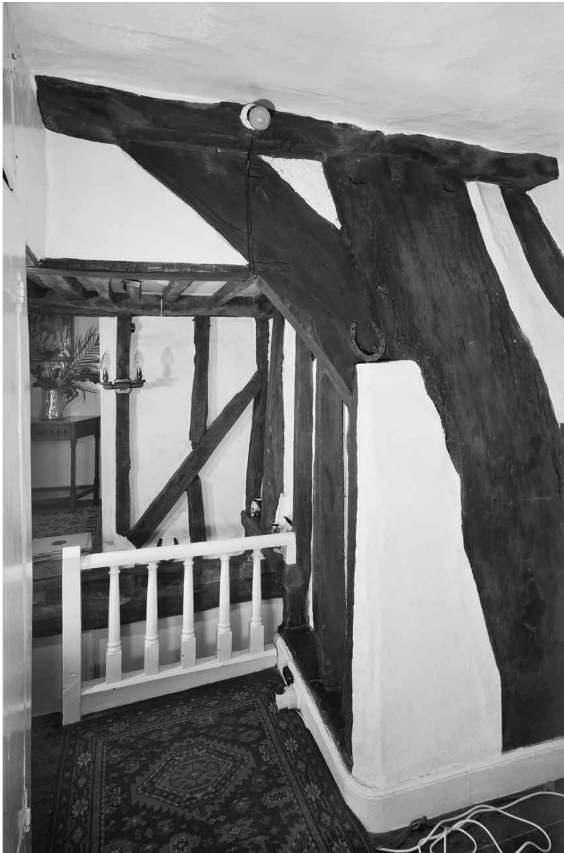
Figure Appendix 3.9: The north side of the west blade of the main range's frame 1, seen from the first floor of the front range. [© Crown Copyright. Historic England Archive, bb72/00615]
