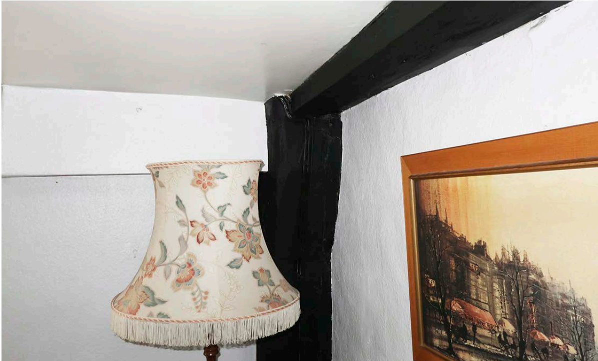
Figure 73: The jowled corner post at the north-east corner of the front range, at first-floor level. [Johanna Roethe © Historic England]
