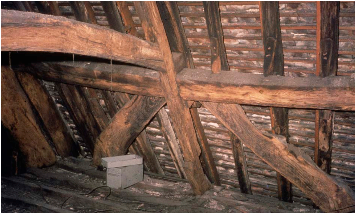
Figure 12: 1960s photograph by Stanley R. Jones, showing part of the two southern bays of the building, including the truss over the solar (bays C and D either side of the east end of frame 4). [© Historic England Archive, SJC01/03/0003]
