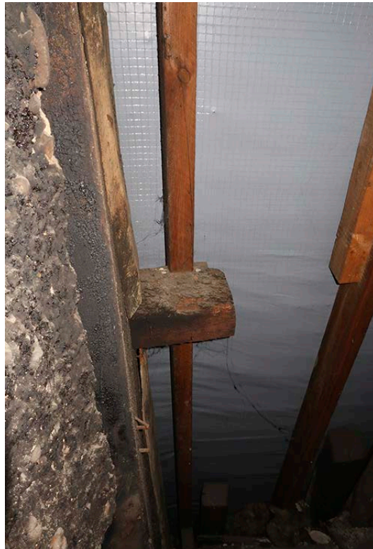
Figure 38: The west end of the north side of frame 1, with smoke blackening to the infill panel and the west cruck blade. [Johanna Roethe © Historic England]
