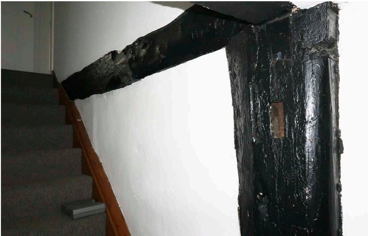
Figure 75: The south post and tiebeam of the central cross frame. [Johanna Roethe © Historic England]
