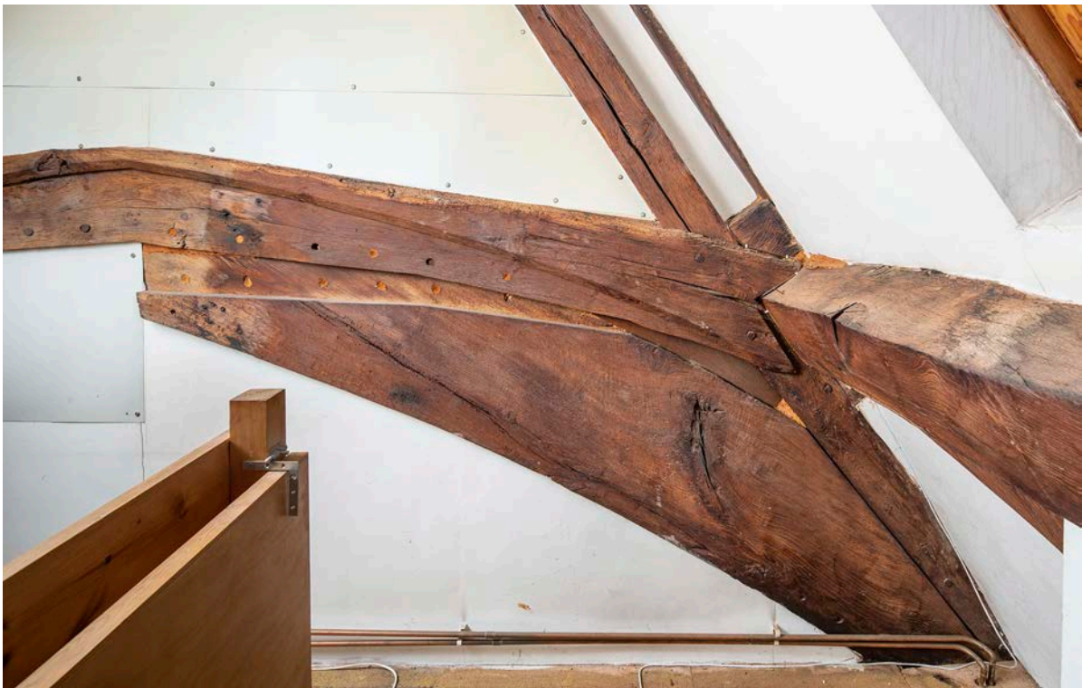
Figure 47: Detail of the birdsmouthed joint of the collar to the main purlin on the east side of bay B. [Steven Baker © Historic England Archive, DP325785]
