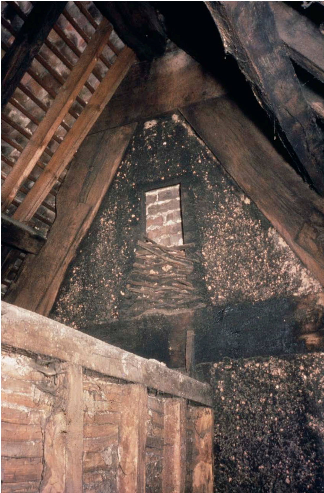
Figure Appendix 1.4: The south side of frame 1, with the smoke vent. To the left is the inserted partial attic. [© Historic England Archive, SJC01/03/0008]
