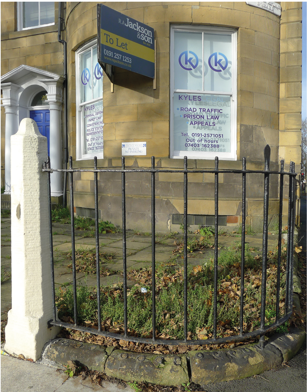
Figure 23: No. 19 has coping stones which show the original position of the iron uprights of the railings. The gateposts may also be original. [Lucy Jessop © Historic England]
