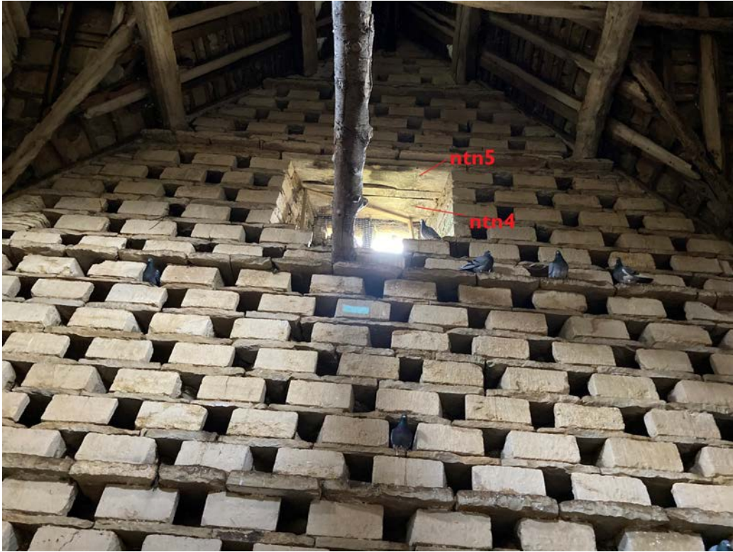
Figure 4: View of the internal west wall, showing the lintels sampled as ntn4 and ntn5 (photograph Penny and David Hanks)
