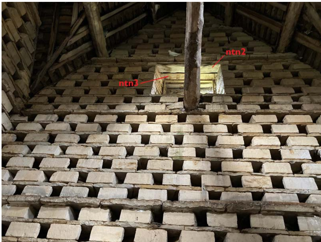
Figure 3: View of the east internal wall showing the lintels sampled as ntn2 and ntn3 (photograph Penny and David Hanks)
