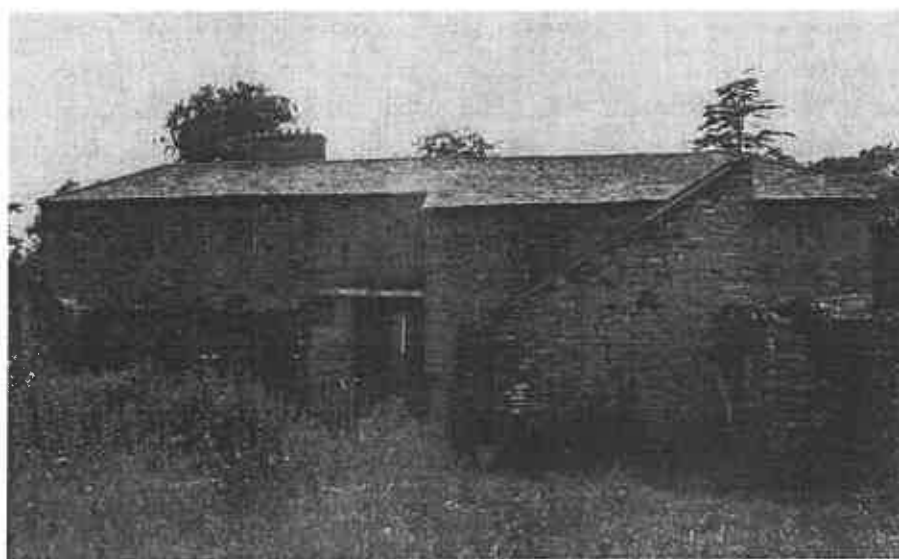
Fig.18 The east elevation of the east wing showing slit and square vents in the barn wall. (NMR: MF 000223/20)
