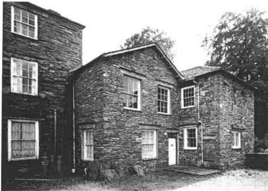
Fig.19 Extended west link block projecting beyond the rear of the main block. (NMR: BB007278)
